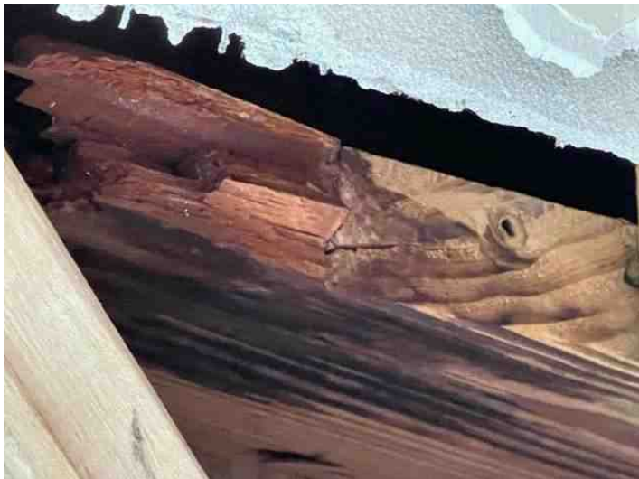
Wood Rot in Trusses
