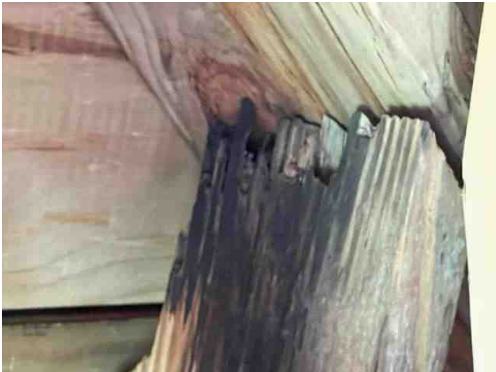
Wood Rot in Trusses
