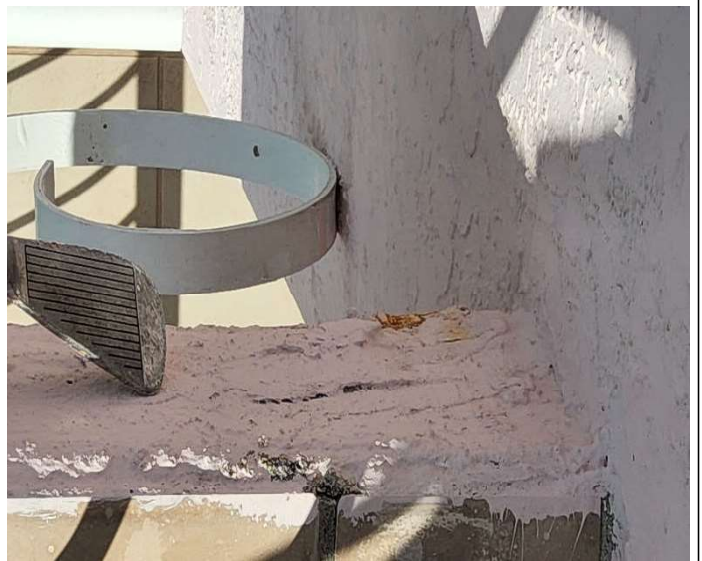
Photo # 28. Stucco delamination and rust spot at the balcony slab edge.
