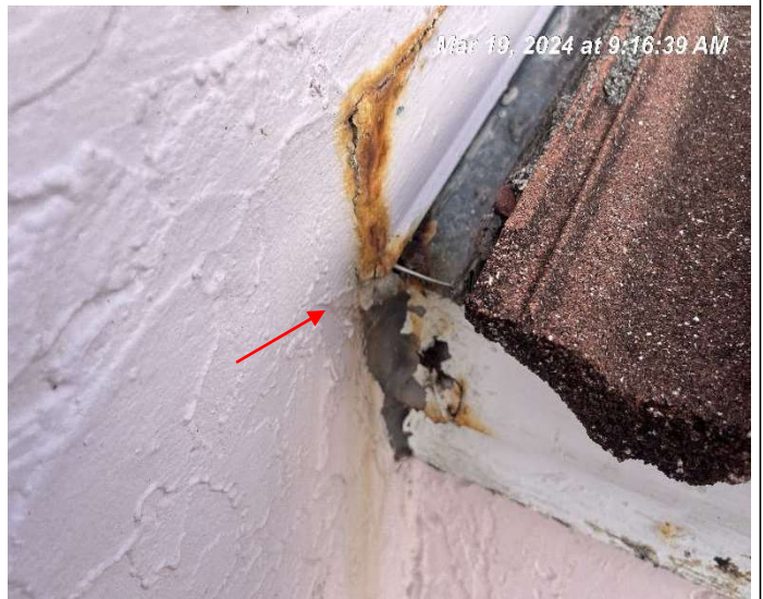
Photo # 20. Corrosion stains at the roof flashing.
