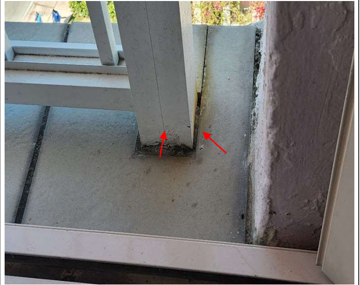
Photo # 34. Missing sealant/grout and pitting corrosion at the balcony railing post.
