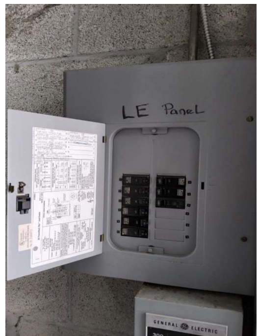
Photo # 12. Item 7.5. Meter Electrical Room. Panelboard LE. Missing proper circuit identification.
