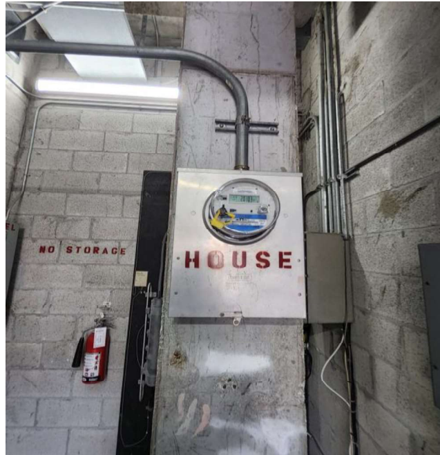
Photo # 4. Item 4.1.b. Meter Electrical Room. Meter House.
