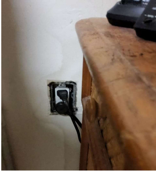
Photo # 17. Item 16.c. Maintenance office. Missing cover for receptacles.
