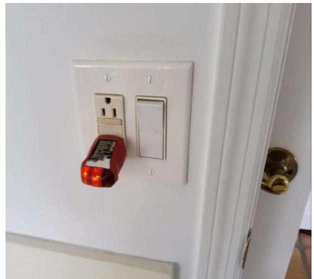
Photo # 32. Item 28.2. Missing GFCI protection for receptacles in the bathroom- test fail.
