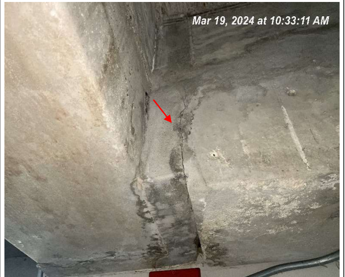
Photo # 40. Concrete crack at the beam of the basement garage.
