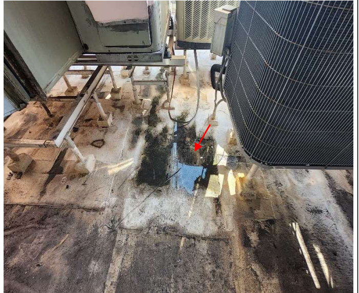
Photo # 18. Water ponding at the lower flat roof.
