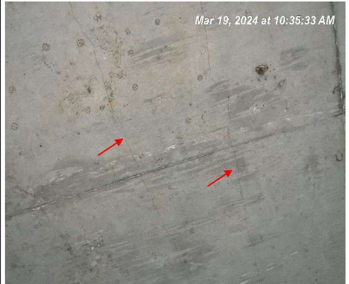
Photo # 42. Concrete cracks at the ceiling slab of the basement garage.
