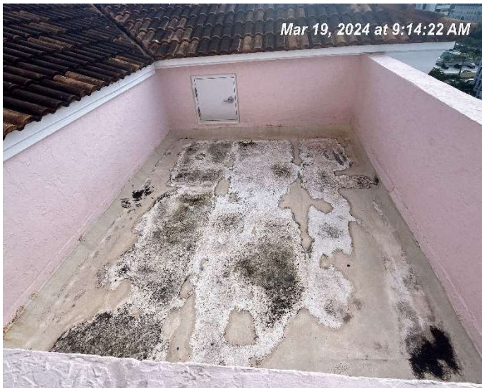
Photo # 19. Water ponding stains at the PH floor flat roof.
