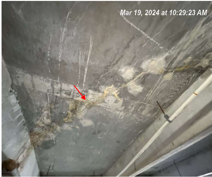
Photo # 37. Concrete crack with water stains and efflorescence at the ceiling slab of the basement garage.
