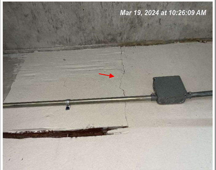
Photo # 36. Concrete crack at the wall of the basement garage.
