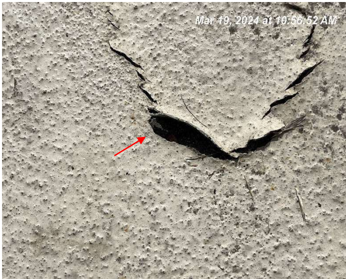
Photo # 47. Delaminated waterproofing coating at the parking deck.
