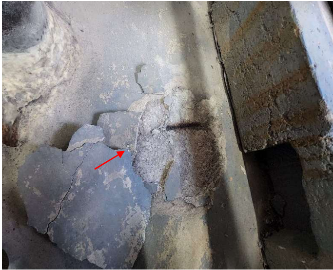
Photo # 45. Cracked and spalled concrete with exposed corroded rebar at the Generator & Fire Pump Room.
