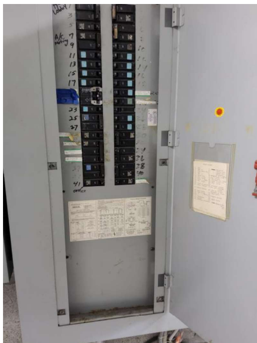
Photo # 11. Item 7.4.b. Meter Electrical Room. Panelboard HOUSE. Missing screws.
