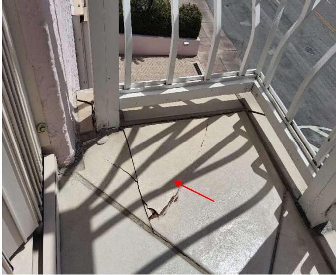
Photo # 25. Cracked tiles at the balcony around the railing post.
