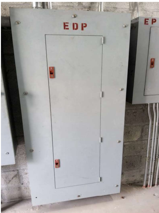
Photo # 7. Item 7.1. Meter Electrical Room. Panelboard EDP. Missing screws.
