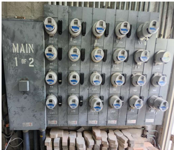
Photo # 3. Item 4.1.a. Meter Electrical Room. Meter Units.
