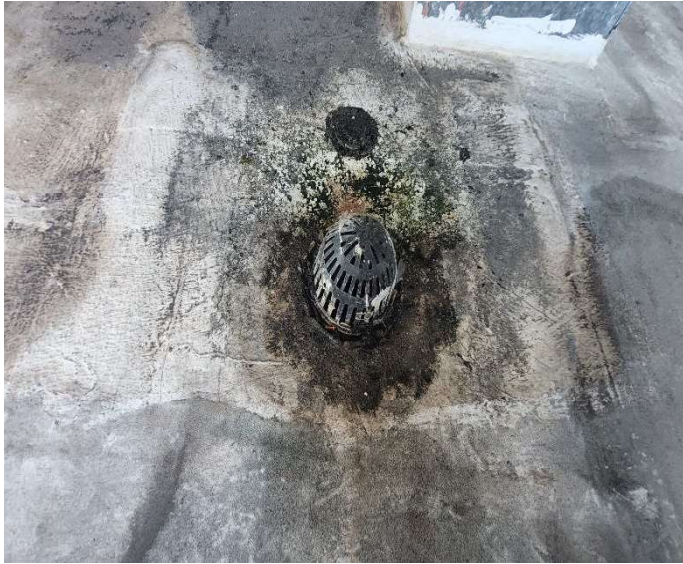
Photo # 13. Primary drain at the lower roof.
