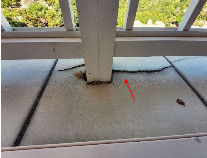
Photo # 33. Cracked tile around the railing post.
