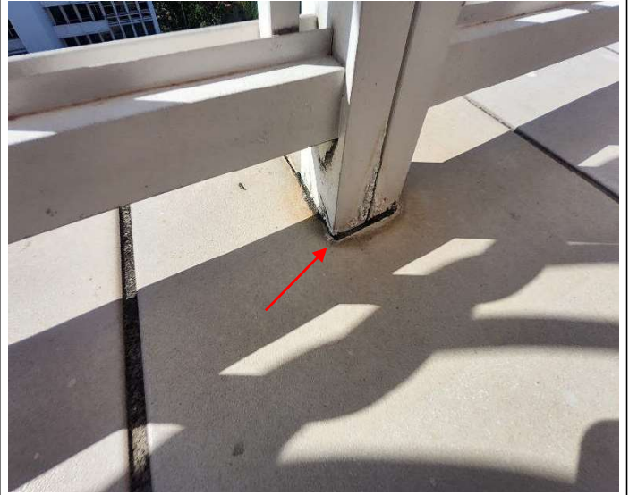
Photo # 30. Pitting corrosion at the balcony railing post throughout.
