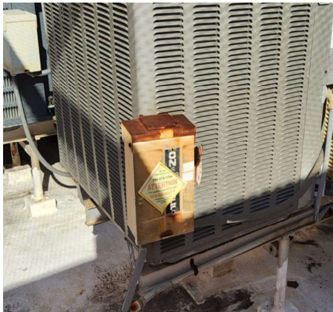
Photo # 27. Item 27.b. Roof. Disconnect Switch is unsafely rusted.
