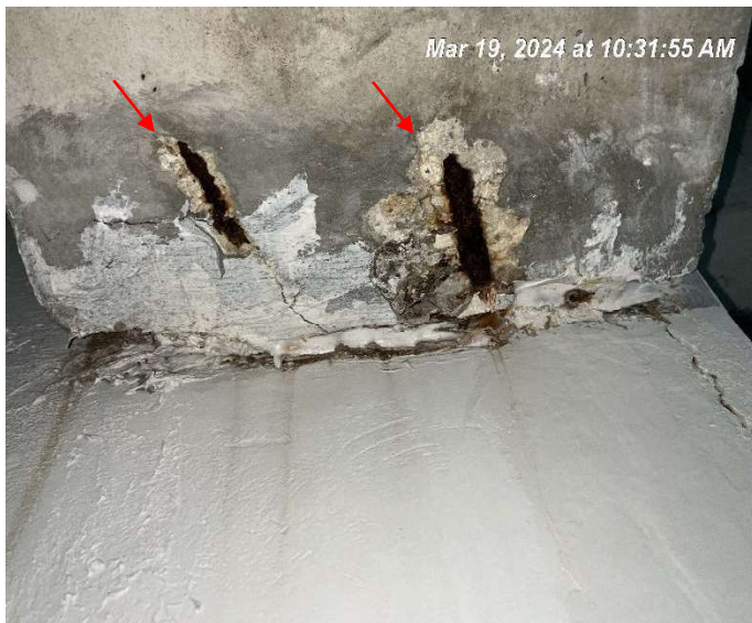
Photo # 39. Spalled concrete with exposed corroded rebar at the beam of the parking garage.
