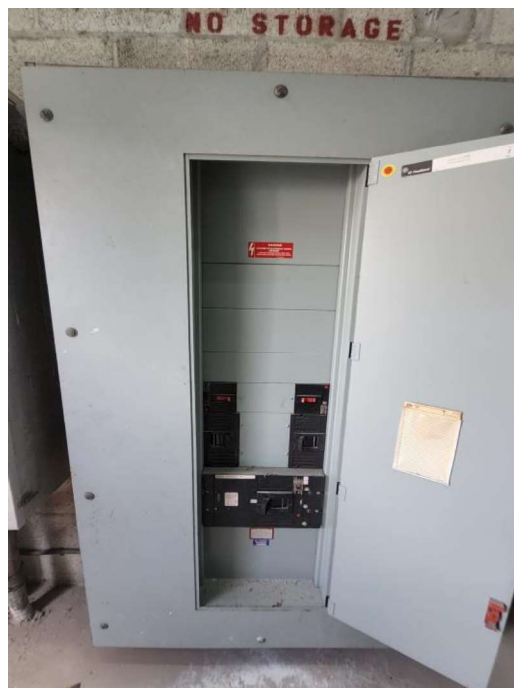
Photo # 2. Item 3.2. Meter Electrical Room. Panelboard. Main 2 of 2. Missing proper circuit identification.
