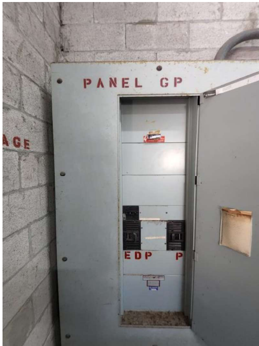
Photo # 13. Item 7.6. Meter Generator - Fire Pump Room. Panelboard GP. Missing proper circuit identification.
