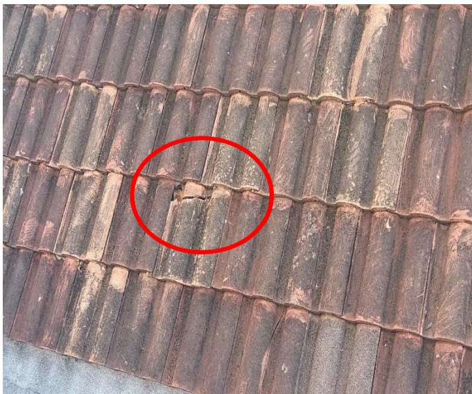
Photo # 23. Cracked clay barrel tile at the PH floor roof.
