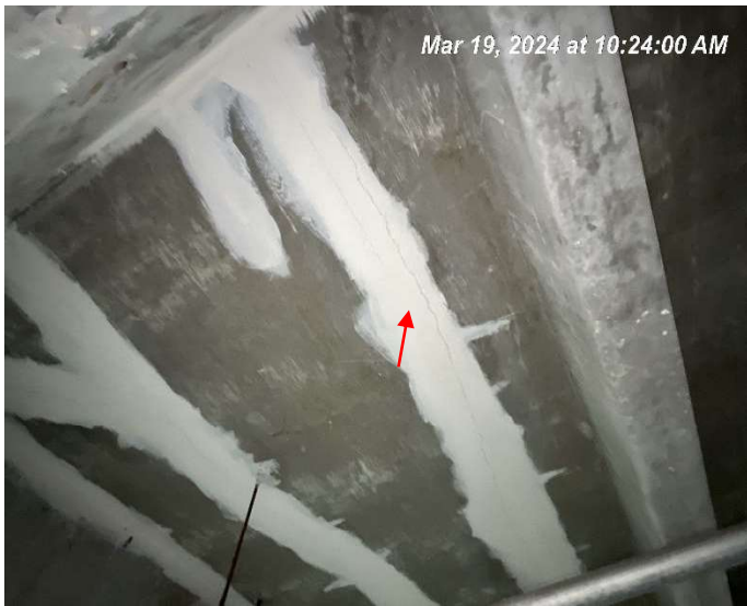
Photo # 35. Concrete crack at the ceiling slab of the basement garage.
