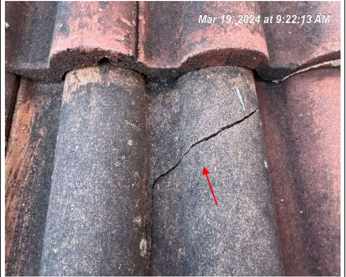
Photo # 22. Cracked clay barrel tile at the PH floor roof.
