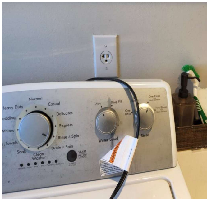
Photo # 35. Item 28.4. Missing GFCI protection for receptacles in the laundry.
