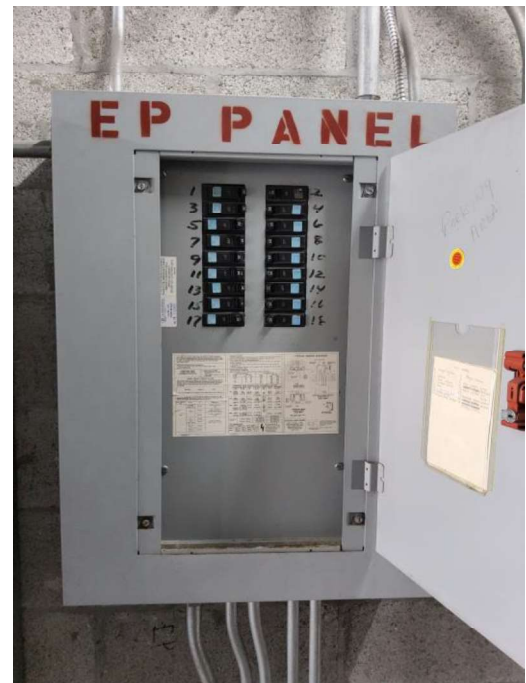
Photo # 8. Item 7.2. Meter Electrical Room. Panelboard EP. Missing proper circuit identification.
