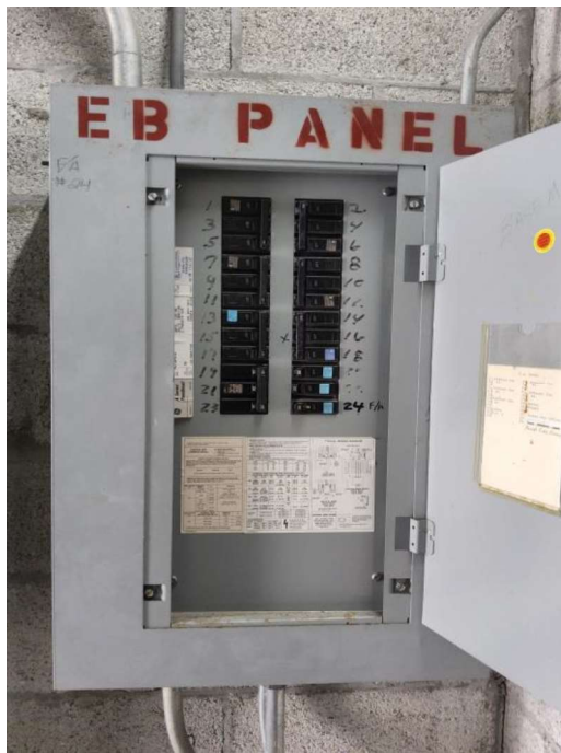
Photo # 9. Item 7.3. Meter Electrical Room. Panelboard EB.
