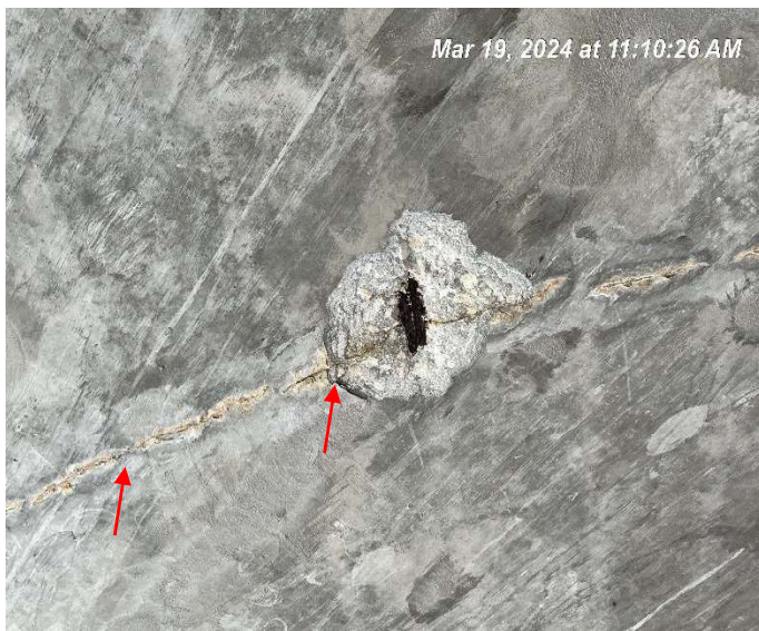
Photo # 43. Cracked and spalled concrete with exposed corroded rebar at the ramp ceiling slab (East Side)
