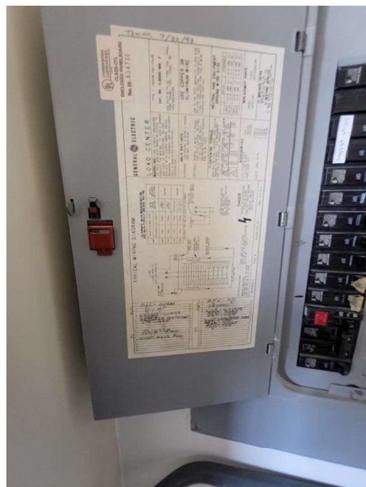
Photo # 40. Item 28.7. Electrical panel missing or incomplete proper circuit directory.
