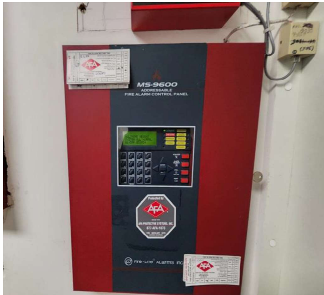
Photo # 19. Item 20.1. Level G. Fire Alarm Central Panel.
