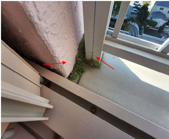
Photo # 31. Biological growth and pitting corrosion at the balcony railing post.
