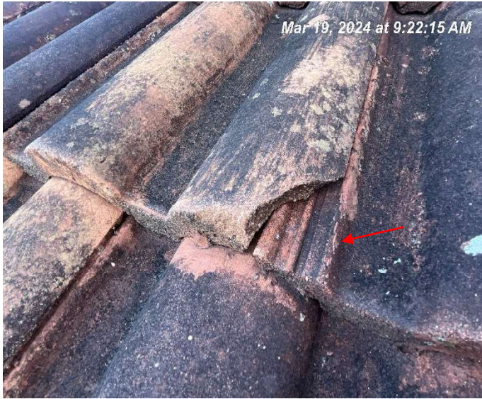
Photo # 21. Chipped clay barrel tile at the PH floor roof.
