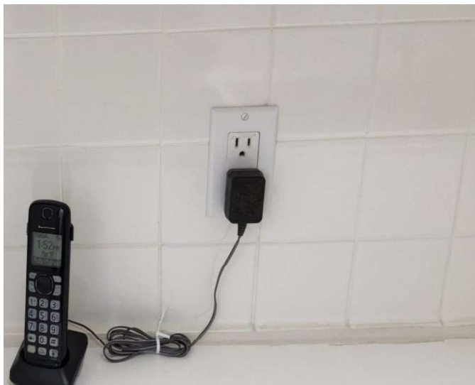
Photo # 15. Item 16.a. Conference Area. Kitchennete. Missing GFCI protection for receptacle - Test Fail.
