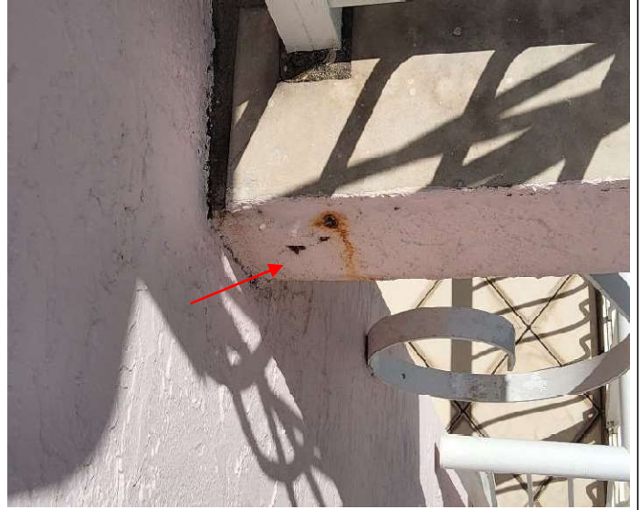
Photo # 26. Rust spot at the balcony slab edge.
