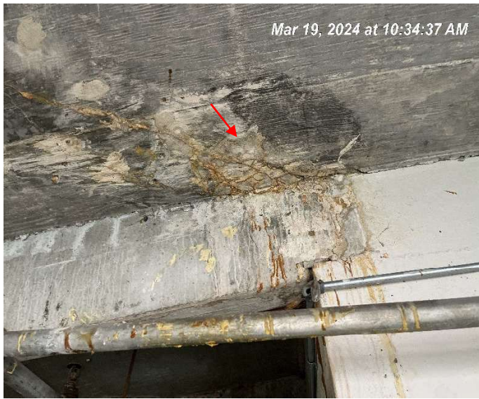
Photo # 41. Concrete crack with water stains and efflorescence at the ceiling slab of the basement garage.
