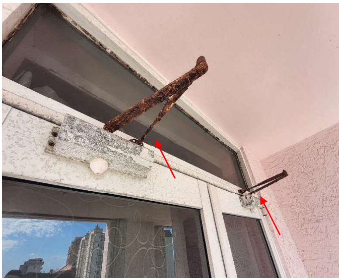
Photo # 27. Corroded door closer at the balcony throughout.
