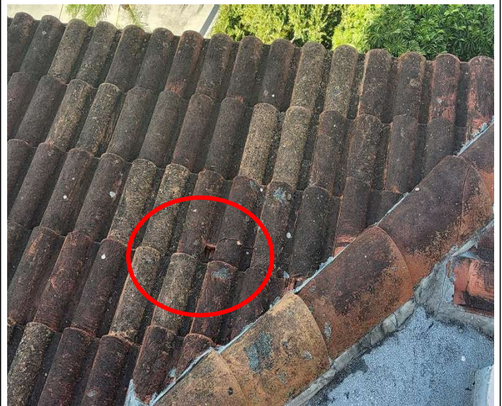
Photo # 24. Cracked clay barrel tile at the PH floor roof.
