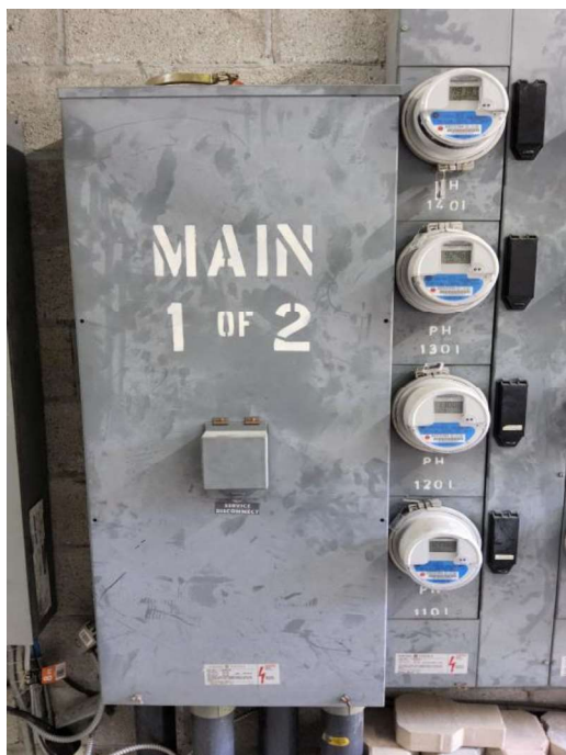
Photo # 1. Item 3.1. Meter Electrical Room. Disconnect Switch. Main 1 of 2.
