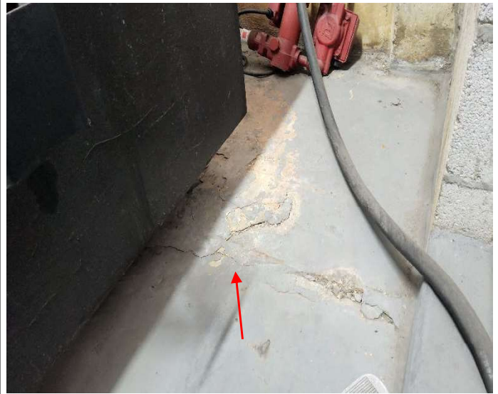
Photo # 46. Cracked and spalled concrete at the Generator & Fire Pump Room.
