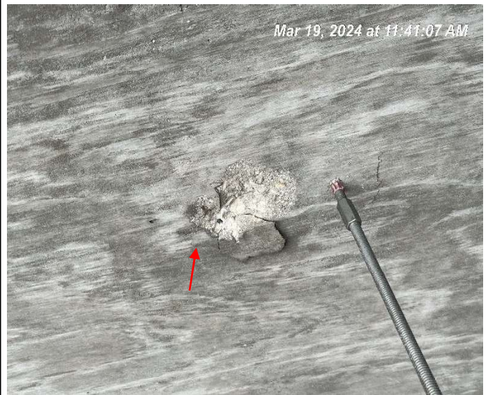
Photo # 44. Cracked and spalled concrete at the ramp ceiling slab (West Side)
