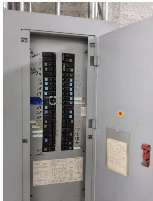
Photo # 10. Item 7.4.a. Meter Electrical Room. Panelboard HOUSE. Missing proper circuit identification.
