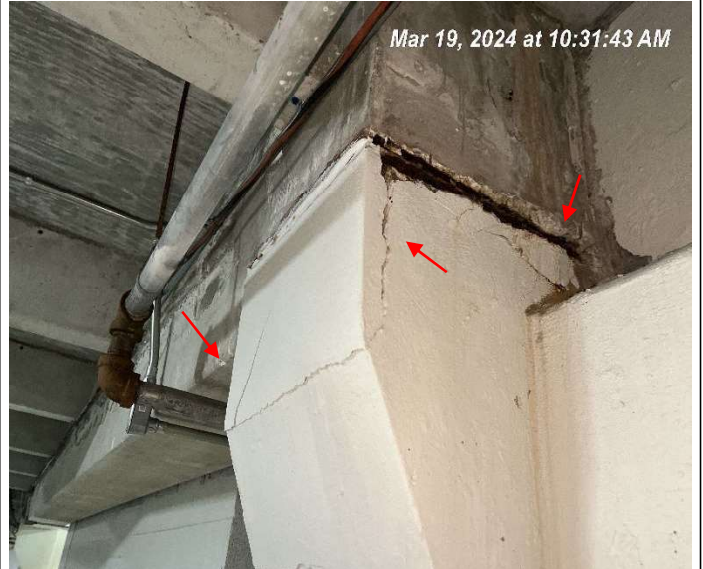
Photo # 38. Cracked and delaminated concrete at the column of the basement garage.
