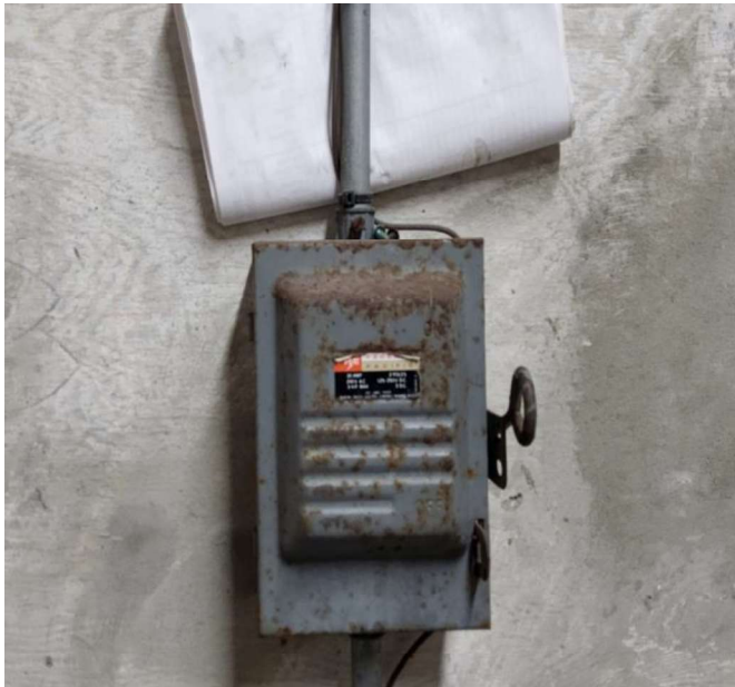
Photo # 25. Item 26.b. Pool pump. Disconnect switch is unsafely rusted.
