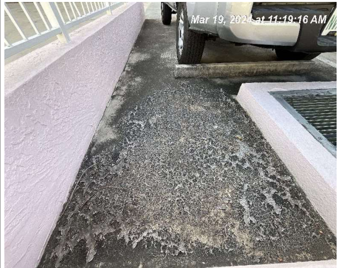
Photo # 48. Deteriorated waterproofing coating at the parking deck.
