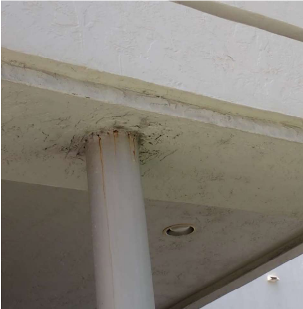
Photo # 35 Column rusting at lobby level at entrance
