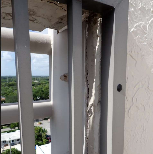
Photo # 15 Cracked stucco at penthouse roof
