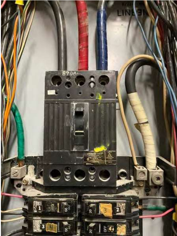
Electrical Equipment - PHOTO-05
