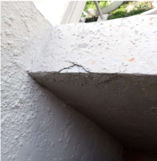
Photo # 51 Spalled stucco on balcony unit 201
