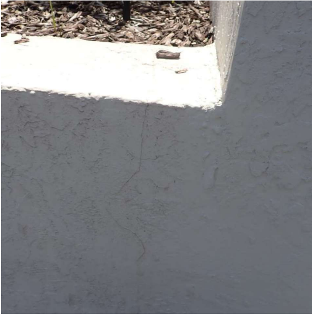
Photo # 11 Cracked stucco at entrance planter wall
