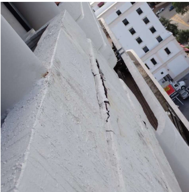
Photo # 17 Cracked stucco at penthouse balcony
