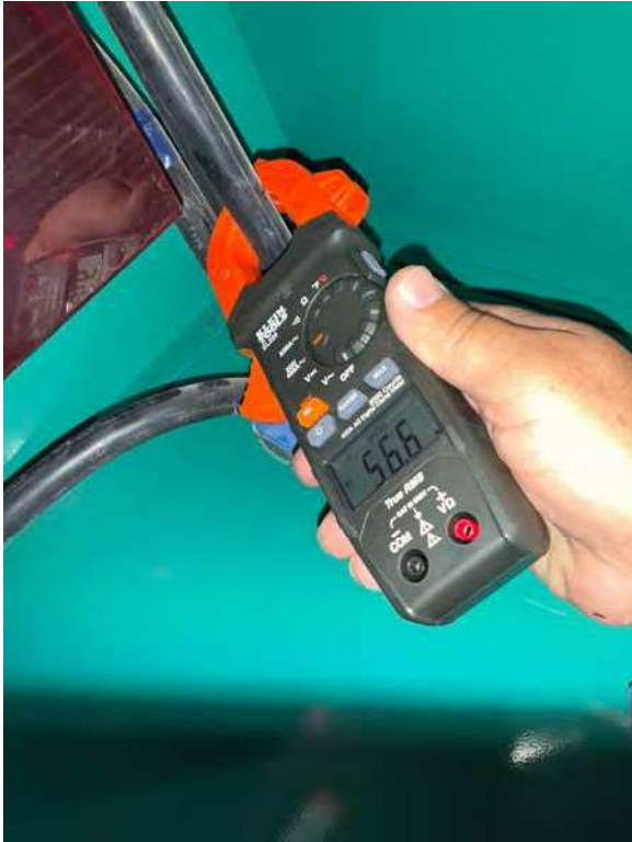
Electrical Equipment - PHOTO-13
