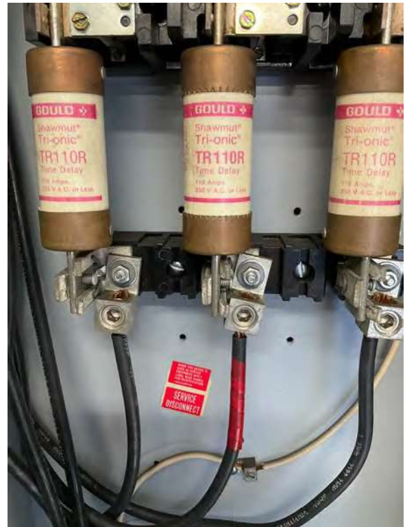
Electrical Equipment - PHOTO-36
