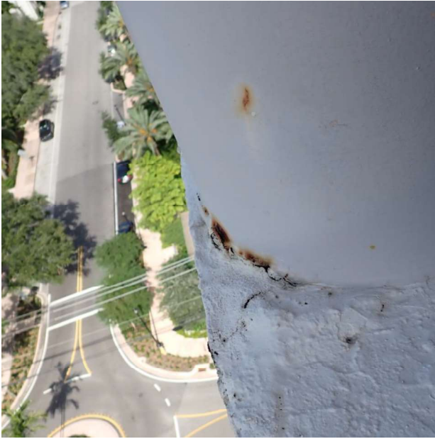
Photo # 39 Corroded column at penthouse
