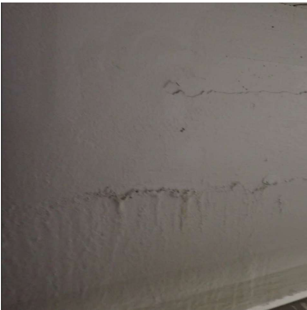
Photo # 78 Sign of water intrusion in garage wall
