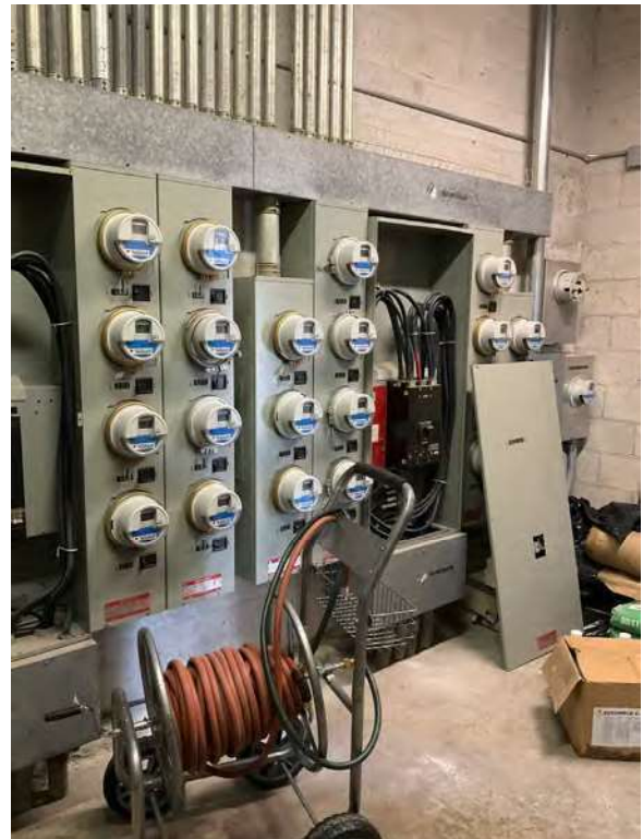
Electrical Equipment - PHOTO-12
