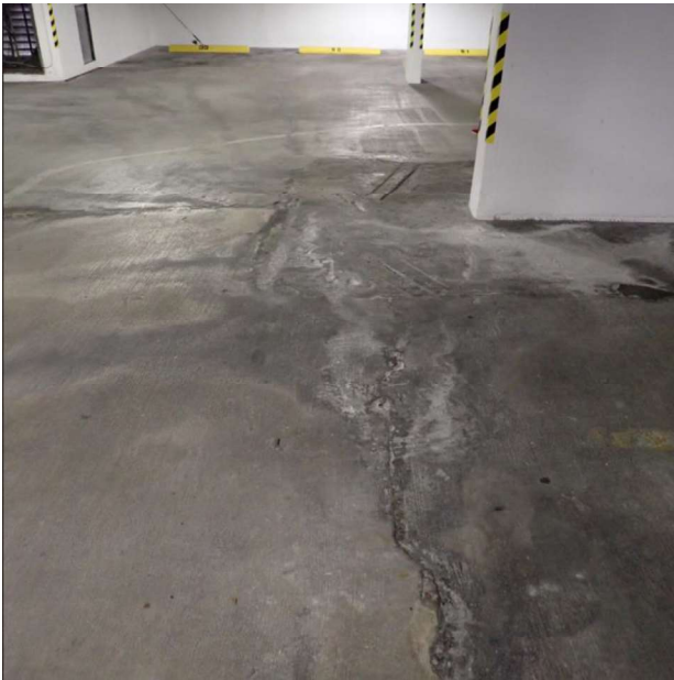
Photo # 82 Crack in garage floor, seemingly around the outline of the footer
