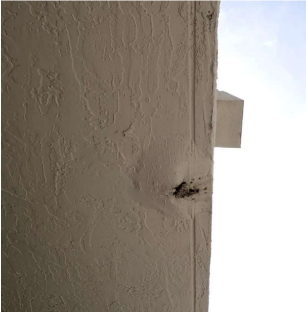
Photo # 49 Water bubble up on balcony above 1102
