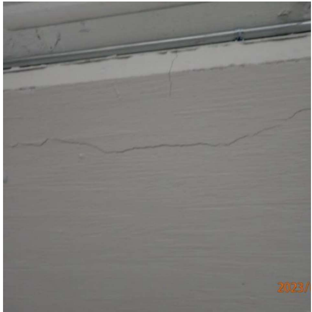
Photo # 75 Crack in garage beam and ceiling
