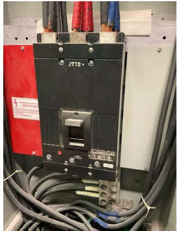
Electrical Equipment - PHOTO-18
