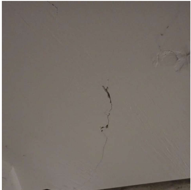
Photo # 71 Wall crack
