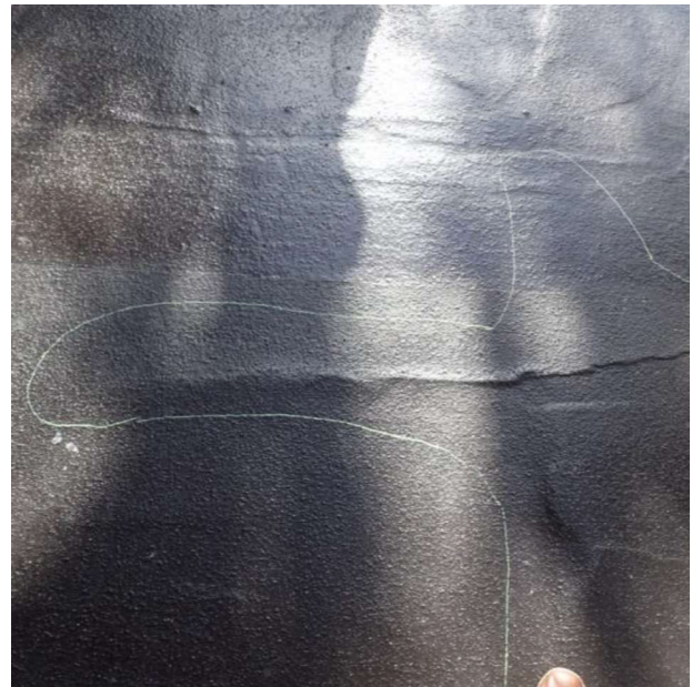
Photo # 34 Driveway cracked and spalled
