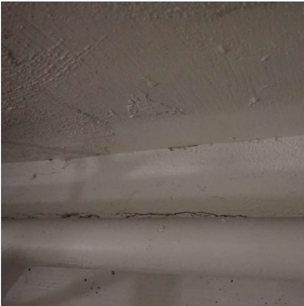
Photo # 70 Crack in garage ceiling near pipes running longitudinal
