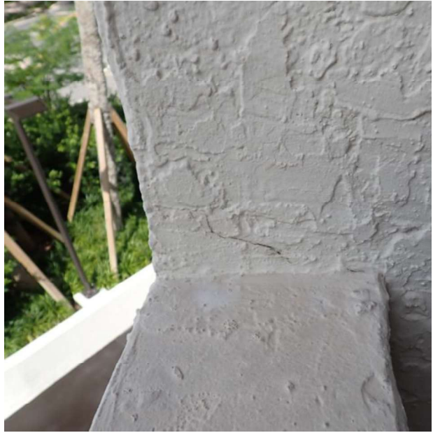
Photo # 54 Cracked stucco on balcony unit 201
