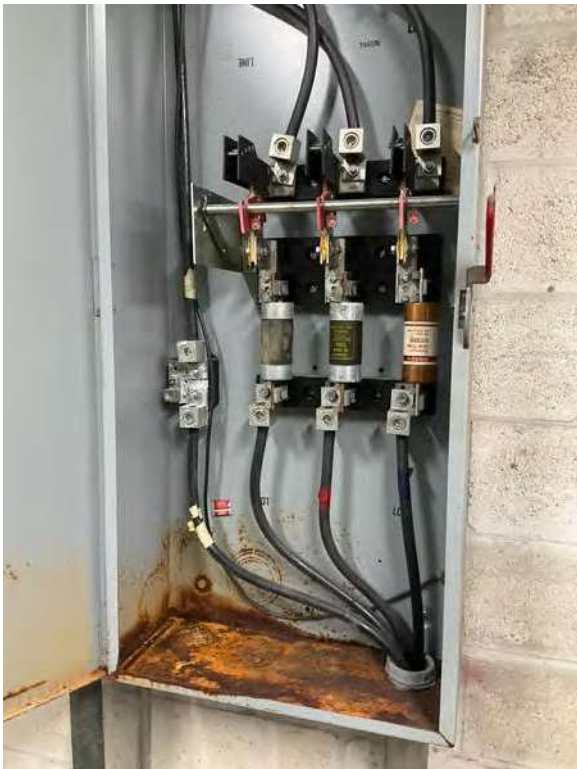
Electrical Equipment - PHOTO-27
