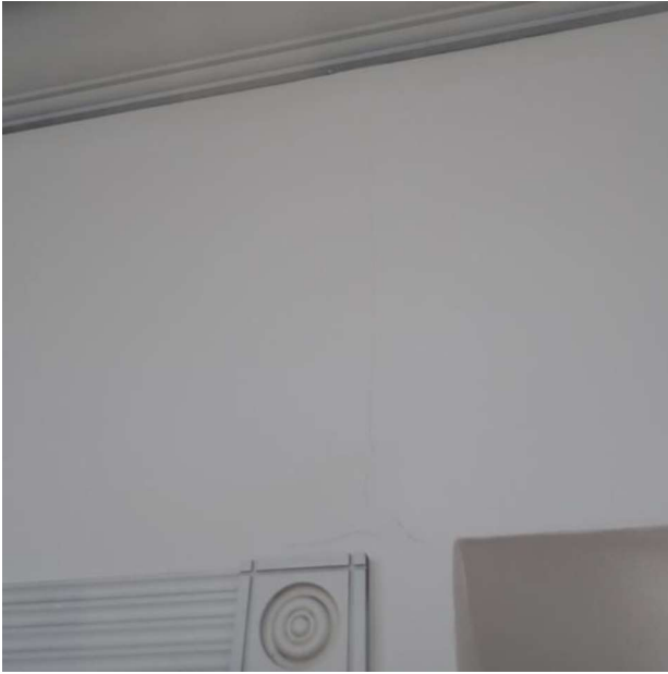
Photo # 57 Wall crack at door in penthouse
