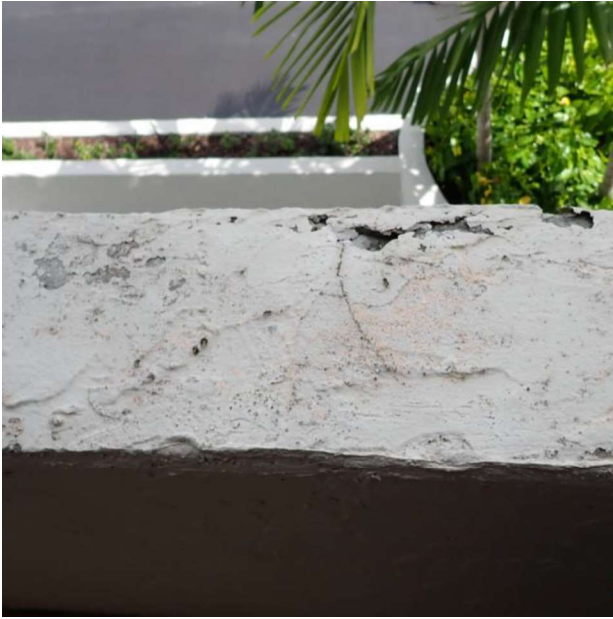
Photo # 53 Spalled stucco on balcony unit 201
