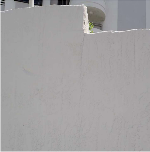
Photo # 3 Cracked stucco at entrance planter wall
