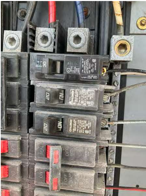
Electrical Equipment - PHOTO-31
