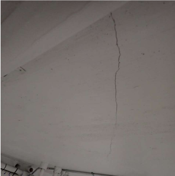
Photo # 72 Crack in garage ceiling
