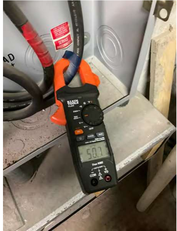
Electrical Equipment - PHOTO-22
