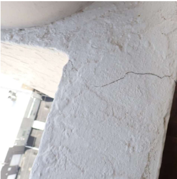
Photo # 29 Cracked stucco at penthouse railing
