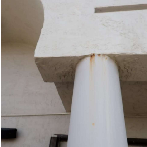
Photo # 40 Corrosion spots on column by pool
