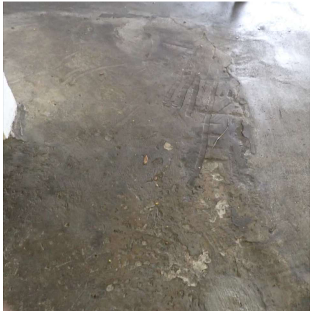
Photo # 83 Crack in garage floor around outline of footer
