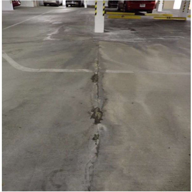
Photo # 81 Crack in garage floor
