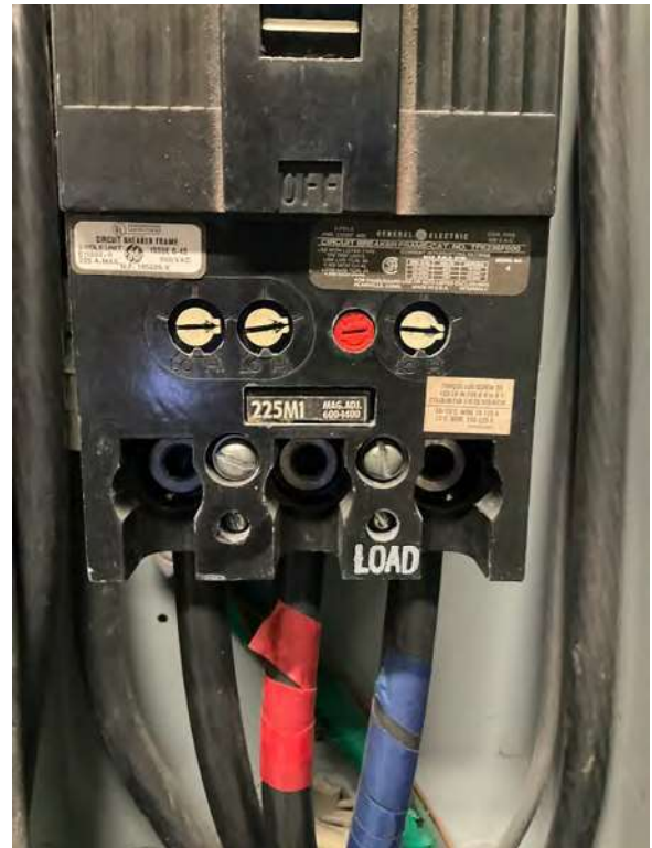
Electrical Equipment - PHOTO-20
