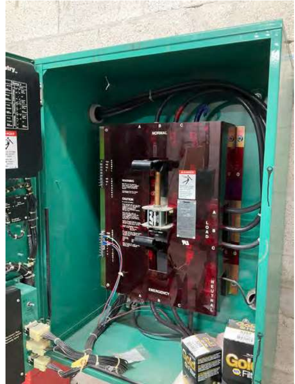
Electrical Equipment - PHOTO-26
