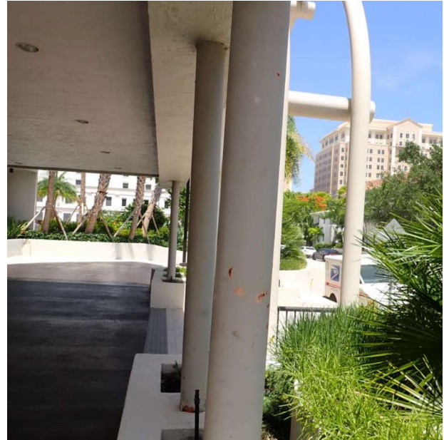
Photo # 36 Rust spots on column at building entrance
