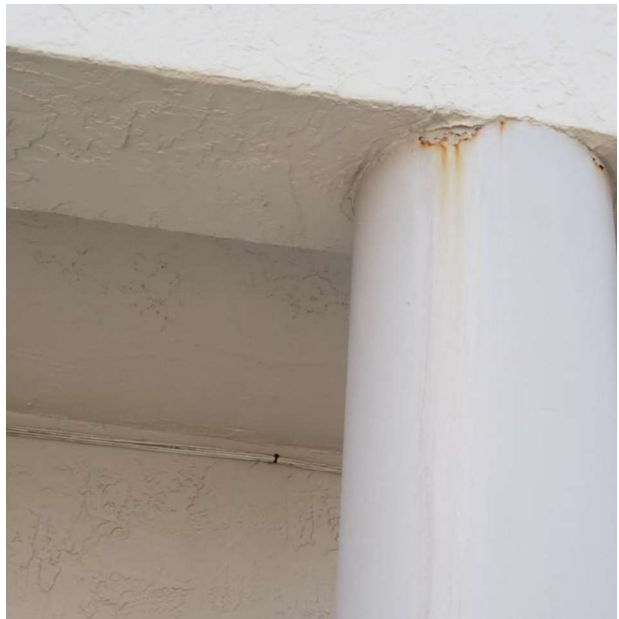
Photo # 42 Corroded column at penthouse
