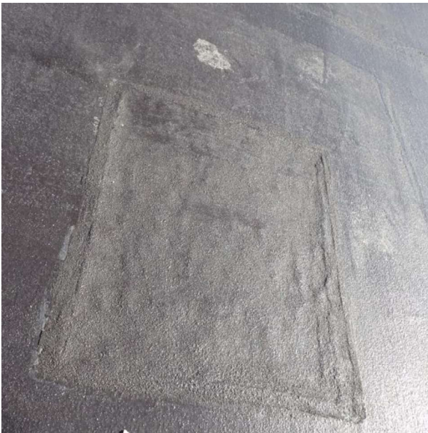
Photo # 33 Driveway cracked and spalled
