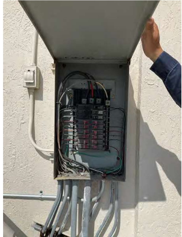
Electrical Equipment - PHOTO-30
