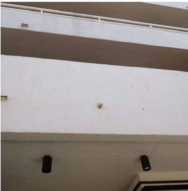
Photo # 5 Vegetation growth in stucco at front balcony of building
