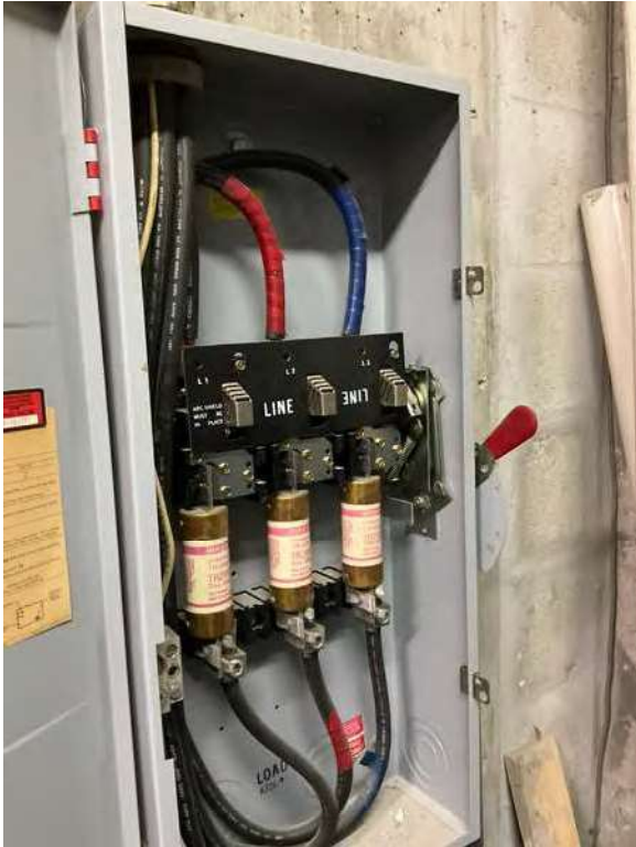
Electrical Equipment - PHOTO-21
