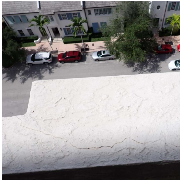
Photo # 48 Cracked stucco on balcony unit 1102
