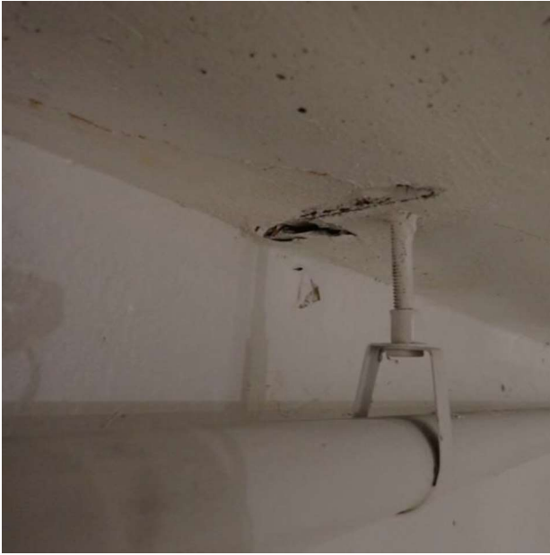
Photo # 76 Spalling concrete in the ceiling
