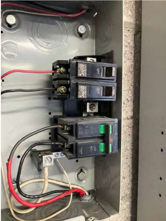
Electrical Equipment - PHOTO-01
