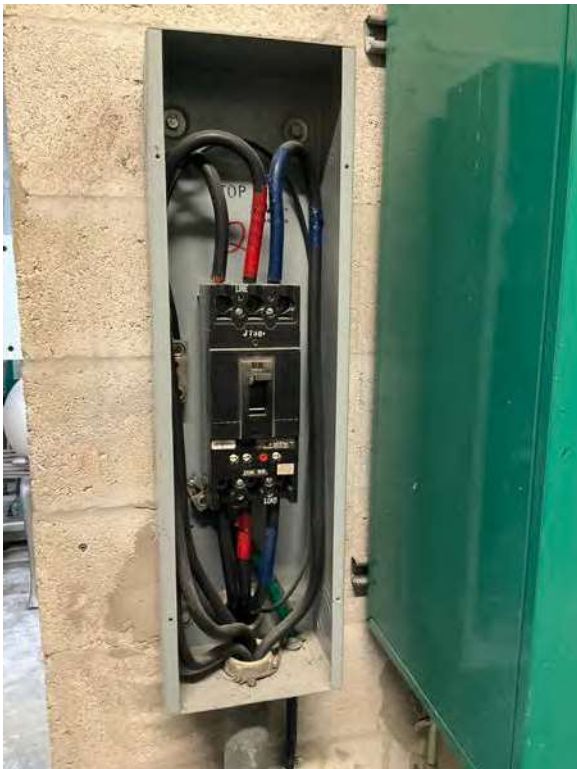
Electrical Equipment - PHOTO-15
