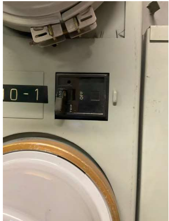
Electrical Equipment - PHOTO-16
