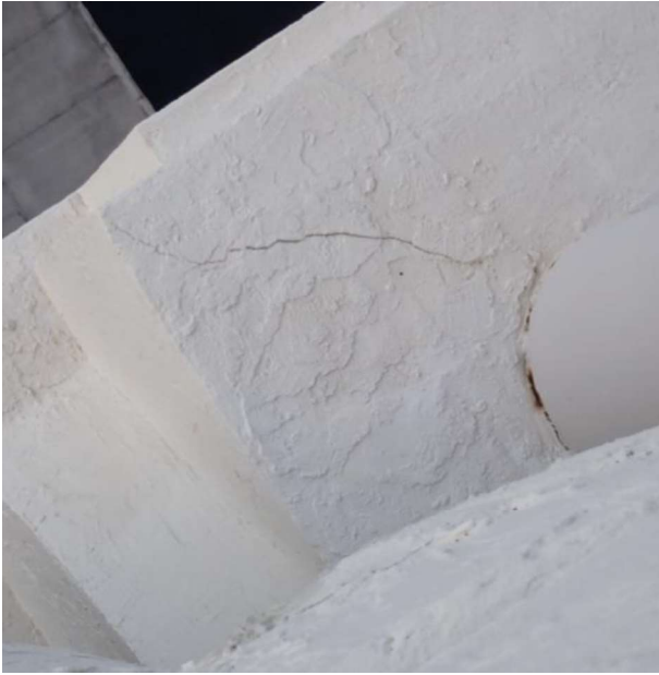
Photo # 19 Cracked stucco at bottom of column
