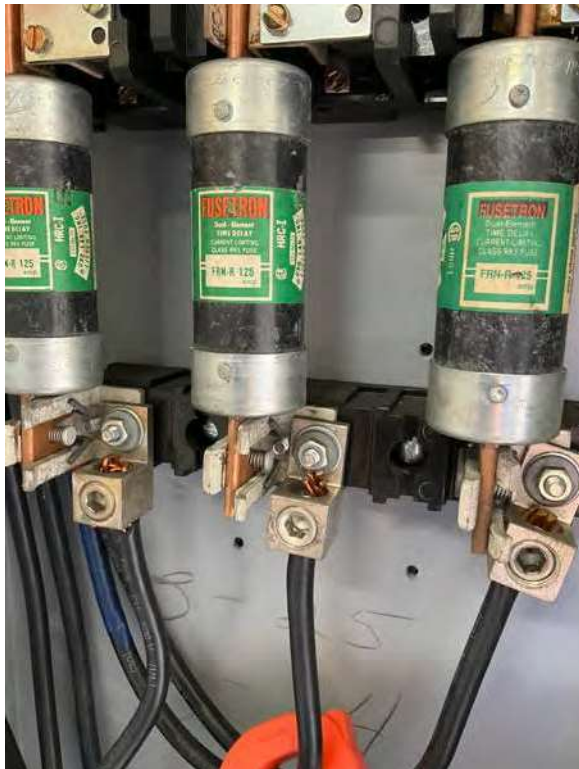
Electrical Equipment - PHOTO-35
