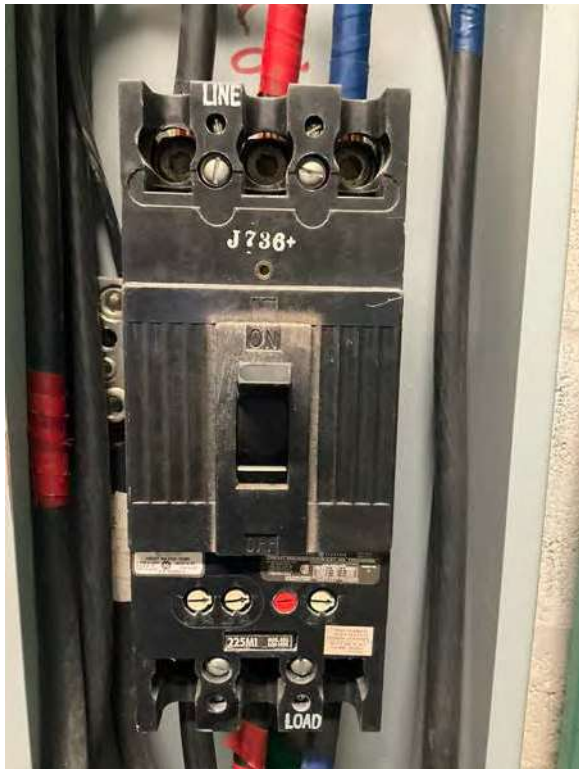
Electrical Equipment - PHOTO-19
