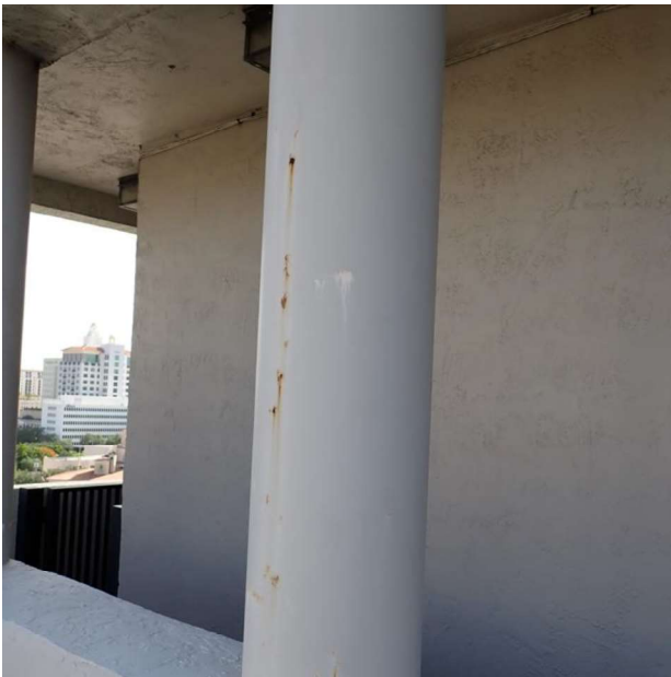
Photo # 41 Corroded column at penthouse
