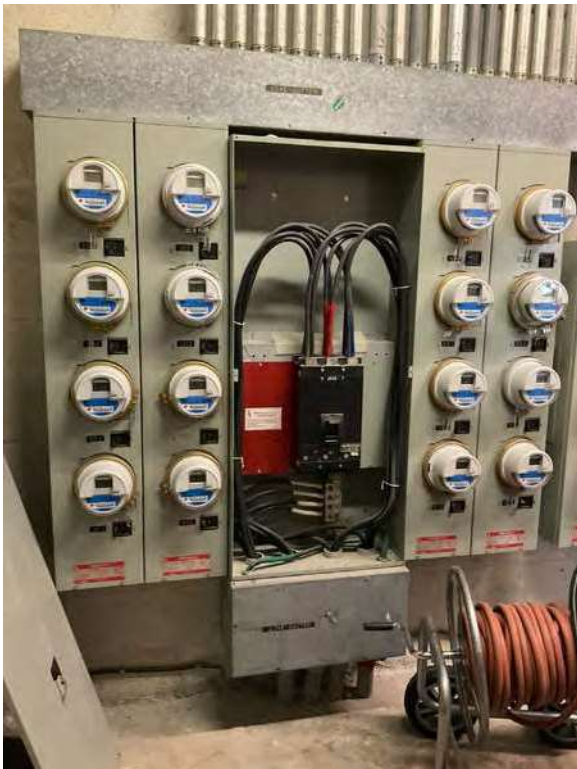
Electrical Equipment - PHOTO-11
