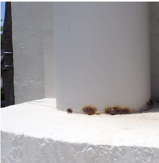
Photo # 37 Corroded column bottom at pool
