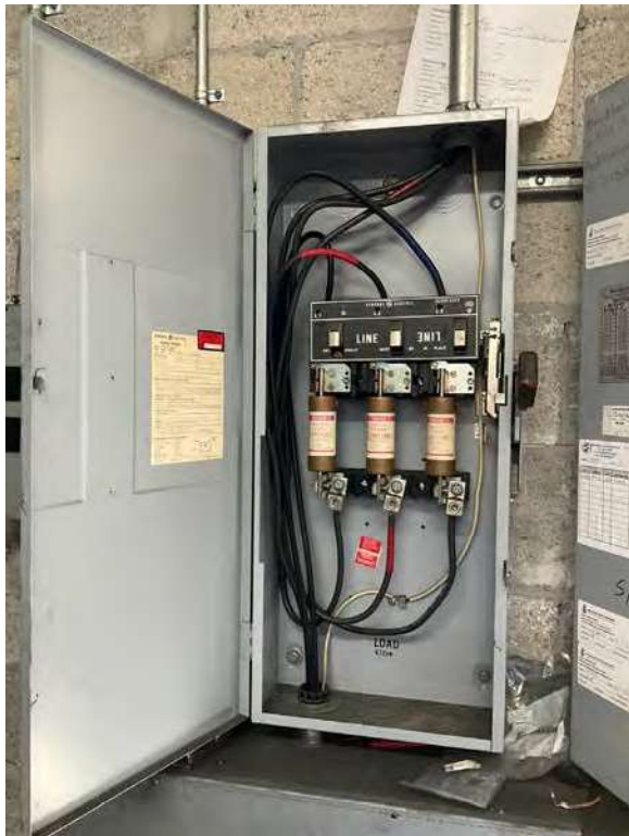
Electrical Equipment - PHOTO-33
