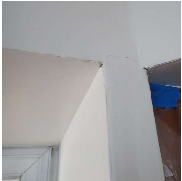
Photo # 56 Wall crack at door in penthouse
