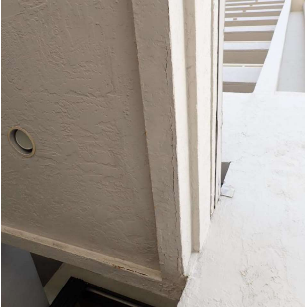
Photo # 7 Cracked stucco at entrance canopy
