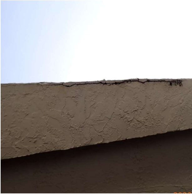
Photo # 27 Cracked stucco at penthouse level railing
