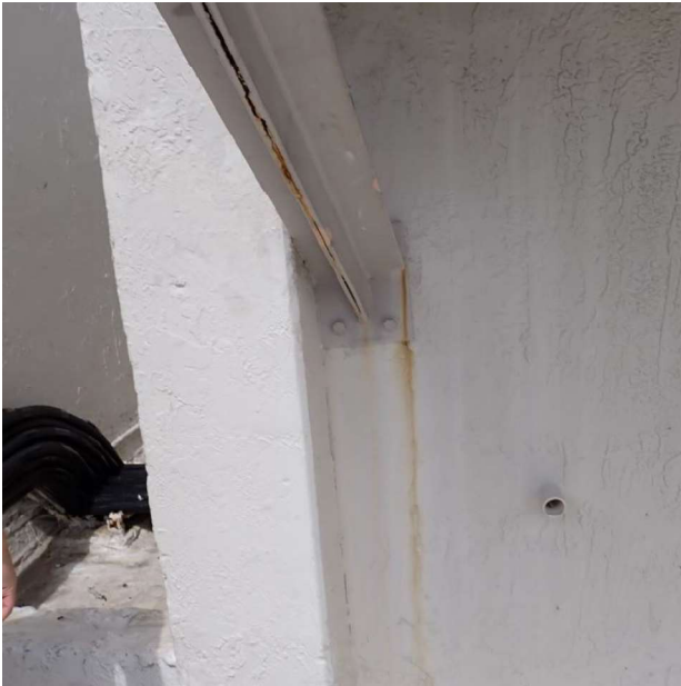
Photo # 60 Corroded bracing frame angles
