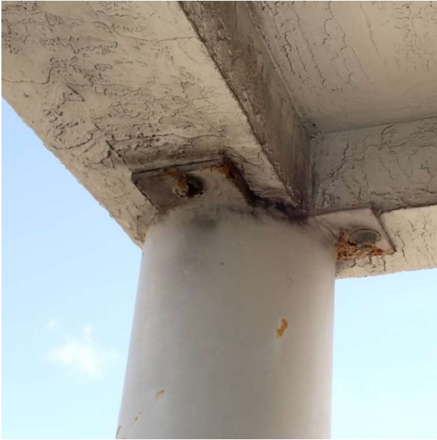
Photo # 43 Corroded column anchors at penthouse
