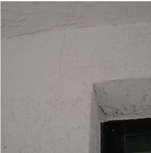
Photo # 1 Stucco crack at pool entrance door
