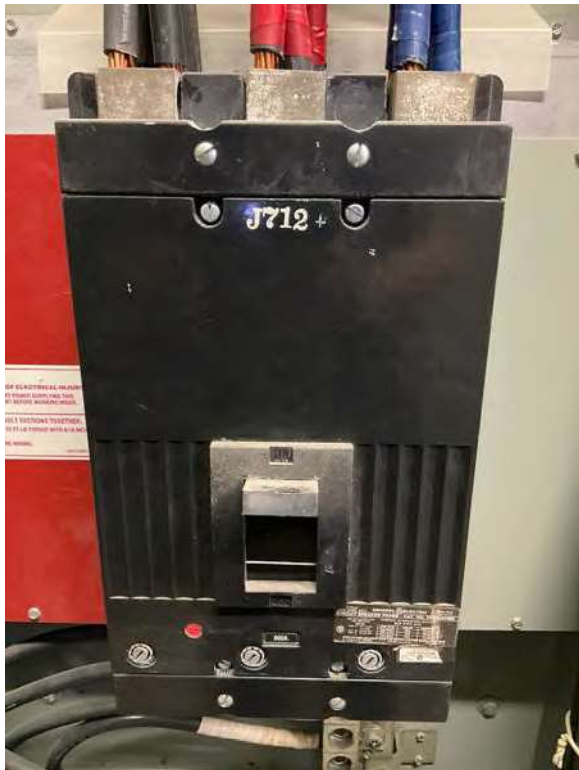
Electrical Equipment - PHOTO-17
