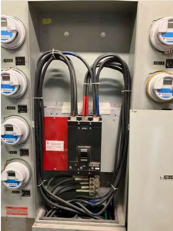
Electrical Equipment - PHOTO-09
