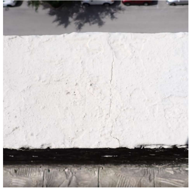
Photo # 50 Cracked balcony stucco in unit 1102
