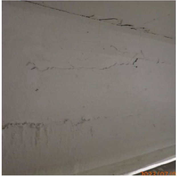
Photo # 77 Spalling concrete in ceiling and wall
