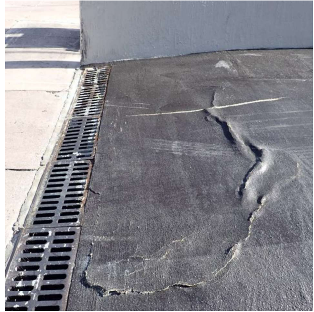
Photo # 32 Driveway cracked and spalled at west ramp
