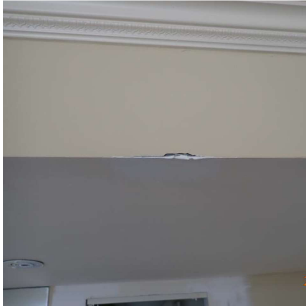
Photo # 58 Wall crack at door in unit 1102
