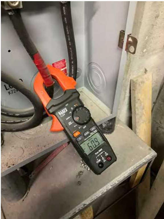
Electrical Equipment - PHOTO-23
