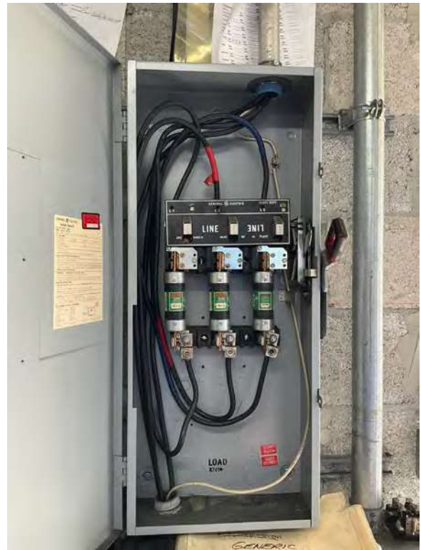
Electrical Equipment - PHOTO-32
