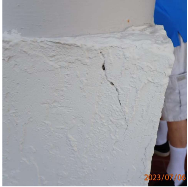
Photo # 28 Crack in stucco at penthouse level
