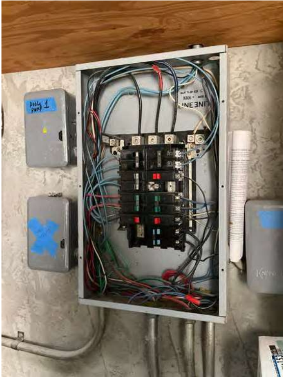
Electrical Equipment - PHOTO-29
