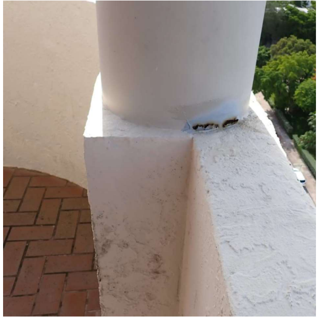
Photo # 44 Corroded column at penthouse
