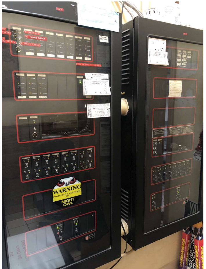
Photo 12 - Fire Alarm System
