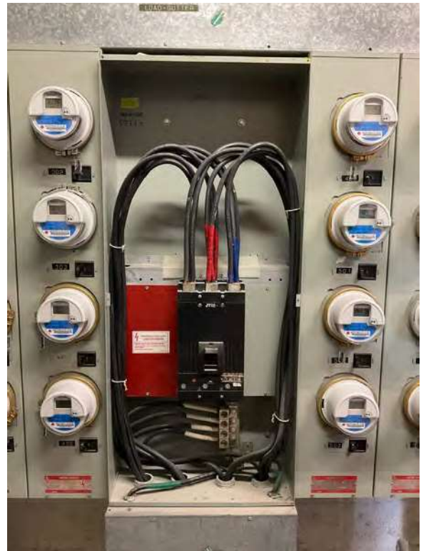
Electrical Equipment - PHOTO-08
