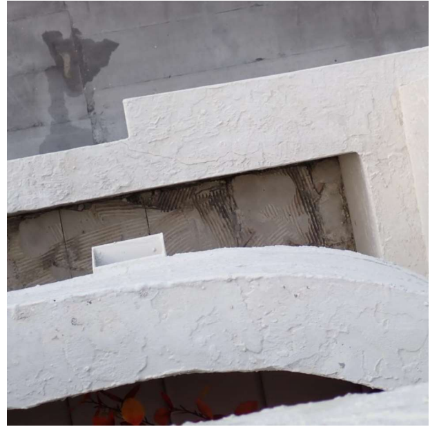
Photo # 20 Cracked balcony on lower floor
