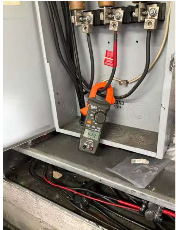
Electrical Equipment - PHOTO-34
