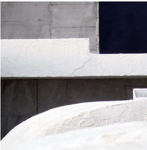
Photo # 21 Cracked balcony at lower level
