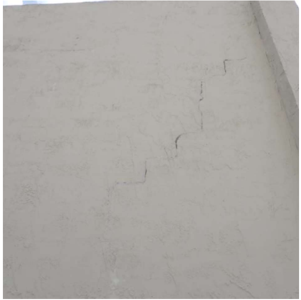
Photo # 63 Stucco crack in wall
