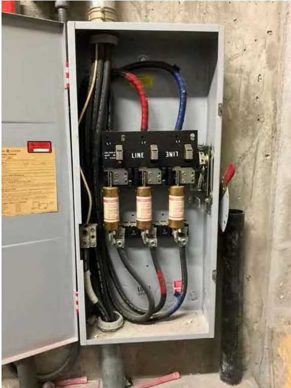
Electrical Equipment - PHOTO-25
