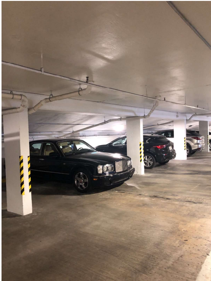
Photo 15 - Wiring in Parking Garage
