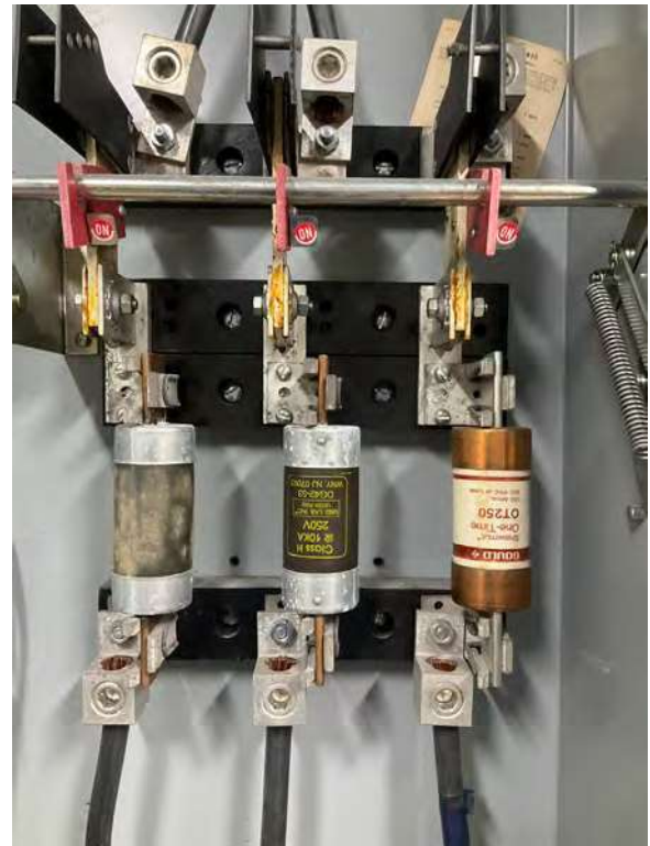
Electrical Equipment - PHOTO-28
