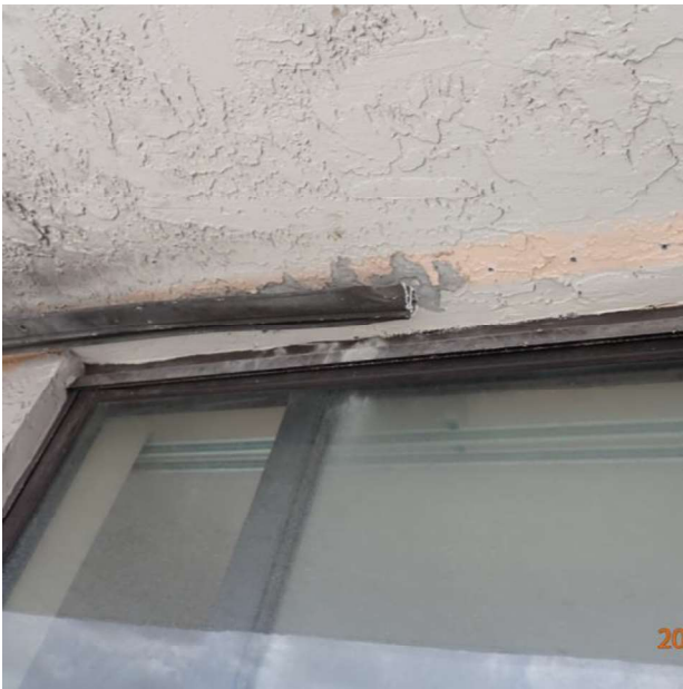
Photo # 59 Previous hurricane shutter bolt holes in unit 1102
