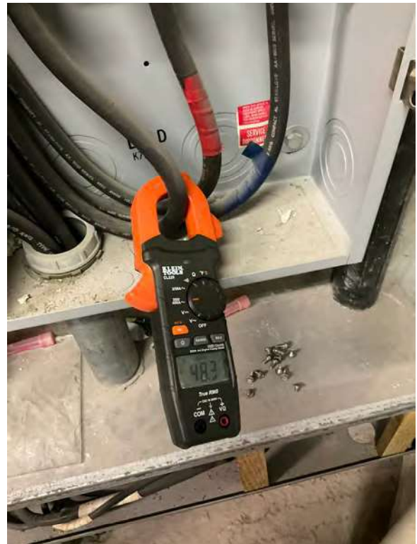
Electrical Equipment - PHOTO-24
