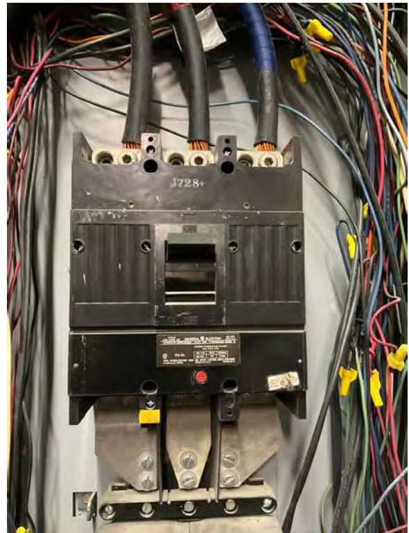
Electrical Equipment - PHOTO-04
