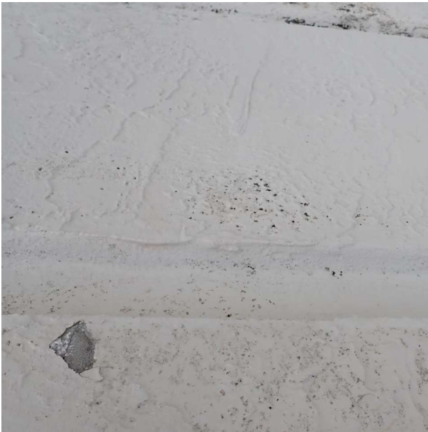
Photo # 47 Spalled stucco on balcony unit 1202
