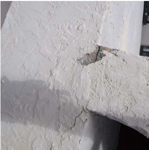
Photo # 25 Cracked balcony wall at penthouse level
