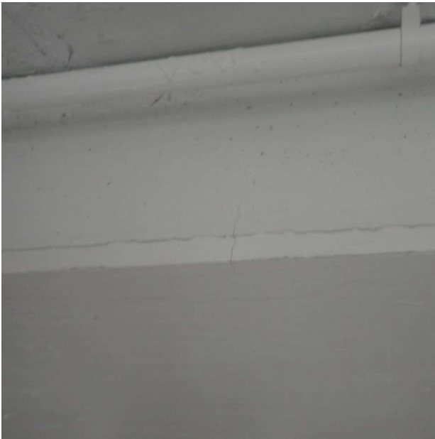
Photo # 74 Crack in garage beam
