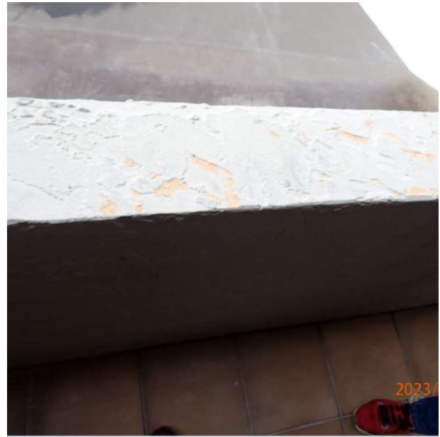
Photo # 52 Chipped paint on balcony unit 201
