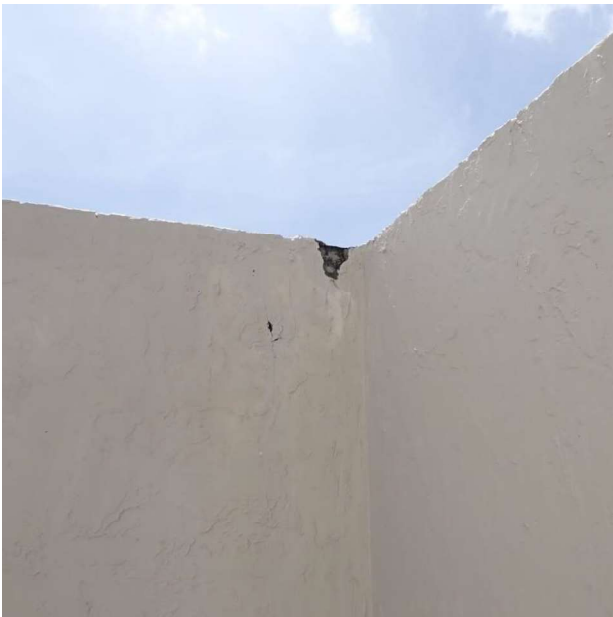
Photo # 64 Spalling stucco
