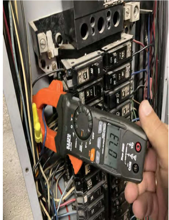
Electrical Equipment - PHOTO-14
