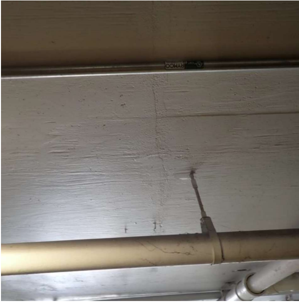
Photo # 68 Crack in garage ceiling
