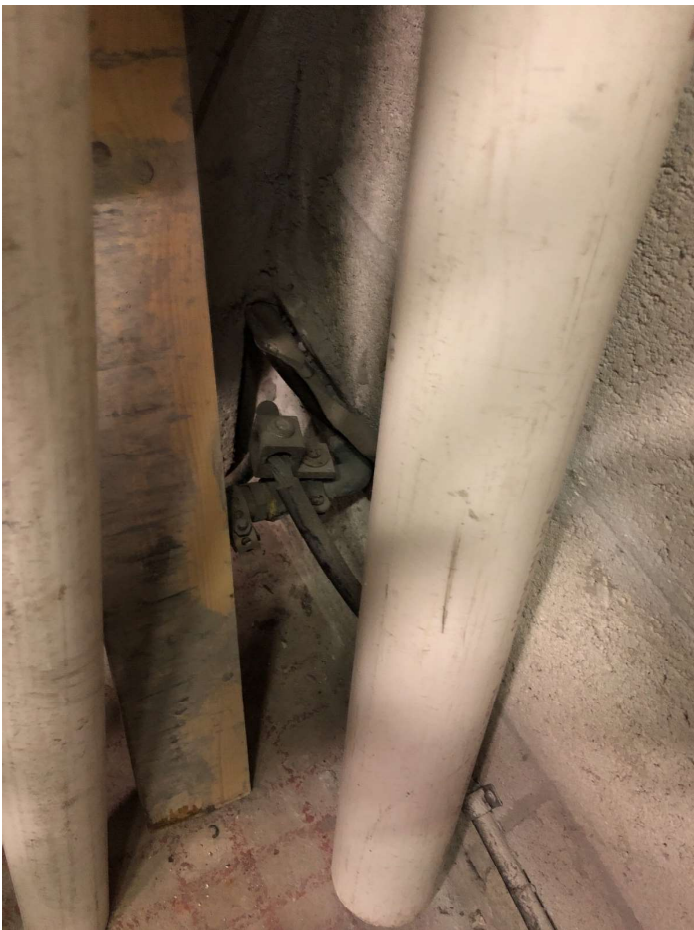
Photo 9 - Grounding of Service
