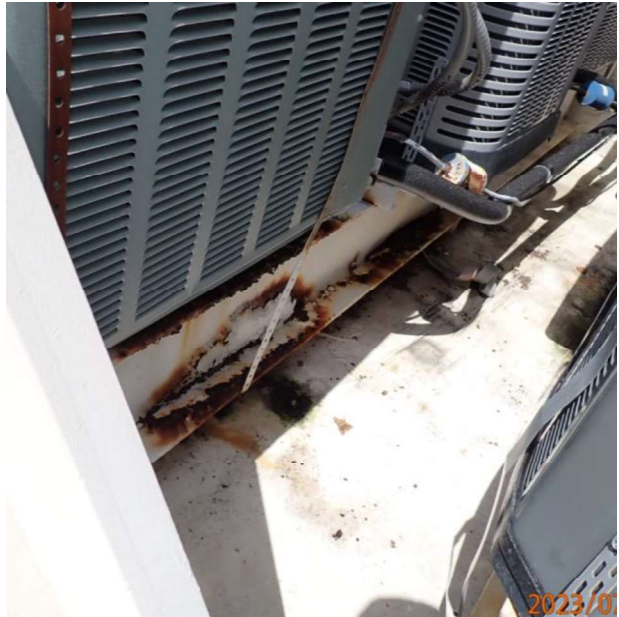
Photo # 61 Corroded machine support members
