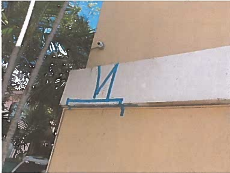
Beam Spall at 2 nd Floor West Main Elevation
