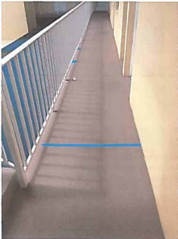
3 rd Floor Catwalk Horizontal Spalls
