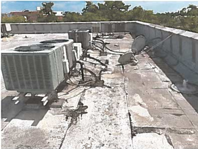
AC Compressors at Roof Deck
