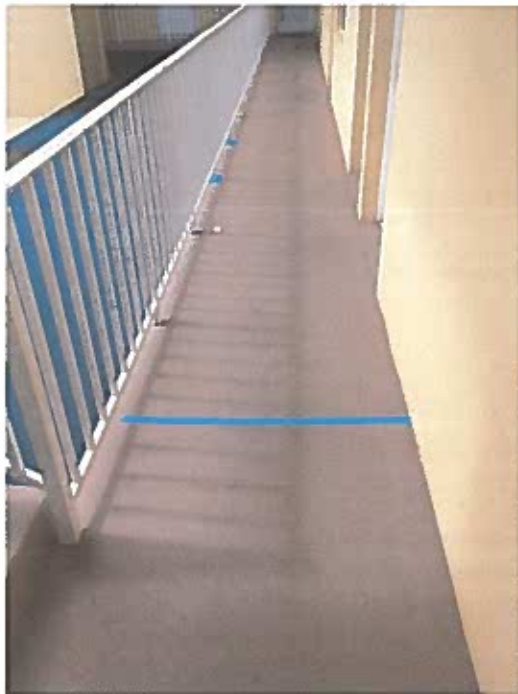
4 th Floor Catwalk Spalls
