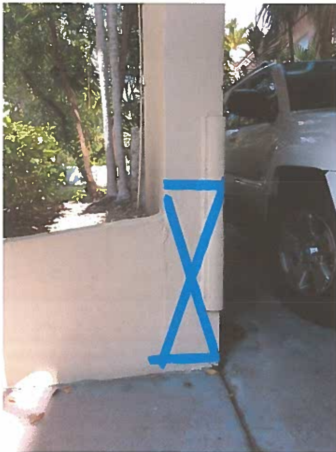
Column Spall at Garage East Entrance
