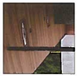
WOOD SIDING OVER MESH
