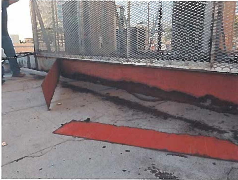
Bottom flange of Steel beam totally corroded
