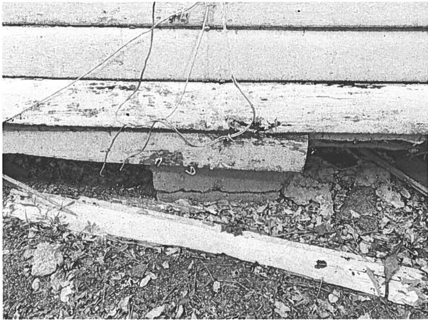
Picture #8 The house is on a crawl space supported by block pedestal without any structural connection
