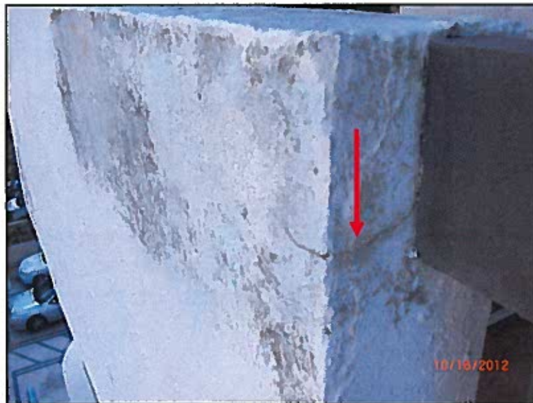
PHOTO # 6: Cracking stucco at balcony railing connection at Unit #407
