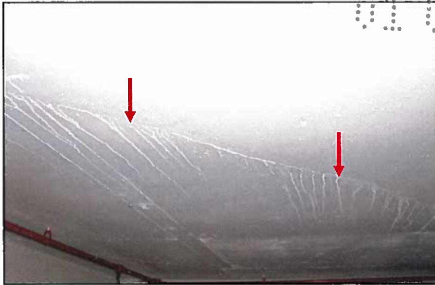
PHOTO # 23: cracking and water intrusion at underside of ramp in front of Parking Space 61
