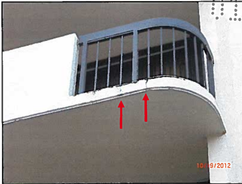
PHOTO # 29: cracking and staining on balcony edge
