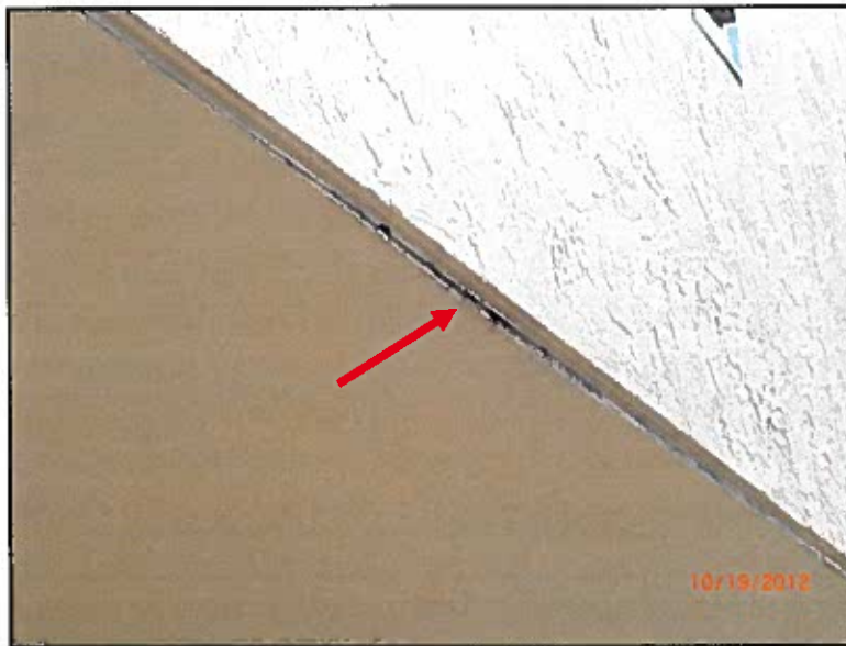
PHOTO # 36: ceiling separation at edge of South overhang
