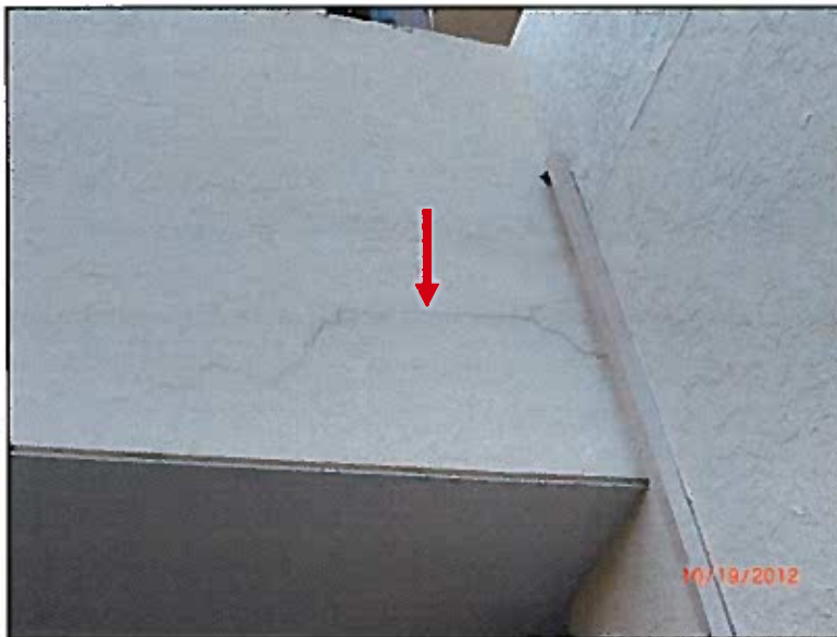
PHOTO # 28: cracking on overhang at West side
