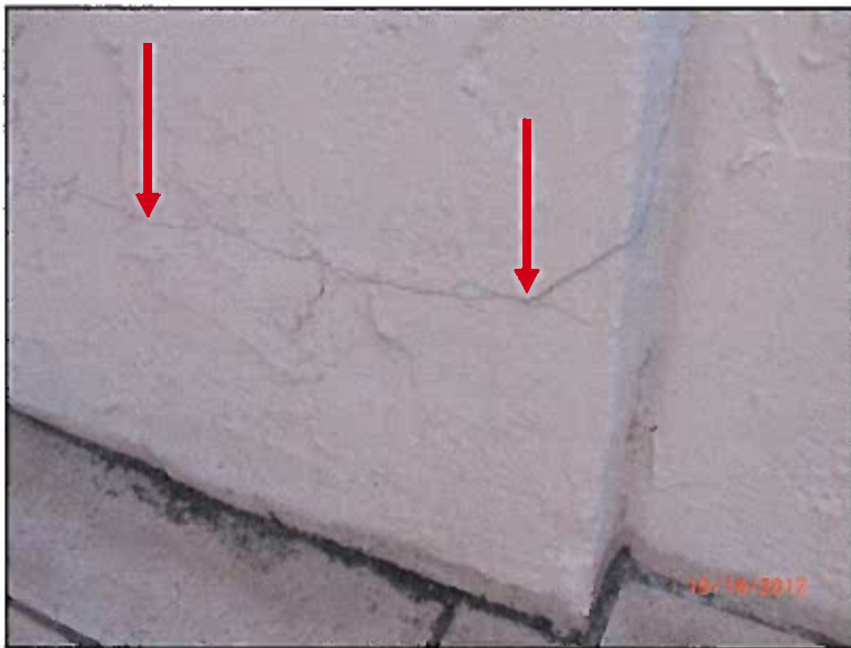
PHOTO # 2: Horizontal cracking/delaminated stucco at balcony wall Unit #219
