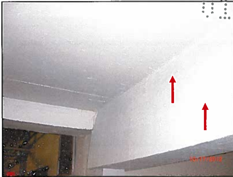
PHOTO # 17: slab cracking and beam cracks next to Parking Space 210
