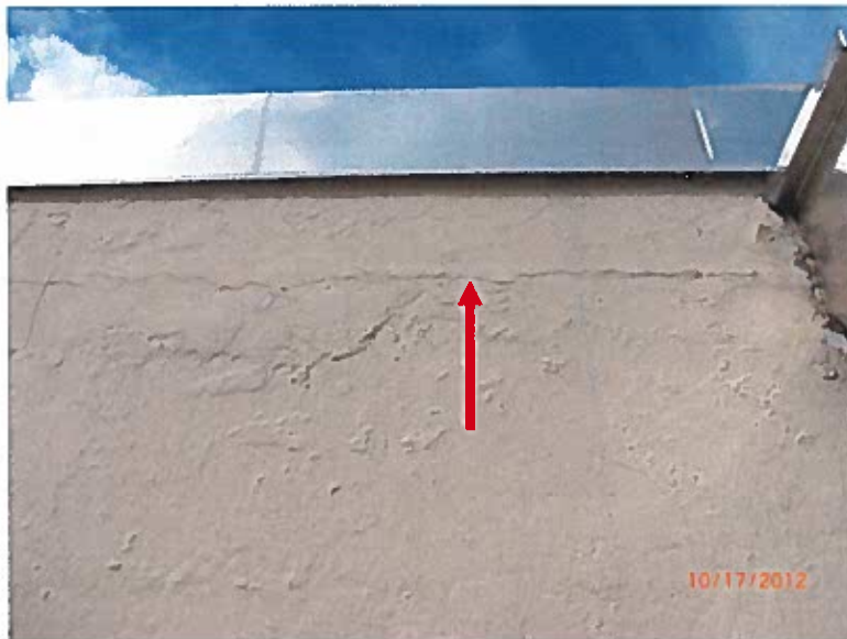
PHOTO # 10: Delaminated/cracking stucco at exterior of east Elevator Machine Room at Roof Area
