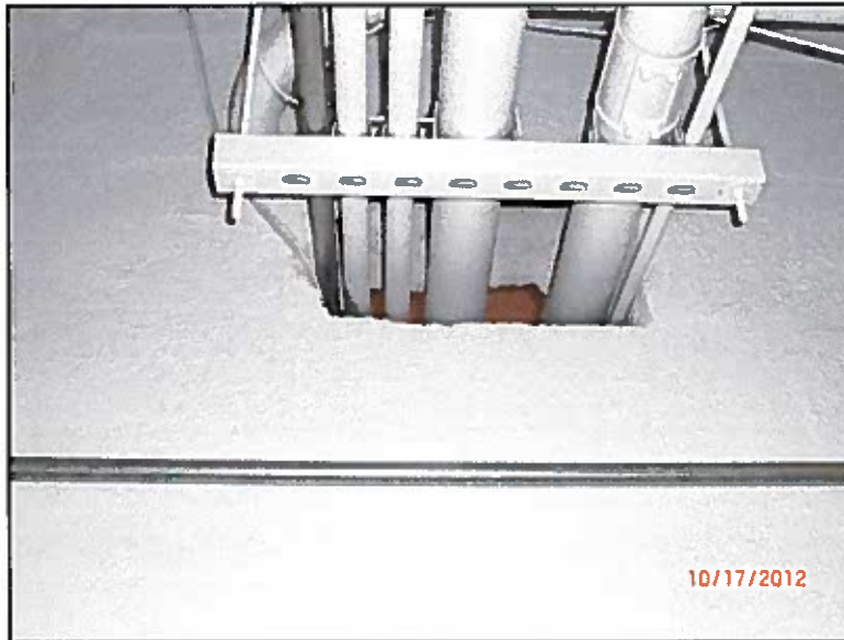
PHOTO # 16: Unsealed wall, pipe penetration at Fire rated assembly (2hr fire rated assembly) Paint Storage Room
