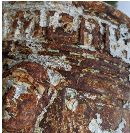
Figure 8. Close-up of lamppost base showing corrosion where paint has worn off. (photo by EverGreene, January 2020)
