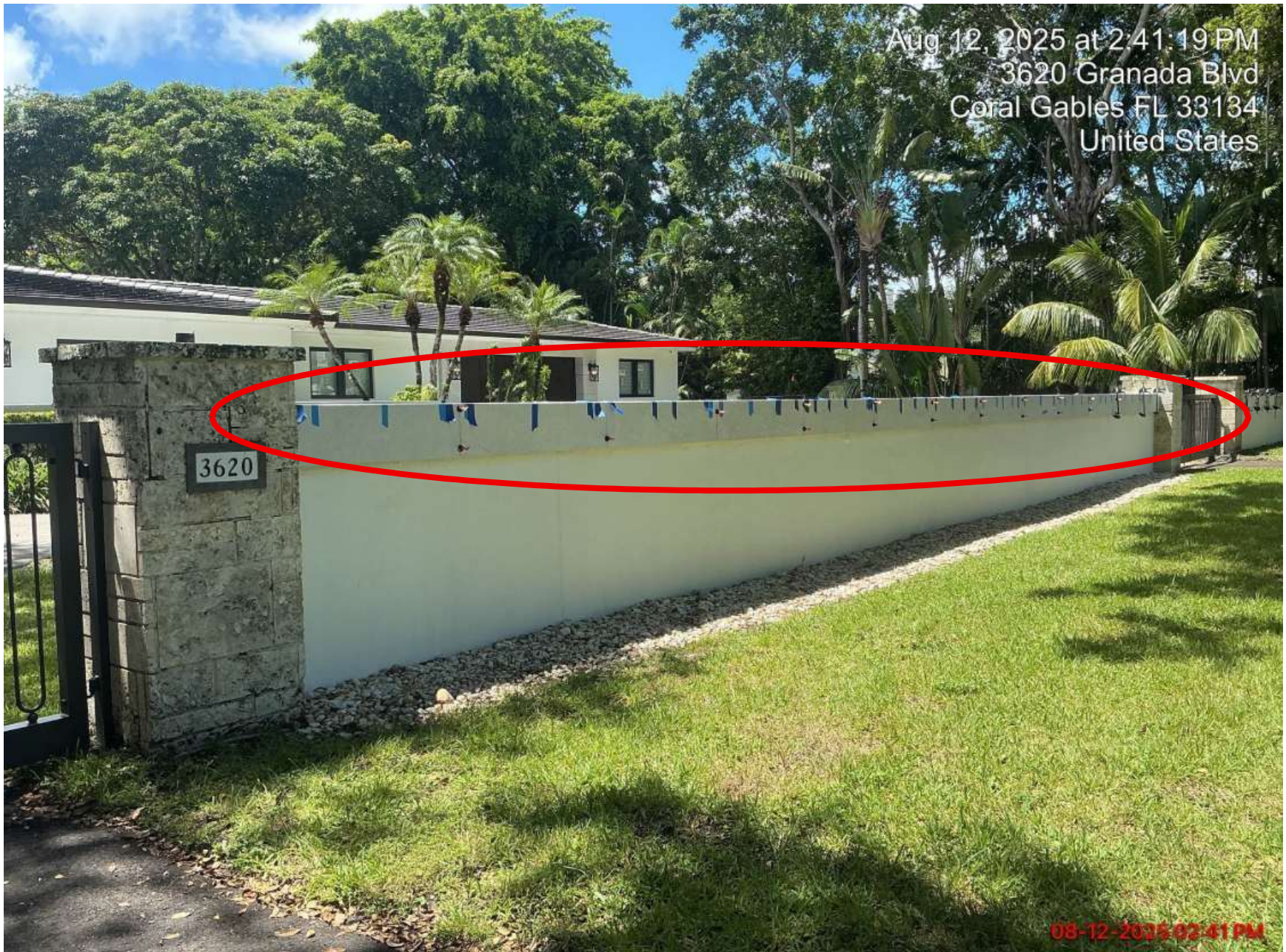
CBS WALL ALTERED WITH TILE CLADDING
