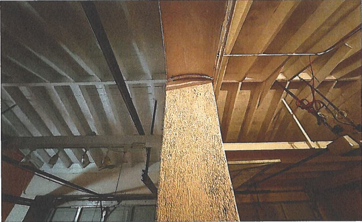
Both garages share center roof joist and roof system. If tried to reverse, most likely entire roof would need to be replaced at extensive cost to client.
