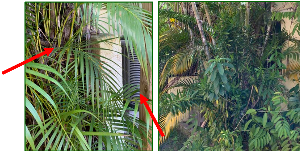
Figures 24: Wing Wall Obscured by Vegetation
