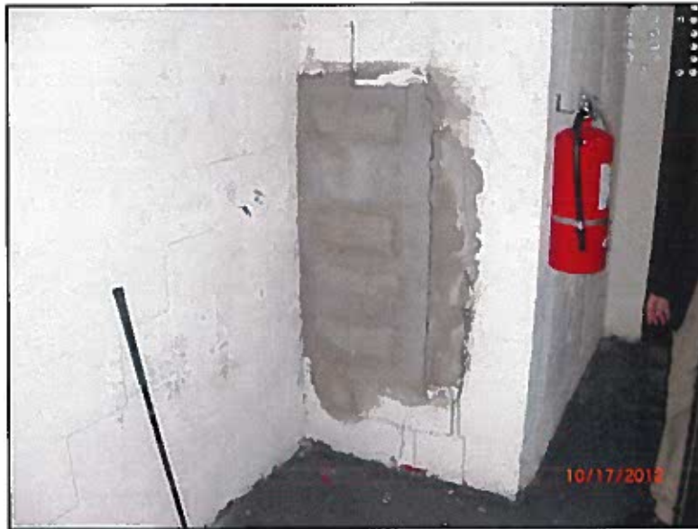
PHOTO # 13: Cracks on block wall at inside of West Elevator Machine Room
