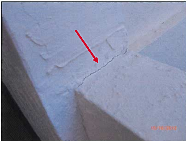
PHOTO # 8: Cracking at connection between balcony wall and bldg. column at Unit #219
