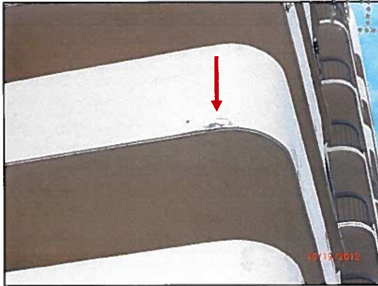
PHOTO # 33: cracking and staining at bottom of fourth floor balcony wall on east
