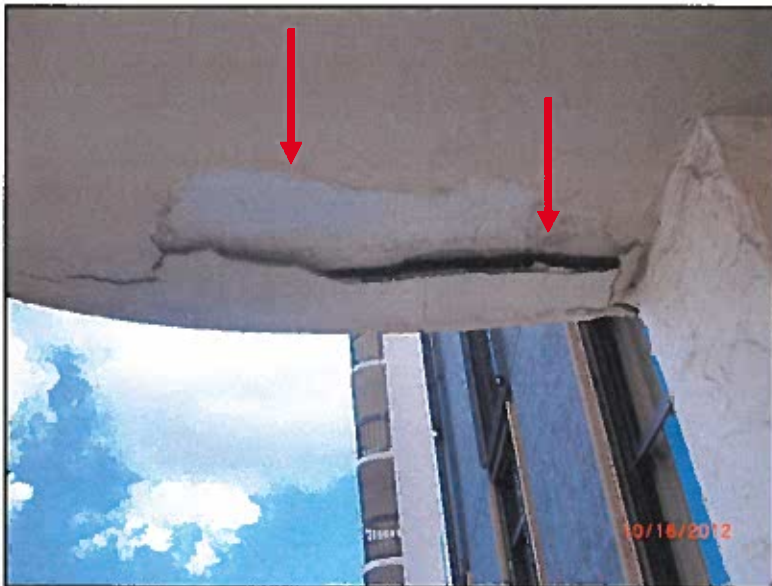
PHOTO # 4: Concrete spalling/exposed steel rebar at balcony ceiling at Unit #219
