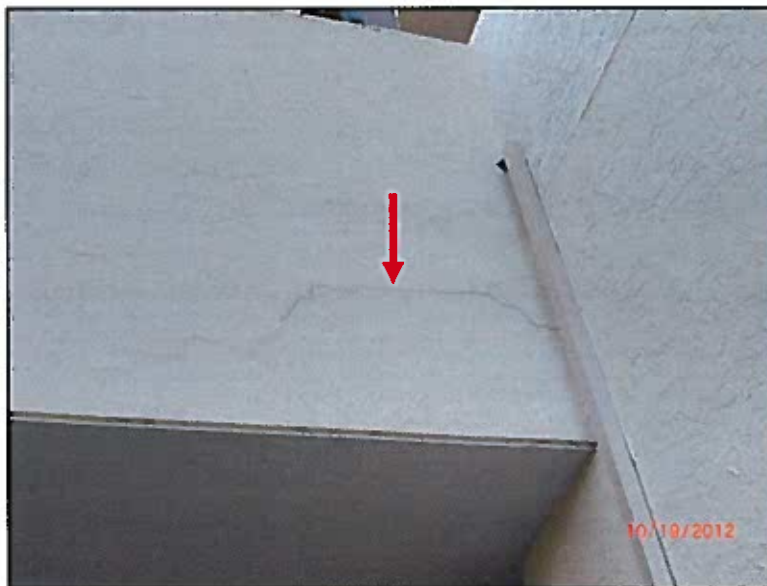
PHOTO # 28: cracking on overhang at West side
