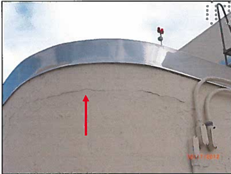
PHOTO # 9: Delaminated/cracking stucco at exterior of Generator Room at roof area
