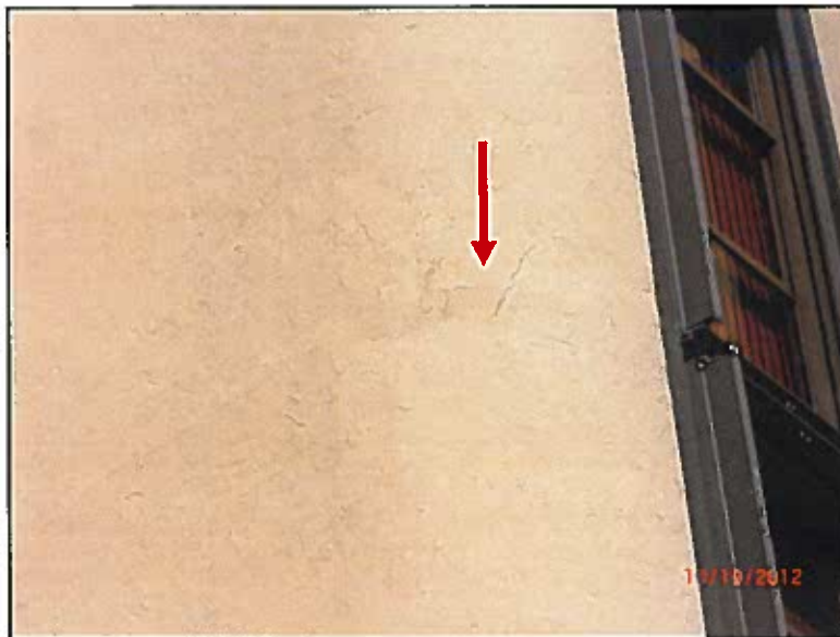
PHOTO # 34: stucco cracking on building wall next to east stairs tower
