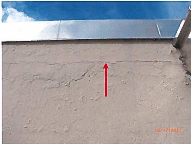
PHOTO # 10: Delaminated/cracking stucco at exterior of east Elevator Machine Room at Roof Area
