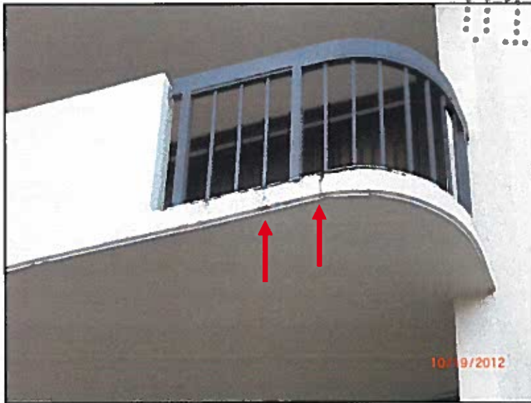
PHOTO # 29: cracking and staining on balcony edge
