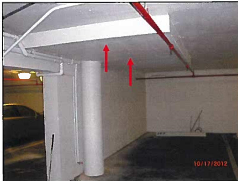
PHOTO # 14: slab cracking at column drop panel next to Parking Space No. 267
