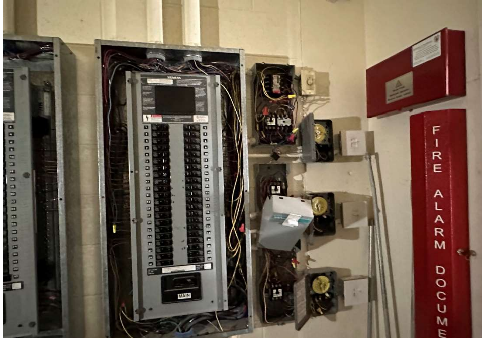
Panel 2LA Opened – Timers Clocks and Relays - 2 nd Floor.
