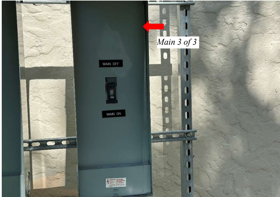
Main 3 of 3 (Labeled 6 of 7) – 400 Amps.
