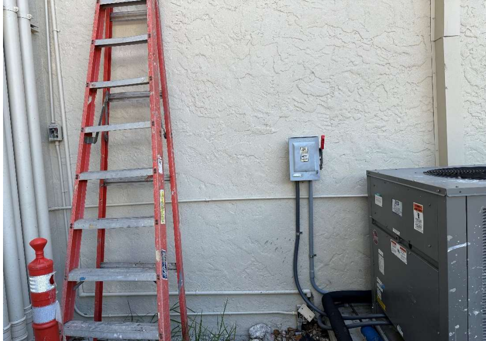
AC Condensing Unit Disconnect
