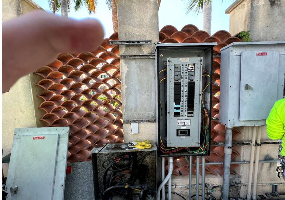
PNL-P.O. – Chiller Area
