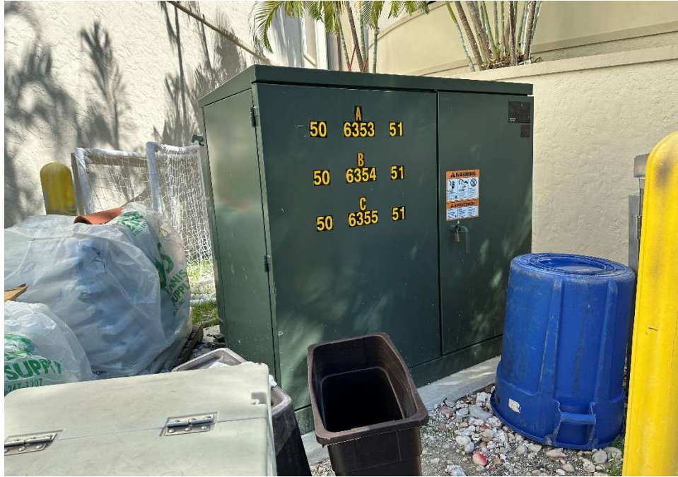
FPL Service – 3 Phase 277/480 Volts, 4 Wire – Pad Mounted Transformer
