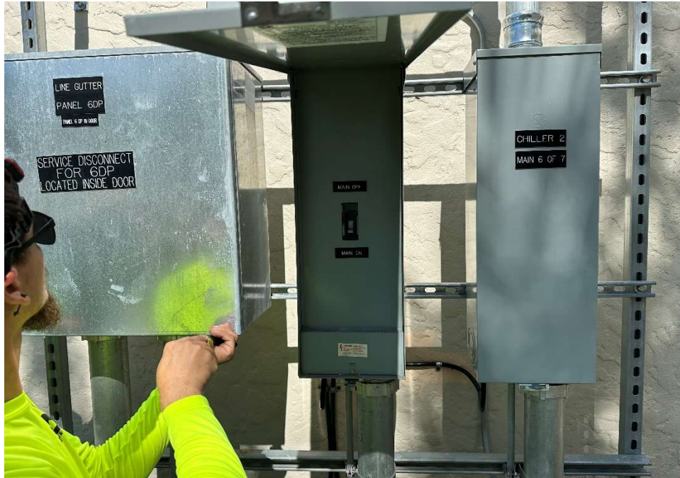
Exterior Location Service Entrance 2 – Mains 1 -3 – 3 Phase, 277/480 Volts
