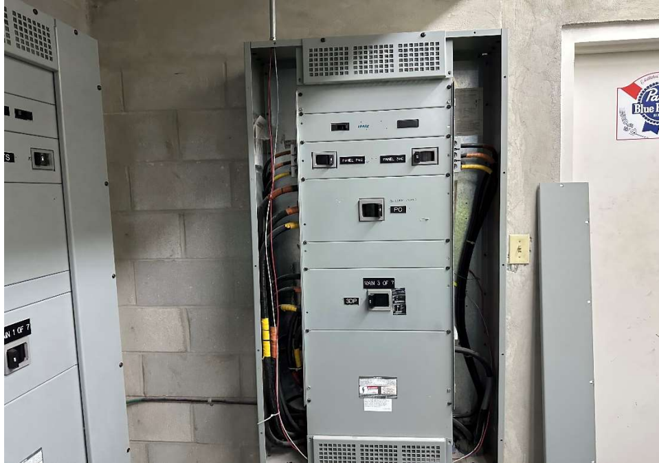
Main 3 of 4 (Labeled 3 of 7) – 600 Amps.
