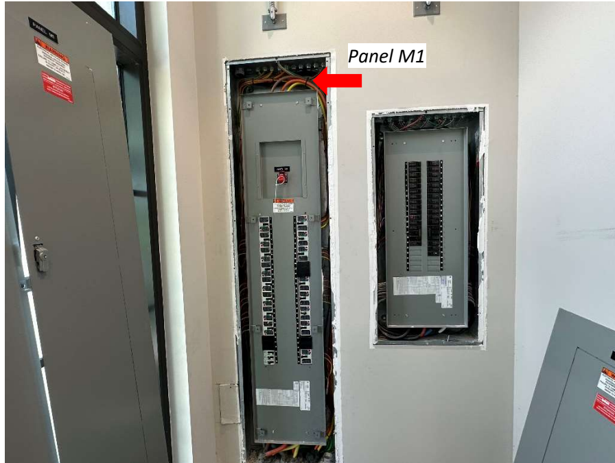
Panel M1 Opened – 1 st Floor.
