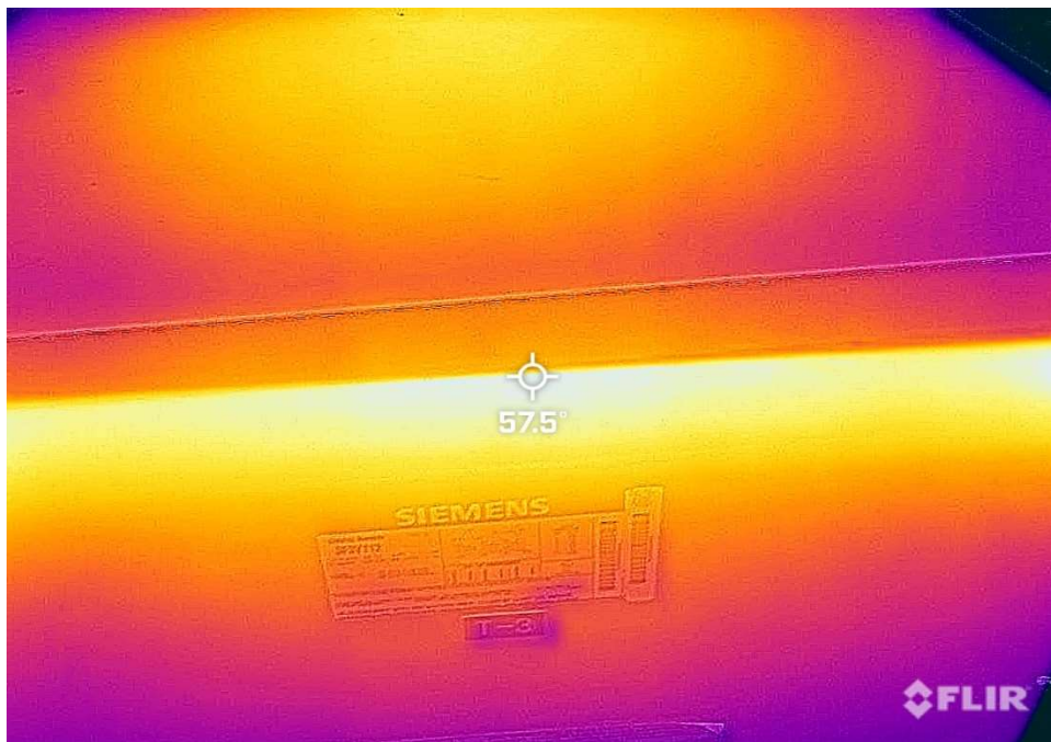
Item 11 : Transformer T-3 at 57.5 Degrees Celsius
