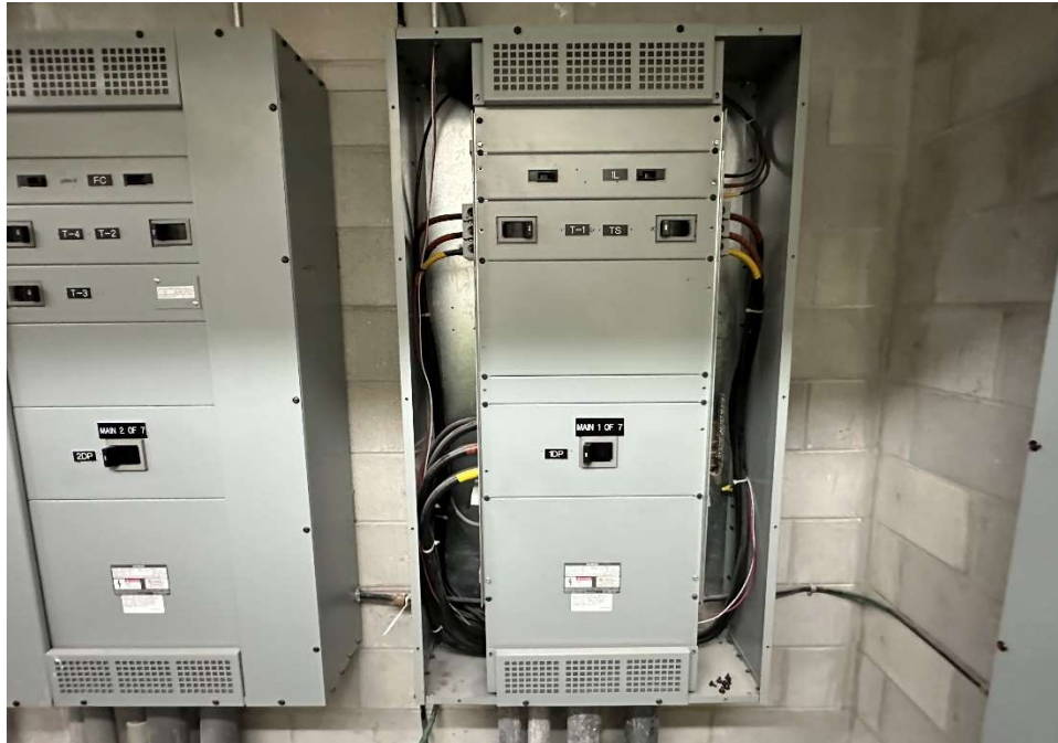
Main 1 of 4 (Labeled 1 of 7) – 600 Amps.
