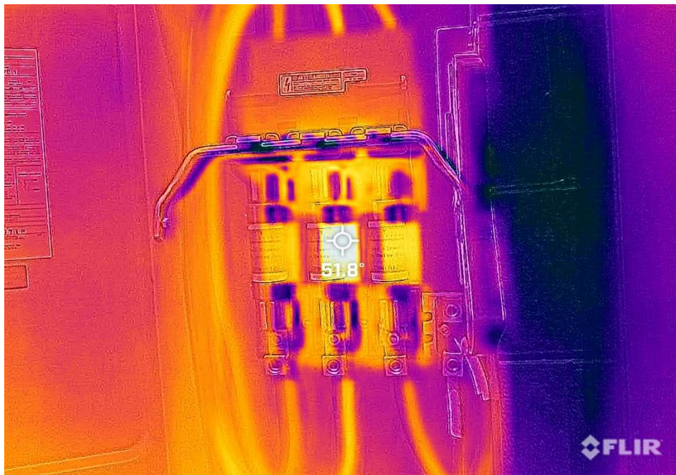
Item 8: Transformer Disconnect at 51.8 Degrees Celsius (delta 21.8C)
