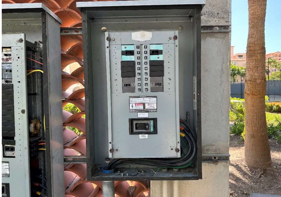
PNL-1AC – Chiller Area
