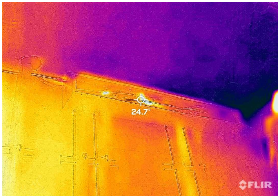
Item 70: Gutter at 24.7 Degrees Celsius (delta 1.7C)
