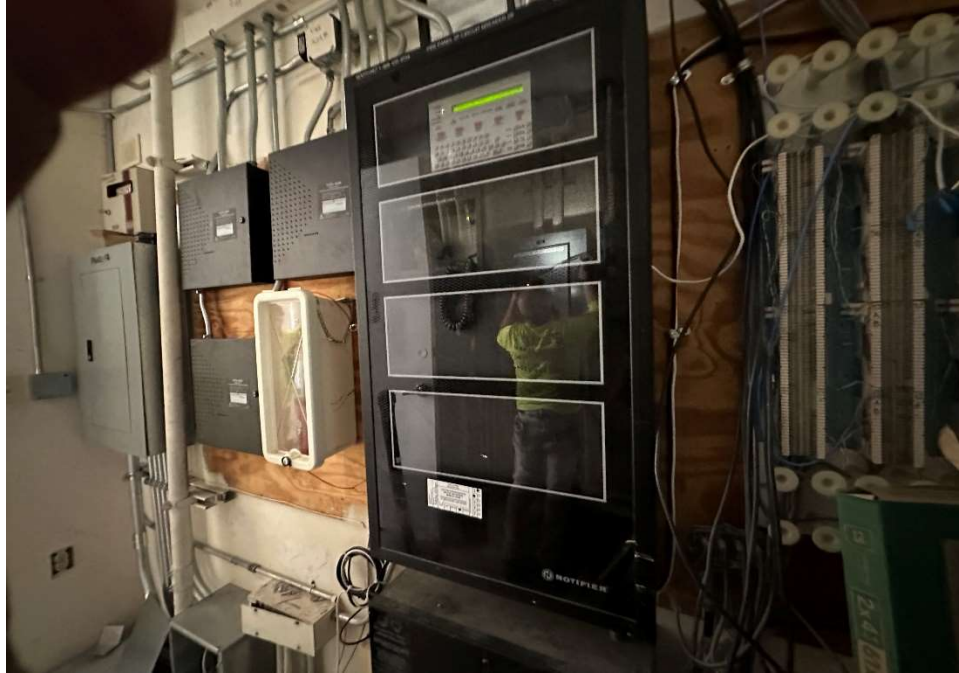
Fire Alarm Control Panel (FACP) – 3 rd Floor
