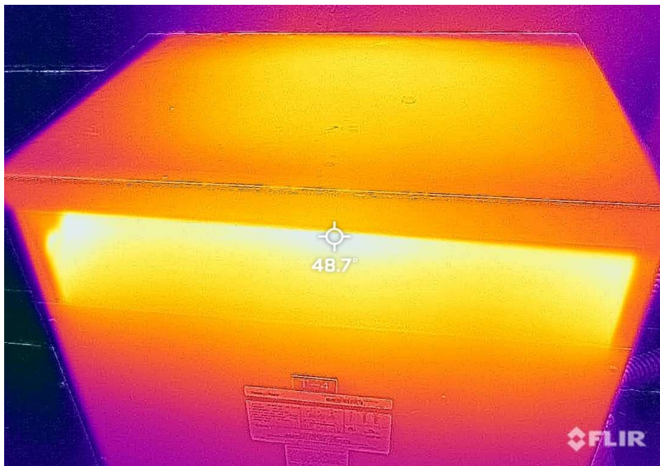
Item 12 : Transformer T-4 at 48.7 Degrees Celsius
