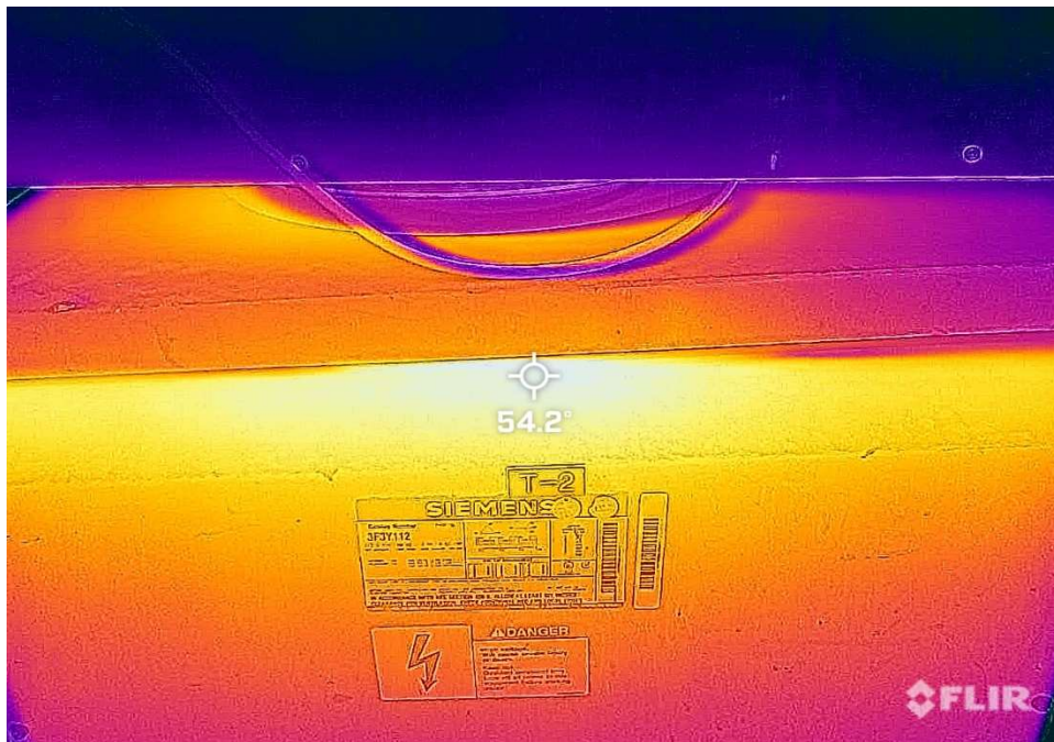
Item 26: Transformer T-2 at 54.2 Degrees Celsius
