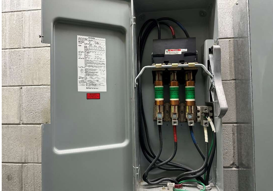
Transformer Disconnect Opened
