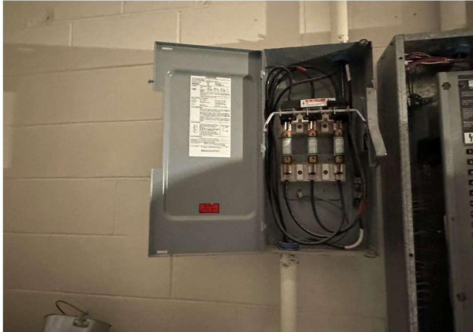
Transformer T-1 Disconnect
