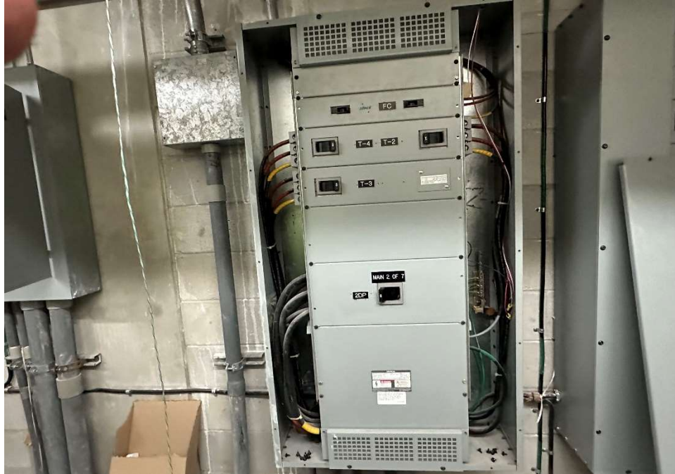
Main 2 of 4 (Labeled 2 of 7) – 600 Amps.
