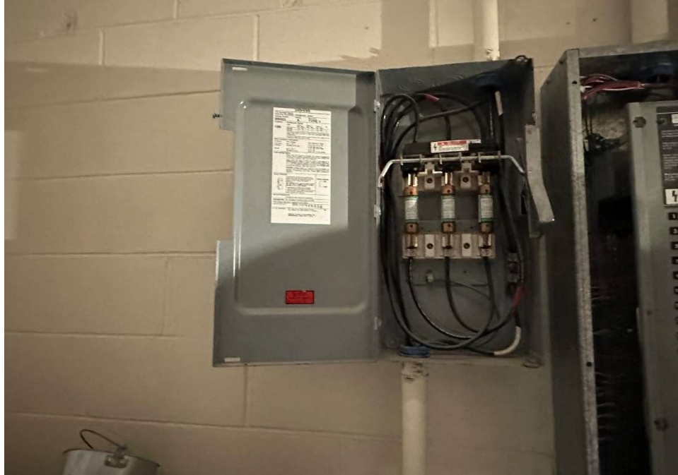
Transformer PNL 3L Disconnect.
