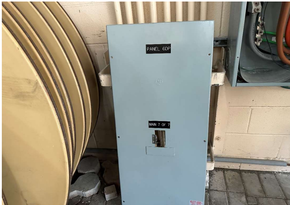
Interior Location of Service Main Panel DP – Service Entrance 2
