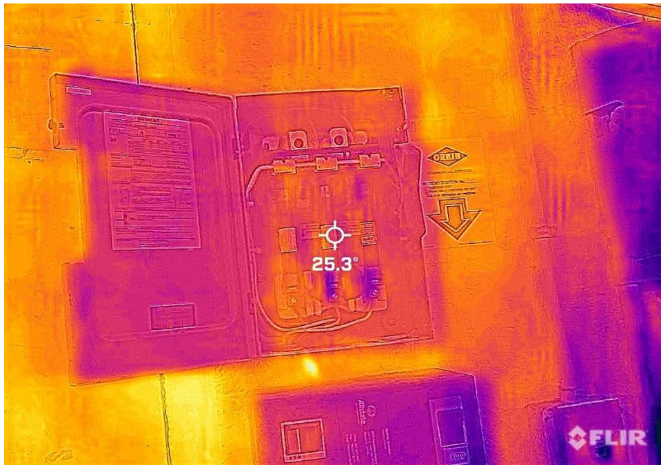
Item 51: Disconnect 2 at 25.3 Degrees Celsius (delta 2.3C)
