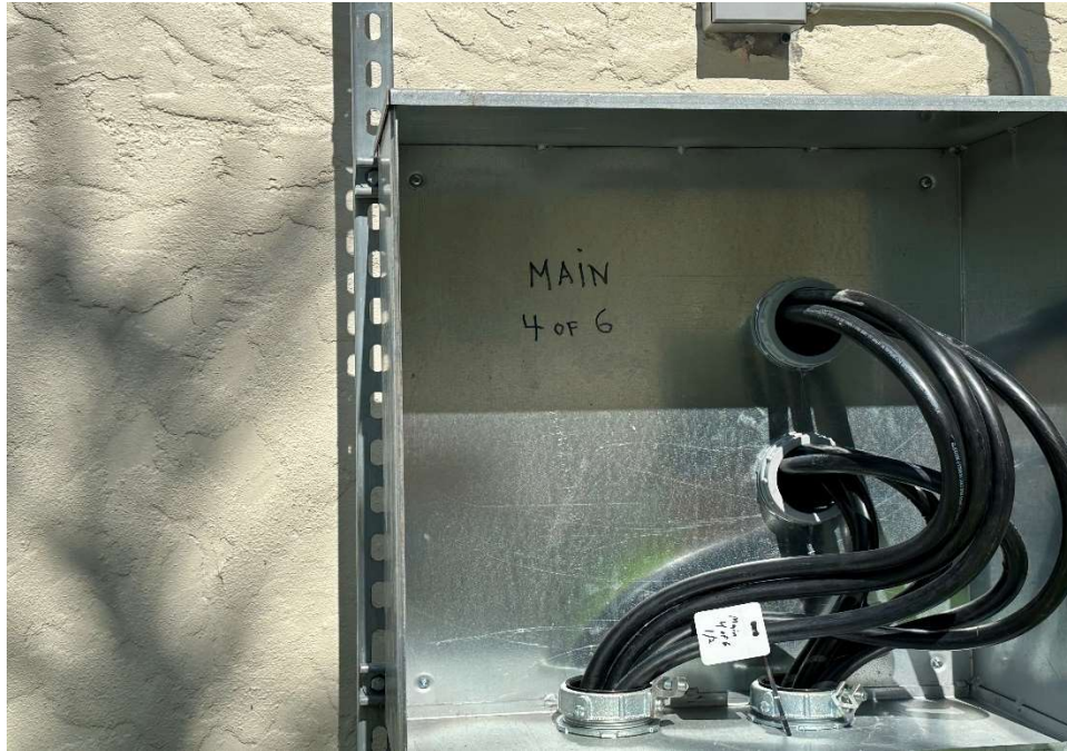
Pull Box for Main 1 of 3 (labeled 4 of 6) – Panel DP Located on Interior Wall
