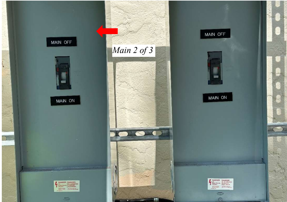
Main 2 of 3 (Labeled 5 of 7) – 400 Amps.
