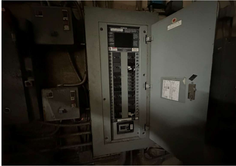
Panel 3AC – Located in Kitchen Mezzanine (above 2 nd Floor)
