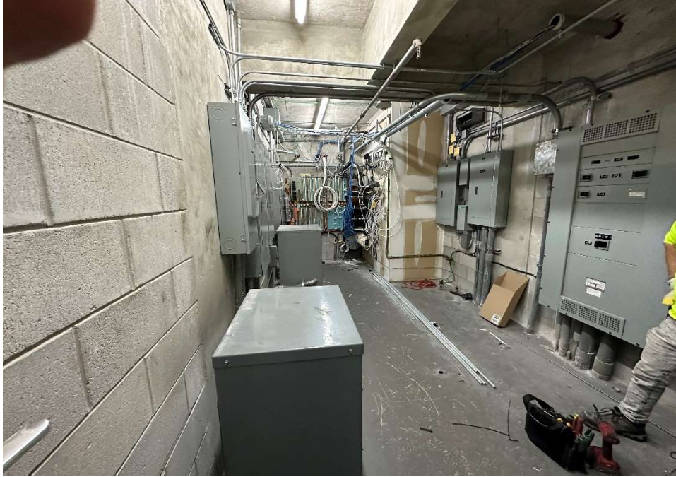
Main Electrical Room Layout from Entrance Door -
