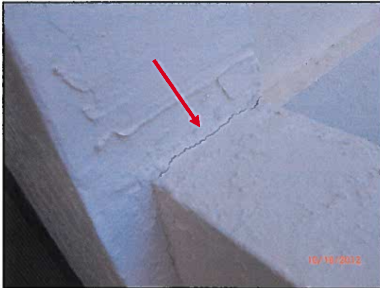
PHOTO # 8: Cracking at connection between balcony wall and bldg. column at Unit #219
