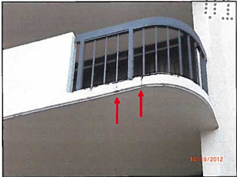
PHOTO # 29: cracking and staining on balcony edge
