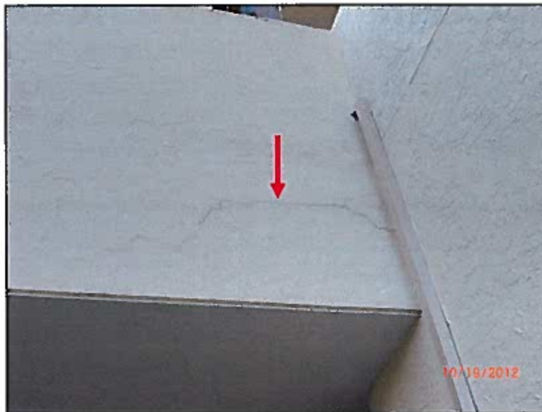
PHOTO # 28: cracking on overhang at West side
