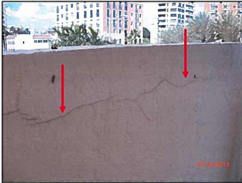
PHOTO # 3: Horizontal cracking on balcony block wall concrete cap at Unit #219
