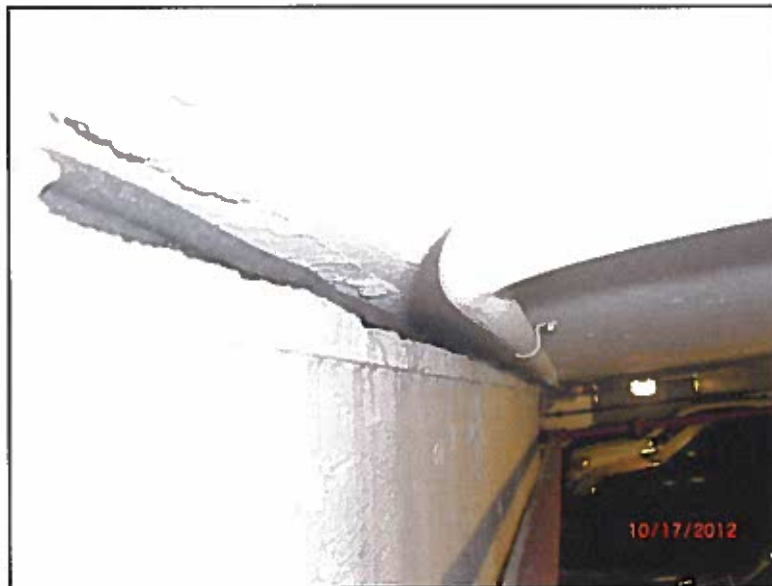
PHOTO # 22: trench drain drop ceiling opening between Parking Spaces 314 & 327
