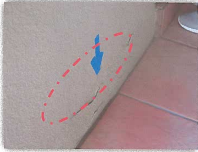
Repair spalling concrete on interior hallway walls at/near units 204, 205 & 401.
