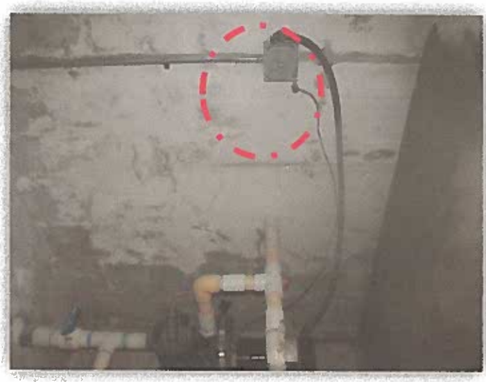
Replace bonding at pool motor with proper wiring and method(s).
