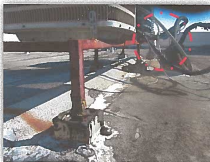
Replace deteriorated service wiring conduits at all rooftop A/C condensing units.
