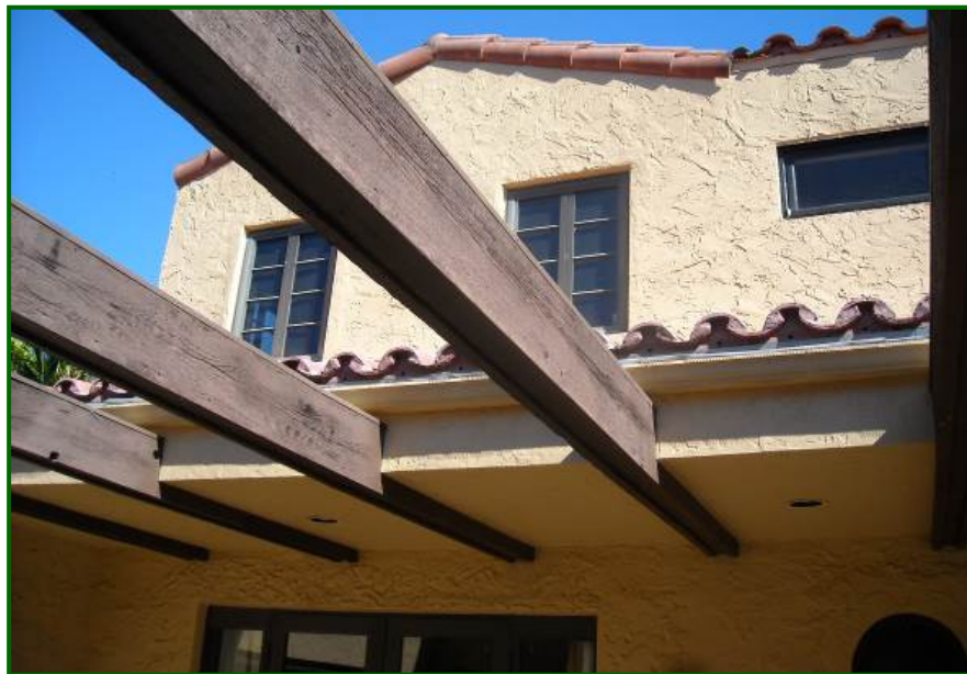
Figure 20: South Façade, Roof Ridge and Second Story Wall Repair Permit #33127, 1989 [top] Current Photo, 2018 [bottom]
