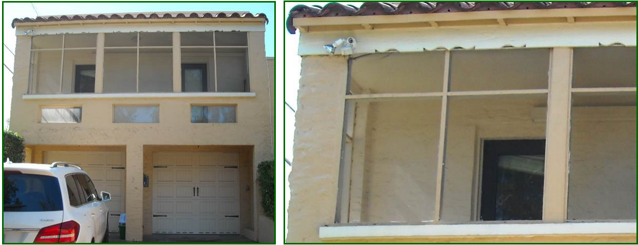
Figure 15: Side (North) Façade, Eastern section, 2018 Two-story Garage and Apartment Loggia Loggia northeast corner detail
