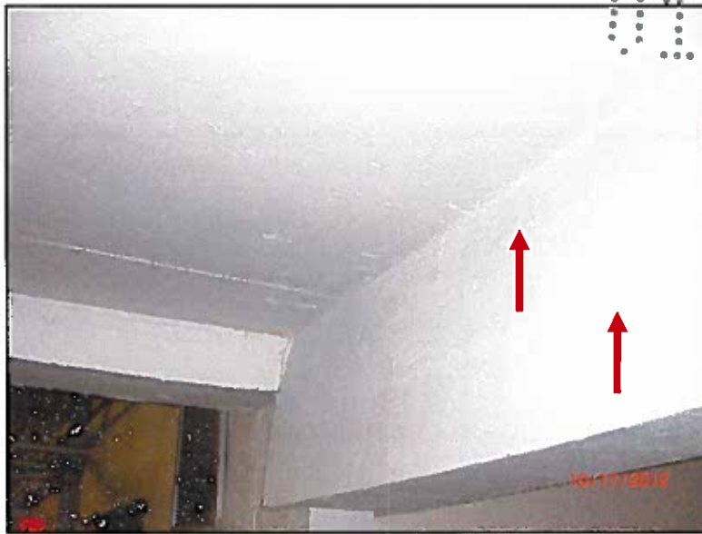
PHOTO # 17: slab cracking and beam cracks next to Parking Space 210
