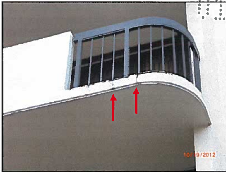
PHOTO # 29: cracking and staining on balcony edge
