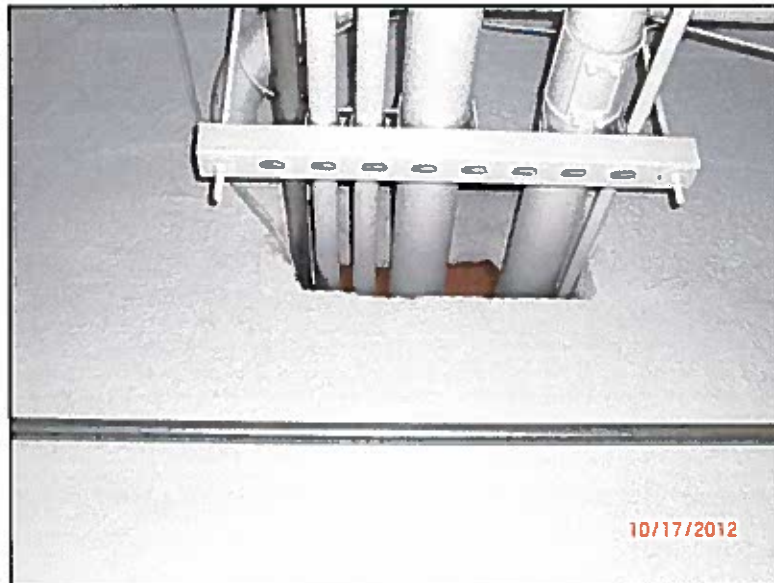
PHOTO # 16: Unsealed wall, pipe penetration at Fire rated assembly (2hr fire rated assembly) Paint Storage Room
