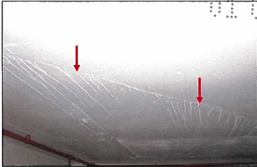
PHOTO # 23: cracking and water intrusion at underside of ramp in front of Parking Space 61
