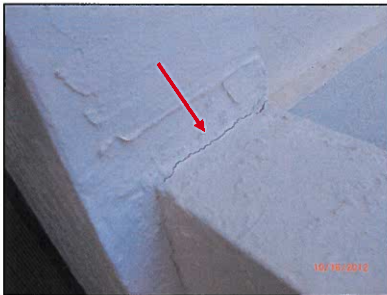
PHOTO # 8: Cracking at connection between balcony wall and bldg. column at Unit #219
