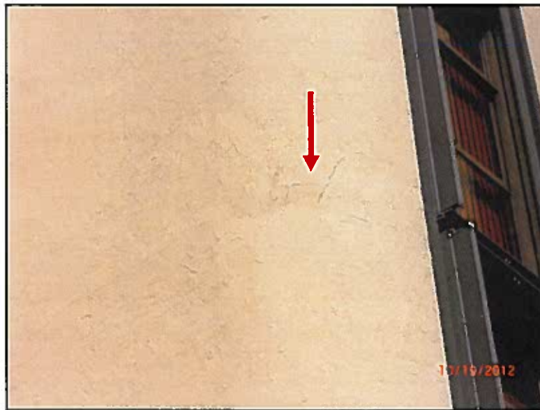
PHOTO # 34: stucco cracking on building wall next to east stairs tower
