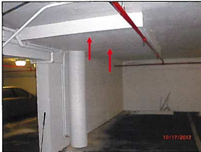
PHOTO # 14: slab cracking at column drop panel next to Parking Space No. 267
