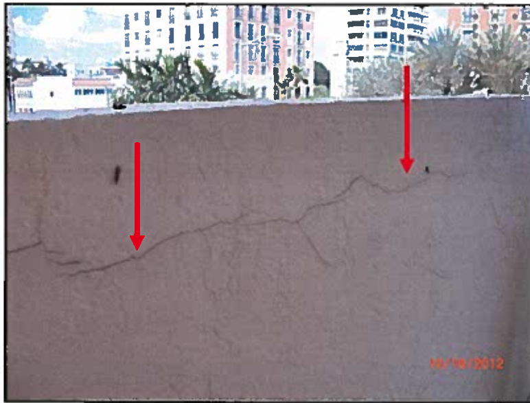
PHOTO # 3: Horizontal cracking on balcony block wall concrete cap at Unit #219
