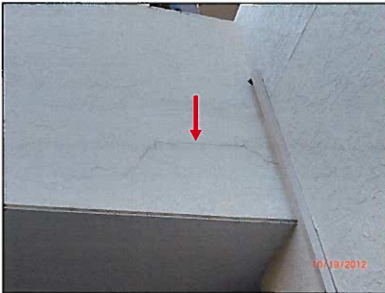
PHOTO # 28: cracking on overhang at West side
