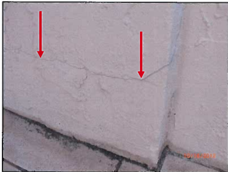
PHOTO # 2: Horizontal cracking/delaminated stucco at balcony wall Unit #219
