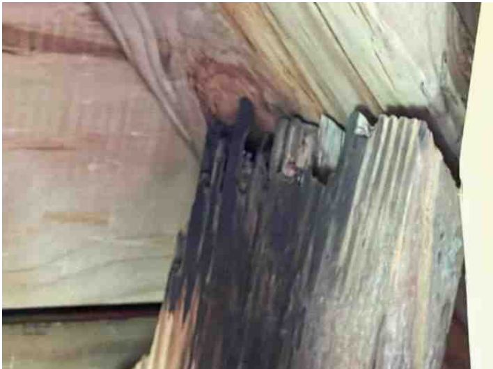
Wood Rot in Trusses
