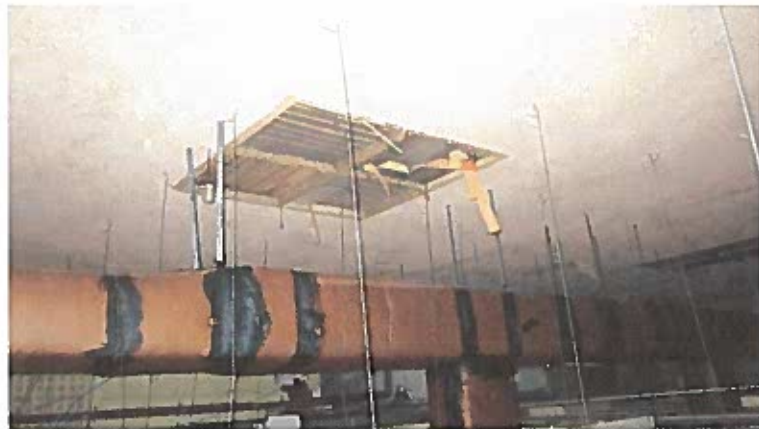
Photograph #6 of underside of concrete slab over main meeting hall first floor roof south wall.
