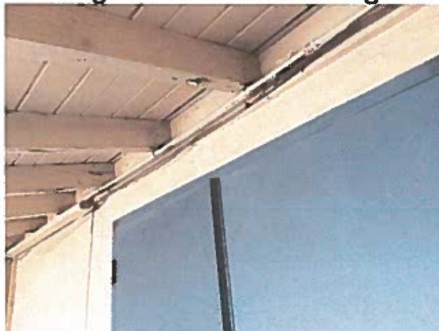
Photograph #5 of previous termite damage at Parking Courtyard Shelter roof joist and deck.
