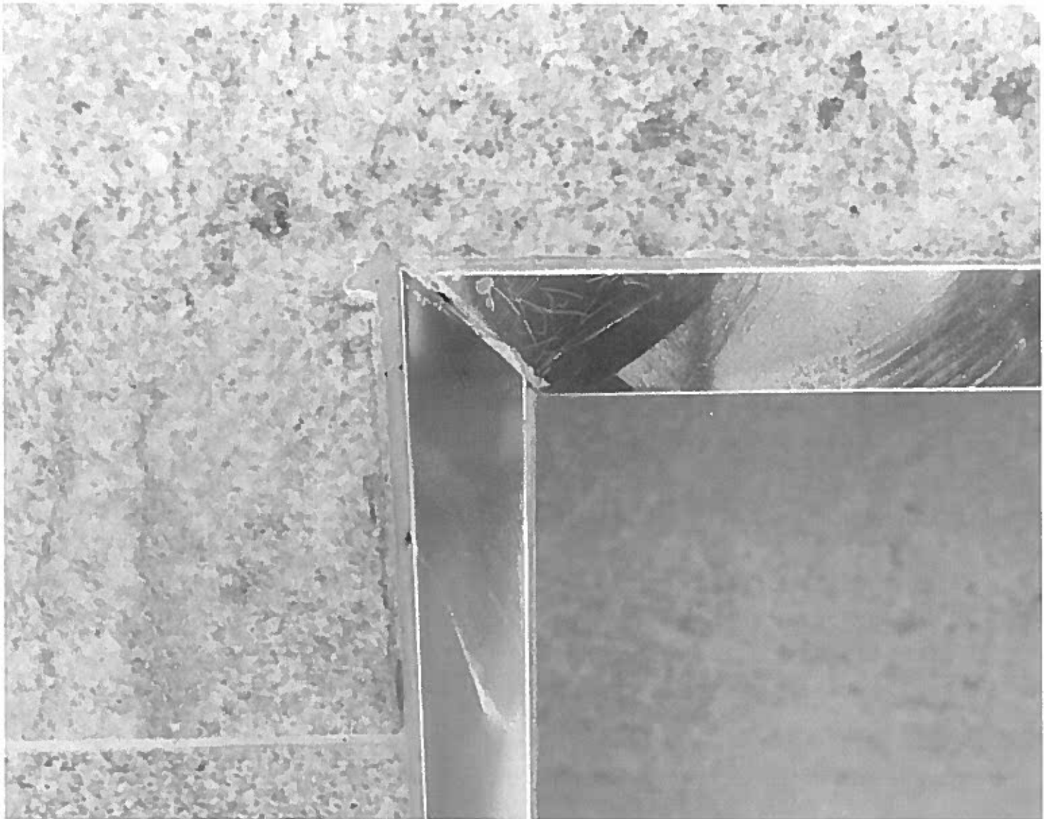
Poorly cut mitered joint of stainless steel insert. Most mitered joints are not flush and many have sharp edges.
