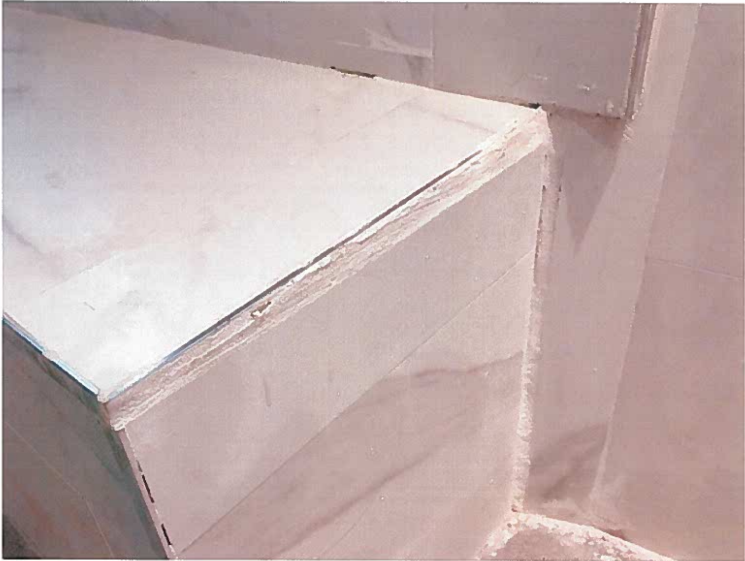
Master bathroom shower bench. Note poor workmanship of tiles and stainless steel insert.
