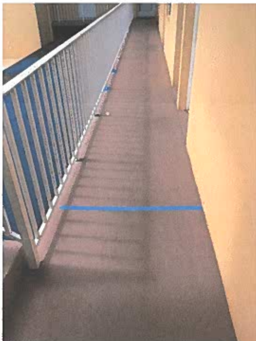
4 th Floor Catwalk Spalls
