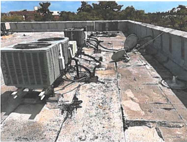
AC Compressors at Roof Deck
