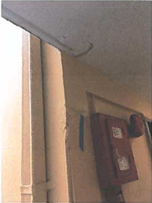
3 rd Floor Overhead Spall
