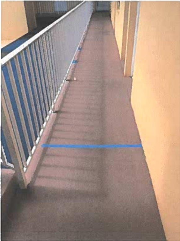
3 rd Floor Catwalk Horizontal Spalls
