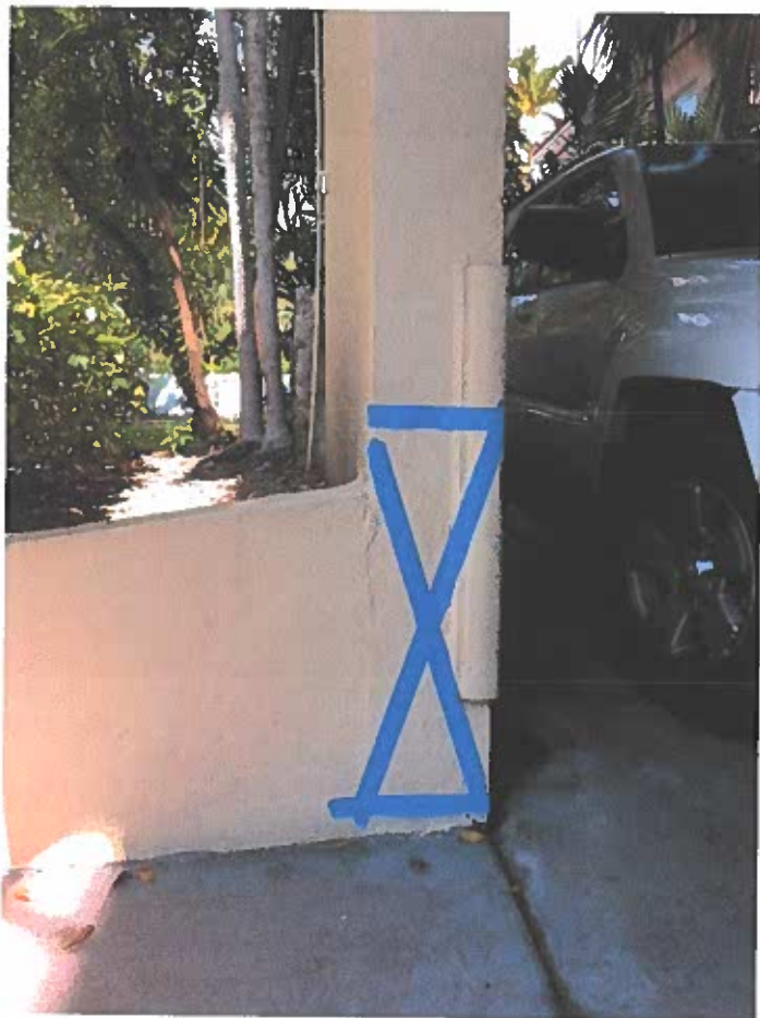
Column Spall at Garage East Entrance
