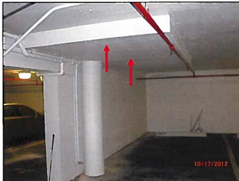
PHOTO # 14: slab cracking at column drop panel next to Parking Space No. 267
