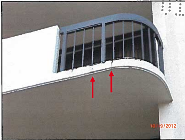
PHOTO # 29: cracking and staining on balcony edge
