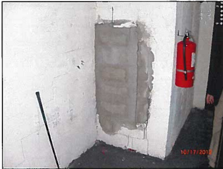
PHOTO # 13: Cracks on block wall at inside of West Elevator Machine Room
