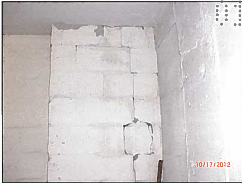
PHOTO # 11: Step cracking at corners of east side Elevator Machine Room
