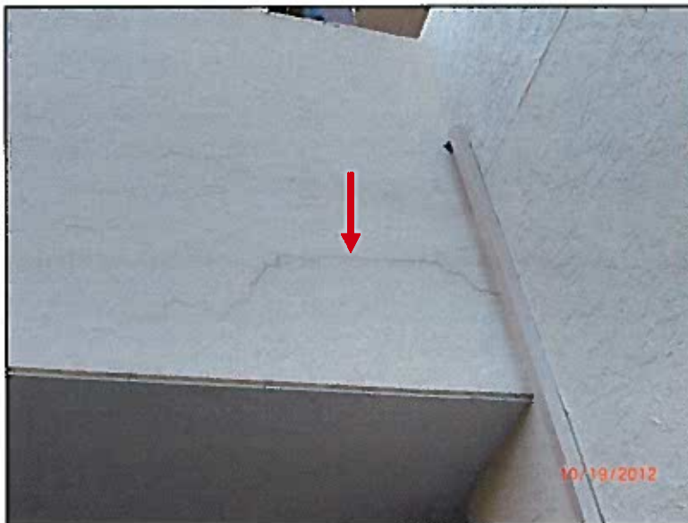
PHOTO # 28: cracking on overhang at West side
