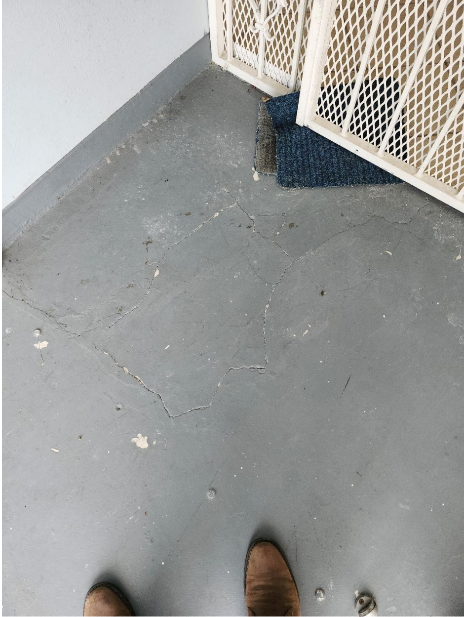
Cracking in the landing of the northern stairs.
