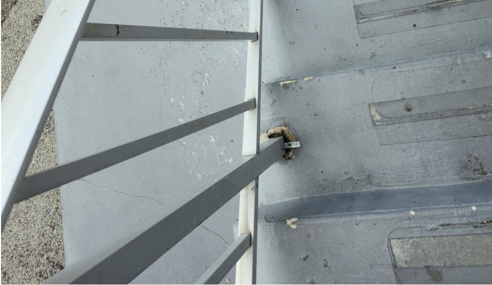
Handrail attachment is weak (the handrails wiggle).
