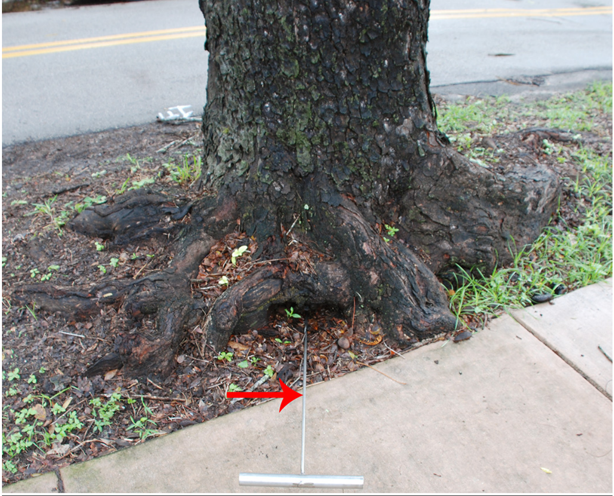
Photo 9 above is the steel spike that I was able to insert into a cavity approximately 8 inches on the west side of the trunk/root collar.
