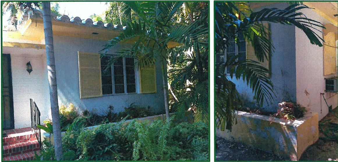
Figure 10: 229 Ridgewood Road, Front (South) Façade, May 2016 eastern bay (left), detail of extended planter (right)
