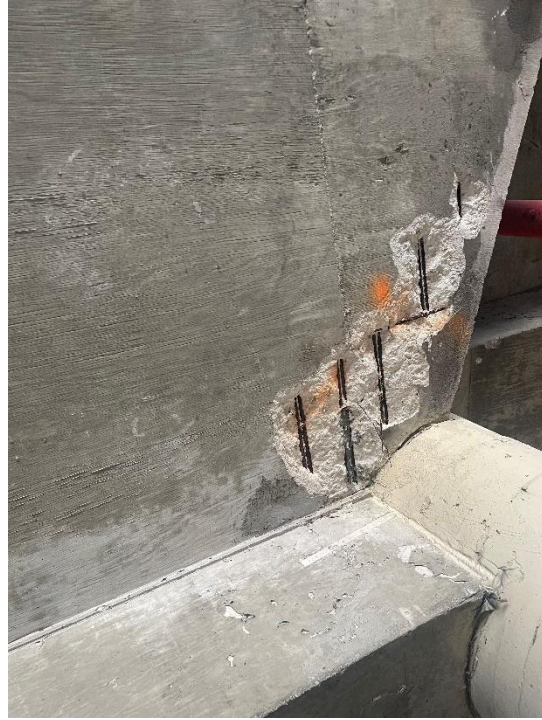
Photo 21: Overhead slab ceiling spalling with exposed reinforcing steel.
