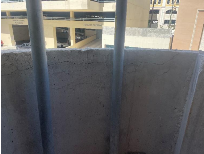
Photo 13: Spalling at the top of the guard rail wall.
