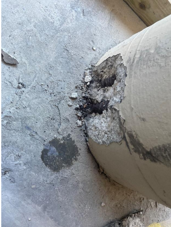
Photo 1: Spalled structural column at its base.
