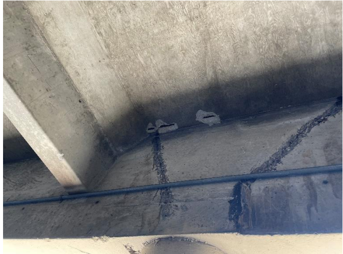
Photo 6: Shear cracks in beams on each side of the supporting column.
