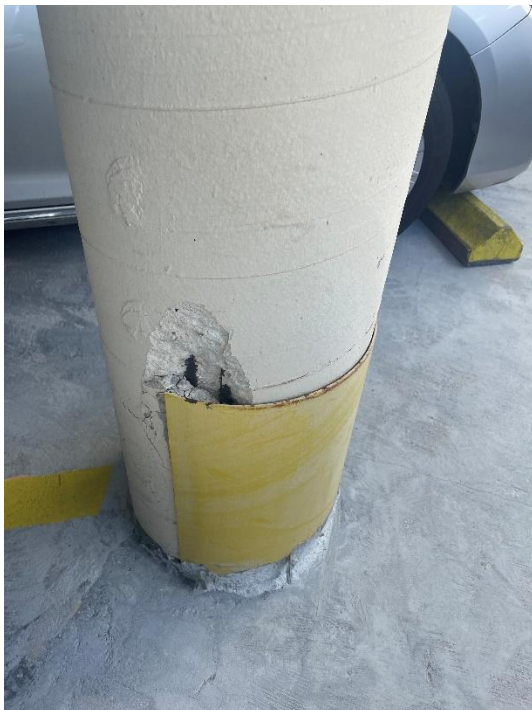
Photo 3: Column spall at steel guard.
