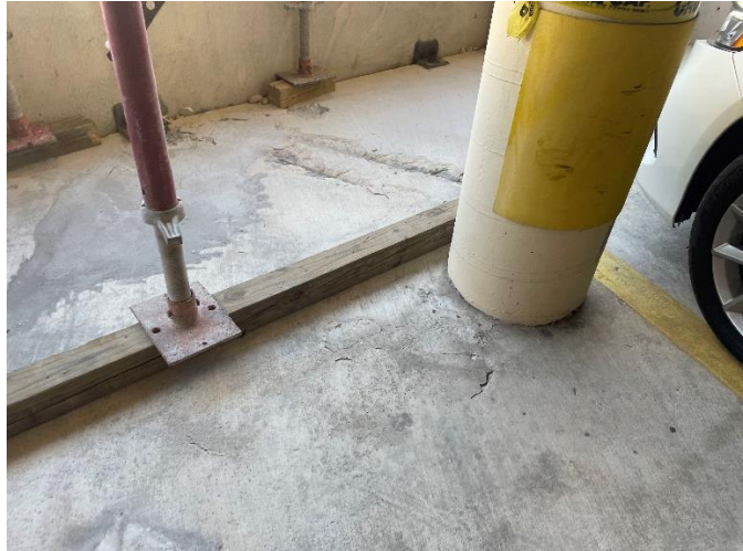
Photo 10: Spalling deck surface at the column.
