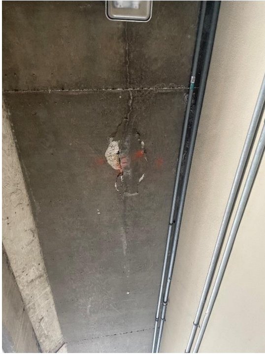
Photo 20: Overhead slab ceiling spalling.
