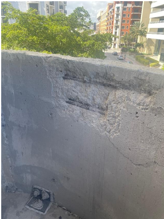
Photo 15: Spalled concrete at the top of a guard rail wall.
