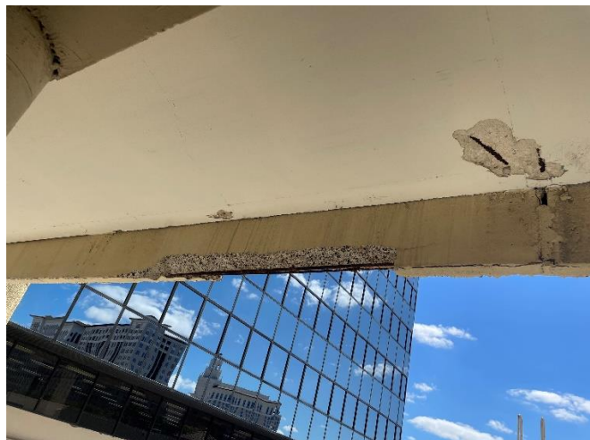
Photo 8: Spalled perimeter beam bottom.
