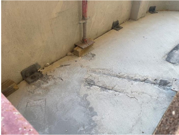
Photo 17: Spalling of the deck surface adjacent to wall/slab connections.
