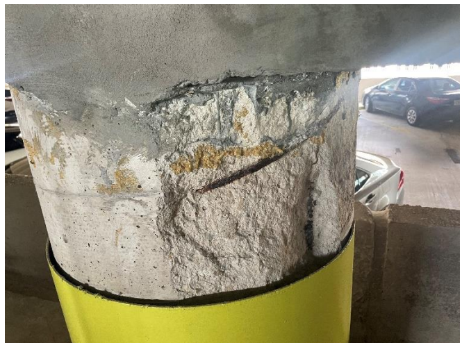
Photo 4: Column spall at column/beam joint.
