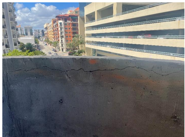
Photo 16: Spalling at the top of the guard rail wall.
