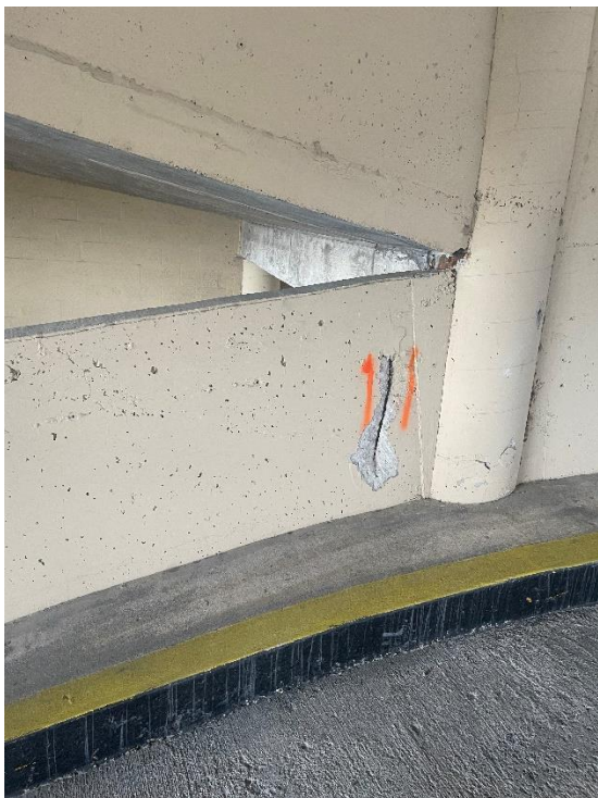
Photo 24: Spalled concrete at a ramp guard rail wall.
