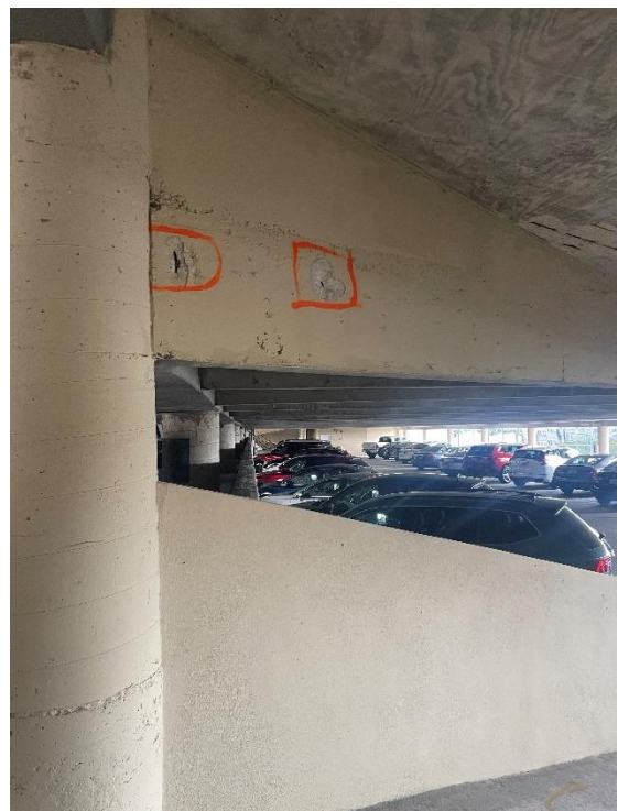
Photo 24: Spalled concrete at a ramp support beam.
