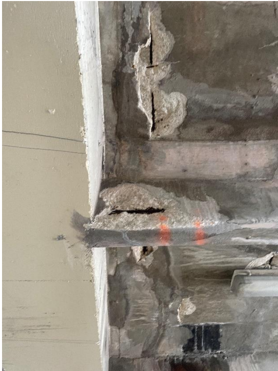
Photo 5: Overhead slab ceiling spall and precast joist end spall.
