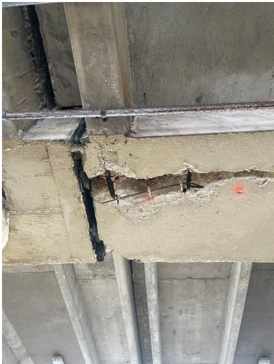
Photo 7: Spalling of beam bottom at what appears to be a support corbel.
