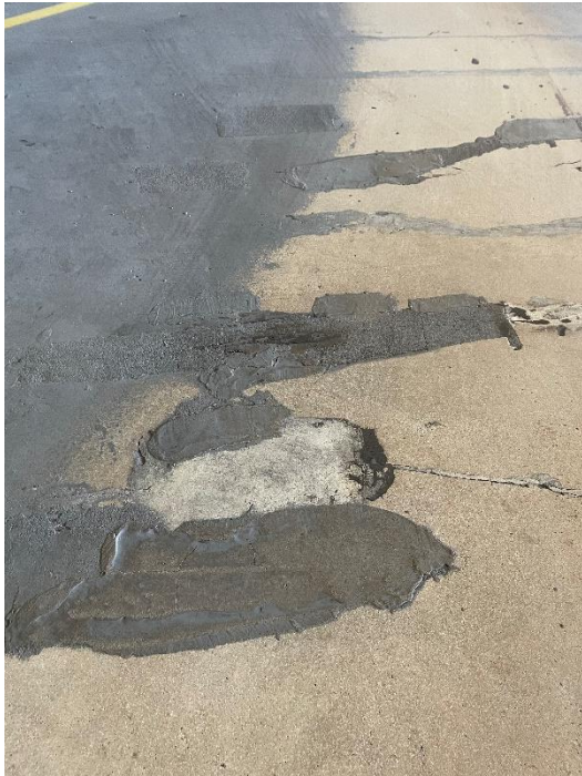
Photo 9: Previously repaired deck spalls and cracks.
