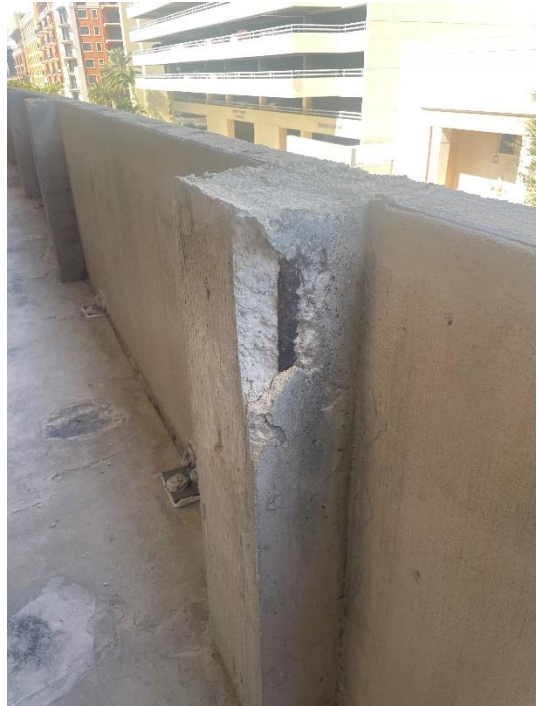
Photo 14: Spalling of the column at the guard rail wall.
