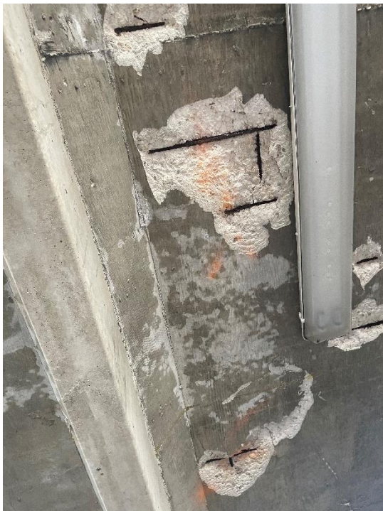
Photo 22: Overhead slab ceiling spalling with exposed reinforcing steel.
