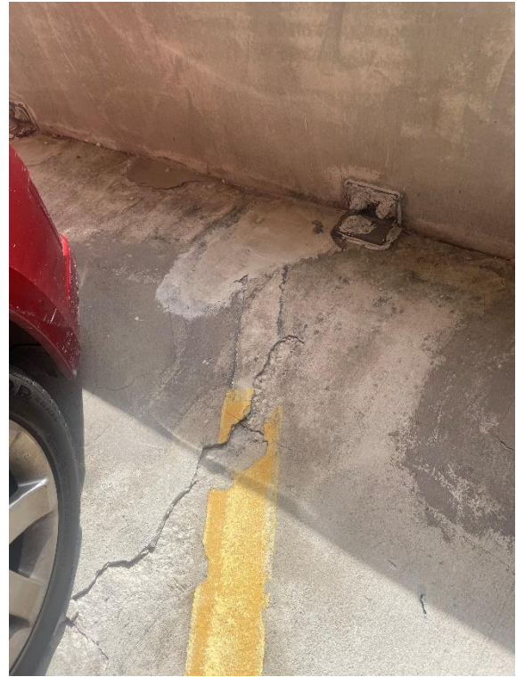
Photo 18: Spalling of the deck surface adjacent to a wall/slab connection.
