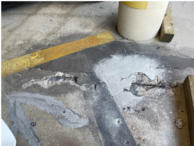
Photo 11: Spalling of deck surface at previous repair.
