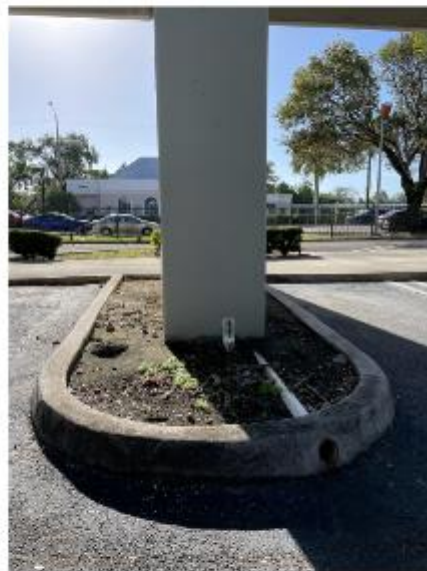
Figure 15 Lack of landscaping in parking curb.
