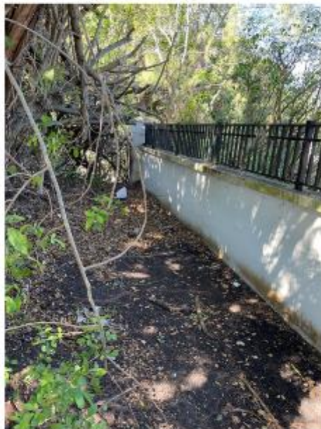
Figure 31 Debris left in embankment behind Blue Road Bridge (874302).
