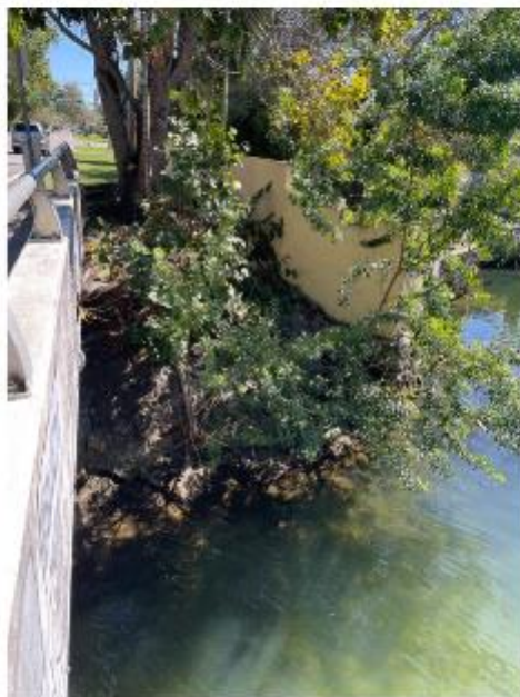
Figure 27 Overgrown landscaping in embankment of Blue Road Bridge (874302).
