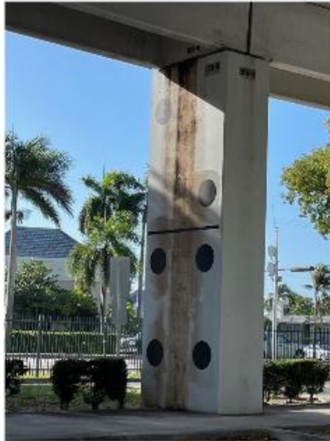
Figure 12 Visible stains on pillars need to be pressure washed.
