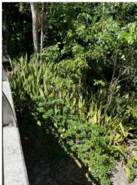
Figure 29 Overgrown landscaping in embankment of Blue Road Bridge (874302).
