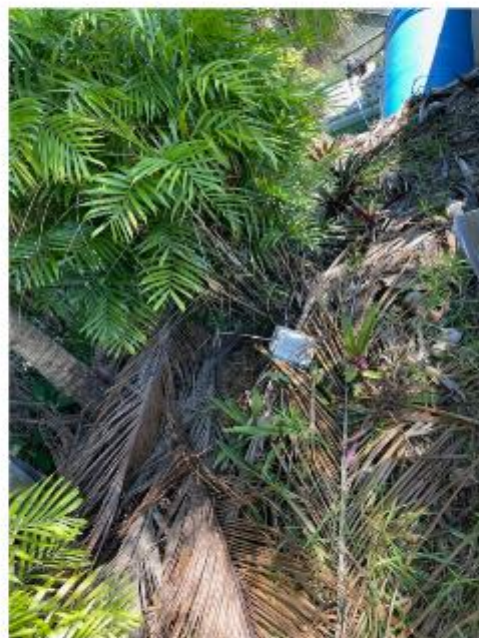
Figure 33 Overgrown and unkept landscaping in embankment of Blue Road Bridge (874302).
