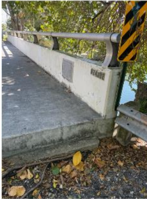
Figure 28 Unfinished sidewalk on Blue Road Bridge (874302).
