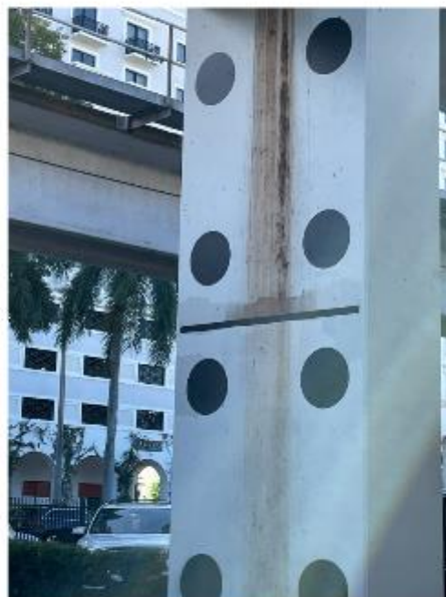
Figure 13 Visible stains on pillars need to be pressure washed.
