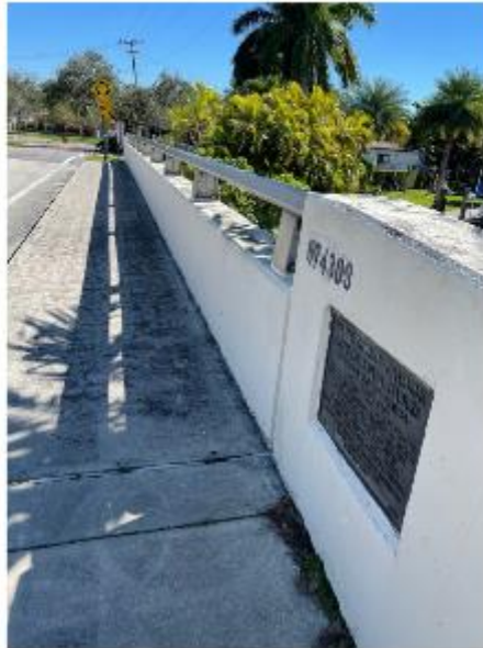
Figure 32 Trash along the embankment of Blue Road Bridge (874303).
