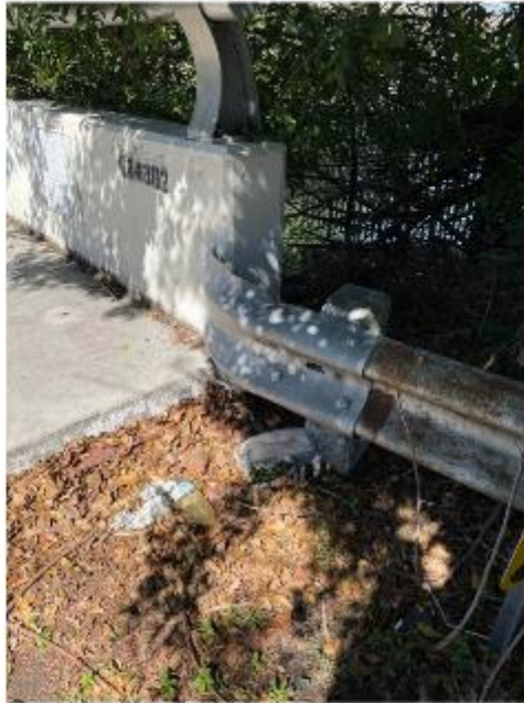
Figure 26 Trash along the embankment of Blue Road Bridge (874302).
