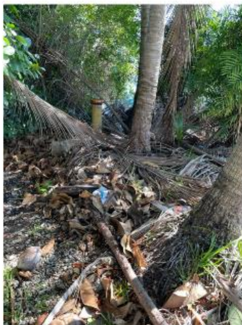
Figure 35 Overgrown and unkept landscaping in embankment of Blue Road Bridge (874302).
