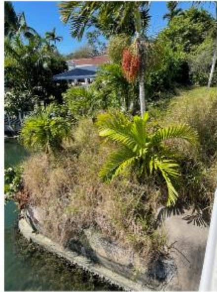
Figure 34 Overgrown landscaping in embankment of Blue Road Bridge (874303).
