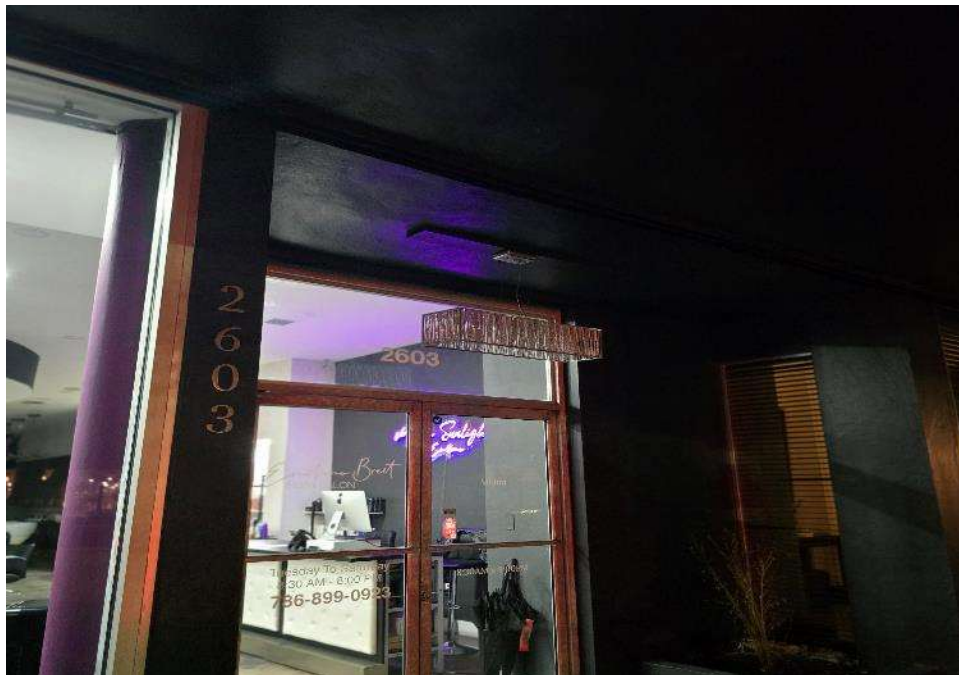
19.2 Bldg. egress lighting (space 2603) - REPAIR LIGHT
