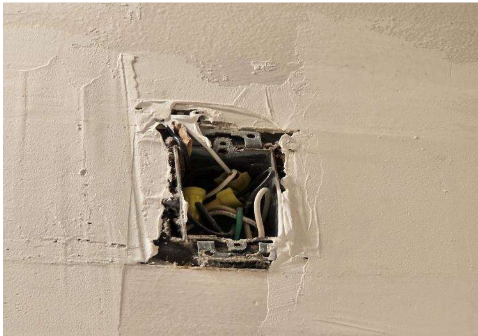
12.2 General conduit/raceways - PROVIDE COVER (KITCHEN SPACE 2603)
