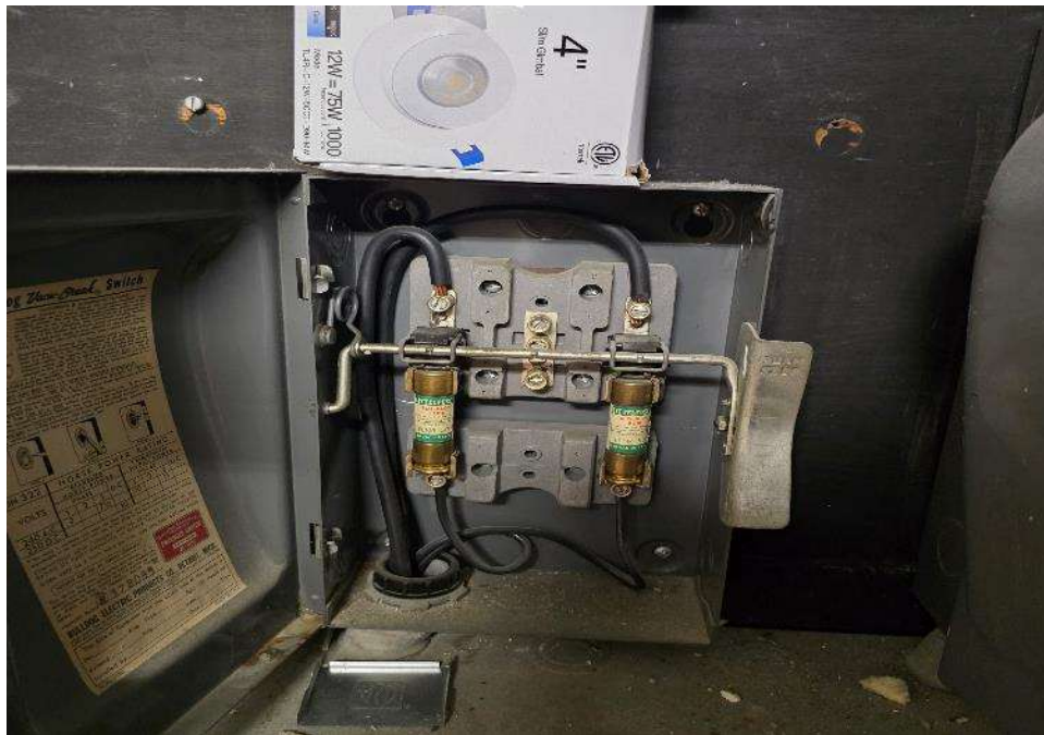
27.2 A C Disconnect switch
