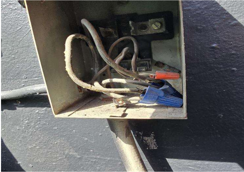
27.5 A C Disconnect switch - REPLACE & PROVIDE GROUND WIRE
