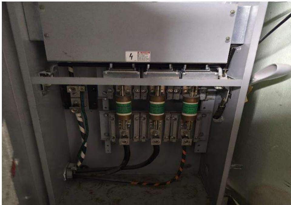
3.3 Space 2603 Main Disconnect 400A
