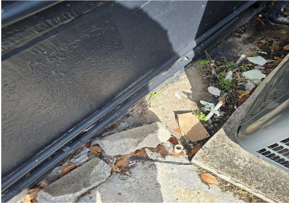
9.2 Grounding of service - REPAIR REQUIRED
