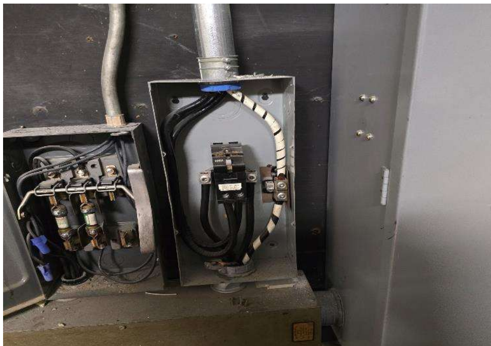
3.5 Space 2603 Panel B Main Disconnect 200A
