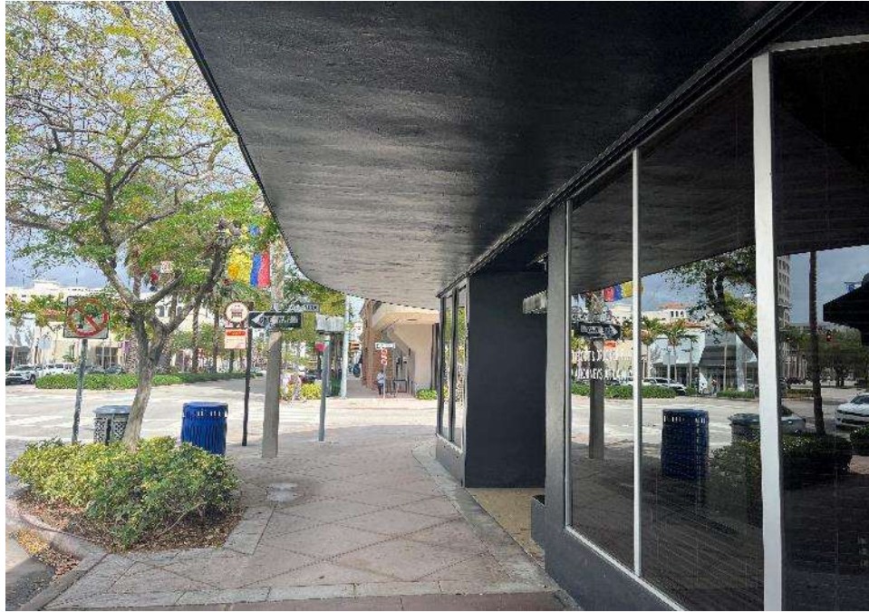
Aluminum-framed storefront along the north and west exterior walls of the building
