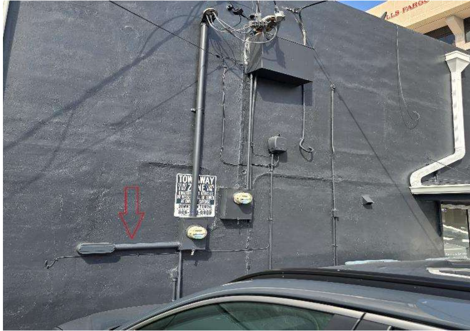
3.6 Space 2605 - MISSING MAIN DISCONNECT
