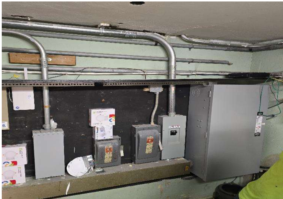
5.1 Space 2603 Equipment area
