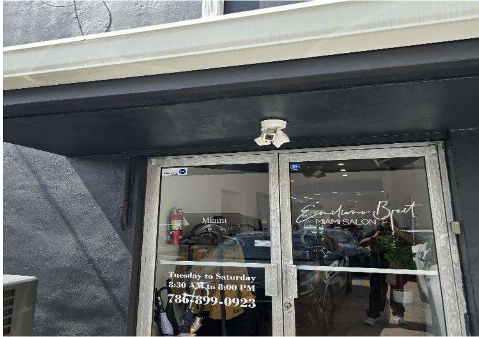
19.1 Bldg. egress lighting - space 2603
