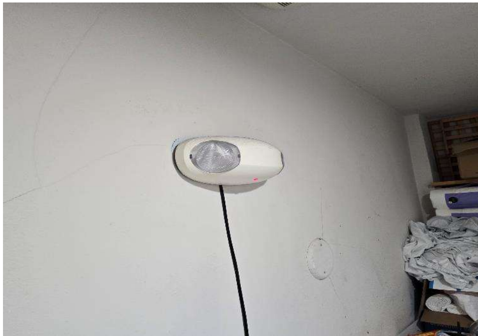
18.3 Emergency lighting – PROVIDE PERMANENT CONNECTION
