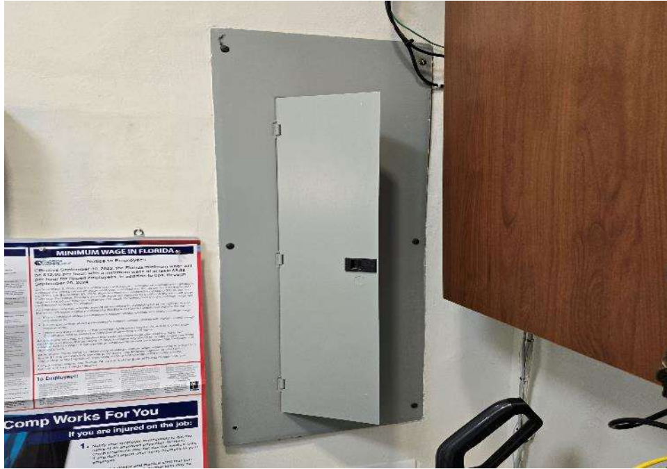
5.2 Space 2605 Equipment area
