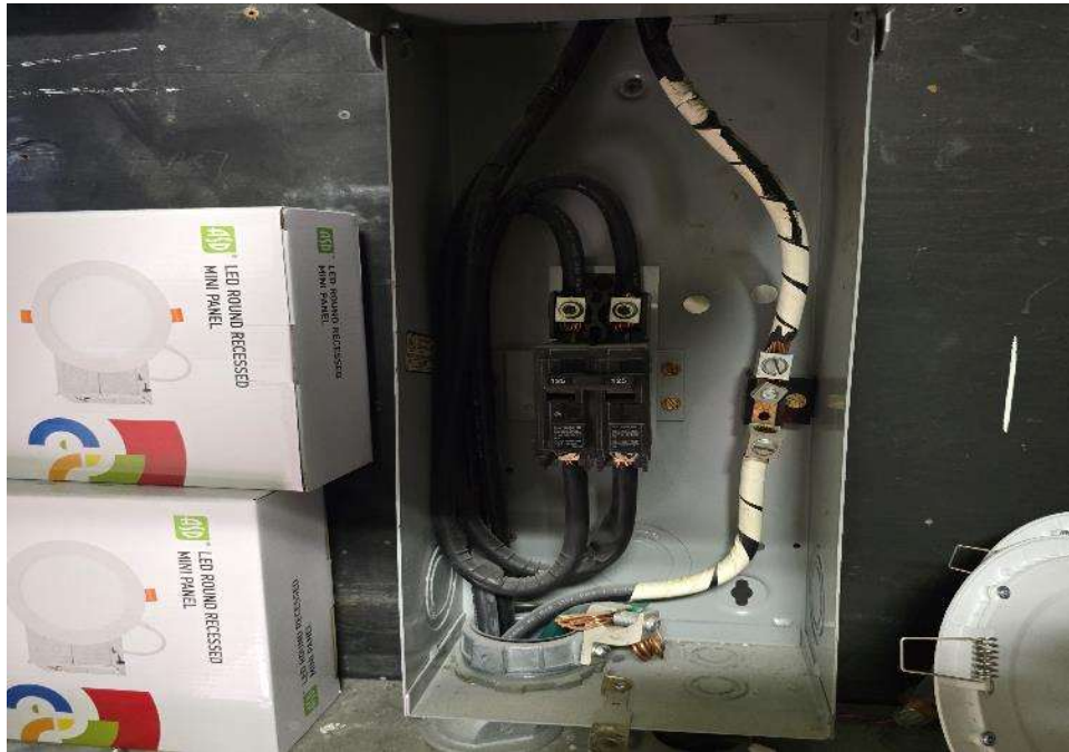
3.4 Space 2603 Panel A Main Disconnect 125A
