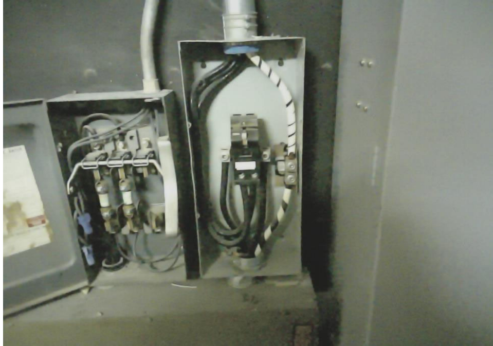
4.2 Main Disconnect Panel A (space 2603)
