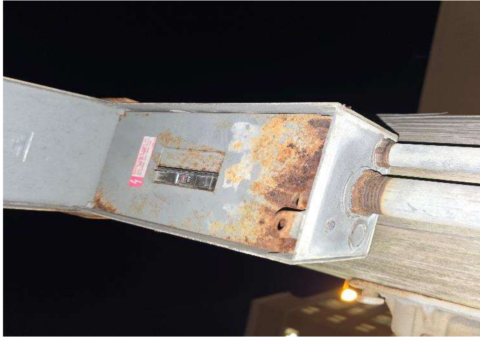
24.1 Wiring in open parking - REPLACE DISCONNECT SWITCH
