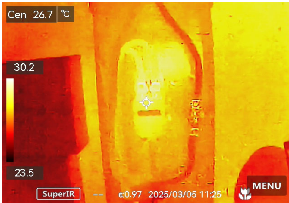
4.3.1 Main Disconnect Panel B (space 2603) – Delta T 1.7 (C)
