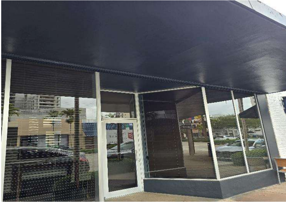
19.3 Bldg. egress lighting (space 2605) - PROVIDE LIGHT
