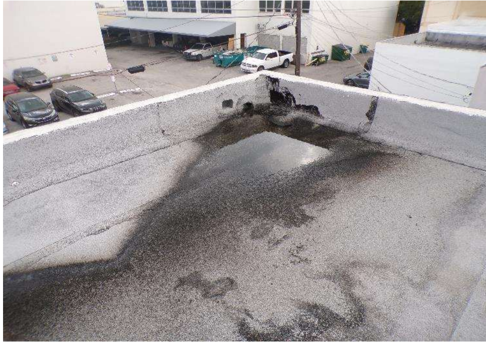
Parapet and overflow scuppers as primary and secondary roof drainage systems
