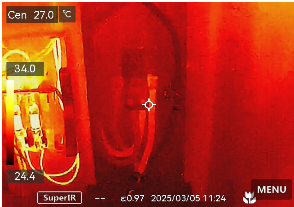
4.2.1 Main Disconnect Panel A (space 2603) – Delta T 2.0 (C°)
