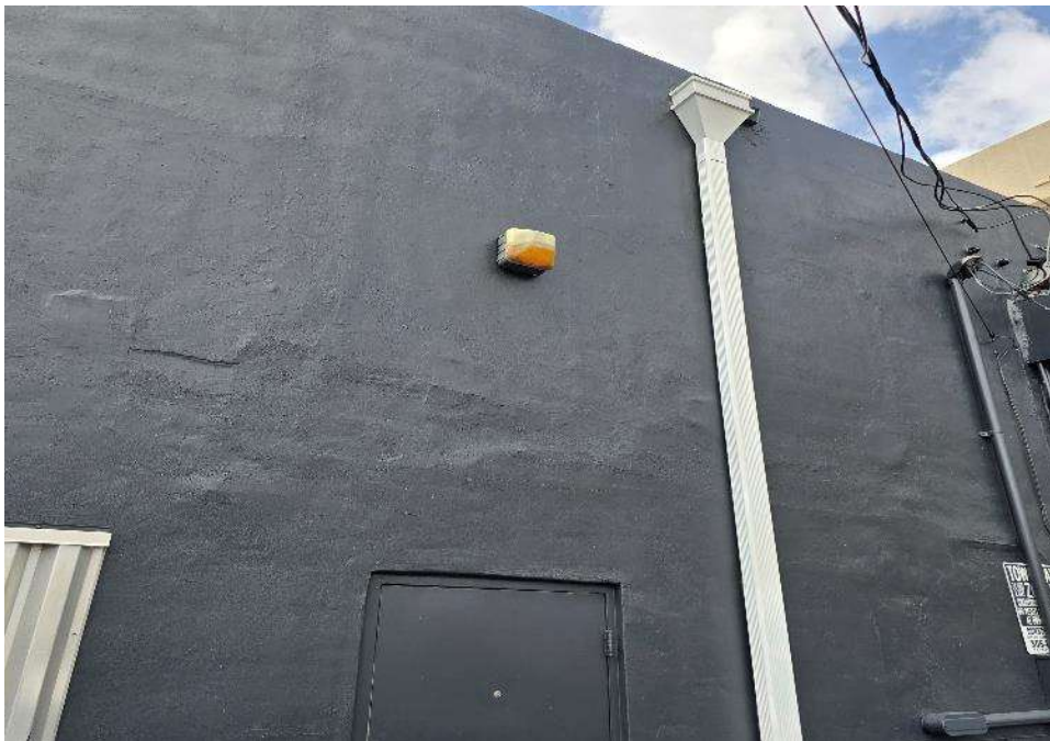
19.4 Bldg. egress lighting (space 2605) - REPLACE LIGHT
