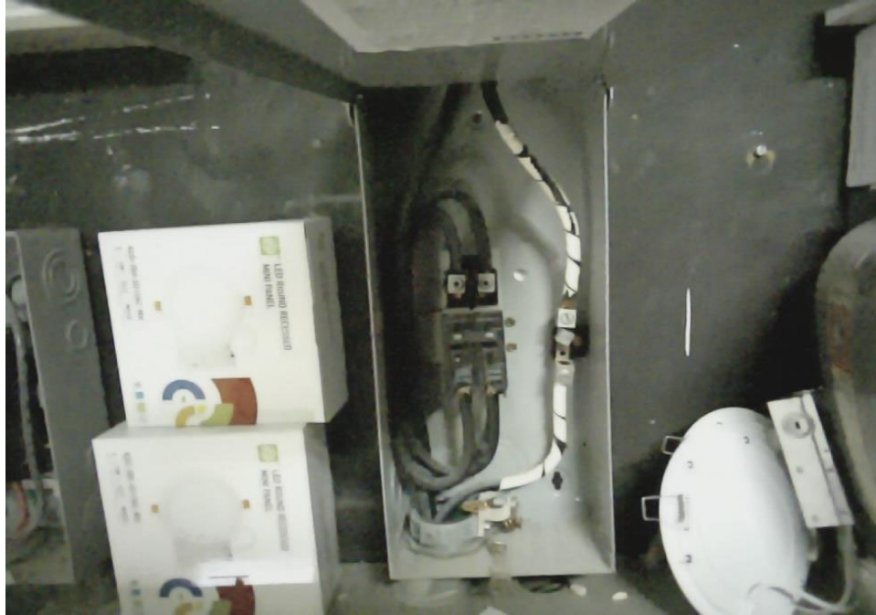
4.3 Main Disconnect Panel B (space 2603)
