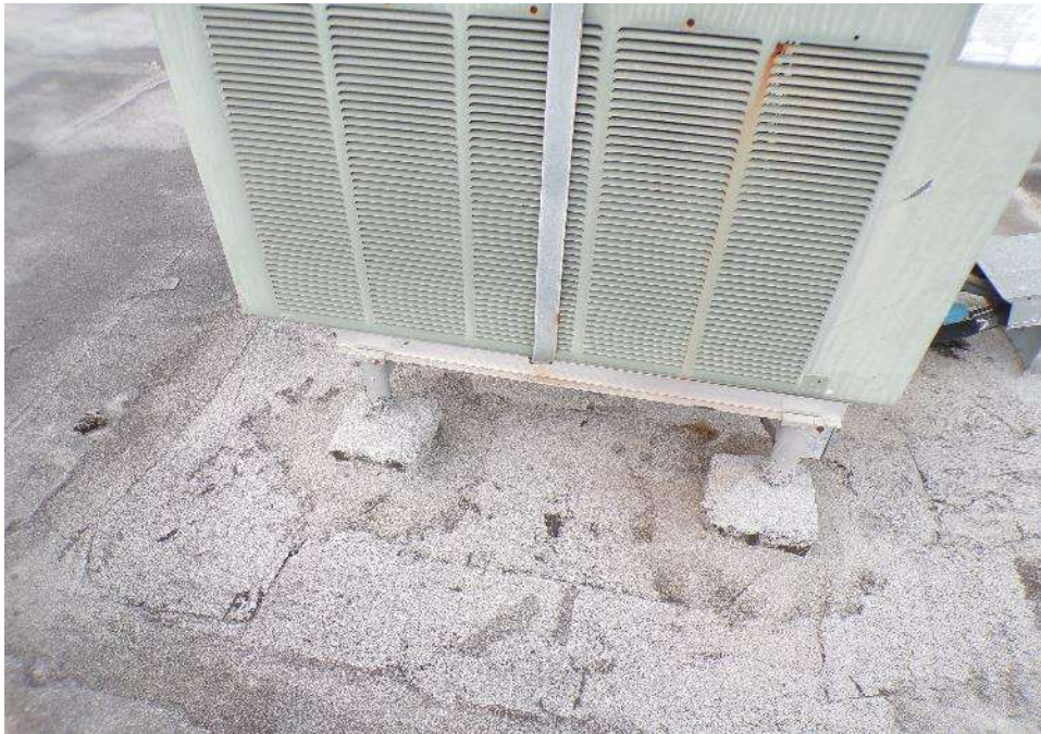
RTU supported by an aluminum stand on the roof
