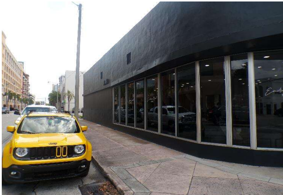
Aluminum-framed storefront along the north and west exterior walls of the building
