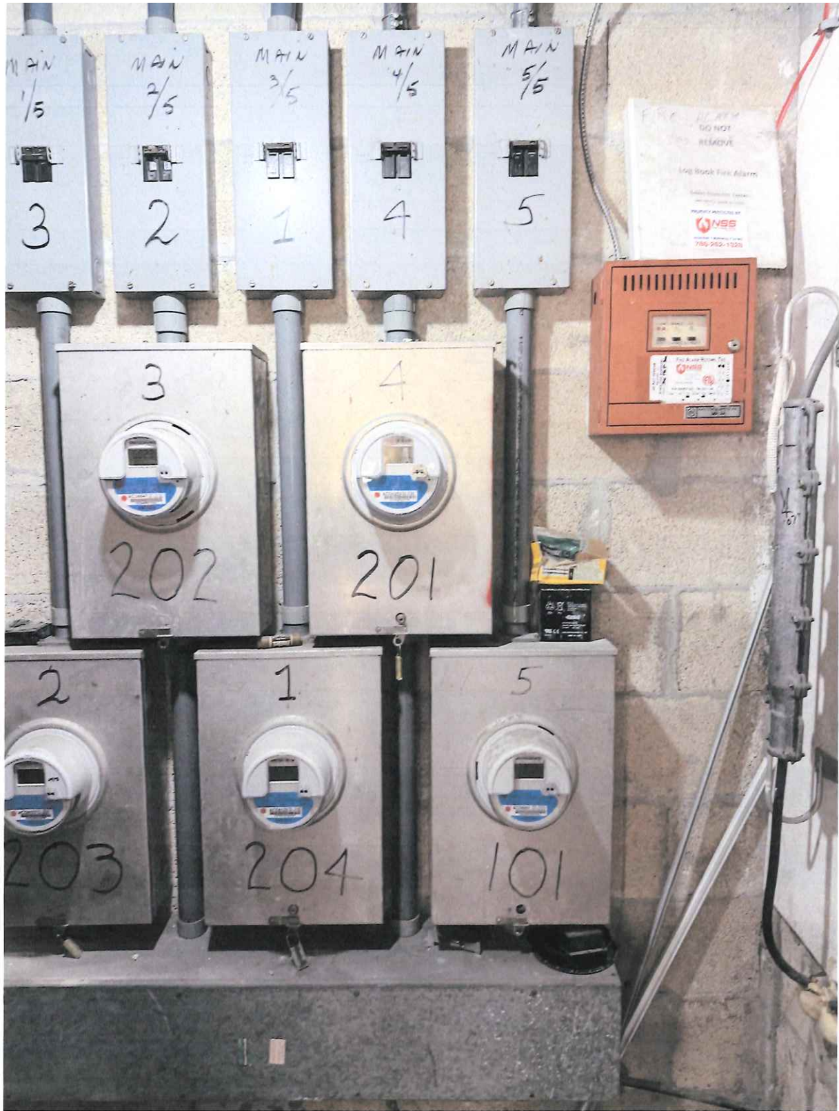
Electrical Room Meters & Mains
