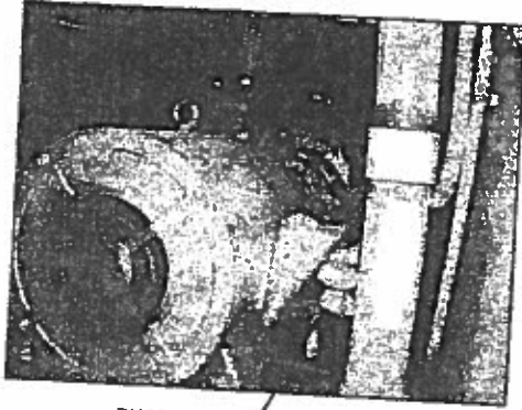
PHOTO #25 BASEMENT WATER PUMP ROOM PROVIDE COVER
