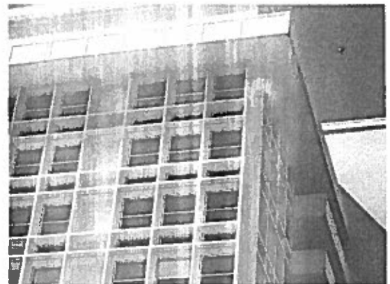
Figure 8-Spalls at Precast Beam at roof
