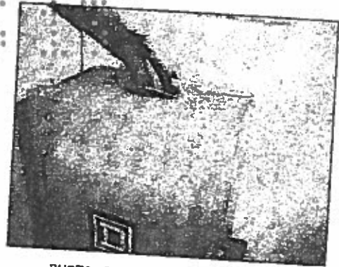
PHOTO #26 BASEMENT WATER PUMP ROOM PROVIDE PROPER CONNECTION TO BOX.
