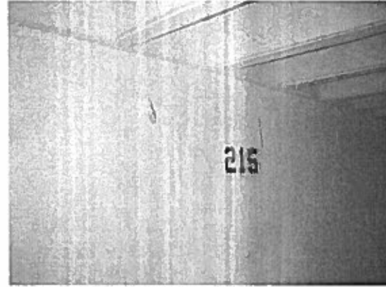
Figure 4-Cracks/Spalls along Garage wall
