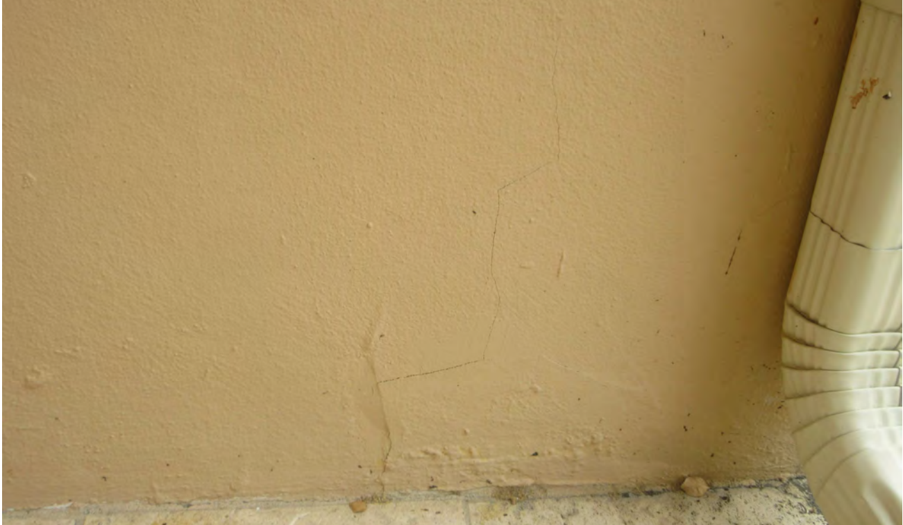
Exterior Wall- Cracking
