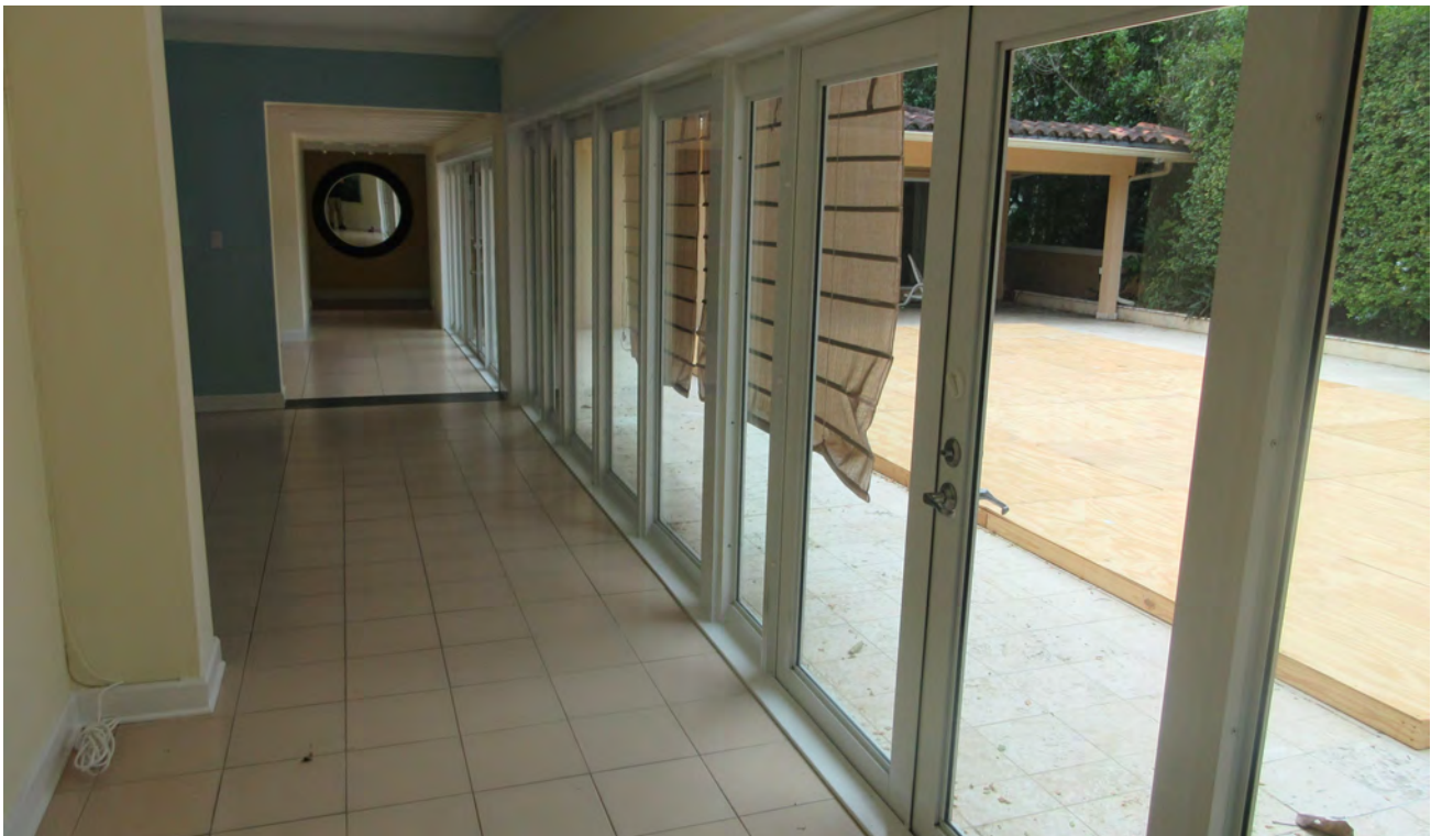
Non-Functional Glass Doors
