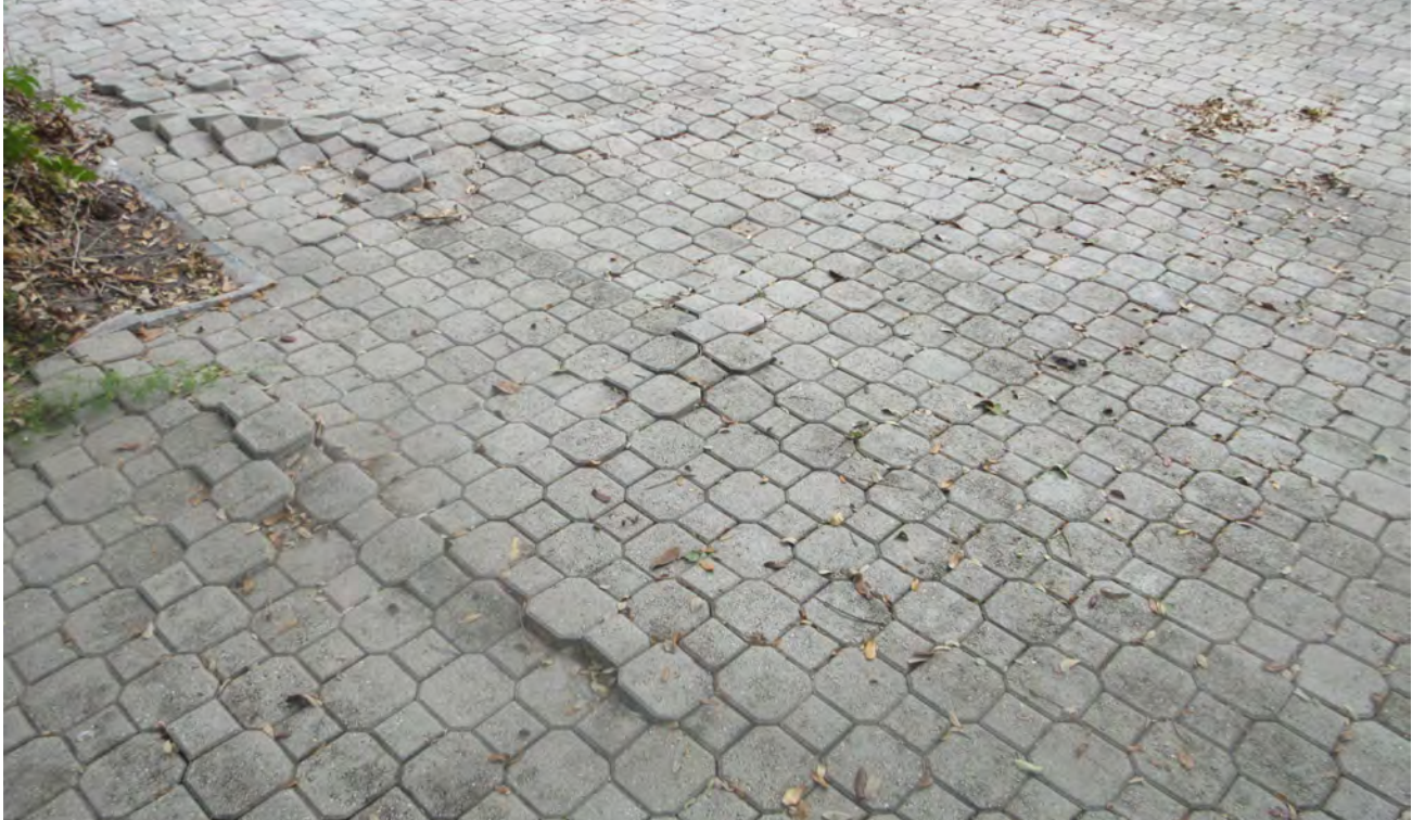
Driveway- Heaving of Pavers
