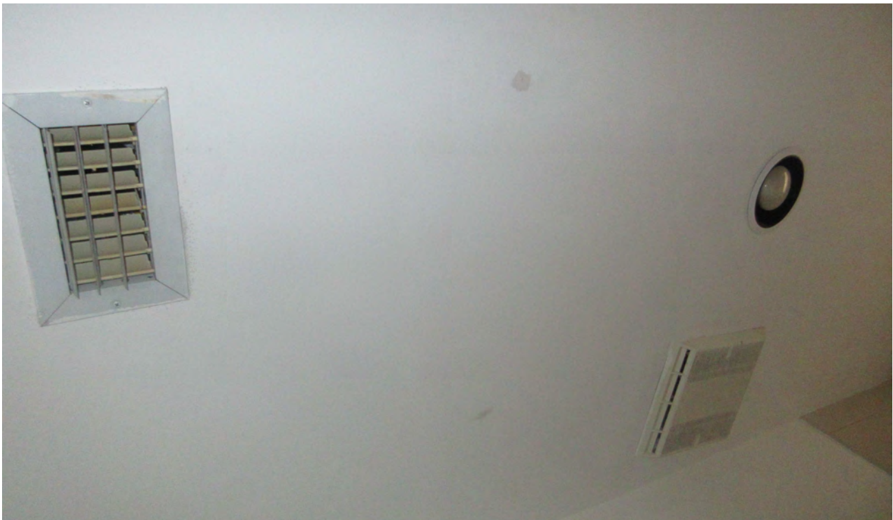
Interior Ceiling- Water Stains
