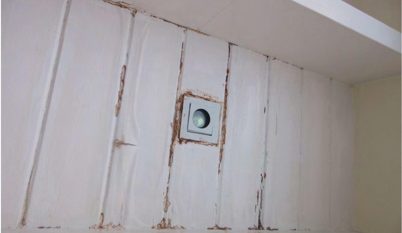
Interior Ceiling- Water Damage and Leaks
