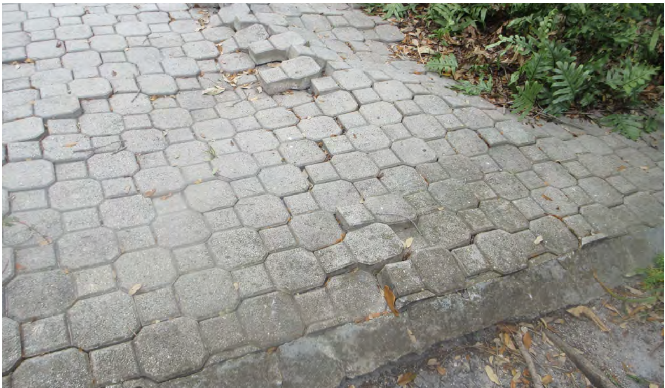
Driveway- Heaving of Pavers
