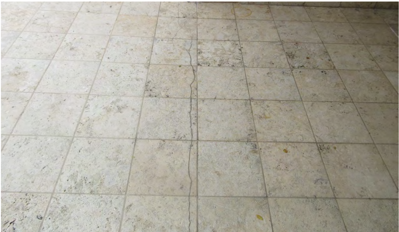
Floor Tile- Cracking
