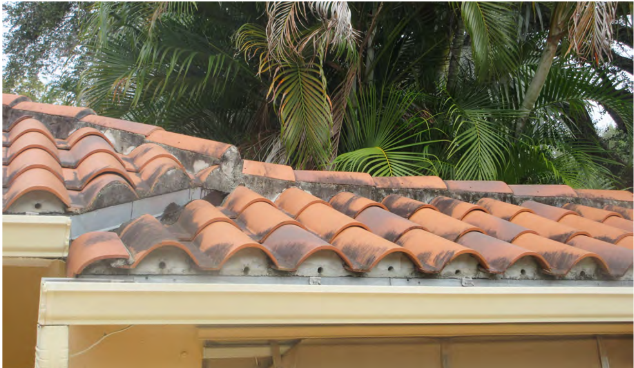
Roof- Patching Evident
