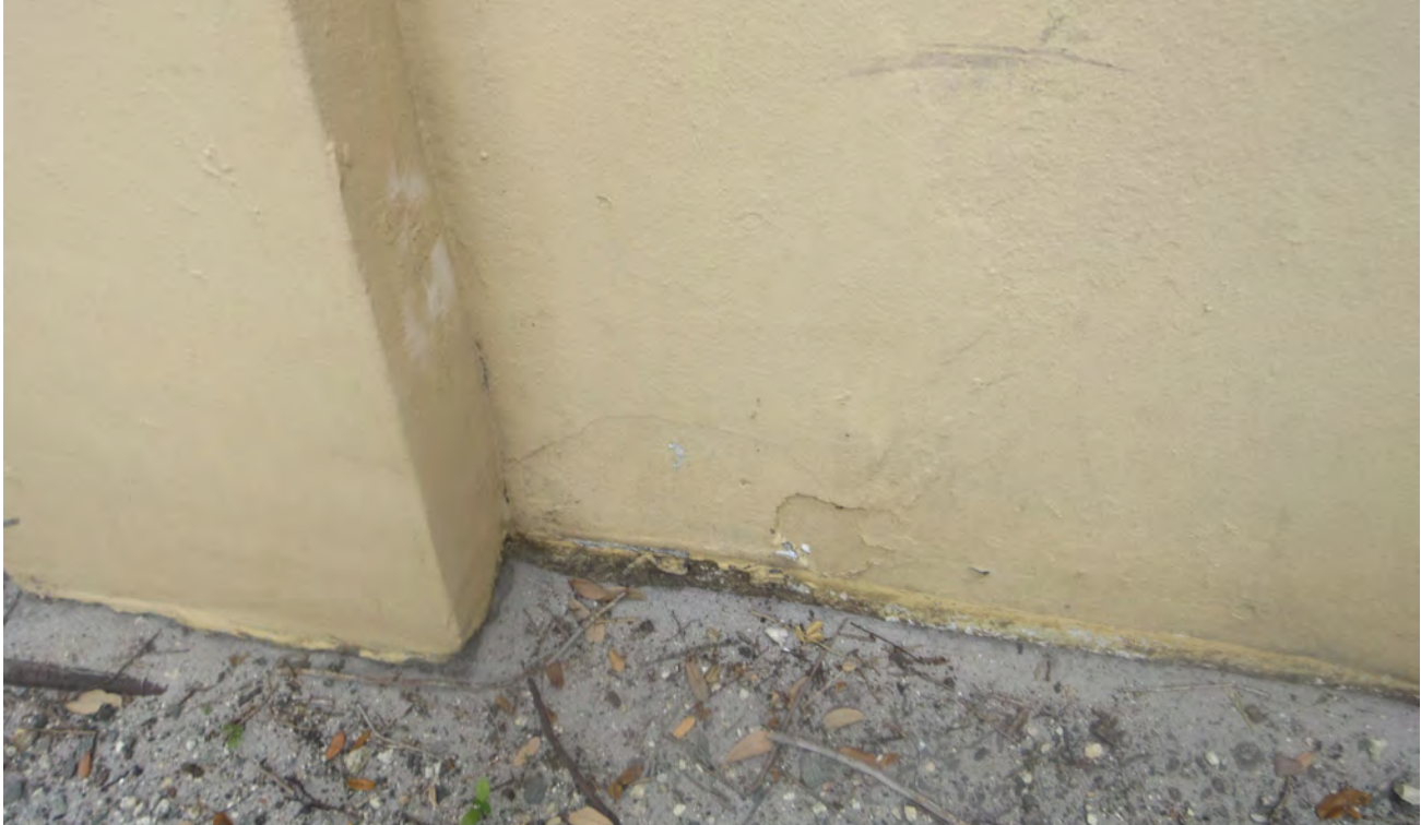
Exterior Walls- Cracking
