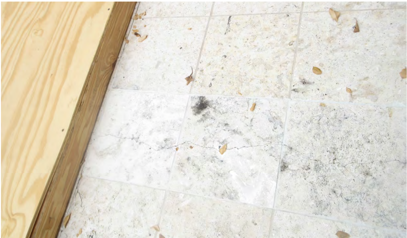
Pool Deck Cracking
