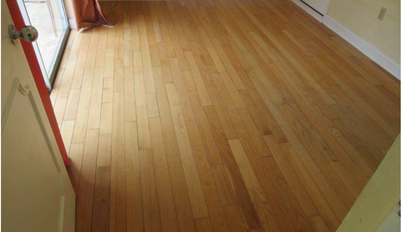
Wood Flooring- Cupping
