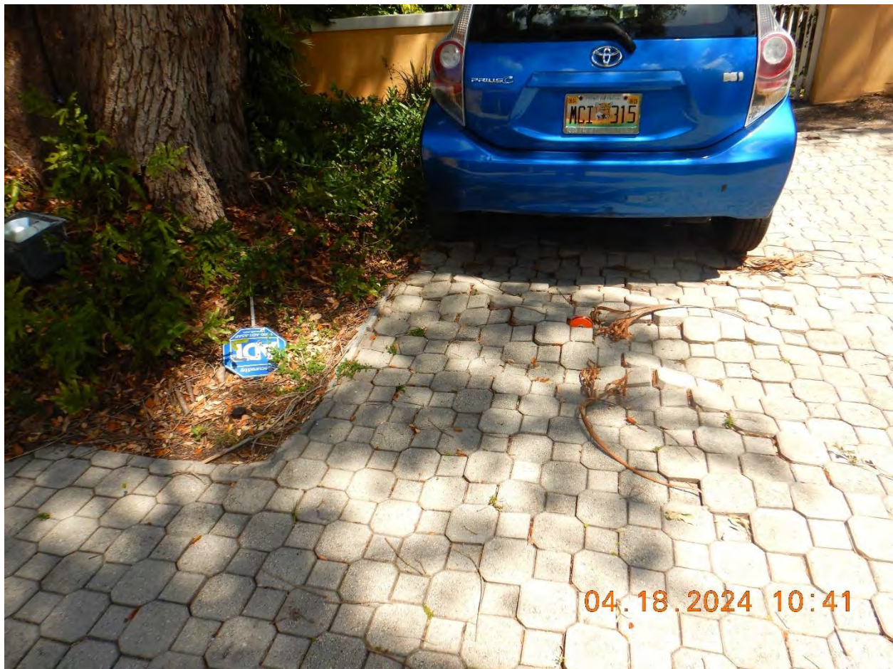
Pavers lifted due to roots.
