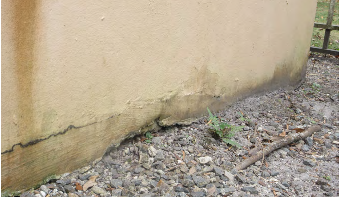
Erosion/Spalling of Foundation
