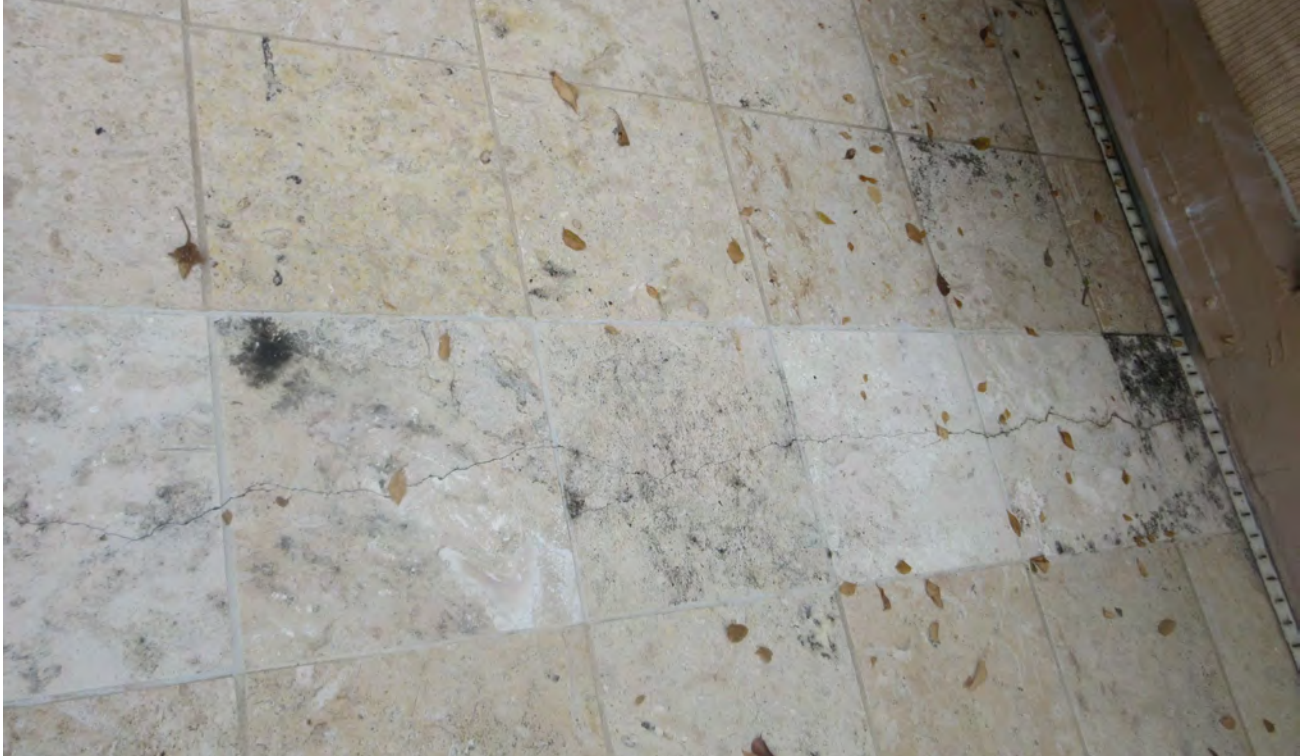
Pool Deck Cracking
