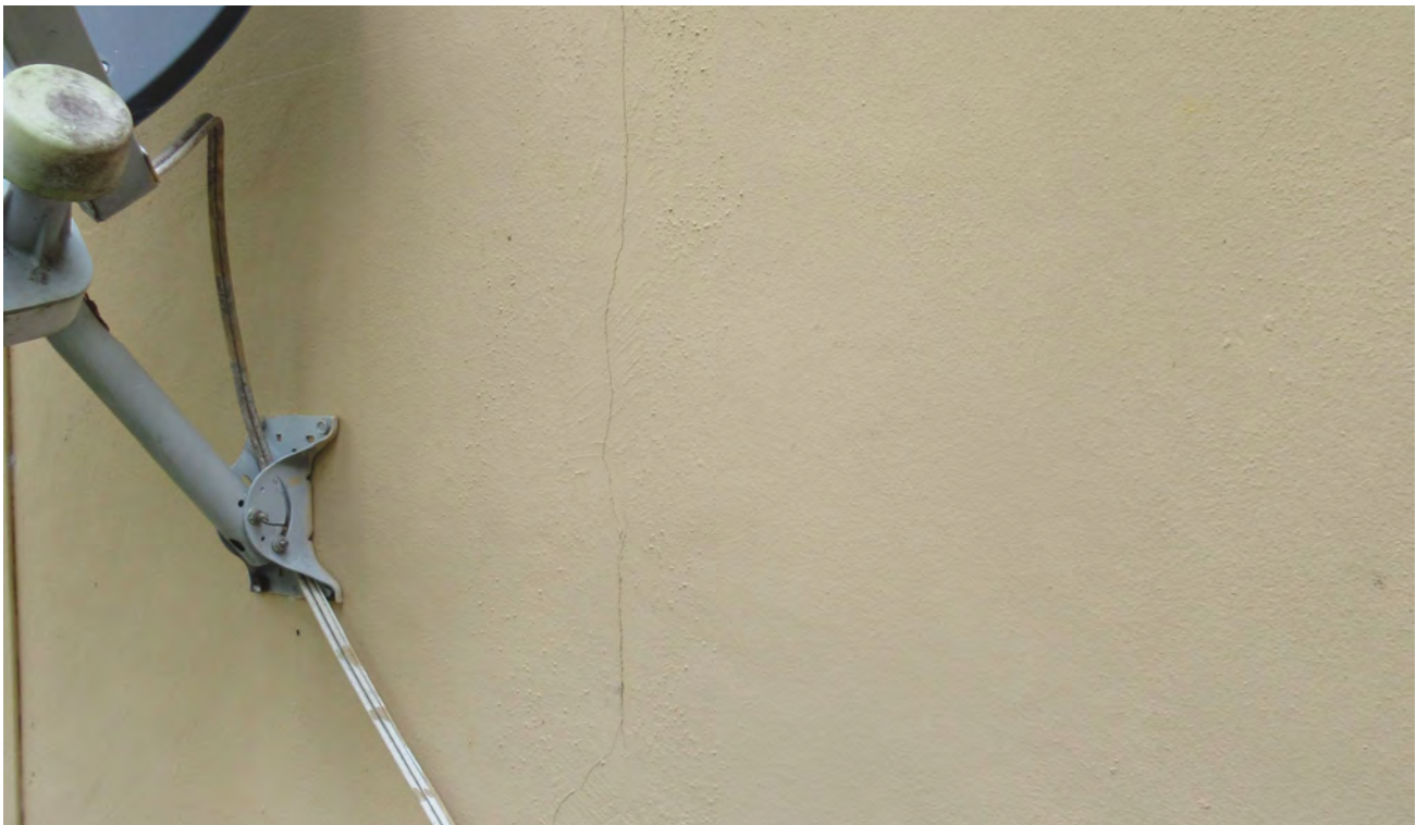
Exterior Walls- Cracking
