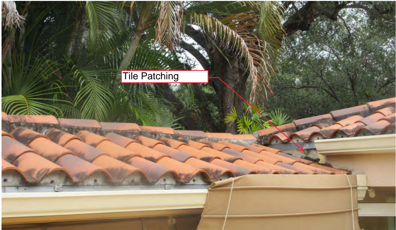
Roof-Degradation of Tiles
