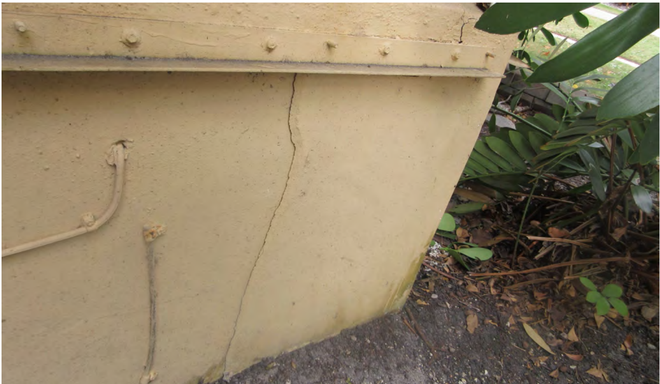
Exterior Wall Cracking - Foundation Failure
