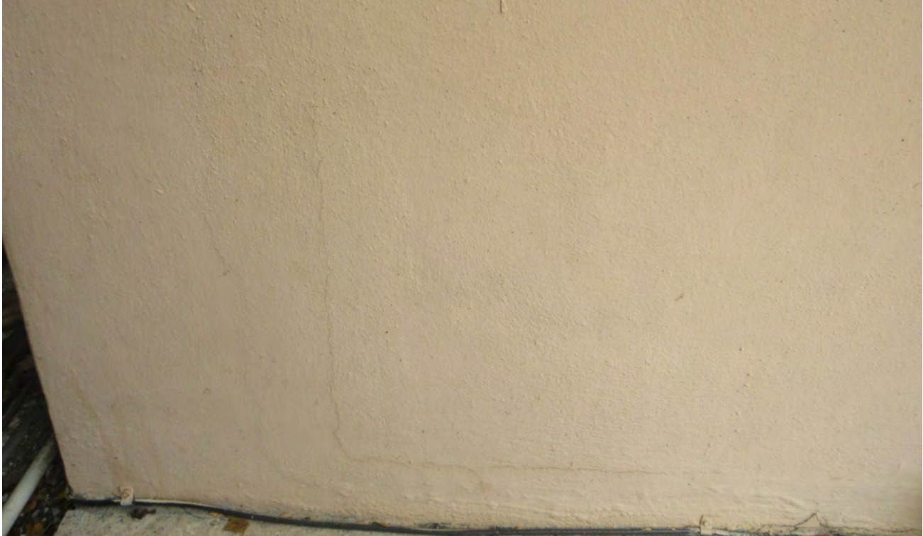
Exterior Walls- Cracking
