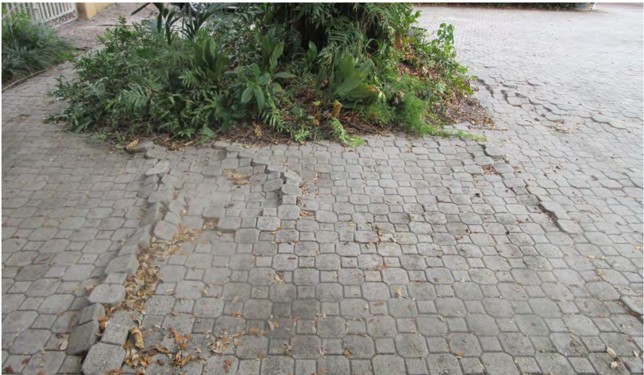
Driveway- Displacement of Pavers
