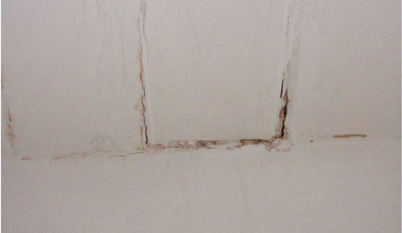
Ceiling- Water Staining
