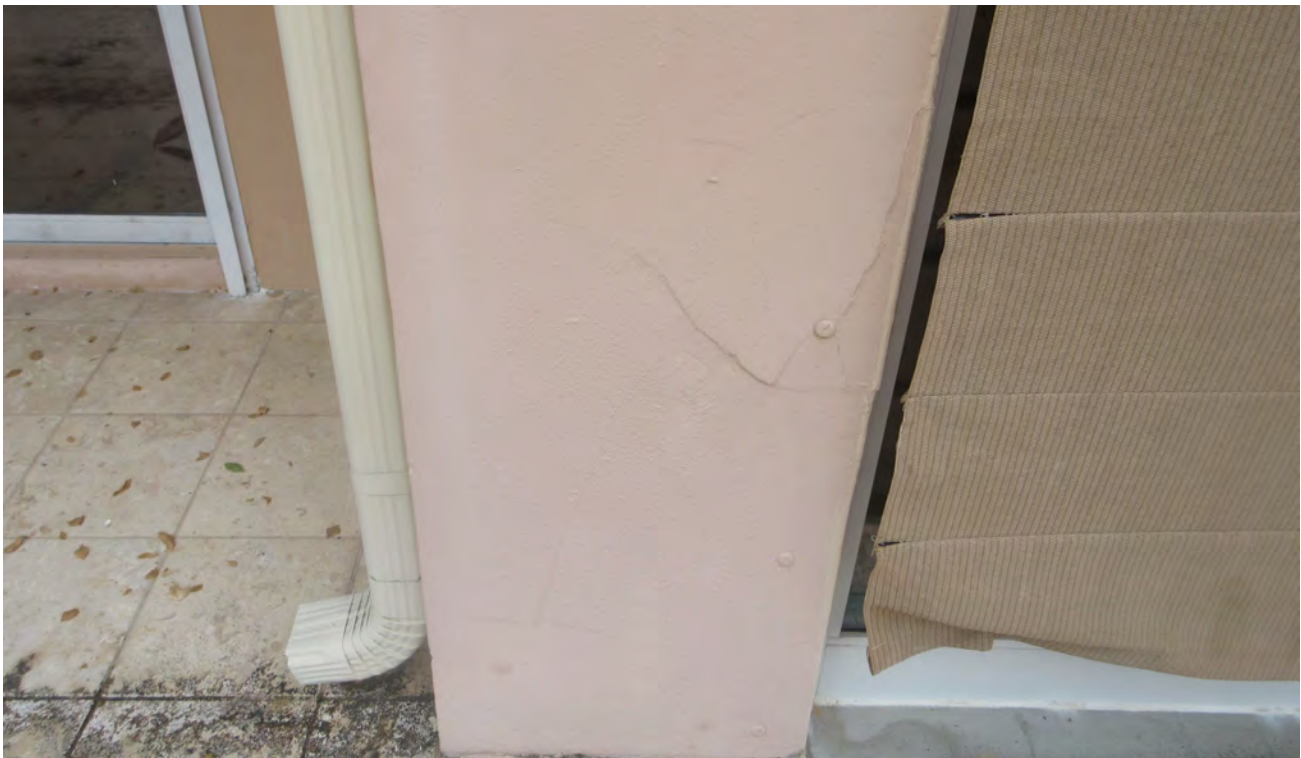
Exterior Wall- Cracking
