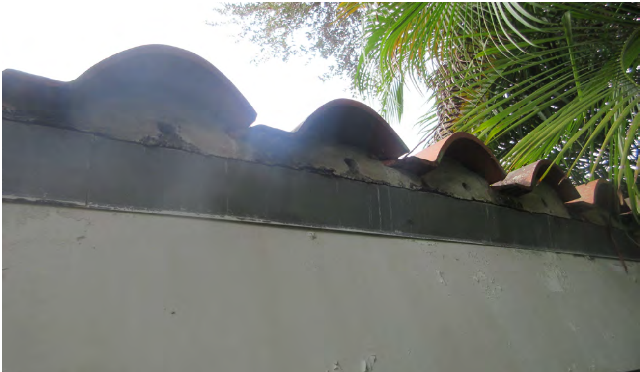
Roof- Degradation of Tile
