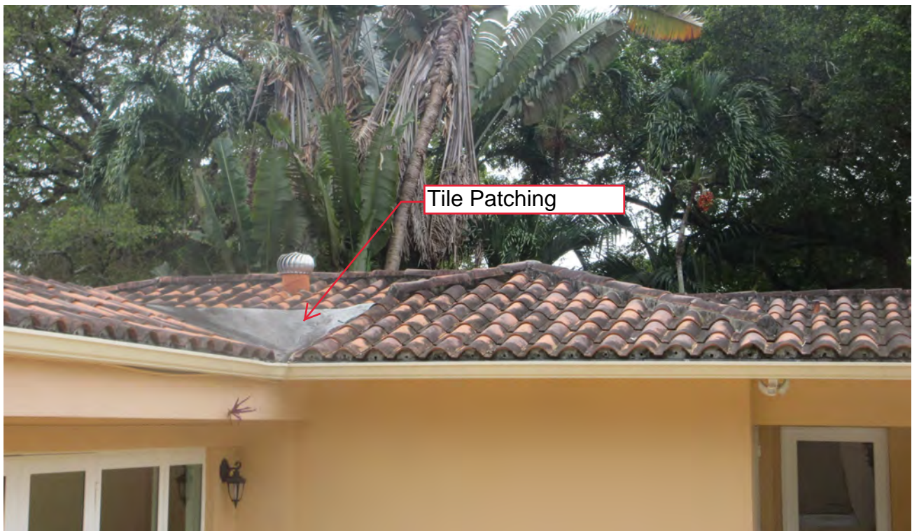
Roof- Degradation of Tiles/Patching
