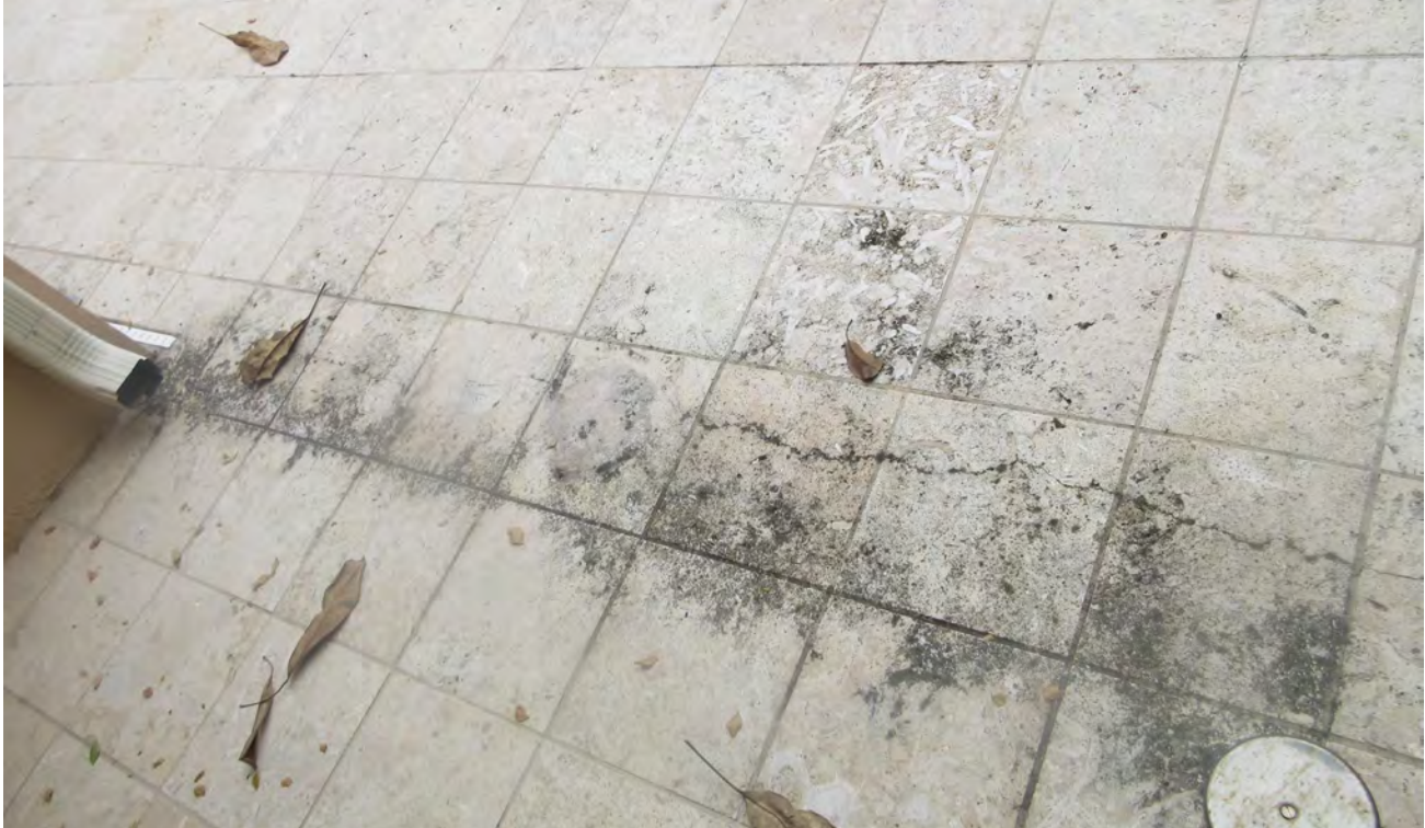
Pool Deck Cracking
