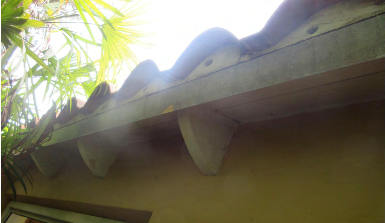
Roof- Degradation of Soffit
