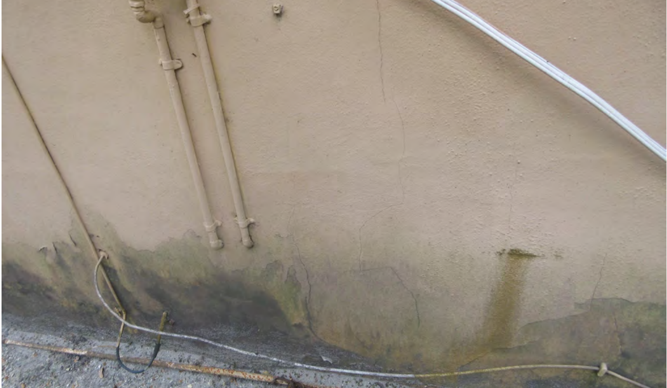
Exterior Walls- Degraded Stucco
