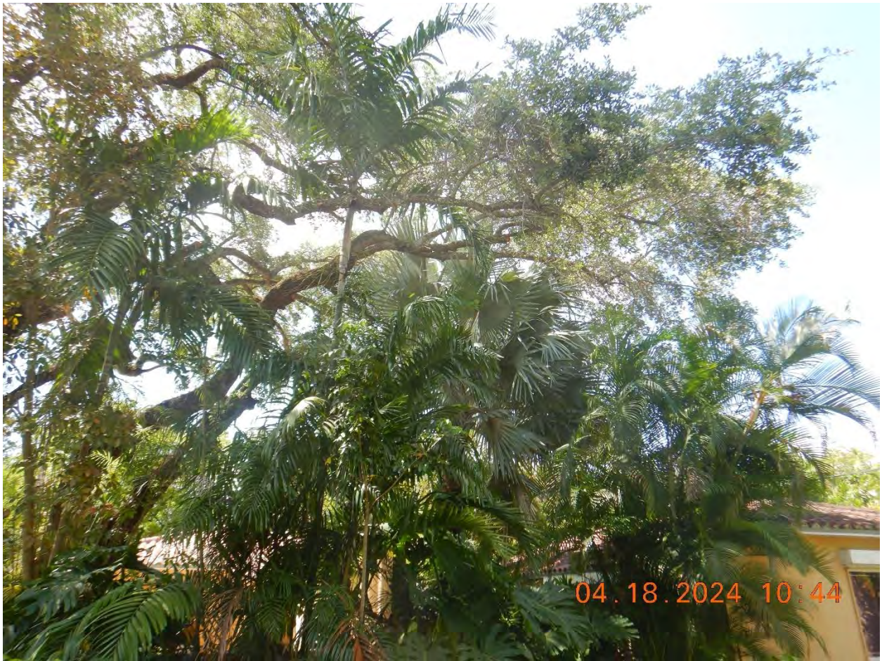
Branches with heavy end weight over roof of living area.
