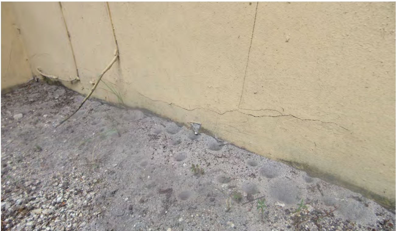
Exterior Wall Cracking - Foundation Failure
