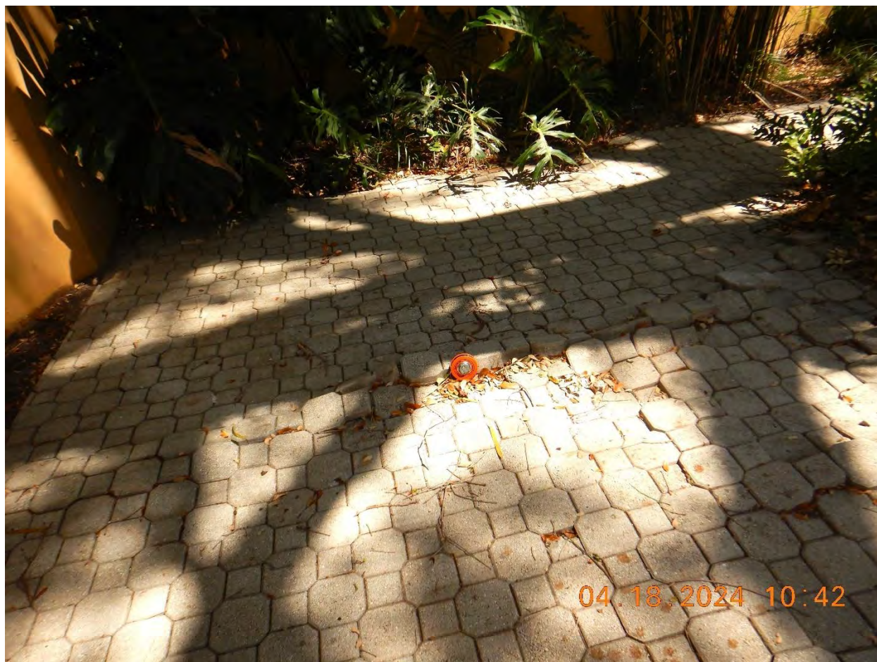
Pavers lifted due to roots.
