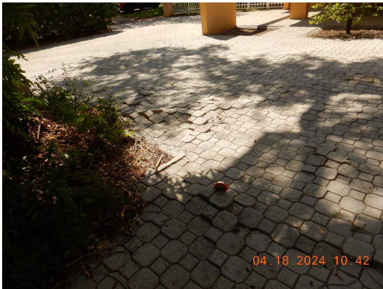
Pavers lifted due to roots.
