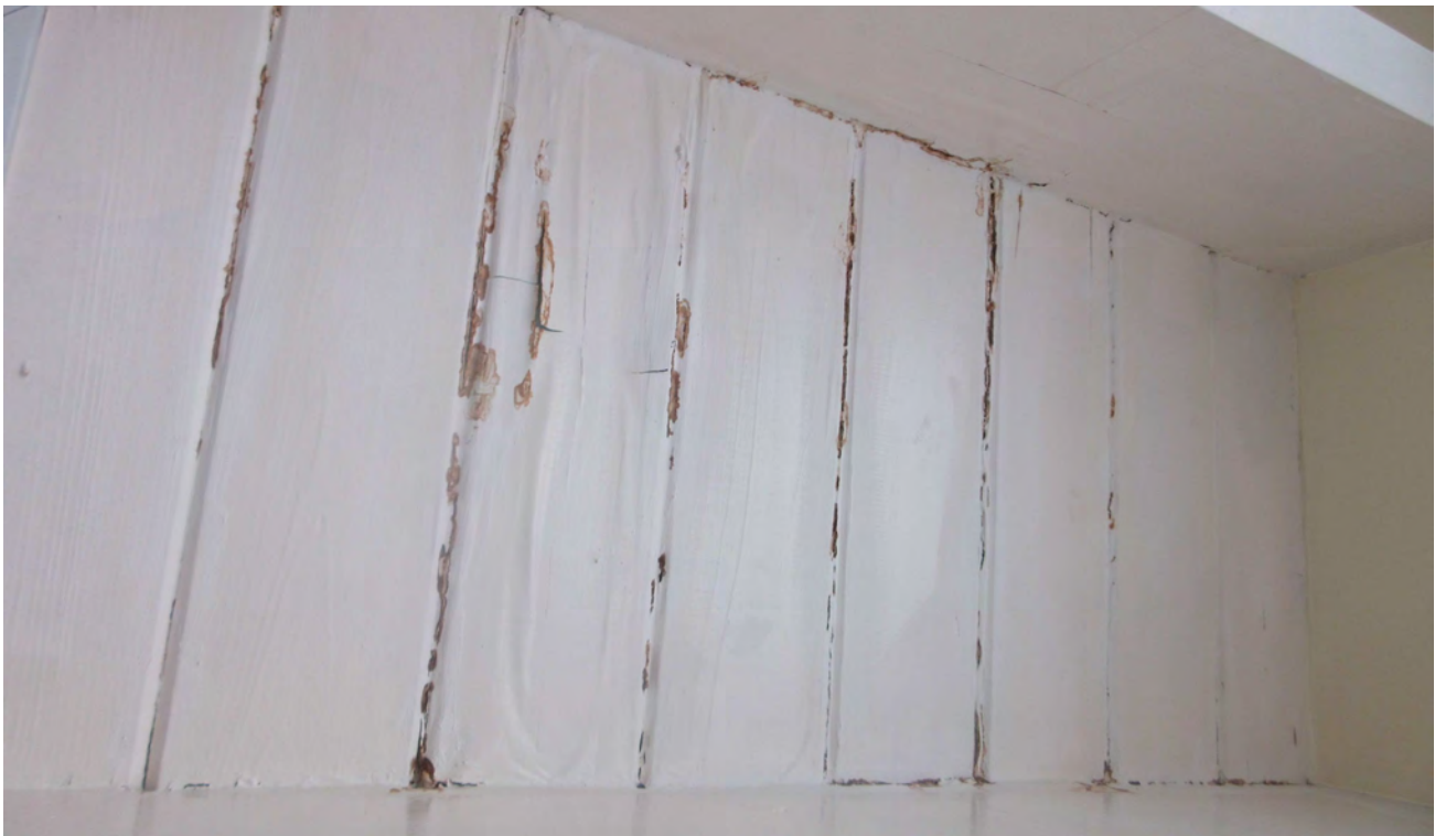
Interior Ceiling- Degradation/Leaks
