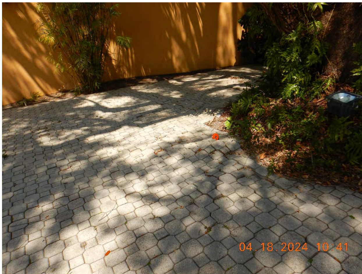
Pavers lifted due to roots.
