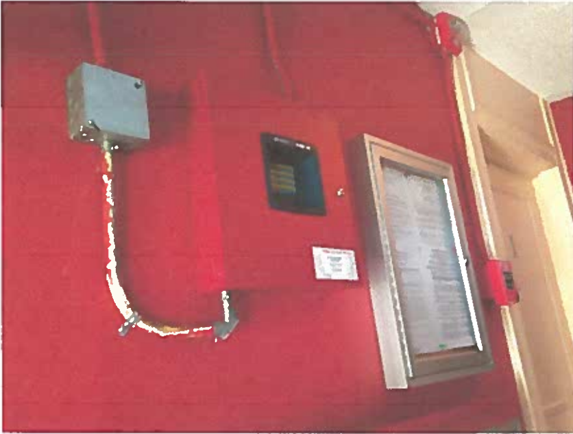
11. FIRE ALARM SYSTEM
