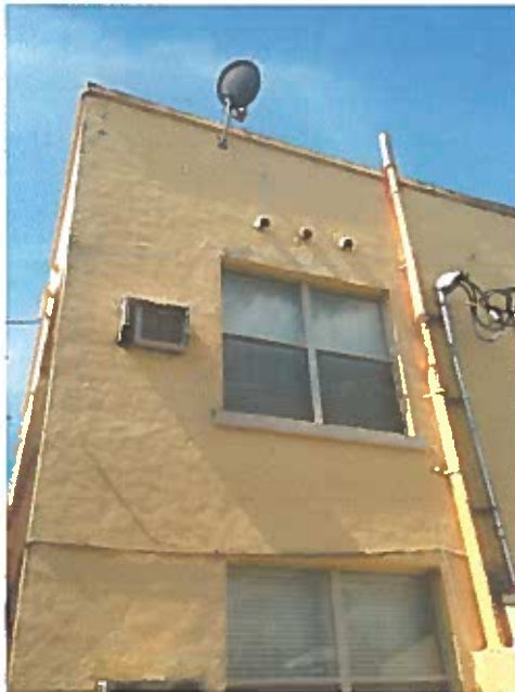
7. PARAPET CRACKS (REAR)
