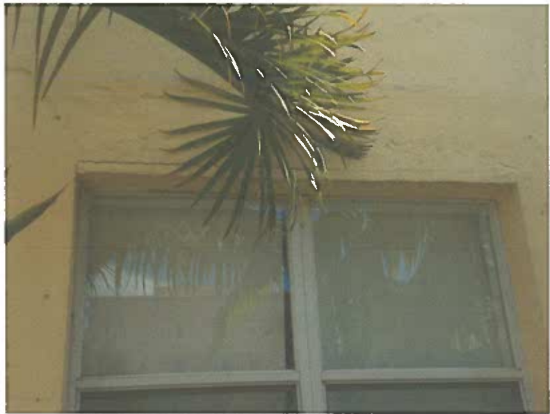
4. EXPANSION CRACK ABOVE WINDOW
