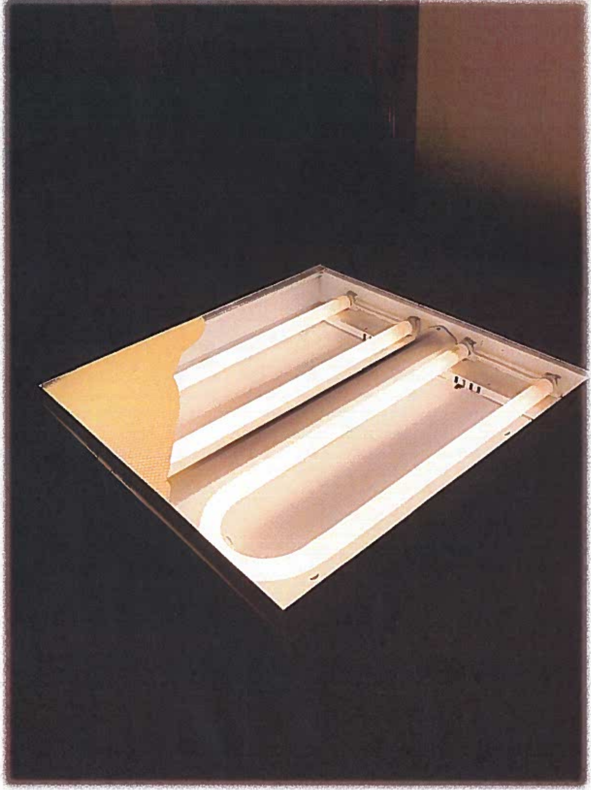
Broken interior light cover
