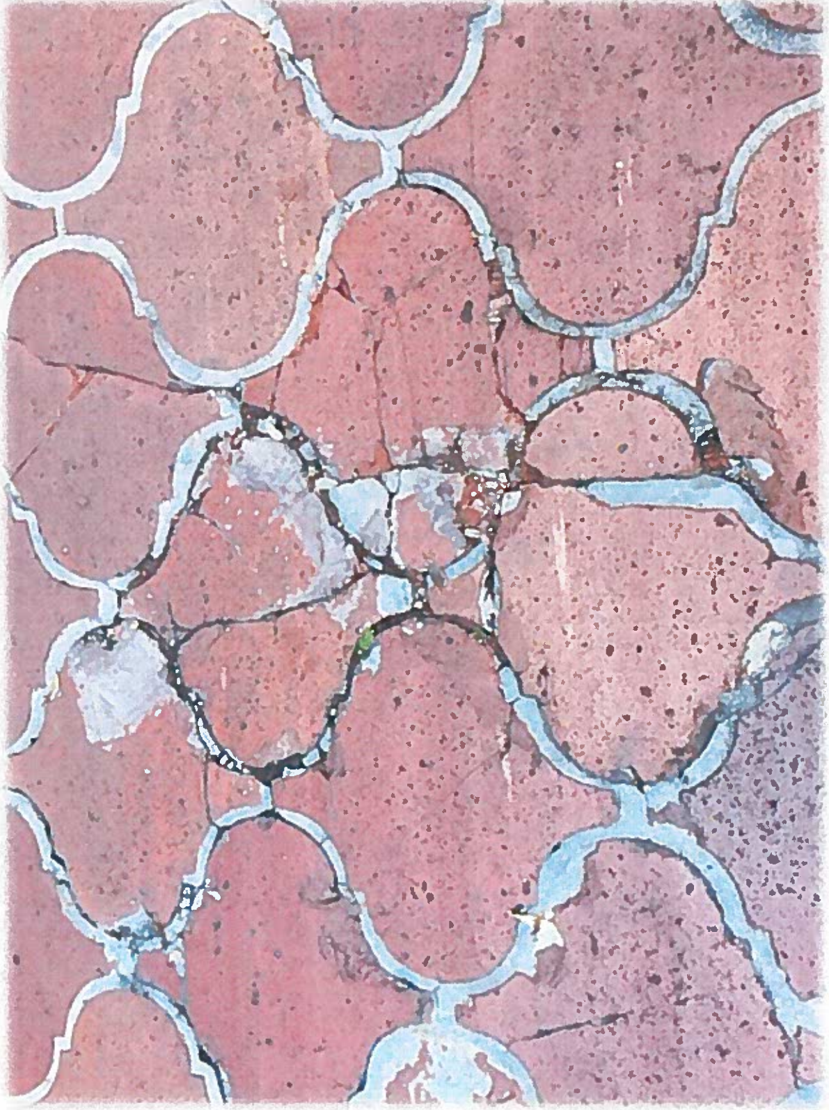
Broken floor tile at the Library entrance
