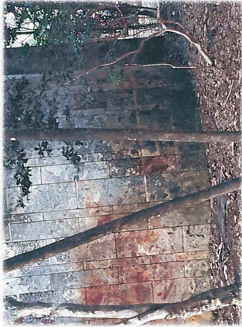
Stained building exterior
