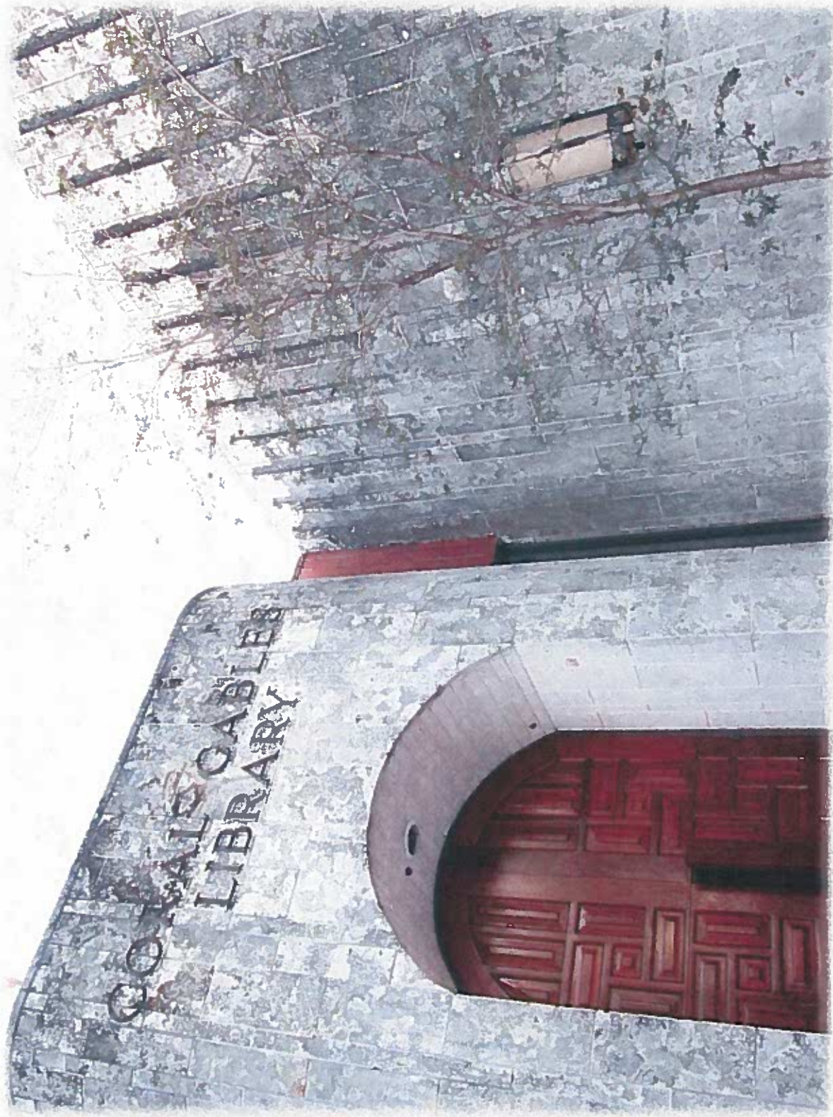
Mold above the Library sign
