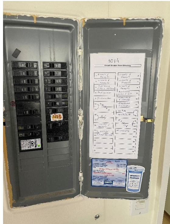
Figure 30: Typical Condo Unit Electrical Panel
