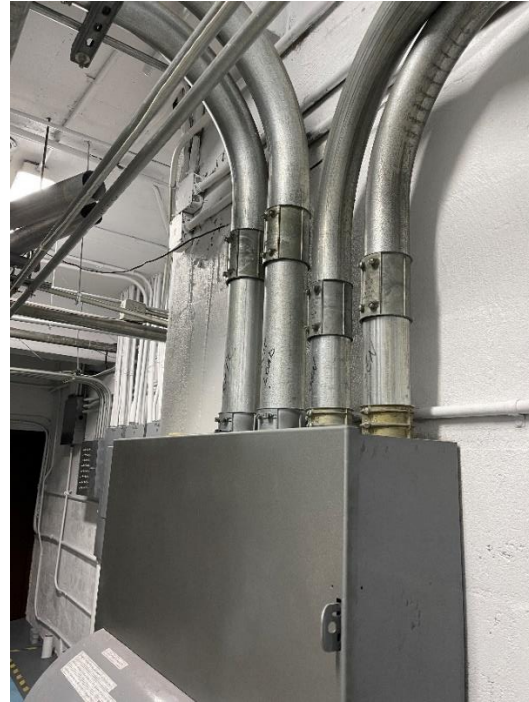
Figure 36: Service Conduit into MTS
