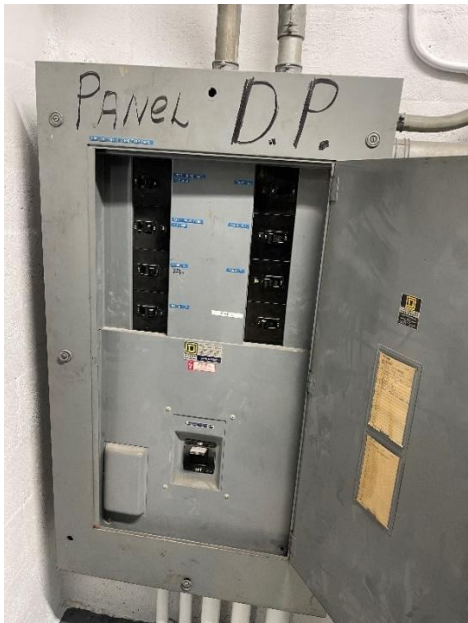
Figure 9: Distribution Panel DP
