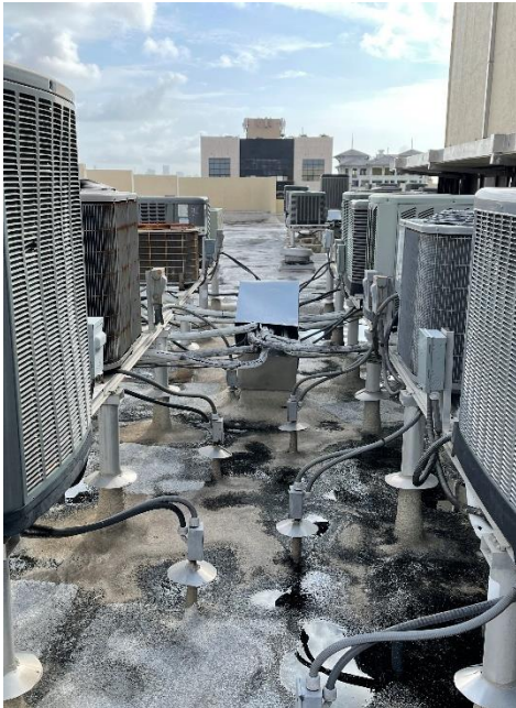
Figure 58: Roof CU Unit Equipment Disconnect
