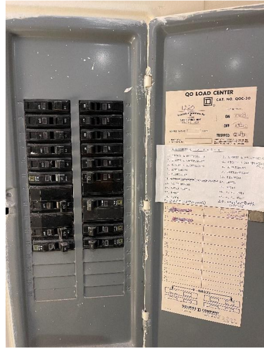
Figure 28: Typical Condo Unit Electrical Panel
