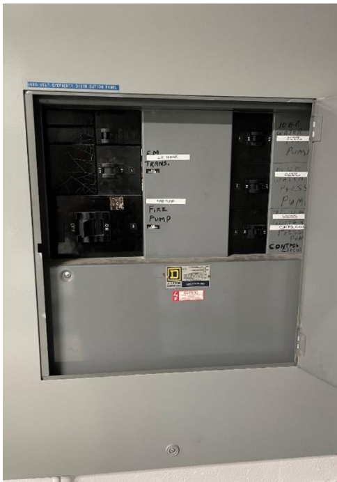
Figure 17: Emergency Distribution Panel
