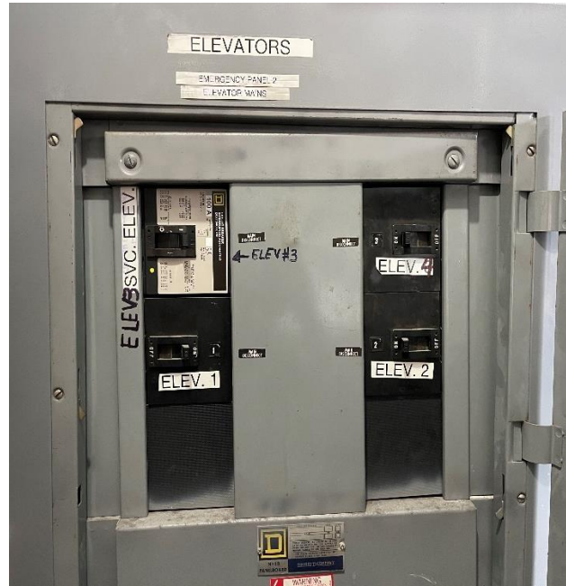
Figure 26: Emergency Panel 2 (Elevators)
