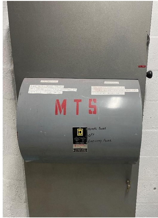
Figure 16: Manual Transfer Switch
