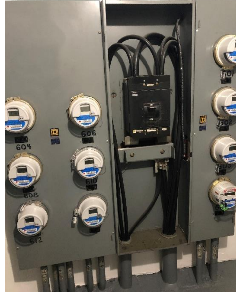
Figure 3: Typical Main Electrical Room & Metering Equipment.
