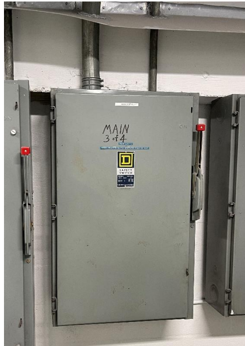
Figure 6: Main 03 of 04 Service Disconnect
