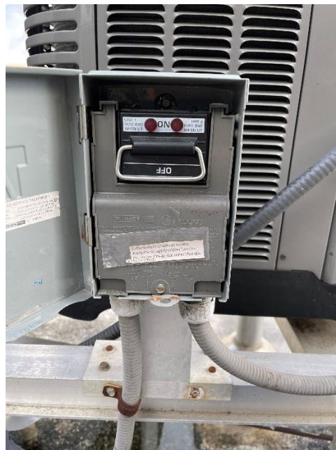
Figure 59: Typical Disconnect Switch for Roof CU Units
