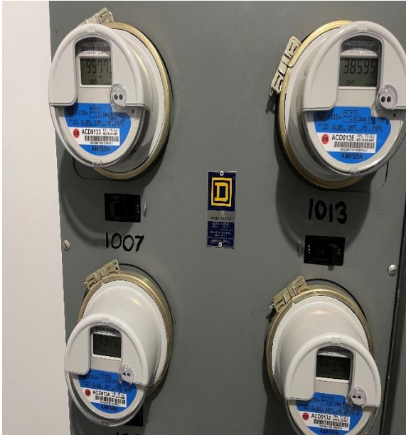
Figure 2: Typical Main Electrical Room & Metering Equipment.
