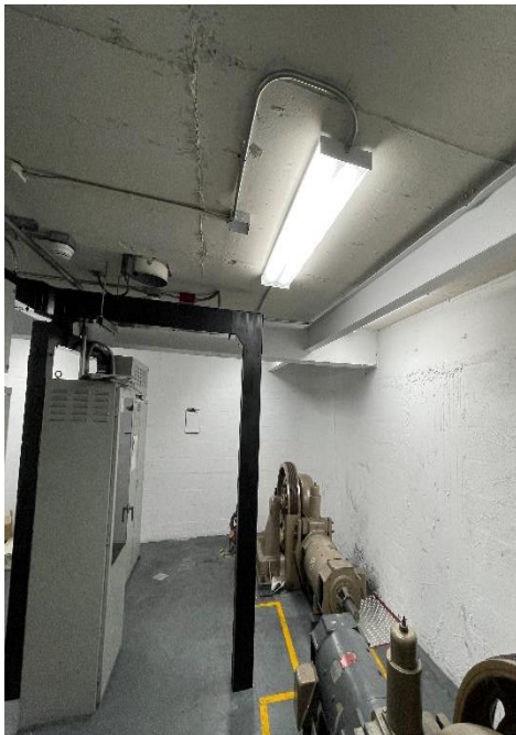
Figure 44: Emergency Lights – Elevator Equipment Room
