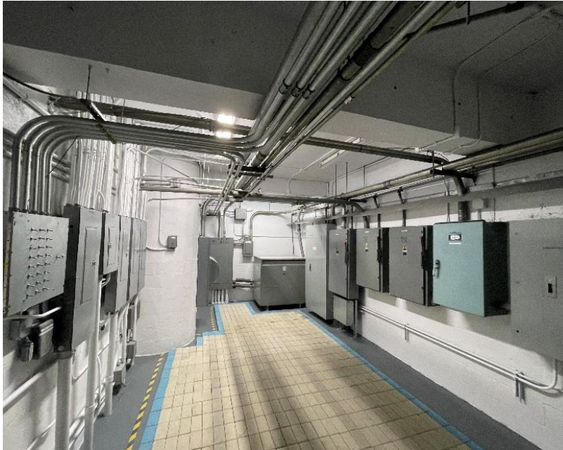
Figure 4: Main Electrical Room & Gutter
