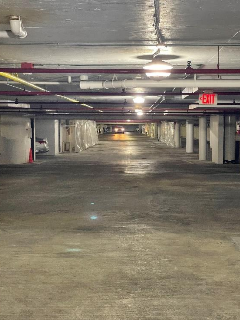
Figure 52: Wiring in Covered Parking Garage
