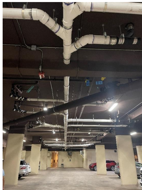
Figure 53: Wiring in Covered Parking Garage
