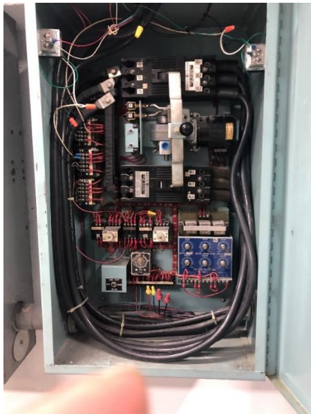
Figure 41: Other Conductors – Emergency Transfer Switch
