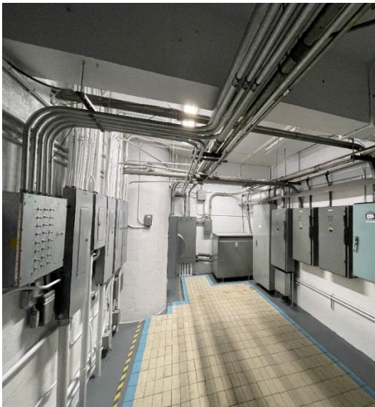
Figure 37: General Conduit Raceway
