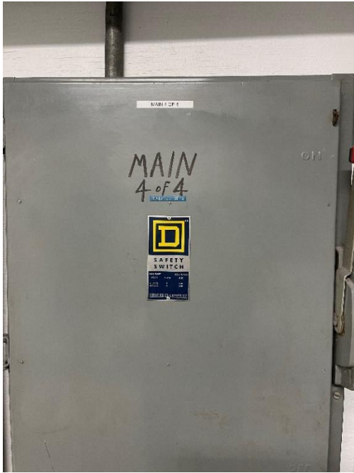
Figure 7: Main 04 of 04 Service Disconnect
