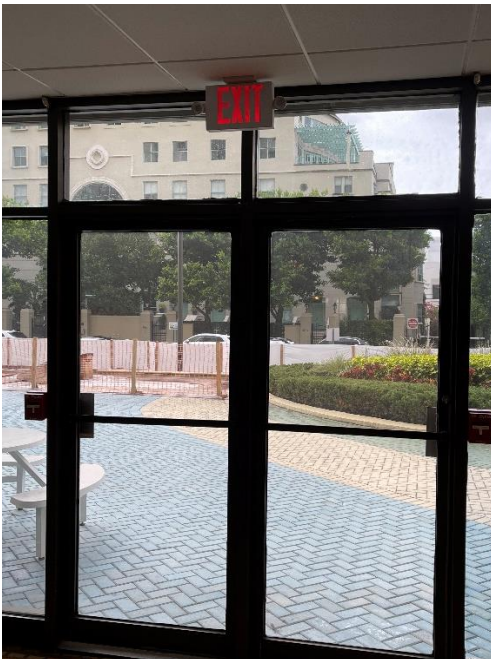
Figure 48: Typical Exit Lights
