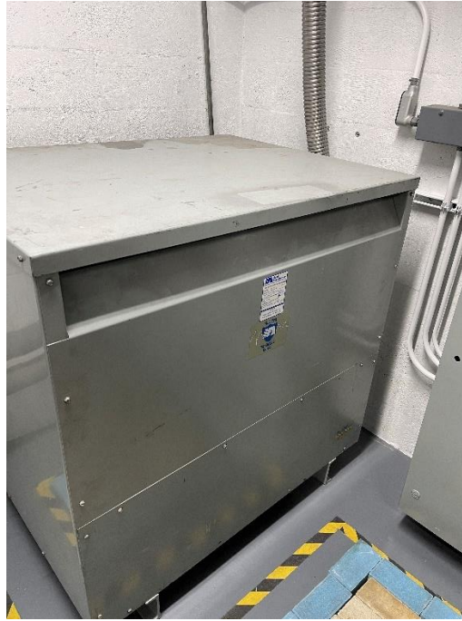
Figure 8: Floor Mounted House Xfmrt
