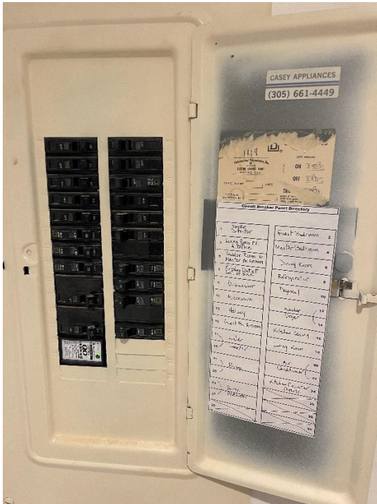
Figure 29: Typical Condo Unit Electrical Panel
