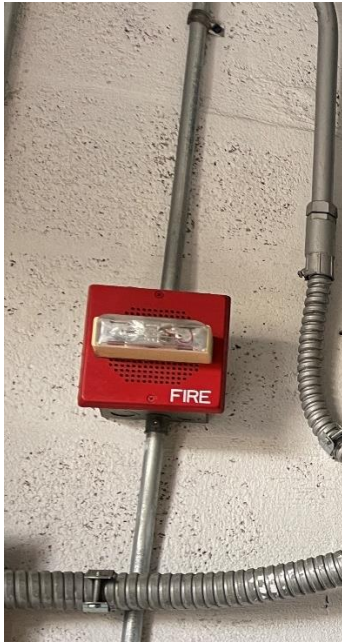
Figure 46: Typical Fire Alarm Speaker Strobe
