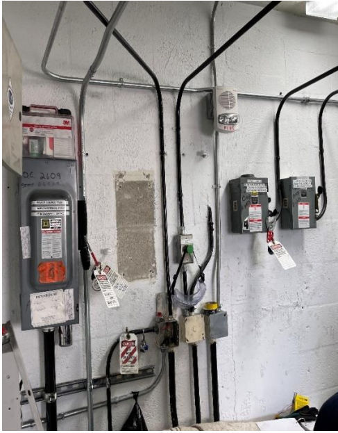
Figure 23: Elevator Machine Disconnects – West Side
