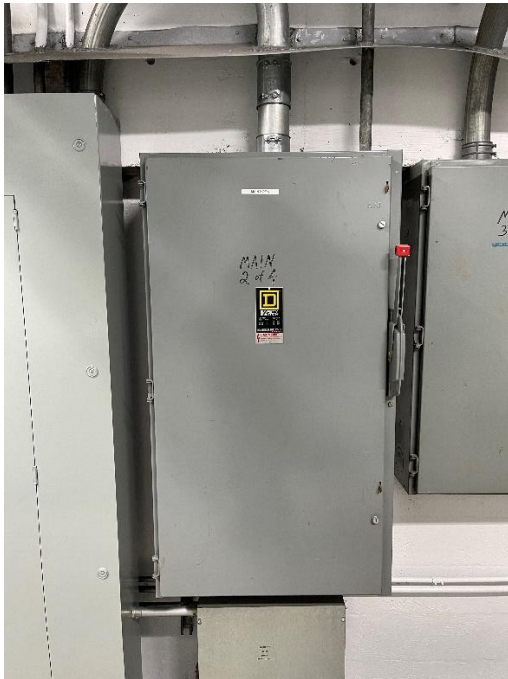
Figure 5: Main 02 of 04 Service Disconnect
