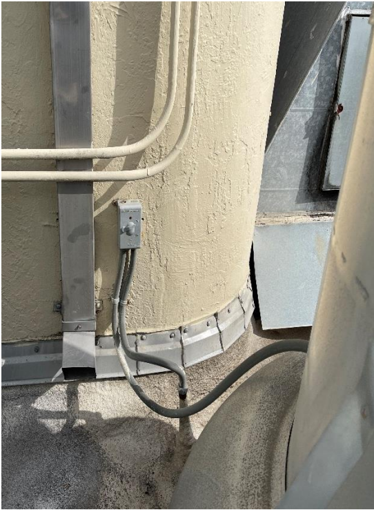
Figure 60: Roof Exhaust Fan Wiring Connection
