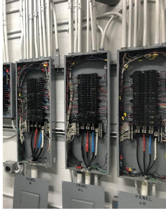
Figure 40: Wires and Cables – Panels M, HL, HR
