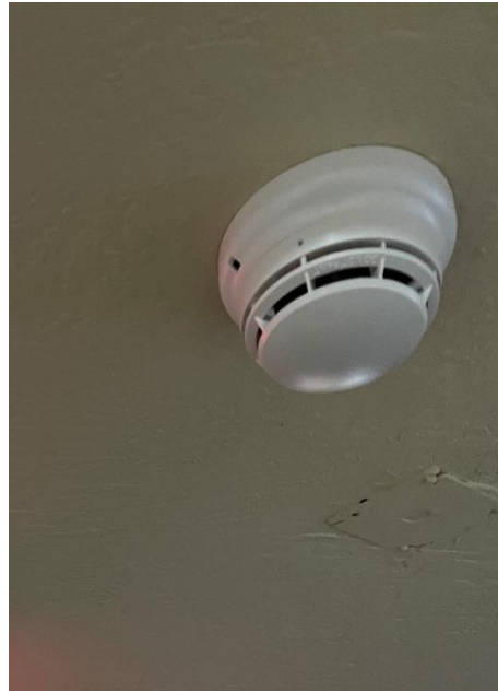
Figure 47: Typical Corridor Smoke detector
