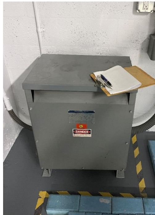
Figure 18: Floor Mounted Emergency Transformer
