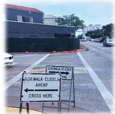
Photo taken on Aragon Ave and LeJeune shows need for sensitivity for pedestrian safety during planning
