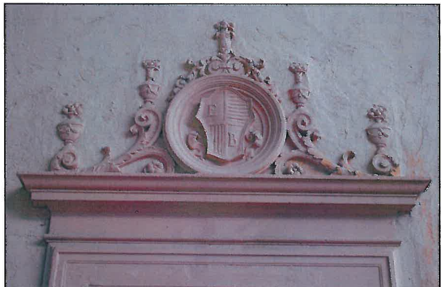
Figures 8 and 9: Main Entry, 2017: Original door behind security door [left]; Detail of decorative ornamentation [right]
