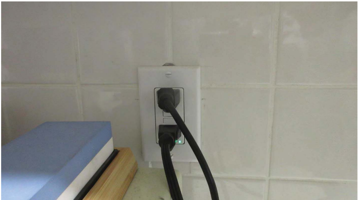
GFCI RECEPTACLE IN KITCHEN.
