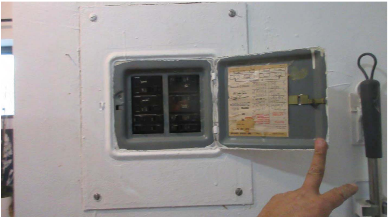
EXTERIOR VIEW OF ELECTRICAL PANEL.
