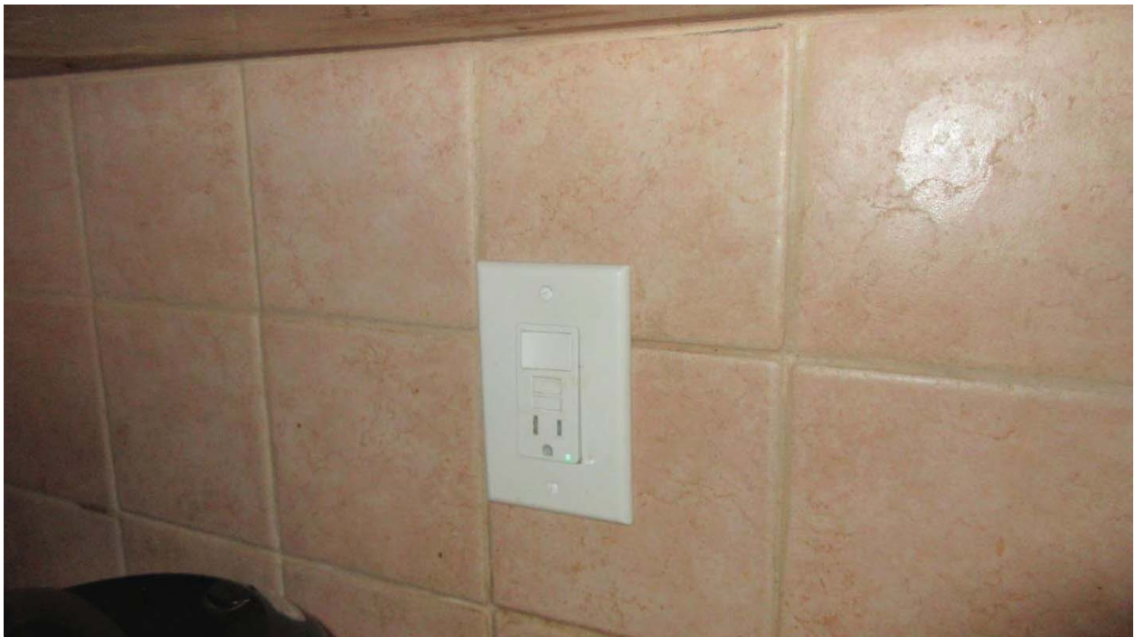
GFCI RECEPTACLE IN KITCHEN.
