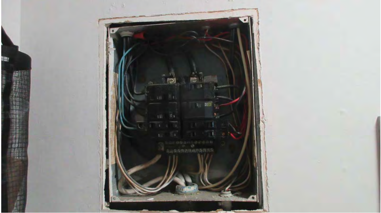
INTERIOR VIEW OF ELECTRICAL PANEL.
