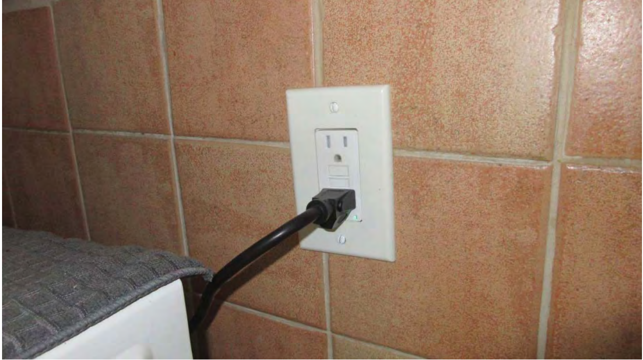
GFCI RECEPTACLE IN KITCHEN.
