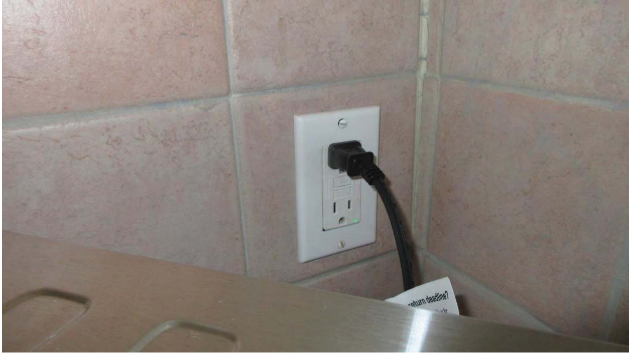
GFCI RECEPTACLE IN KITCHEN.
