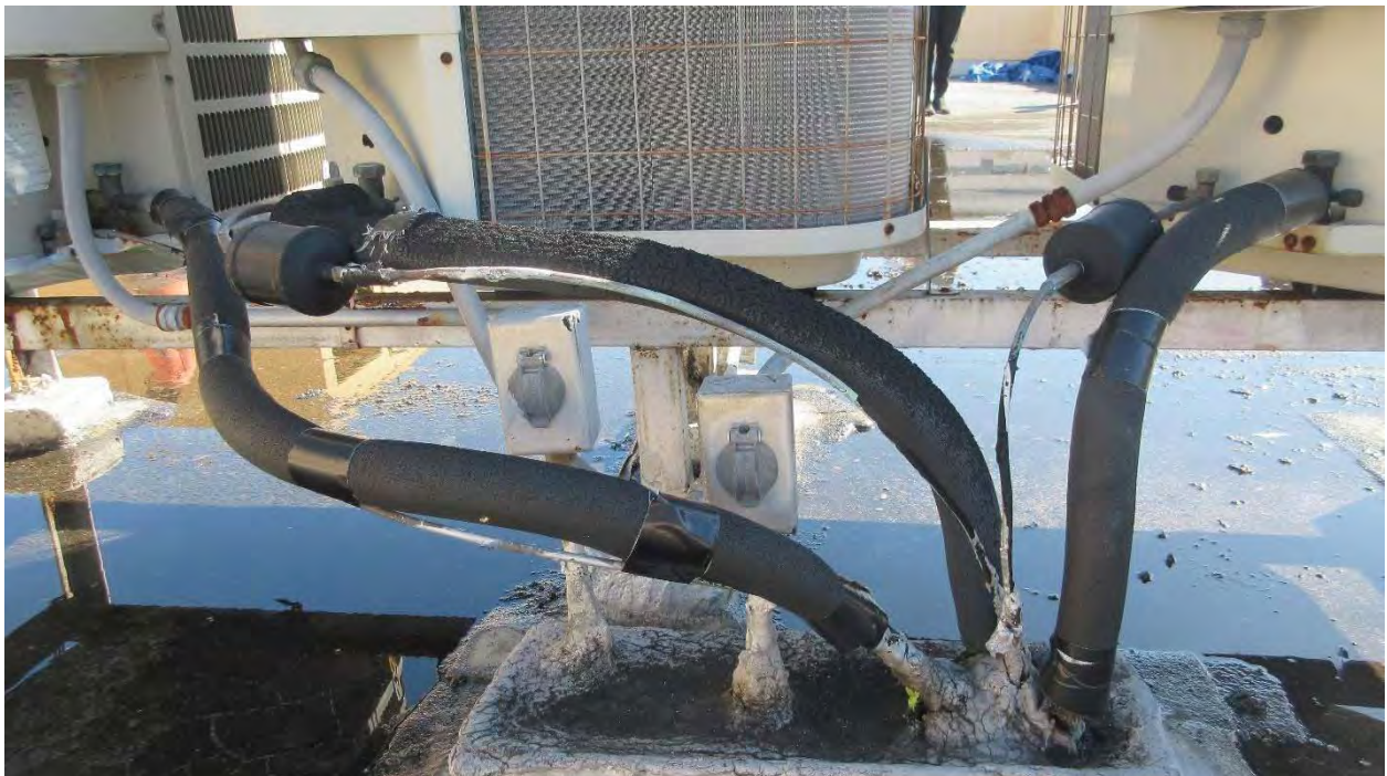
WIRING OF MECHANICAL EQUIPMENT.
