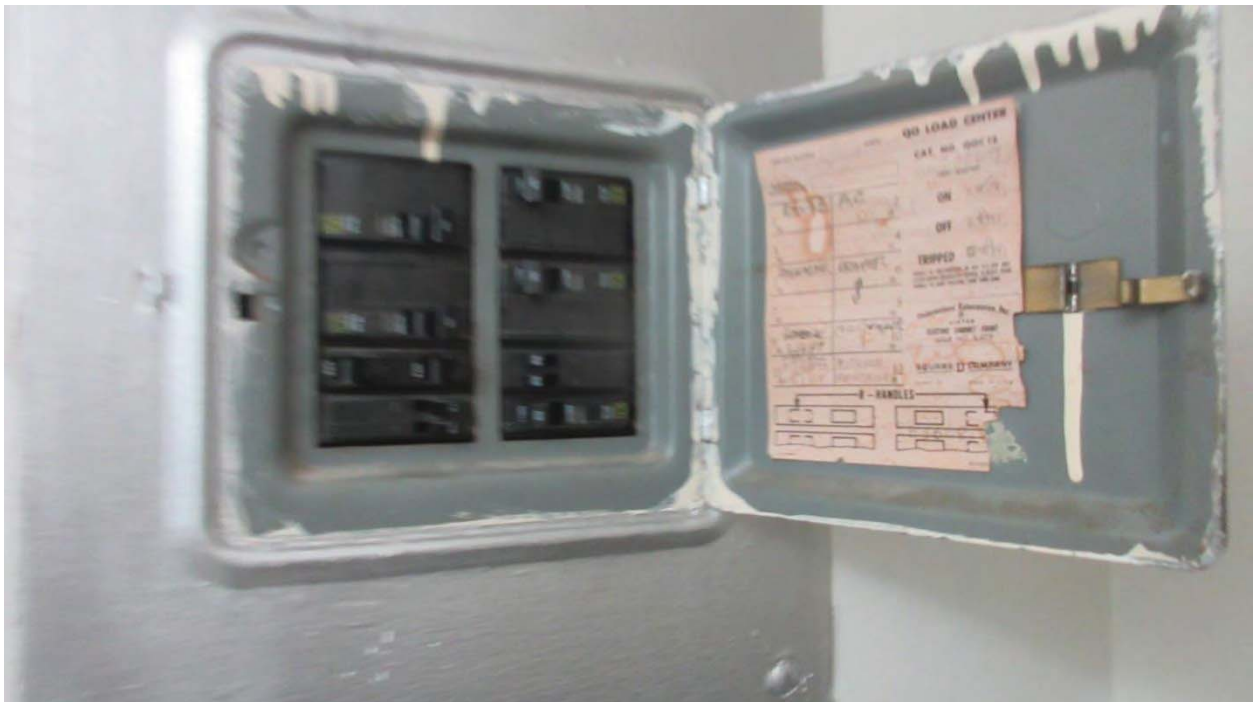
EXTERIOR VIEW OF ELECTRICAL PANEL.
