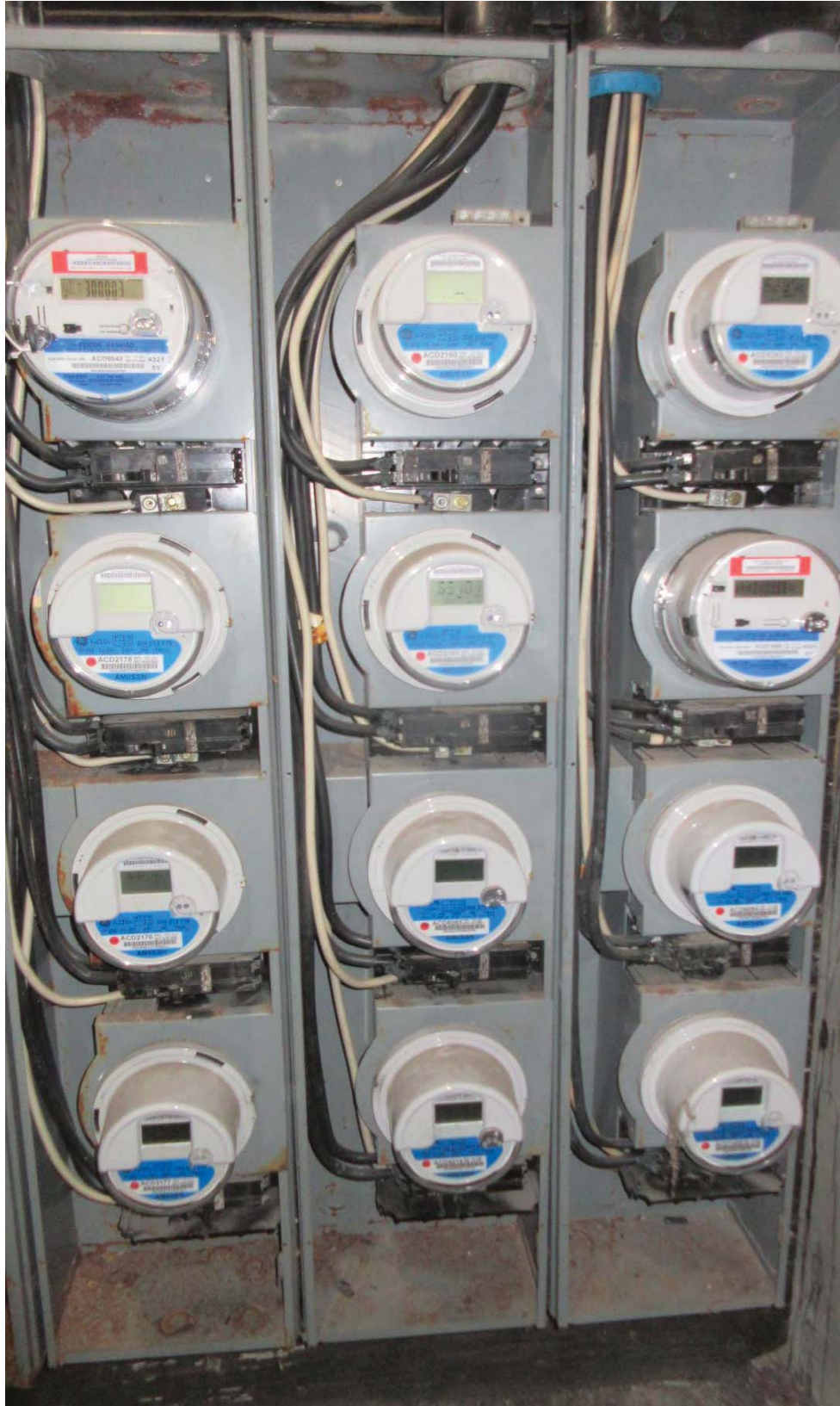
INTERIOR VIEW OF METERS STACK AND DISCONNECT BREAKERS FOR ELECTRICAL PANELS INSIDE THE APARTMENTS.
