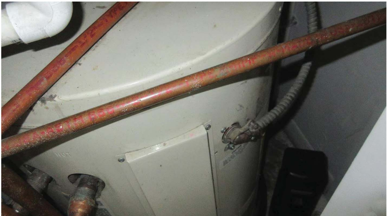
WIRING OF MECHANICAL EQUIPMENT.
