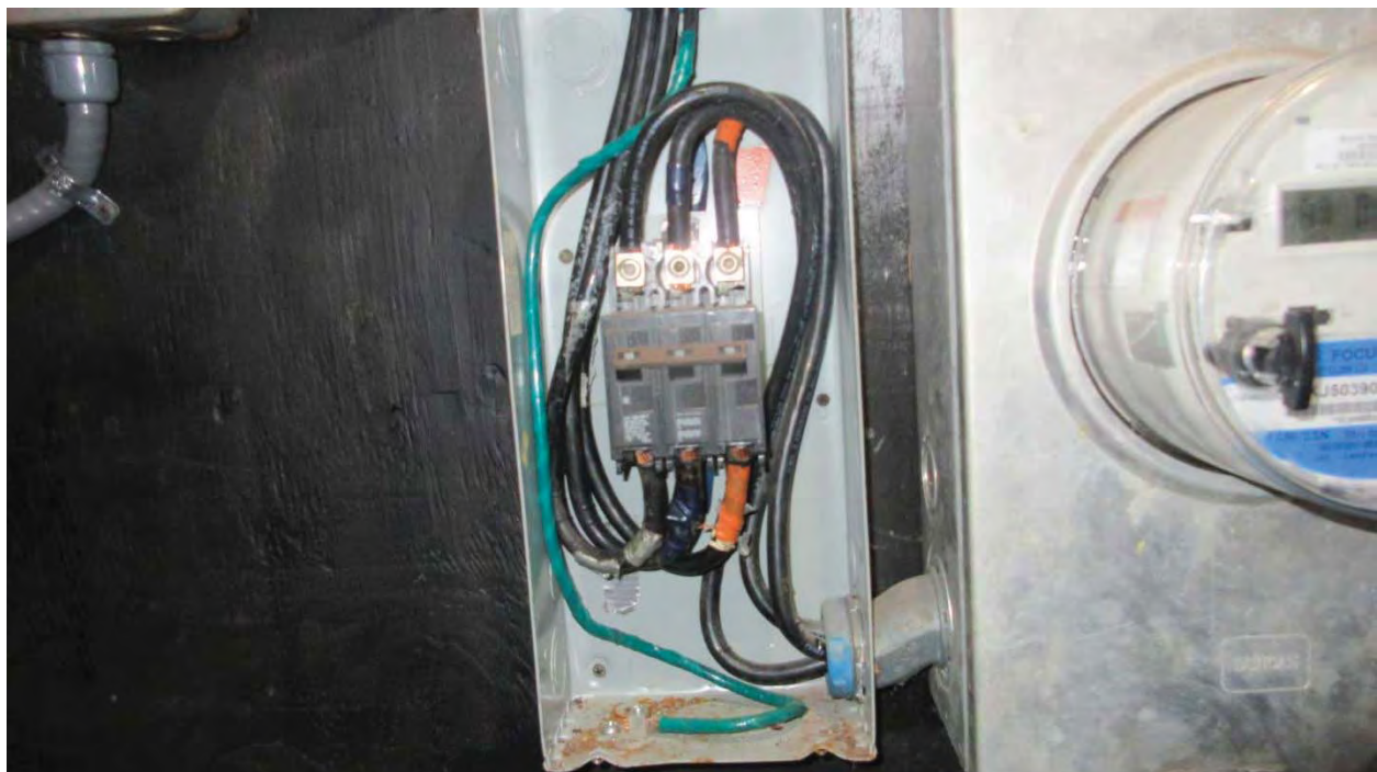
INTERIOR VIEW OF MAIN 2 OF 3 AND METER.
