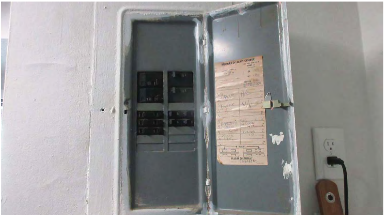
EXTERIOR VIEW OF ELECTRICAL PANEL.
