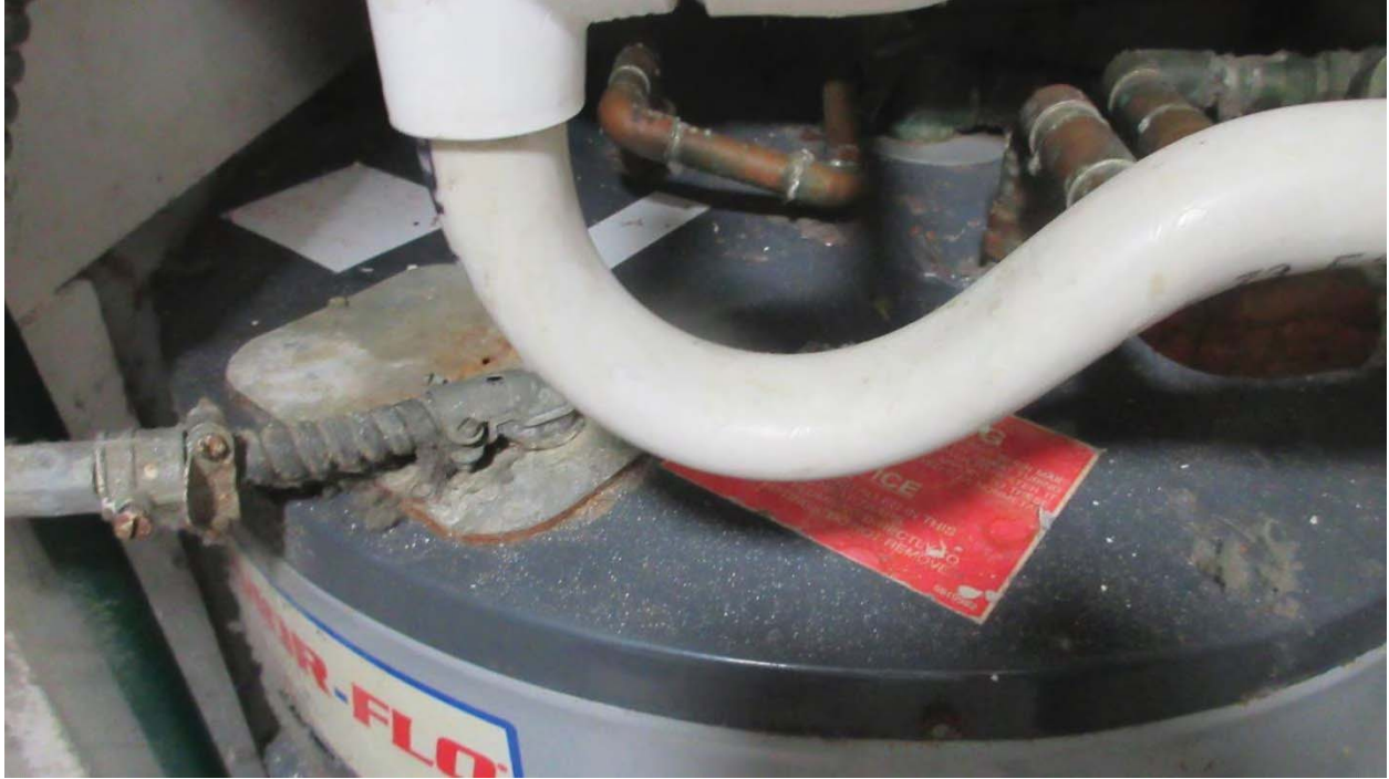
WIRING OF MECHANICAL EQUIPMENT.
