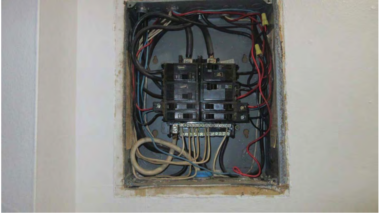
INTERIOR VIEW OF ELECTRICAL PANEL.
