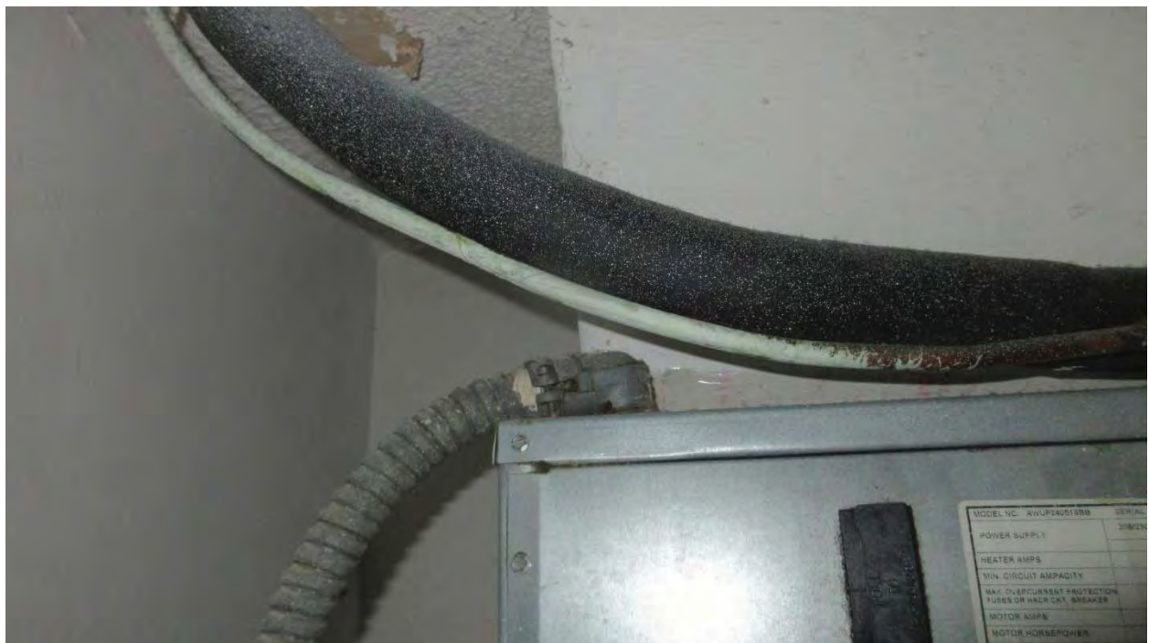
WIRING OF MECHANICAL EQUIPMENT.
