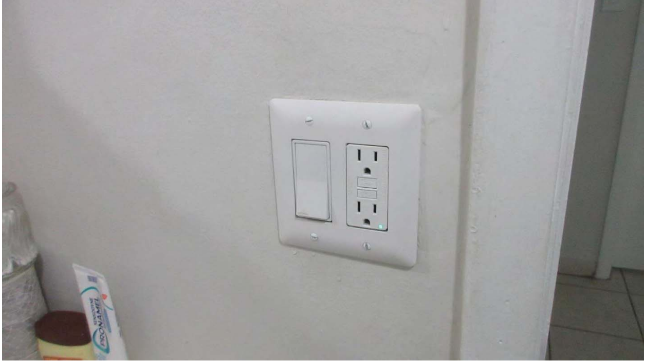
GFCI RECEPTACLE IN BATHROOM.
