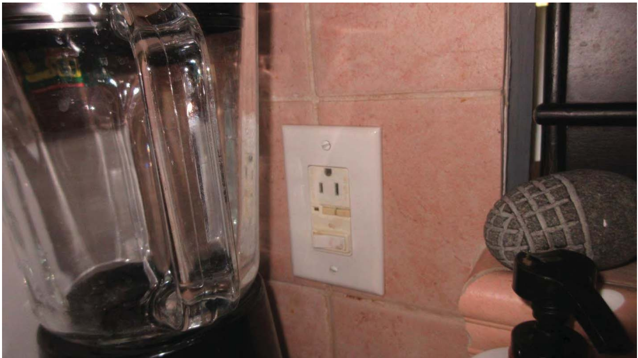
GFCI RECEPTACLE IN KITCHEN.
