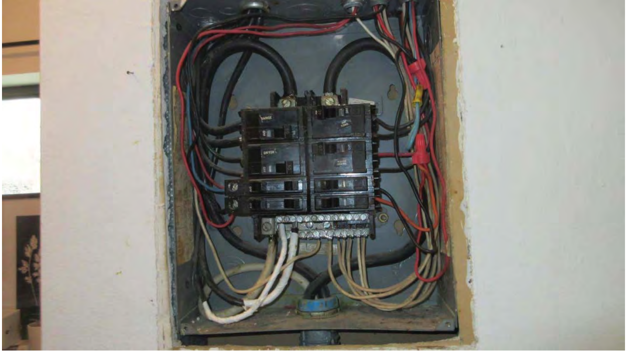
INTERIOR VIEW OF ELECTRICAL PANEL.
