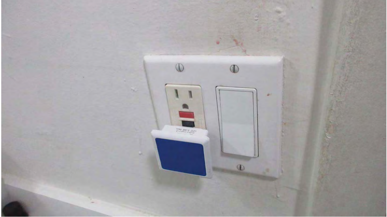
GFCI RECEPTACLE IN BATHROOM.
