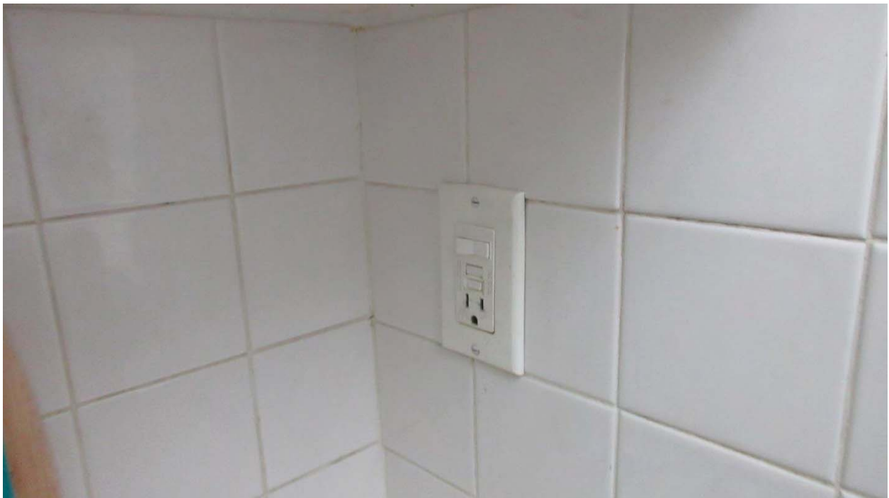
GFCI RECEPTACLE IN BATHROOM.
