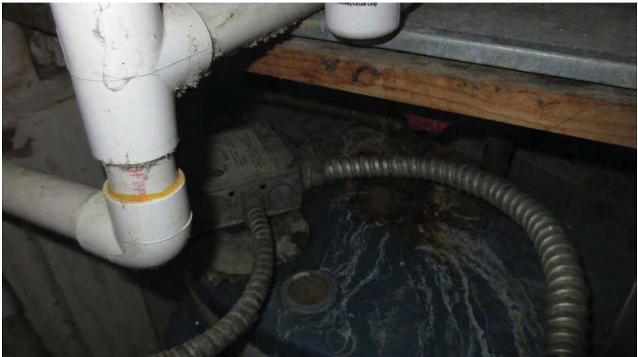
WIRING OF MECHANICAL EQUIPMENT.
