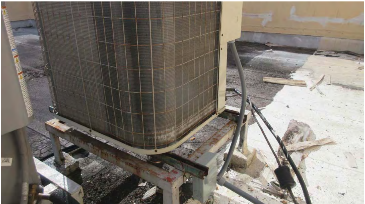
WIRING OF MECHANICAL EQUIPMENT.
