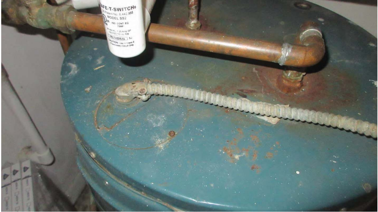
WIRING OF MECHANICAL EQUIPMENT.
