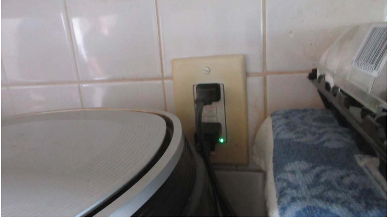
GFCI RECEPTACLE IN KITCHEN.
