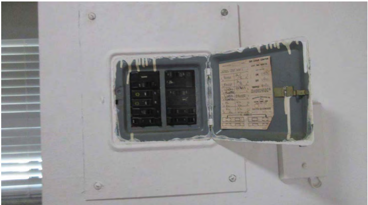
EXTERIOR VIEW OF ELECTRICAL PANEL.
