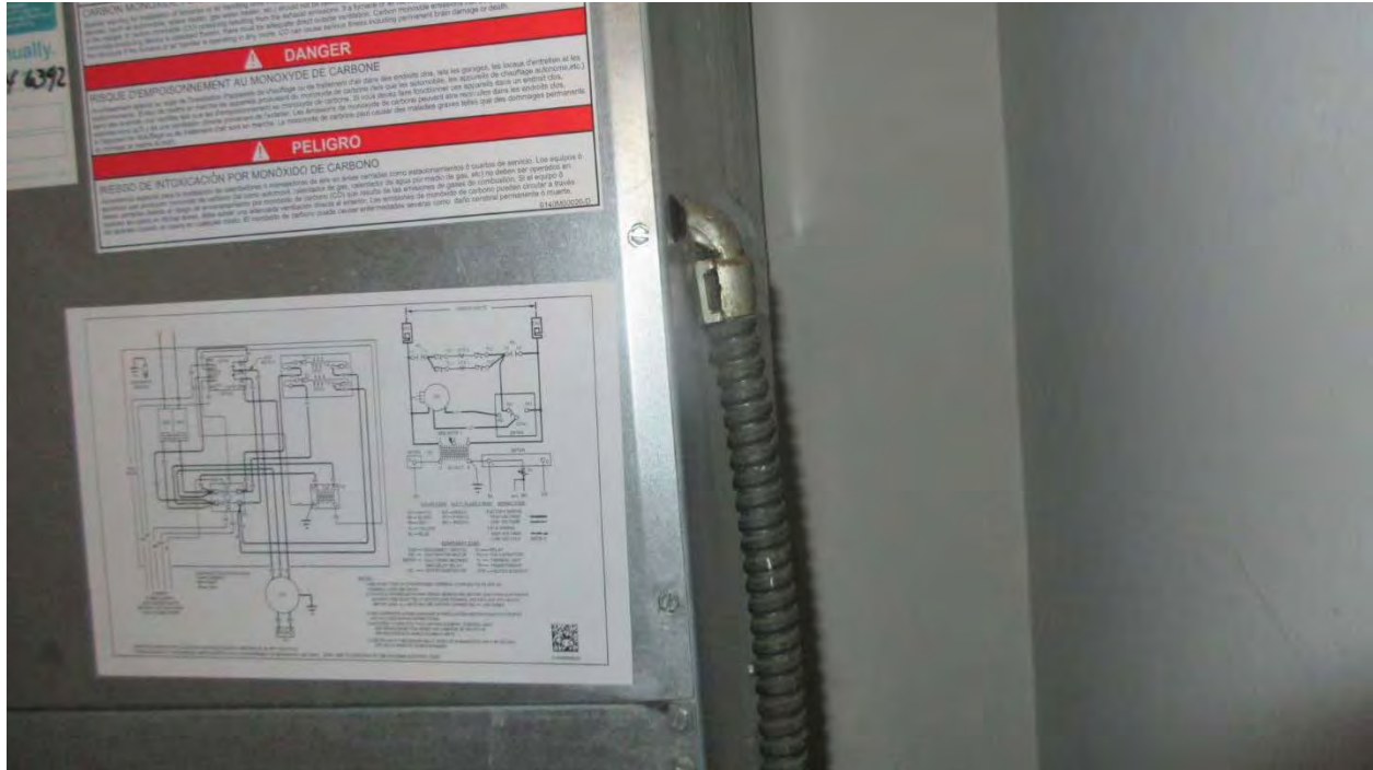
WIRING OF MECHANICAL EQUIPMENT.
