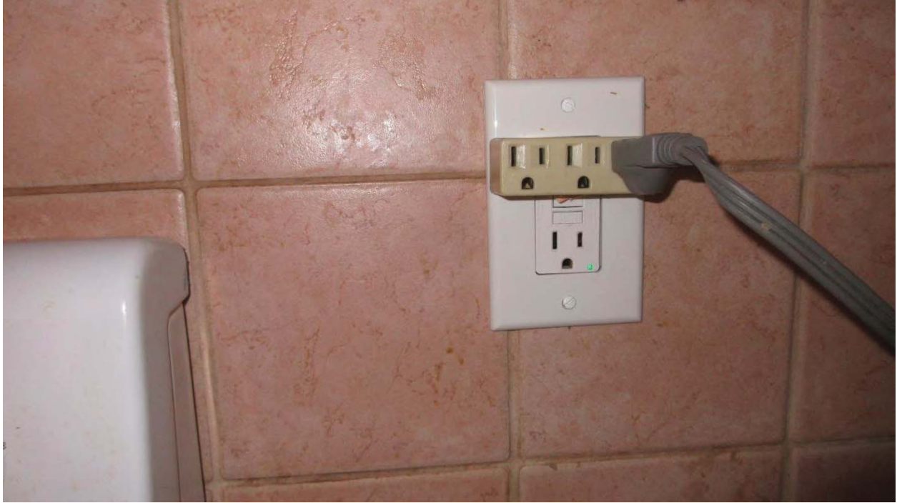
GFCI RECEPTACLE IN KITCHEN.
