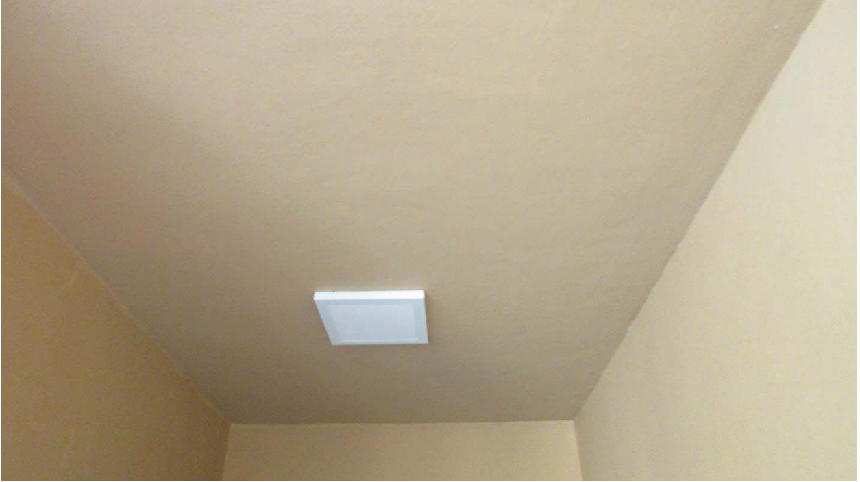
BUILDING SAFETY EGRESS ILLUMINATION.
