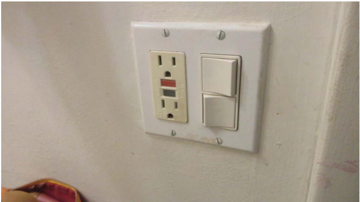
GFCI RECEPTACLE IN BATHROOM.
