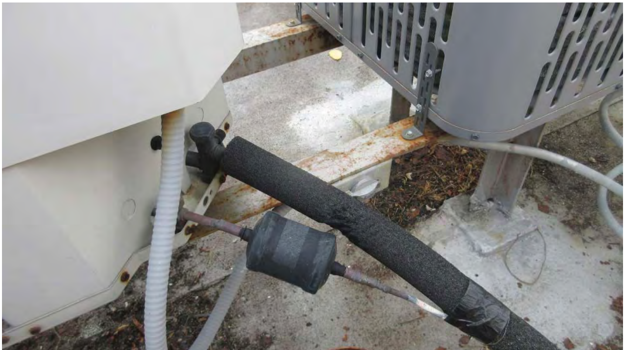
WIRING OF MECHANICAL EQUIPMENT.
