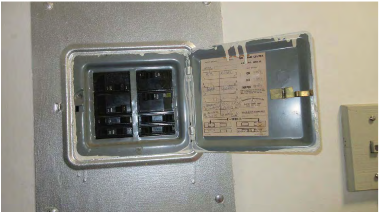
EXTERIOR VIEW OF ELECTRICAL PANEL.
