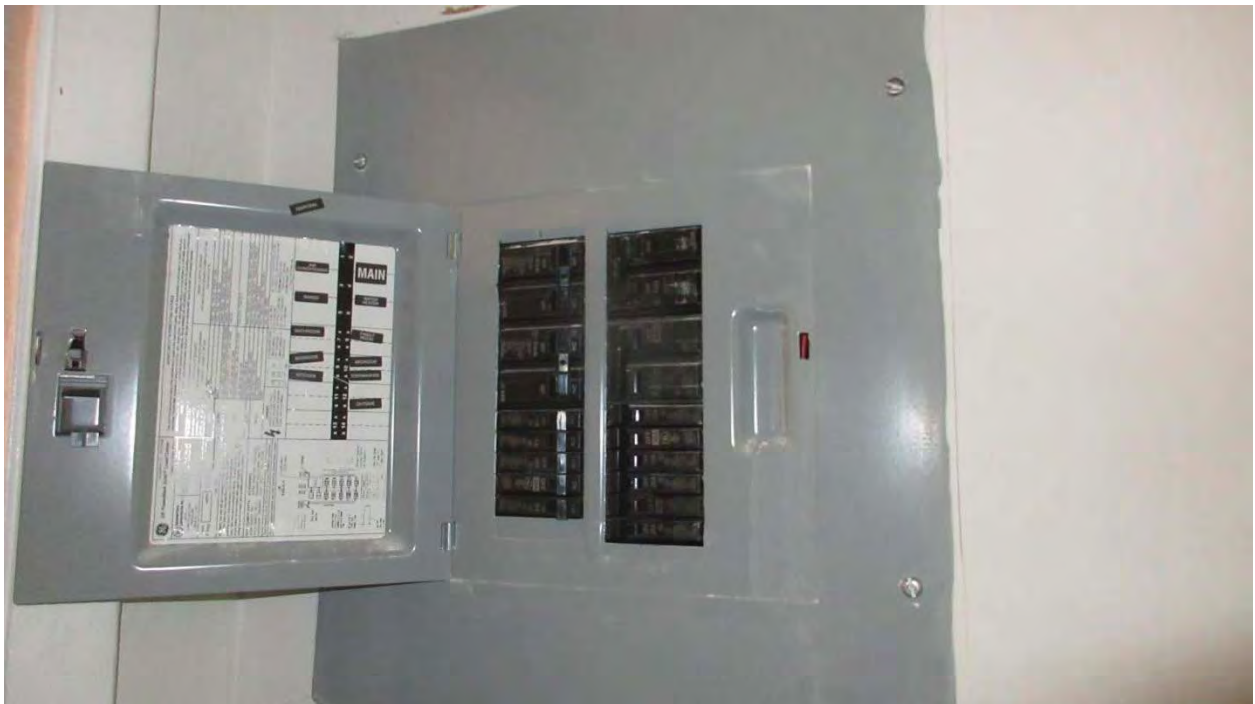
EXTERIOR VIEW OF ELECTRICAL PANEL.
