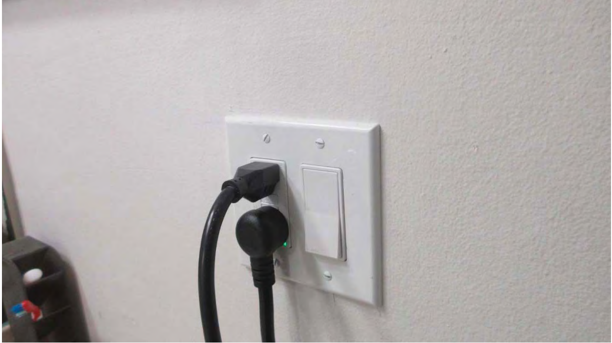
GFCI RECEPTACLE IN KITCHEN.
