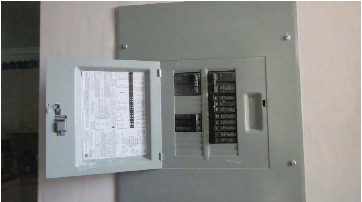
EXTERIOR VIEW OF ELECTRICAL PANEL.
