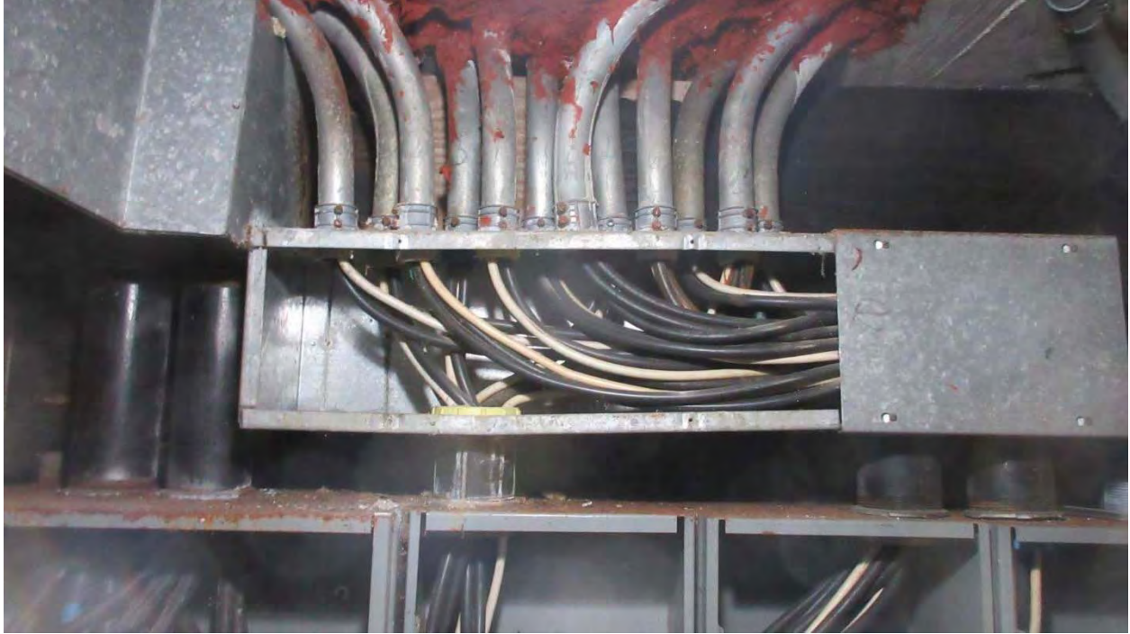
INTERIOR VIEW OF GUTTER, FEEDERS CONDUCTORS AND FEEDERS' CONDUITS.
