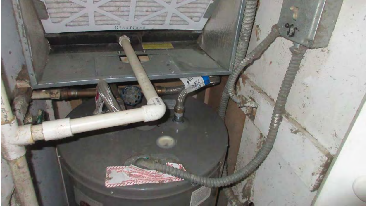
WIRING OF MECHANICAL EQUIPMENT.
