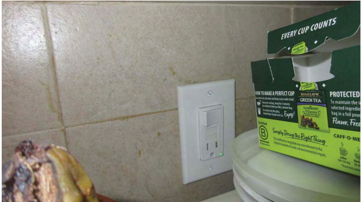
GFCI RECEPTACLE IN KITCHEN.
