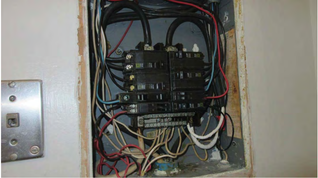
INTERIOR VIEW OF ELECTRICAL PANEL.
