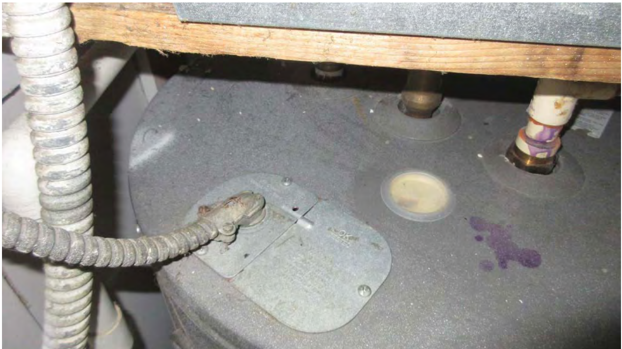
WIRING OF MECHANICAL EQUIPMENT.
