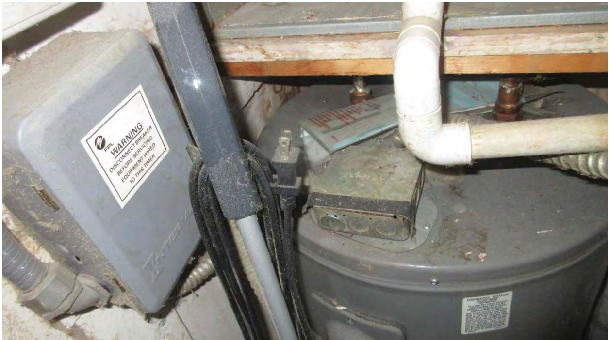
WIRING OF MECHANICAL EQUIPMENT.
