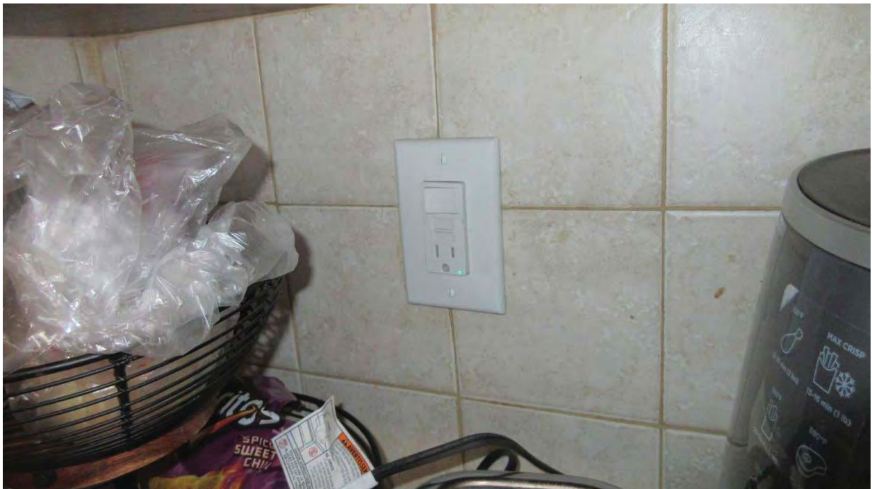
GFCI RECEPTACLE IN KITCHEN.
