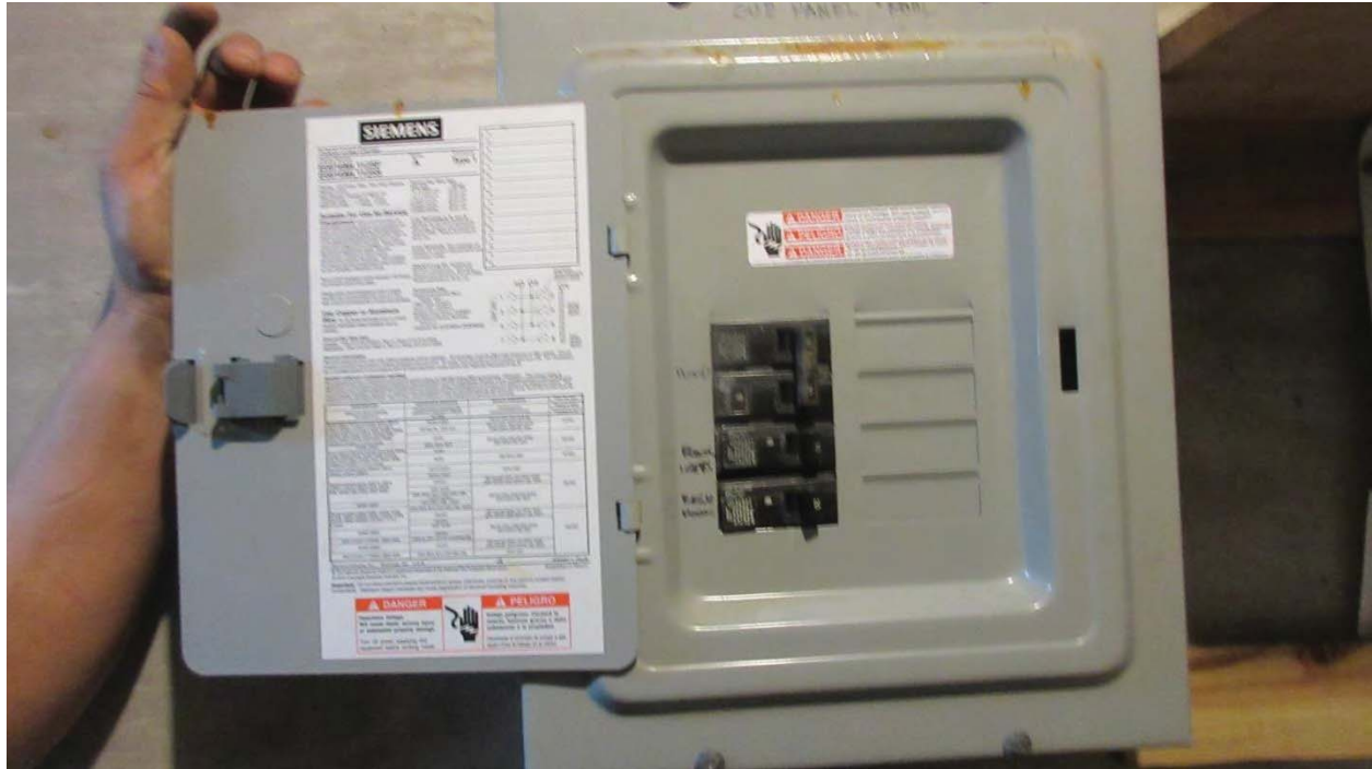
EXTERIOR VIEW OF SUB-PANEL "POOL"
