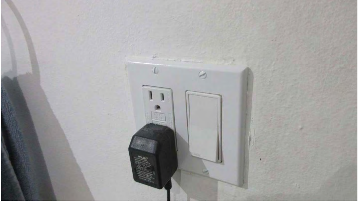
GFCI RECEPTACLE IN BATHROOM.
