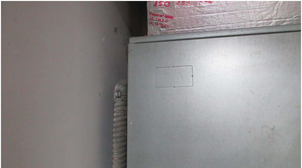
WIRING OF MECHANICAL EQUIPMENT.
