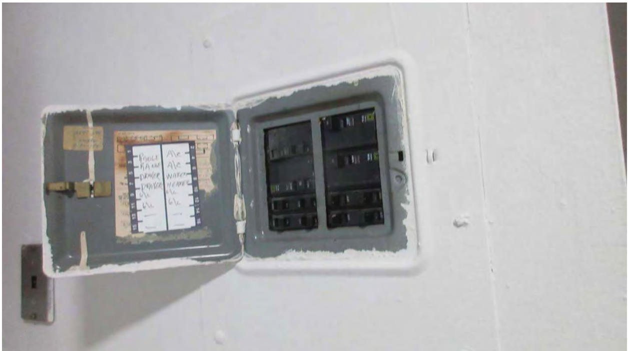
EXTERIOR VIEW OF ELECTRICAL PANEL.
