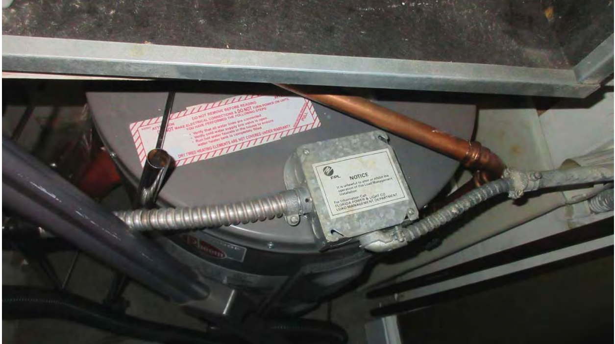
WIRING OF MECHANICAL EQUIPMENT.
