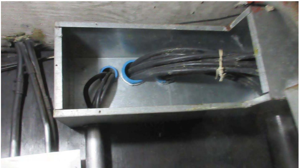
INTERIOR VIEW OF GUTTER AND SERVICE CONDUCTORS.
