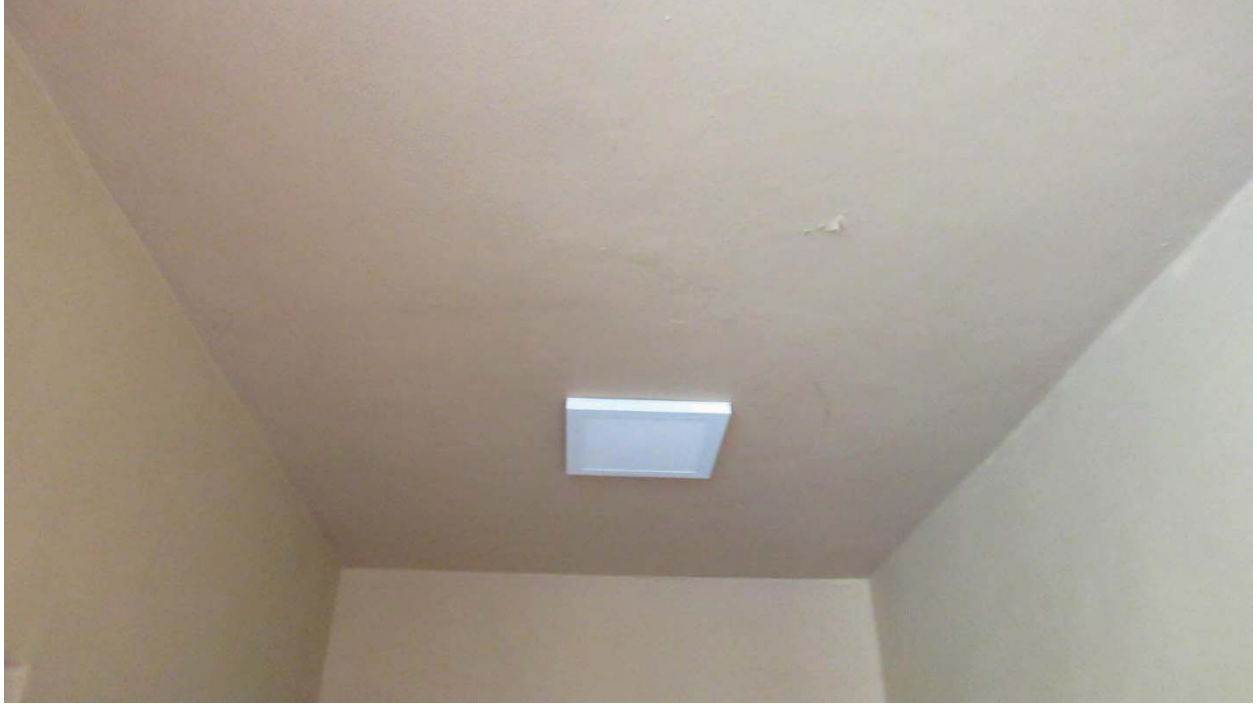
BUILDING SAFETY EGRESS ILLUMINATION.
