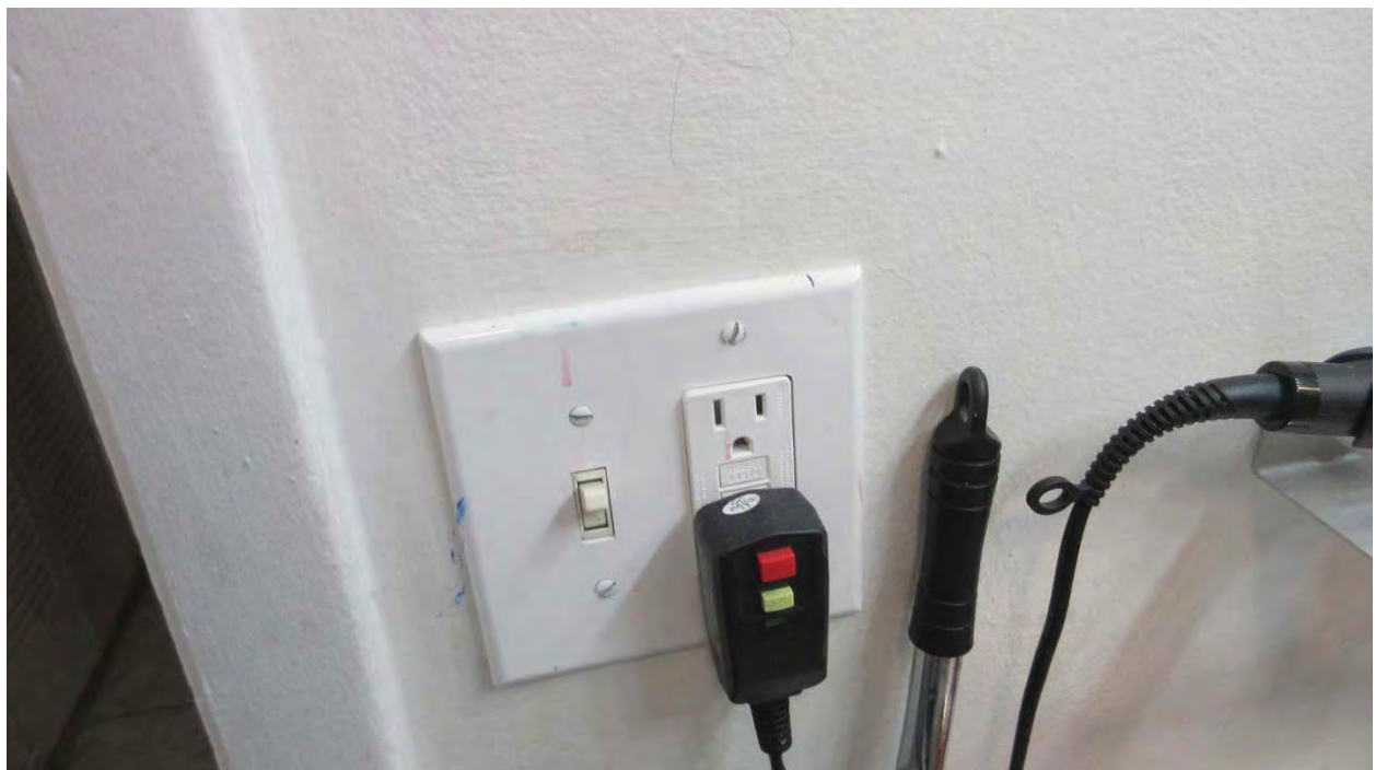
GFCI RECEPTACLE IN BATHROOM.
