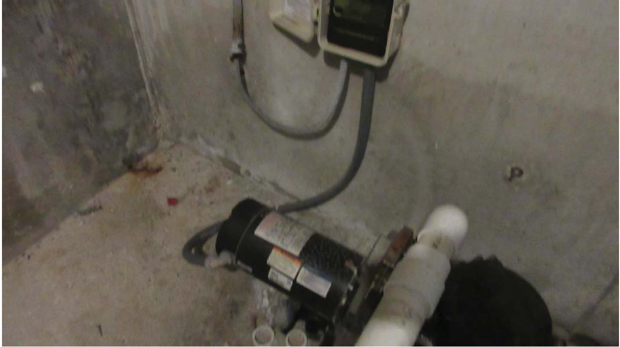
VIEW OF WIRING OF POOL PUMP INSIDE THE POOL EQUIPMENT ROOM.
