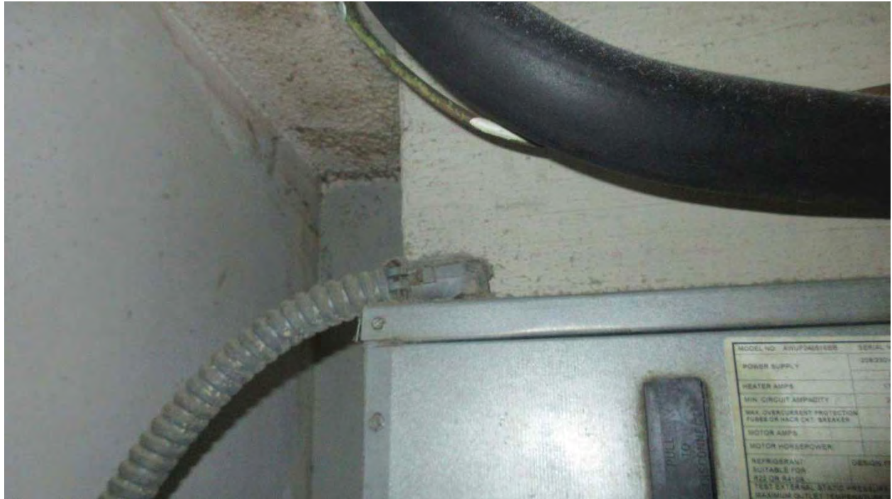
WIRING OF MECHANICAL EQUIPMENT.
