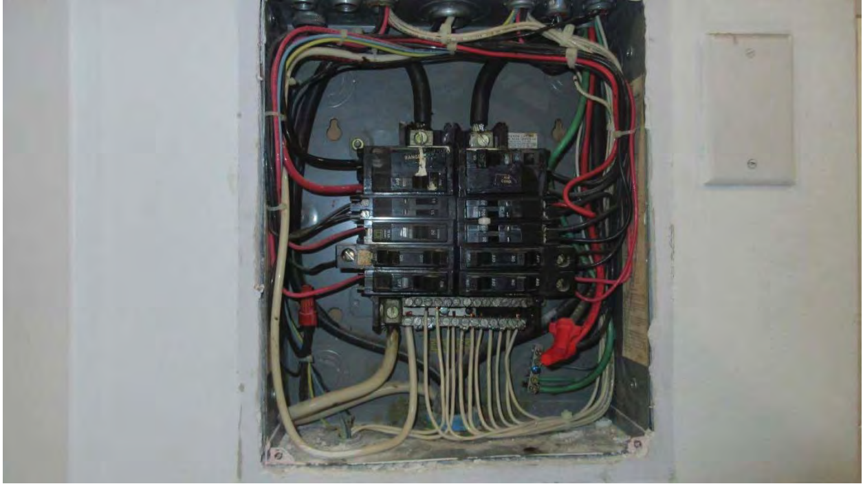
INTERIOR VIEW OF ELECTRICAL PANEL.
