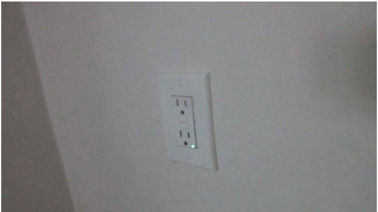
GFCI RECEPTACLE IN BATHROOM.
