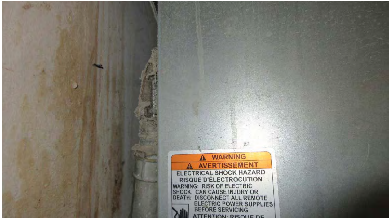
WIRING OF MECHANICAL EQUIPMENT.
