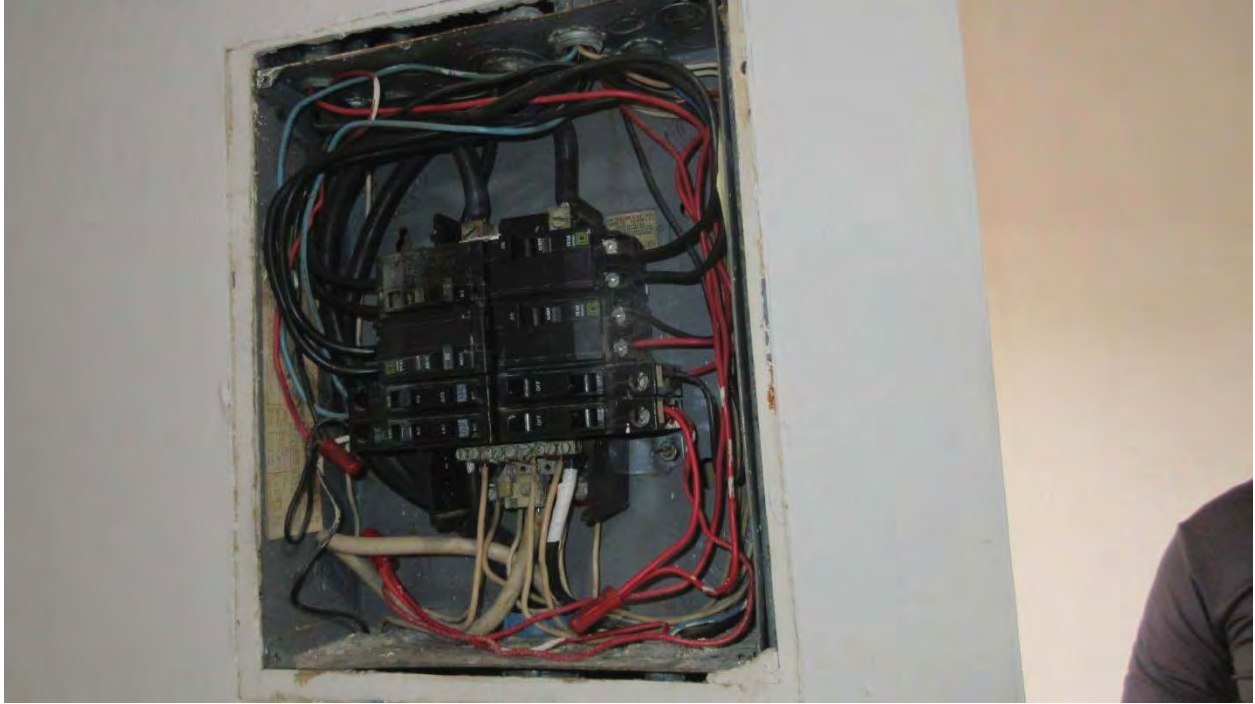
INTERIOR VIEW OF ELECTRICAL PANEL.
