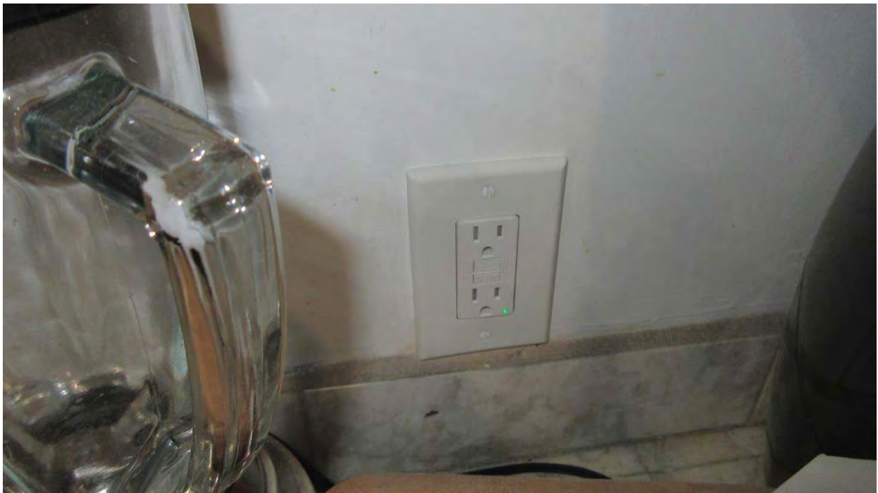
GFCI RECEPTACLE IN KITCHEN.
