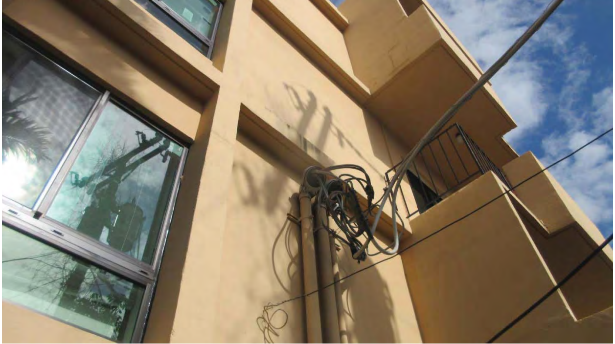
VIEW OF ELECTRICAL SERVICE.
