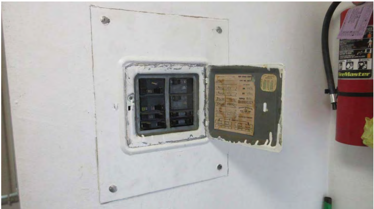
EXTERIOR VIEW OF ELECTRICAL PANEL.
