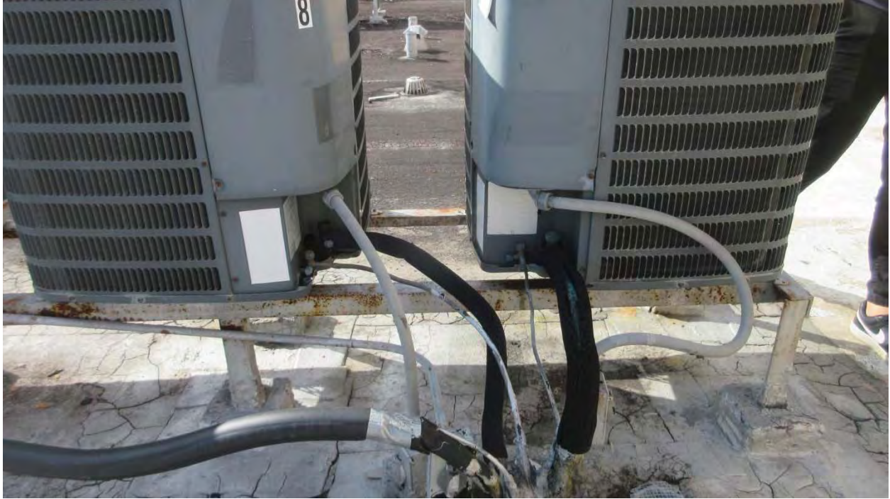
WIRING OF MECHANICAL EQUIPMENT.
