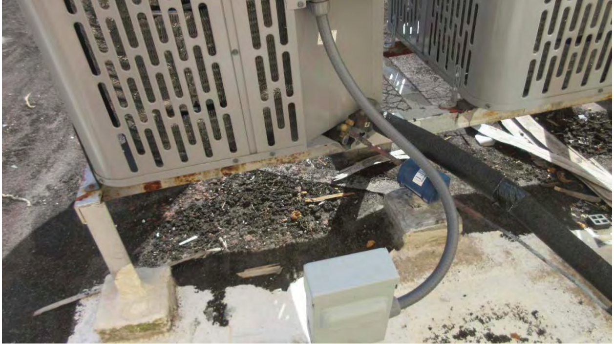
WIRING OF MECHANICAL EQUIPMENT.
