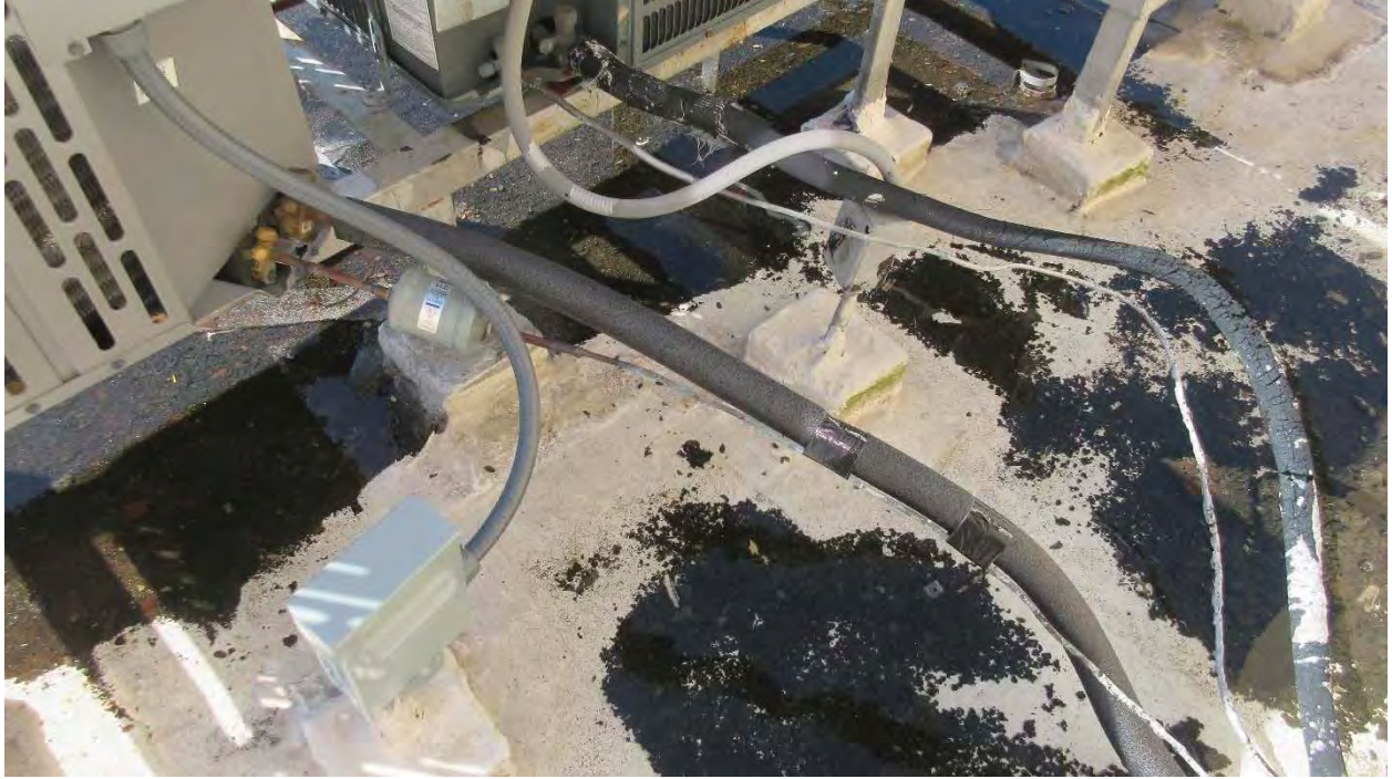
WIRING OF MECHANICAL EQUIPMENT.
