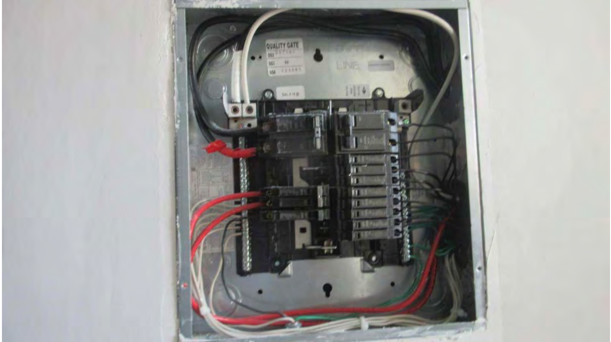
INTERIOR VIEW OF ELECTRICAL PANEL.
