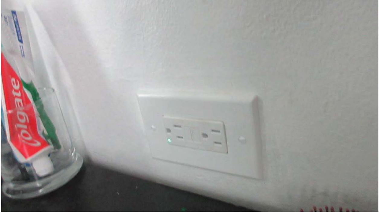
GFCI RECEPTACLE IN BATHROOM.
