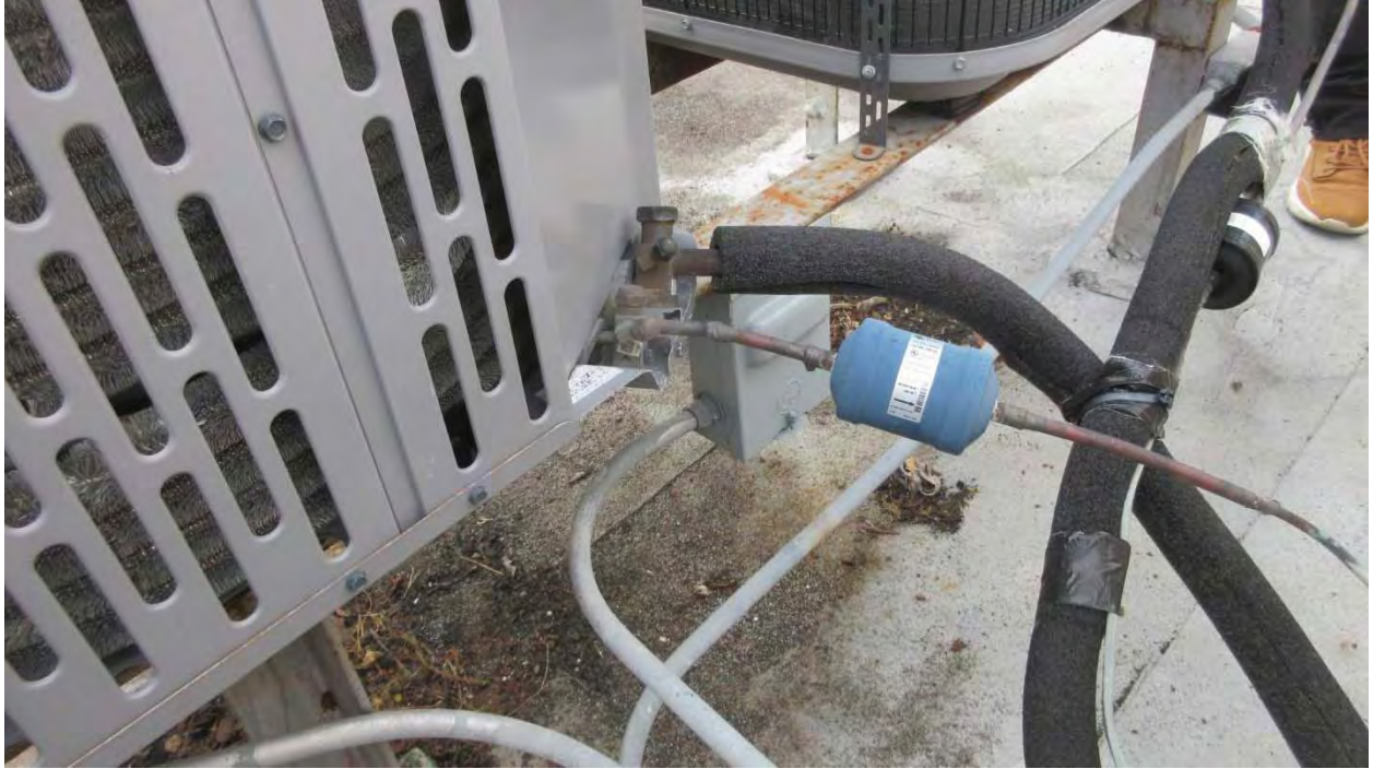
WIRING OF MECHANICAL EQUIPMENT.
