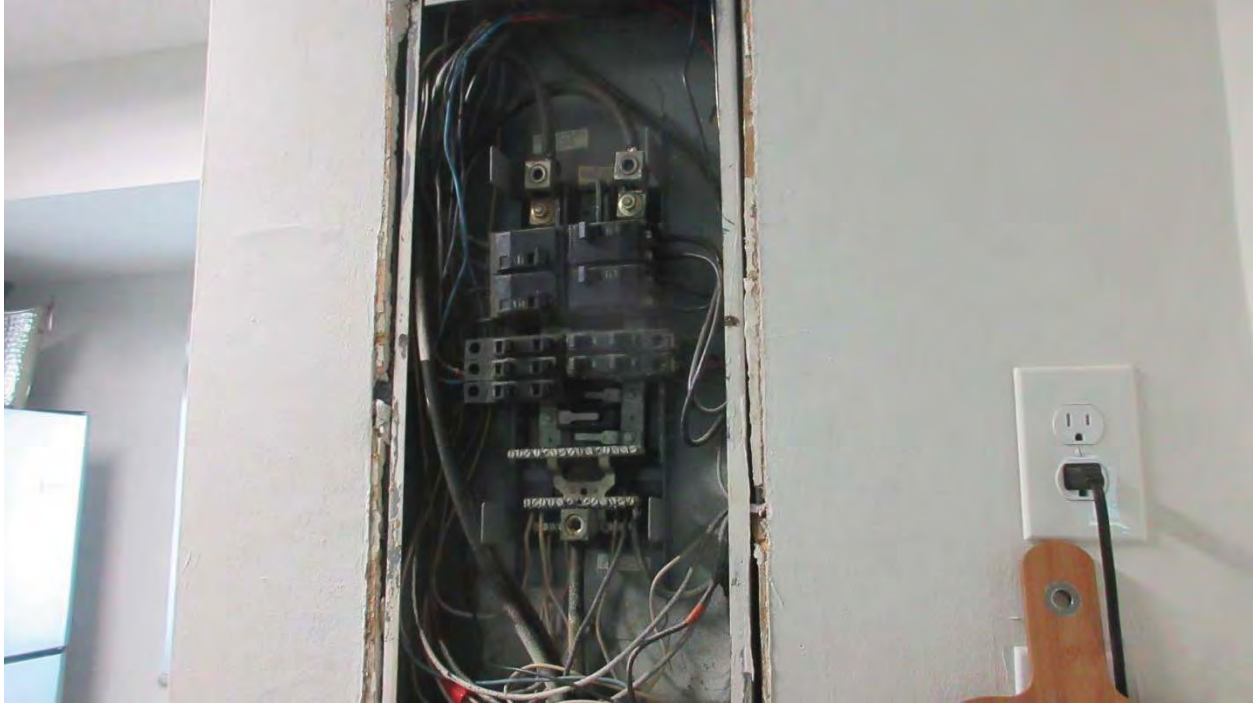
INTERIOR VIEW OF ELECTRICAL PANEL.
