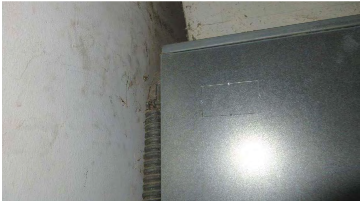
WIRING OF MECHANICAL EQUIPMENT.
