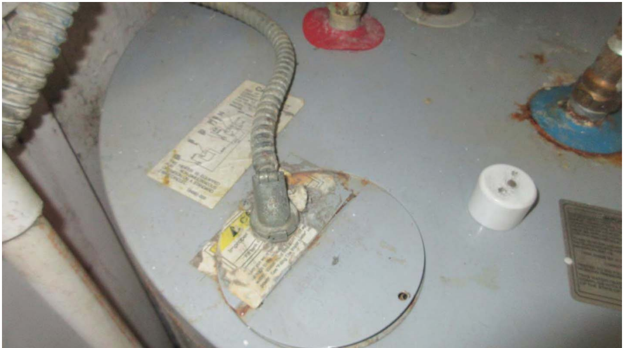
WIRING OF MECHANICAL EQUIPMENT.
