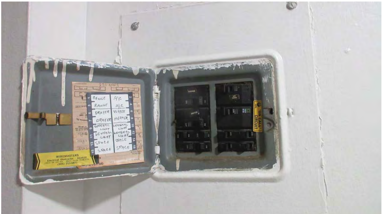
EXTERIOR VIEW OF ELECTRICAL PANEL.
