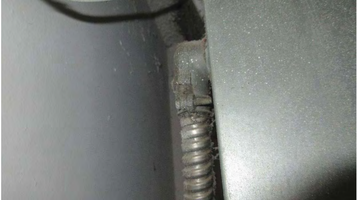
WIRING OF MECHANICAL EQUIPMENT.
