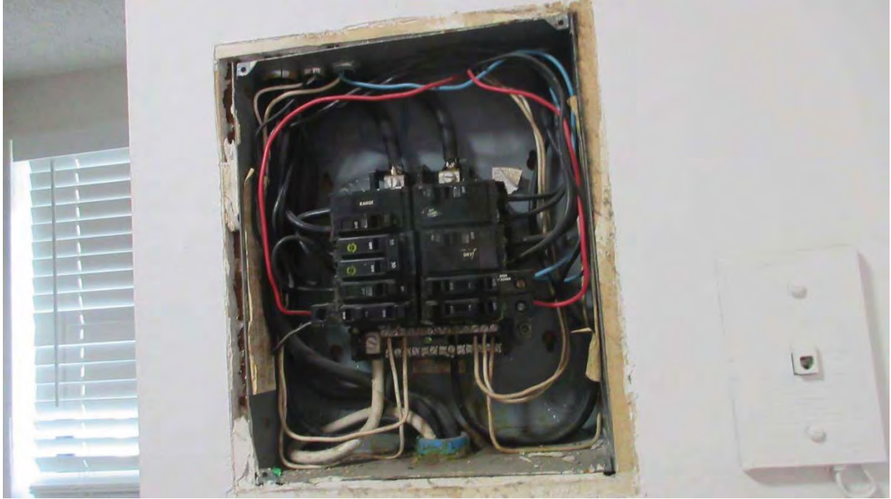
INTERIOR VIEW OF ELECTRICAL PANEL.
