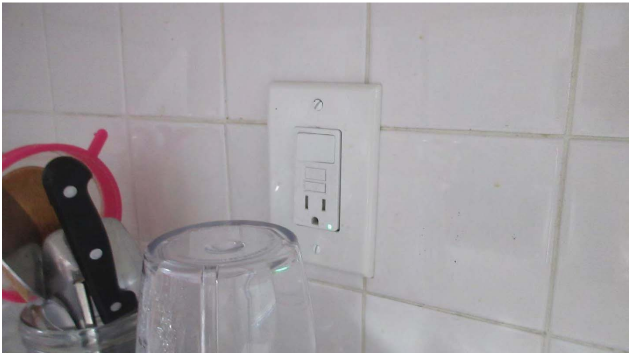
GFCI RECEPTACLE IN KITCHEN.
