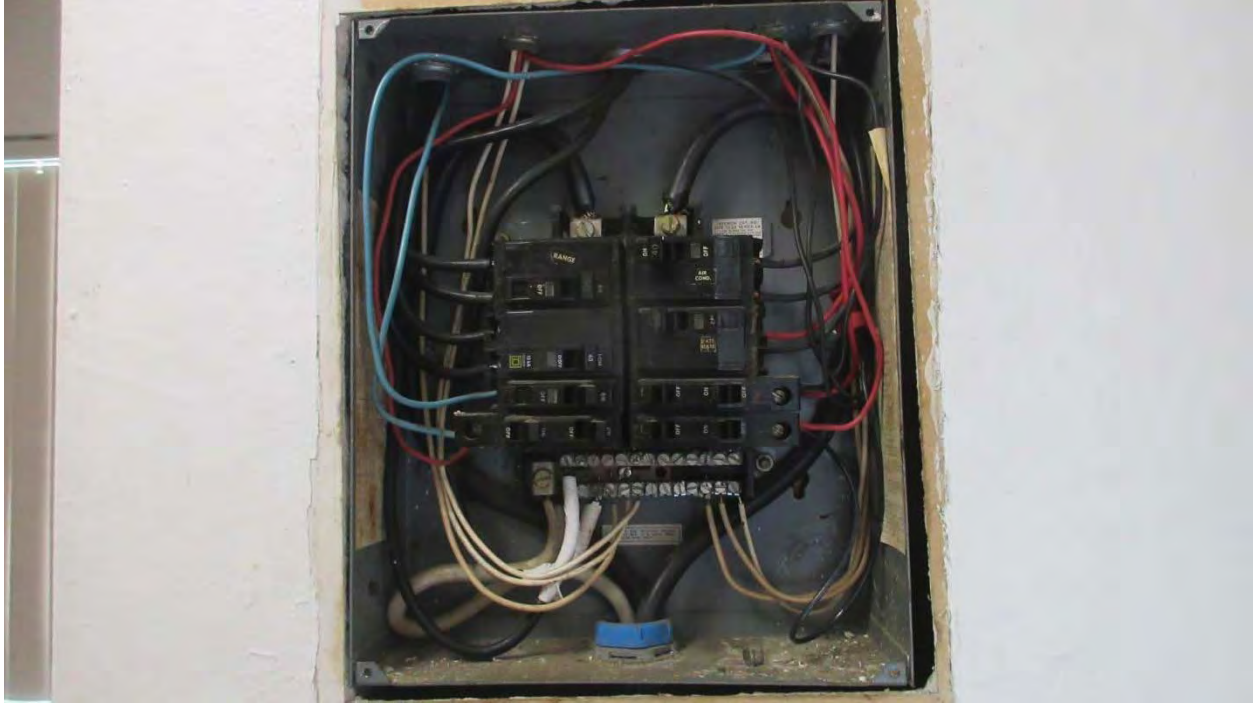
INTERIOR VIEW OF ELECTRICAL PANEL.
