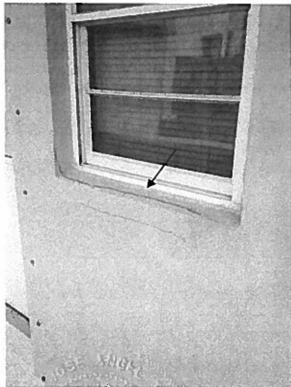
Photograph No. 4 (typical spalling at window sill)
