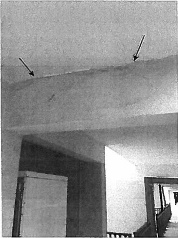
Photograph No. 5 (typical beam spalling)
