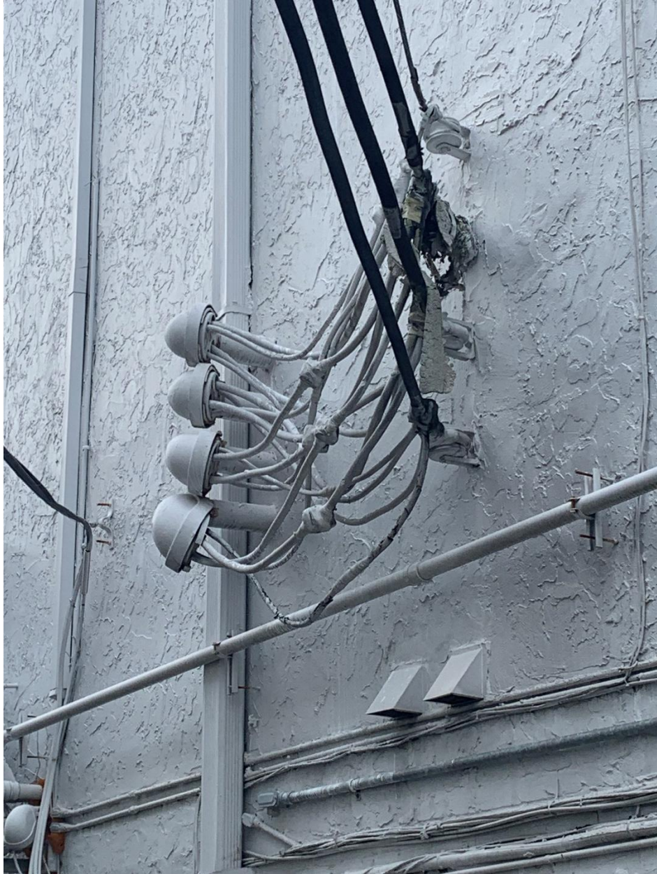
Electrical Photo 3 – 6915 S. Red Road – Electrical Service
