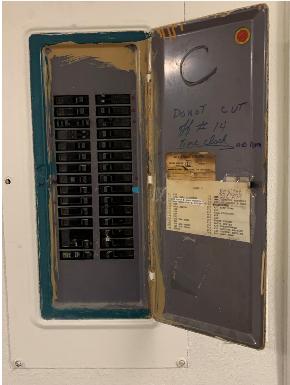
Electrical Photo 8 – 6915 S. Red Road – Electrical Panels
