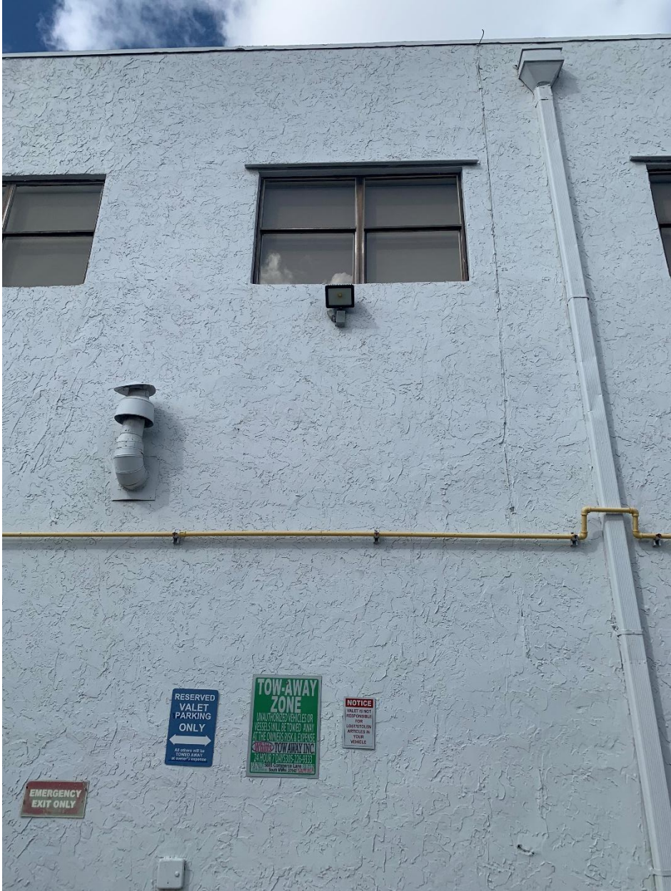
Electrical Photo 19 – 6915 S. Red Road – Egress Illumination
