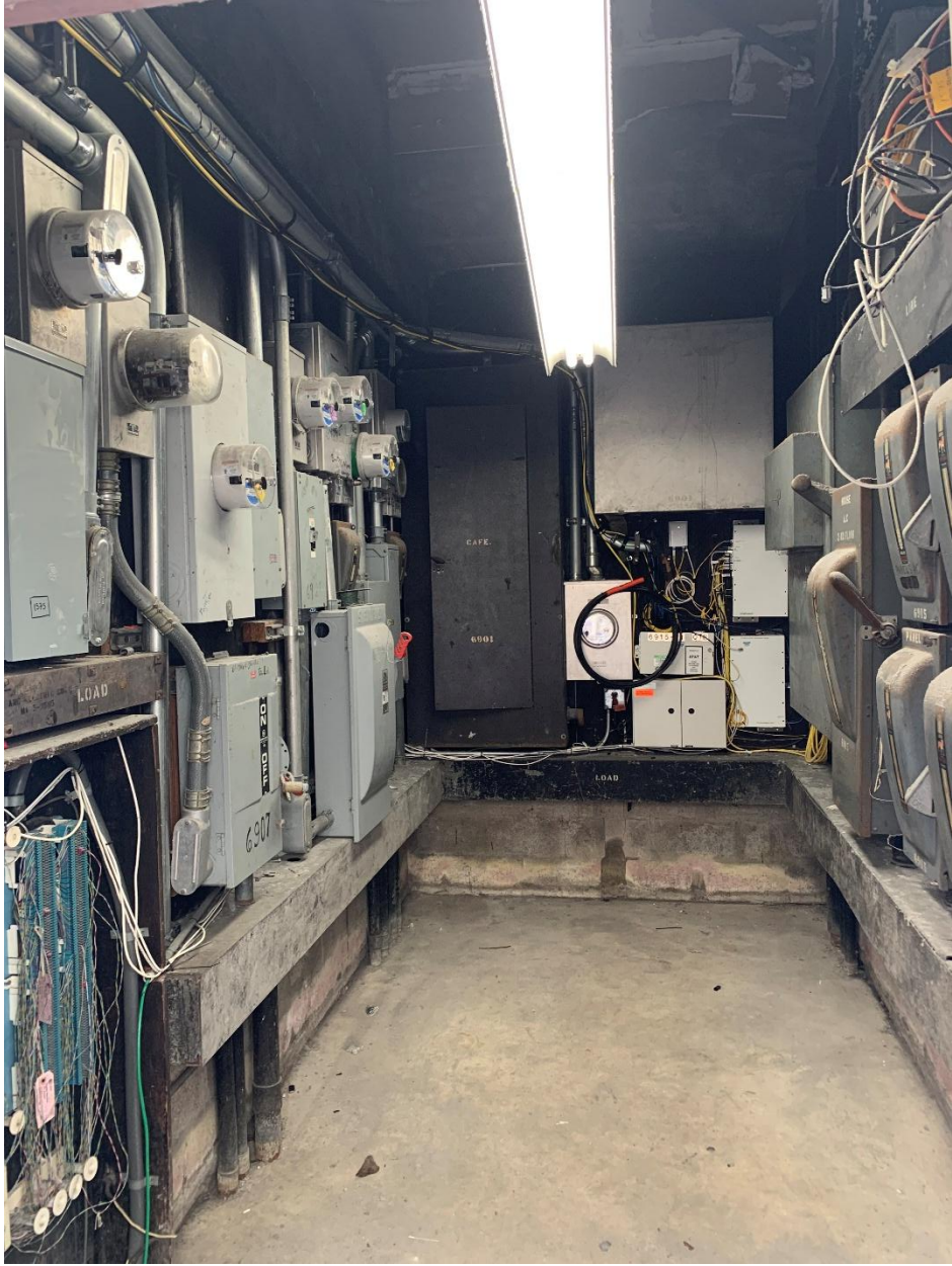
Electrical Photo 5 – 6915 S. Red Road – Electric Room
