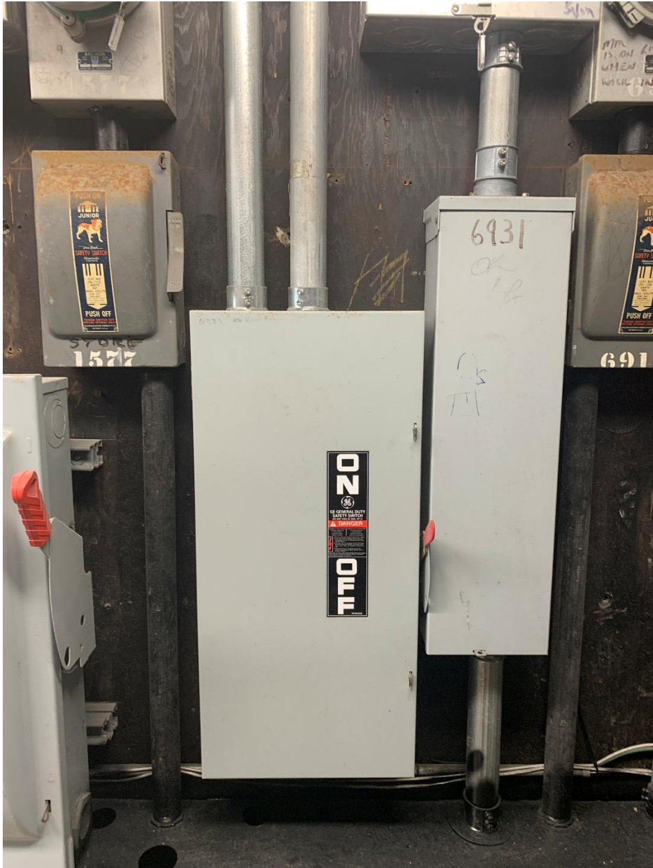
Electrical Photo 12 – 6915 S. Red Road – Raceways
