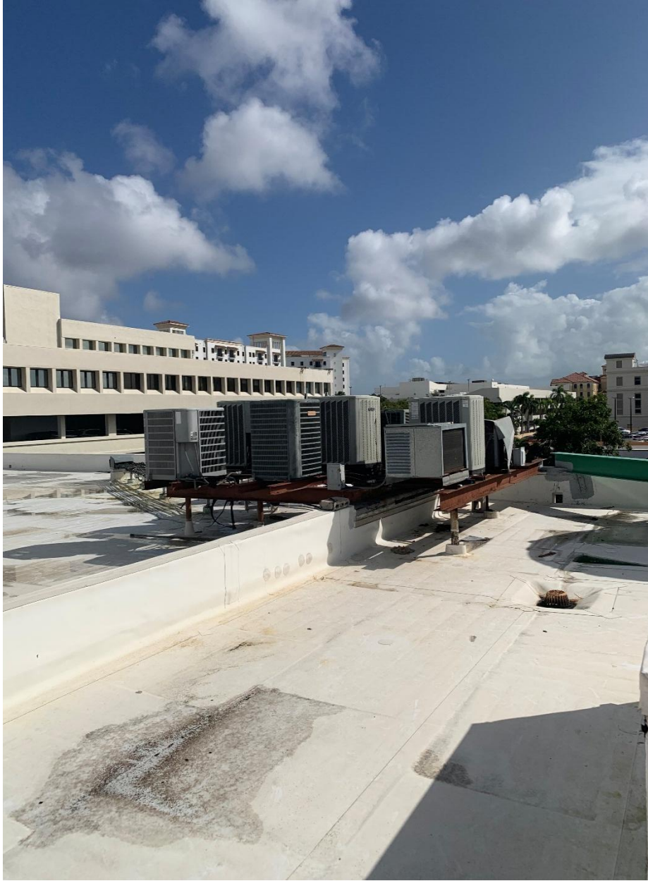
Structural Photo 7a2 – 6915 S. Red Road – Air Conditioning Equipment on Roof
