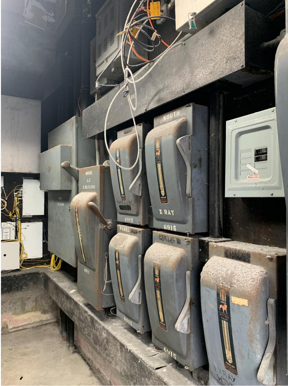
Electrical Photo 6 – 6915 S. Red Road – Gutters
