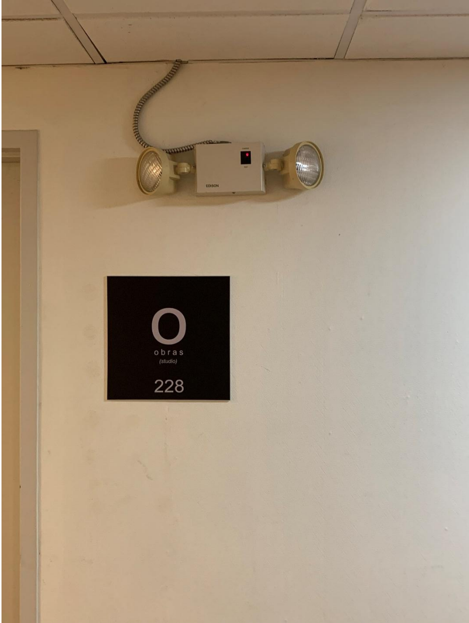
Electrical Photo 18 – 6915 S. Red Road – Emergency Lighting
