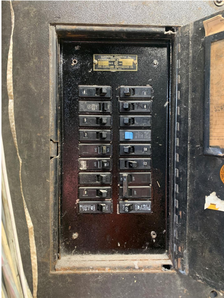
Electrical Photo 7 (1) – 6915 S. Red Road – Electrical Panels
