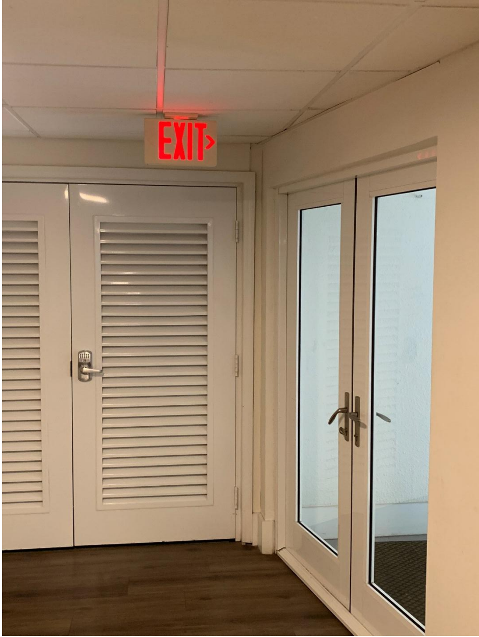
Electrical Photo 22 – 6915 S. Red Road – Exit Light
