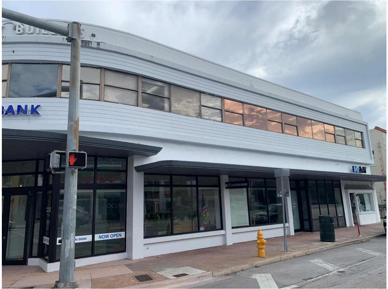
Structural Photo 10 (2) – 6915 S. Red Road – Windows and Storefronts
