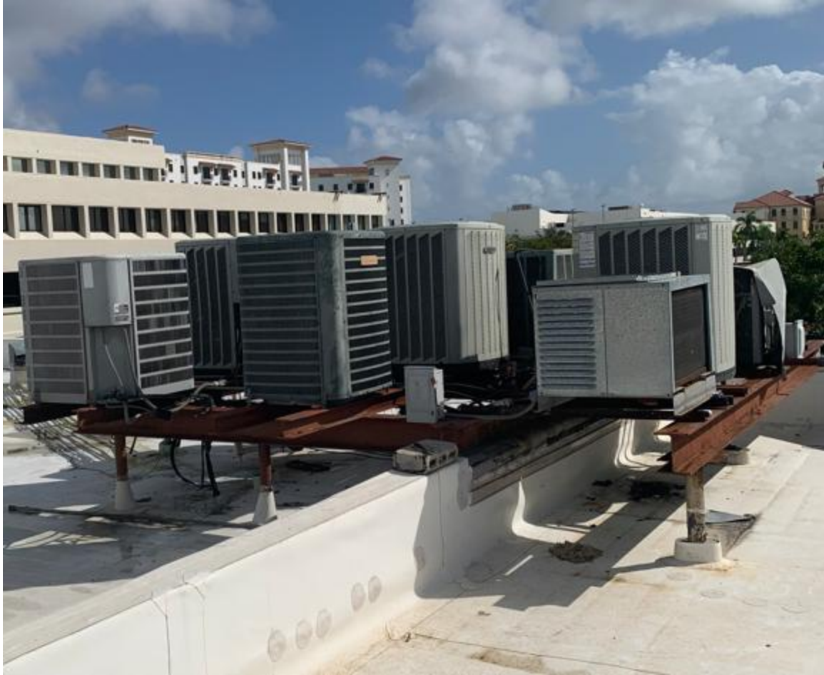
Electrical Photo 27 – 6915 S. Red Road – Wiring to Mechanical Equipment
