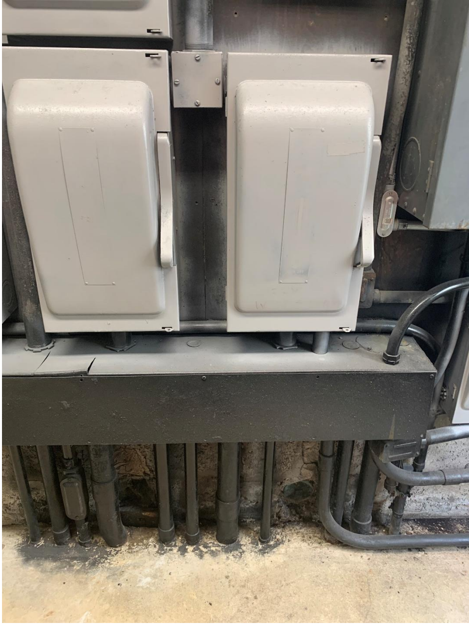
Electrical Photo 9 – 6915 S. Red Road – Grounding
