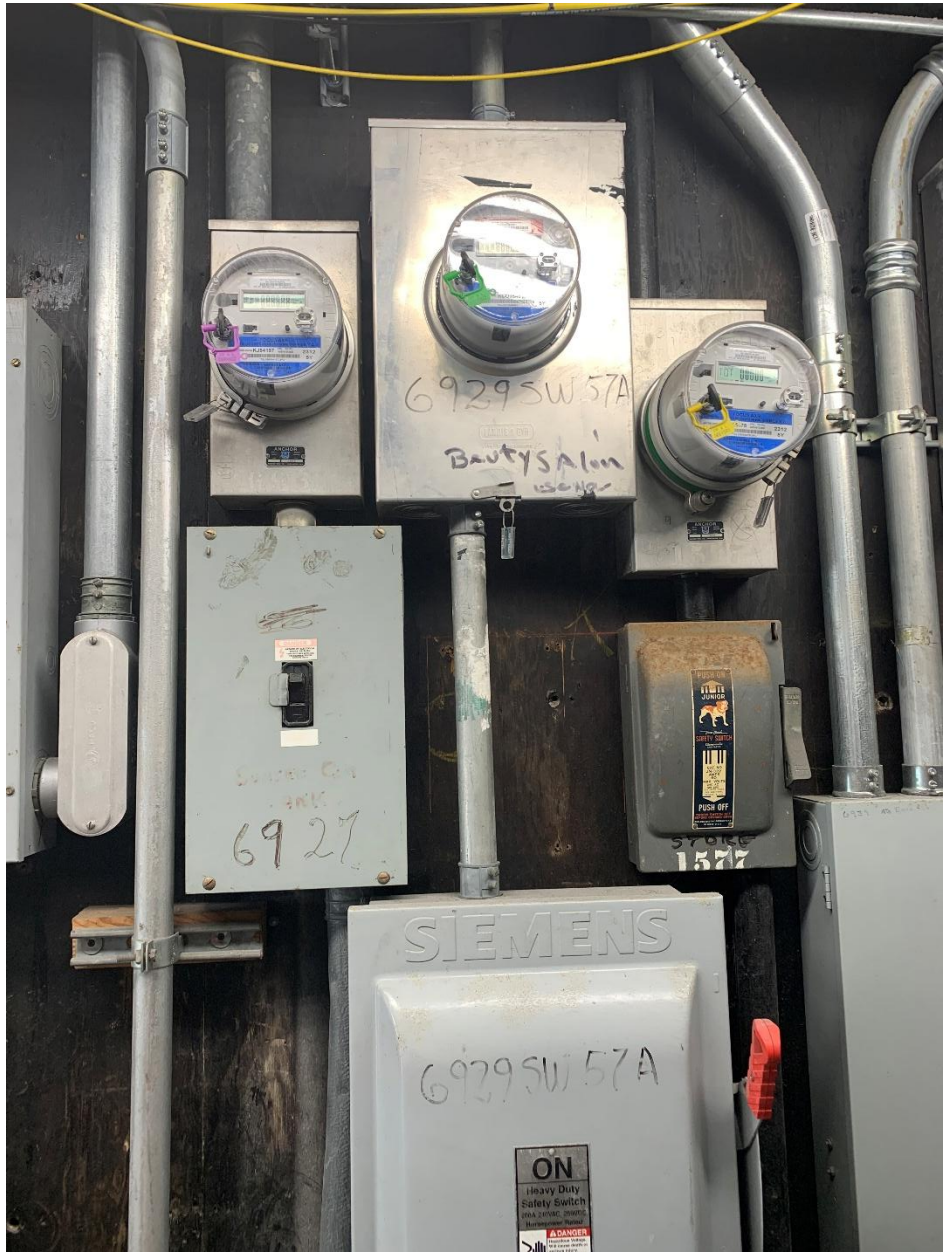
Electrical Photo 4 (3) – 6915 S. Red Road – Metering Equipment
