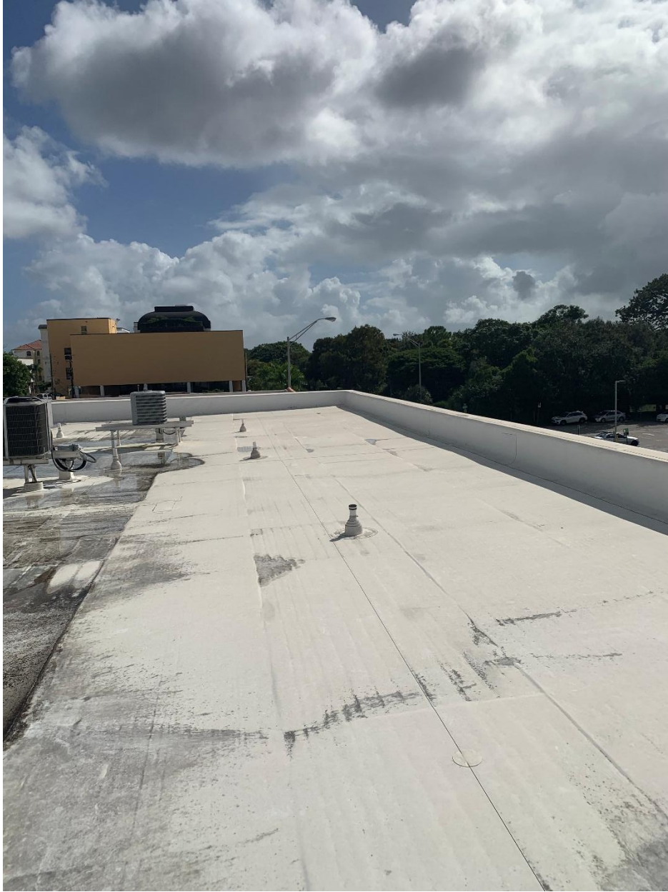
Structural Photo 7a4 – 6915 S. Red Road – Parapet
