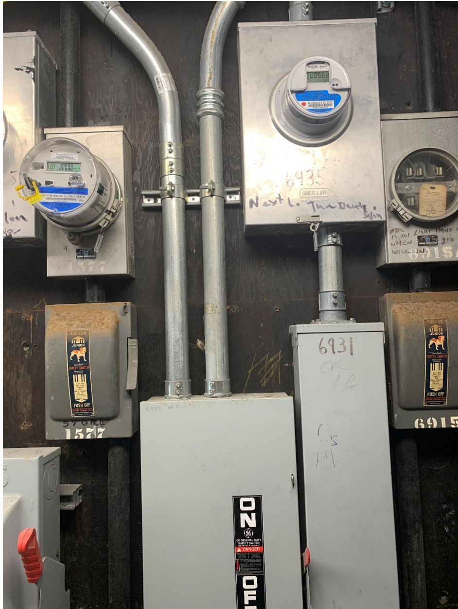
Electrical Photo 4 (4) – 6915 S. Red Road – Metering Equipment
