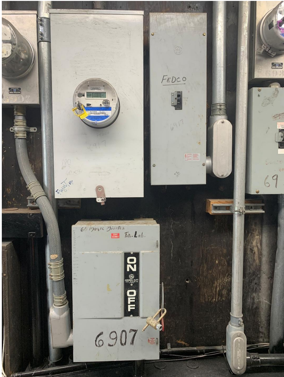
Electrical Photo 4 (2) – 6915 S. Red Road – Metering Equipment
