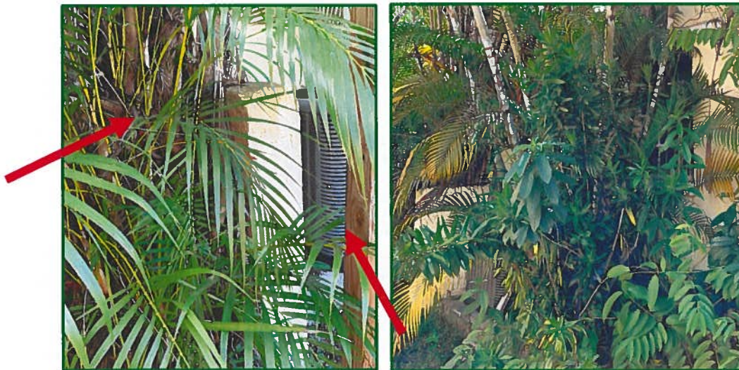
Figures 24: Wing Wall Obscured by Vegetation
