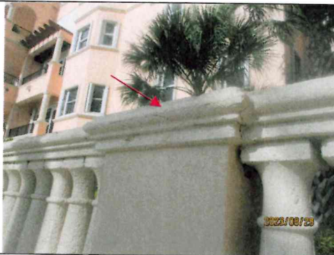
Photo-58: Crack in guardrail cap at the east tower.
