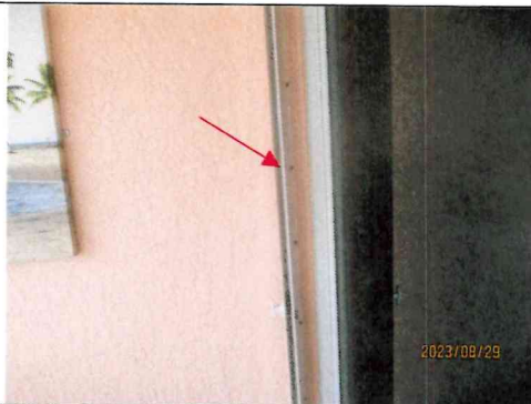
Photo-27: Corroded shutter fasteners anchored to the wall in the balcony of Unit 252.
