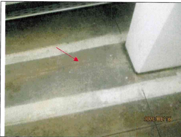
Photo-30: Crack in the floor slab at the ground level parking garage.
