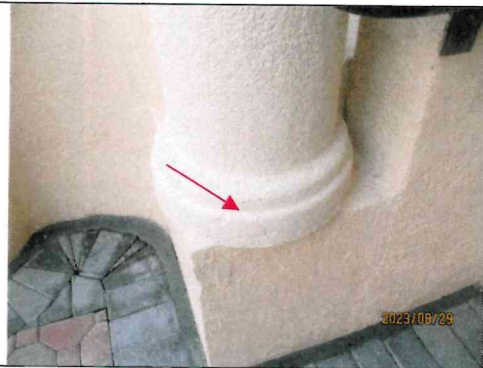
Photo-53: Crack at column base in the east tower.
