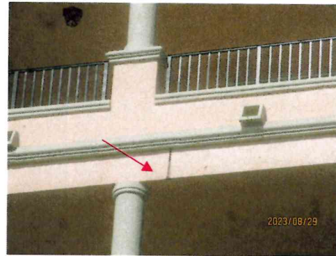
Photo-61: Water/organic stain from curb in the east tower.
