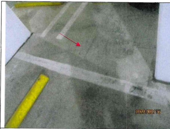
Photo-34: Crack in the floor slab at the ground level parking garage.
