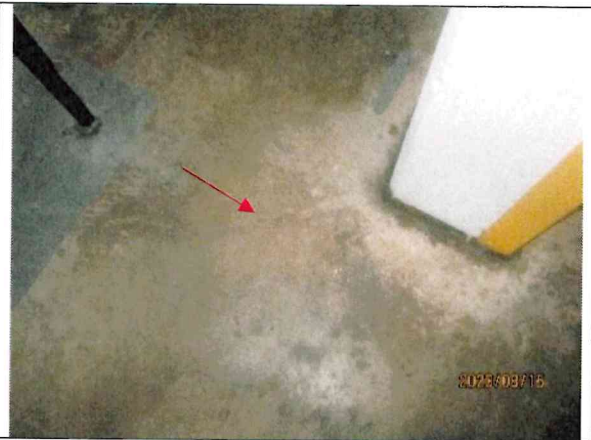
Photo-35: Crack in the floor slab at the ground level parking garage.
