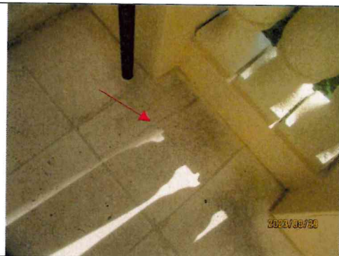
Photo-59: Crack in floor tile at the east tower.
