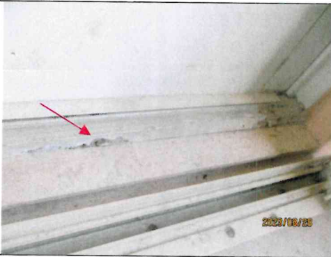
Photo-17: Damaged concrete adjacent to the sliding glass door frame in the balcony of Unit 244.
