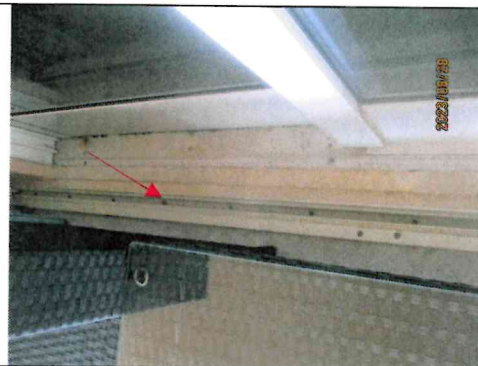
Photo-24: Corroded shutter fasteners anchored to the floor slab in the balcony of Unit 244.
