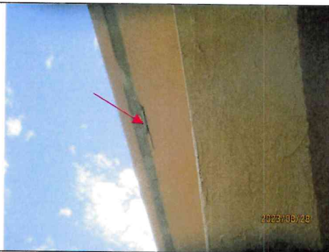
Photo-23: Damaged soffit in the roof of Unit 294.
