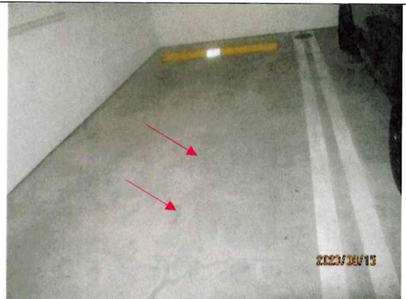
Photo-33: Cracks in the floor slab at the ground level parking garage.
