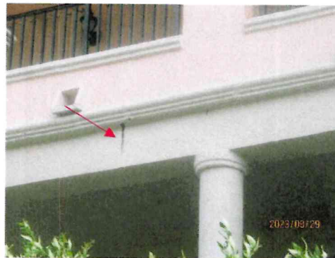
Photo-62: Water/organic stain from curb in the south tower.
