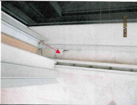
Photo-15: Crack in the tile adjacent to the shutter in the balcony of Unit 258.
