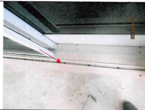
Photo-26: Corroded shutter fasteners anchored to the floor slab in the balcony of Unit 261.
