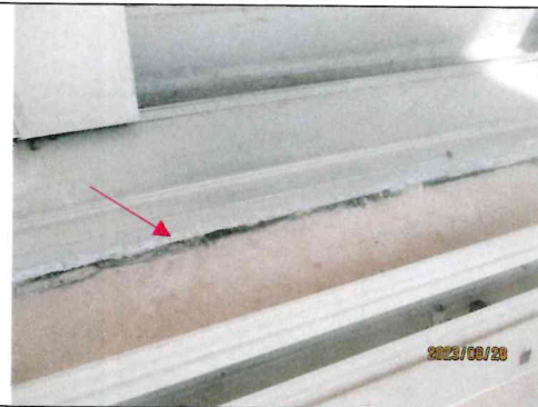
Photo-20: Damaged concrete below the sliding glass door frame in the balcony of Unit 293.
