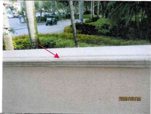
Photo-57: Crack in cap beam at the wall in the north tower.
