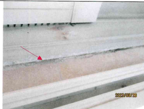
Photo-16: Damaged concrete below the sliding glass door frame in the balcony of Unit 293.
