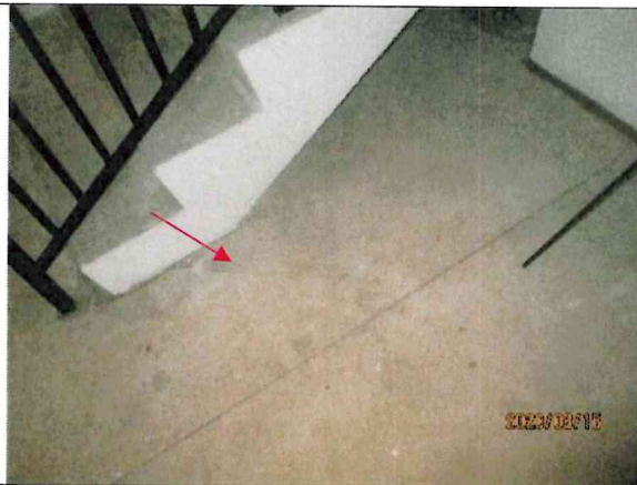
Photo-32: Crack in the floor slab at the ground level parking garage.
