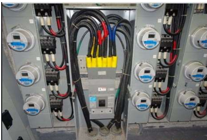
South Tower meter stack
