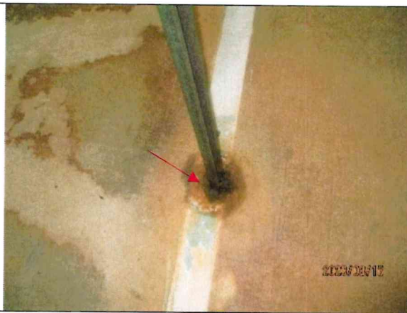
Photo-36: Corrosion stains on the floor slab at the signboard post located at ground level parking garage.
