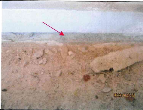
Photo-19: Damaged concrete below the sliding glass door frame in the balcony of Unit 293.
