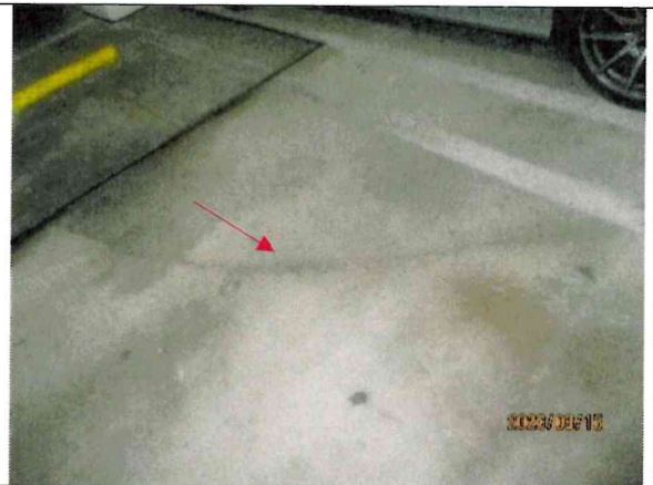
Photo-31: Crack in the floor slab at the ground level parking garage.
