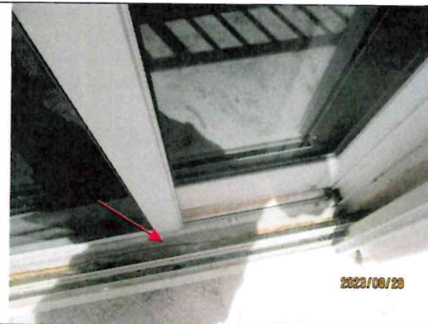
Photo-22: Water ponding adjacent to the shutter in the balcony of Unit 235.
