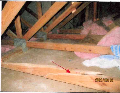
Photo-7: Cracked web support member inside south tower attic.
