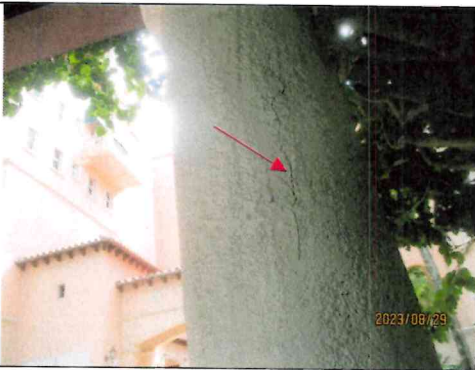
Photo-52: Crack in column in the west tower.
