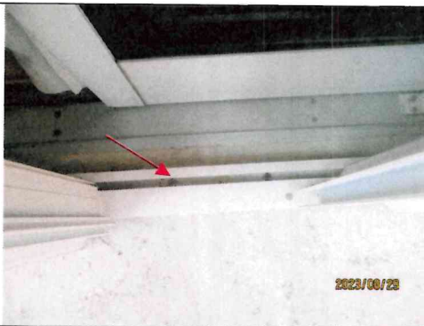
Photo-25: Corroded shutter fasteners anchored to the floor slab in the balcony of Unit 257.
