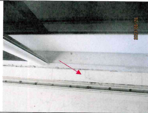
Photo-14: Crack in the tile adjacent to the shutter in the balcony of Unit 243.
