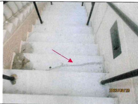
Photo-55: Crack in stairs in the north tower.
