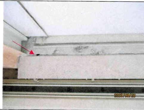
Photo-18: Void in the concrete adjacent to the sliding glass door frame in the balcony of Unit 243.
