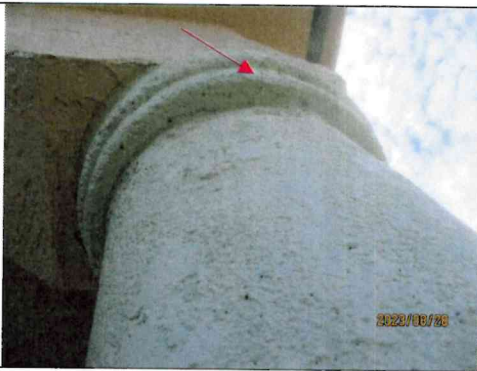
Photo-13: Crack in the column at balcony of Unit 294.
