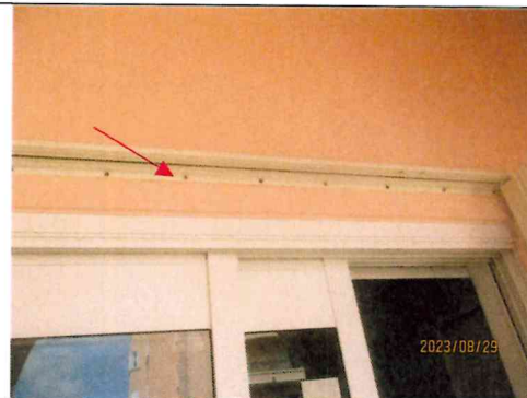
Photo-28: Corroded shutter fasteners anchored to the wall in the balcony of Unit 258.
