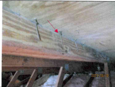
Photo-10: Nails are not inserted in the top chord of truss inside north tower attic.
