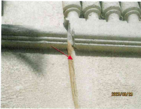
Photo-60: Crack in expansion joint at the east tower.
