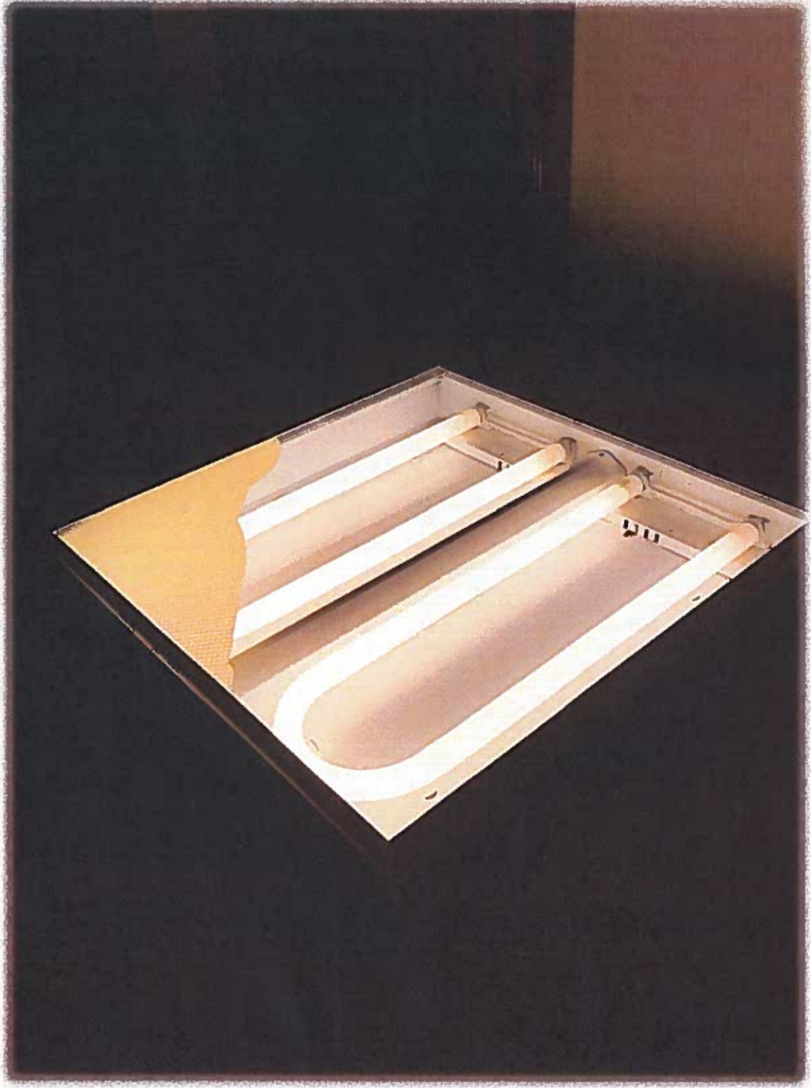
Broken interior light cover
