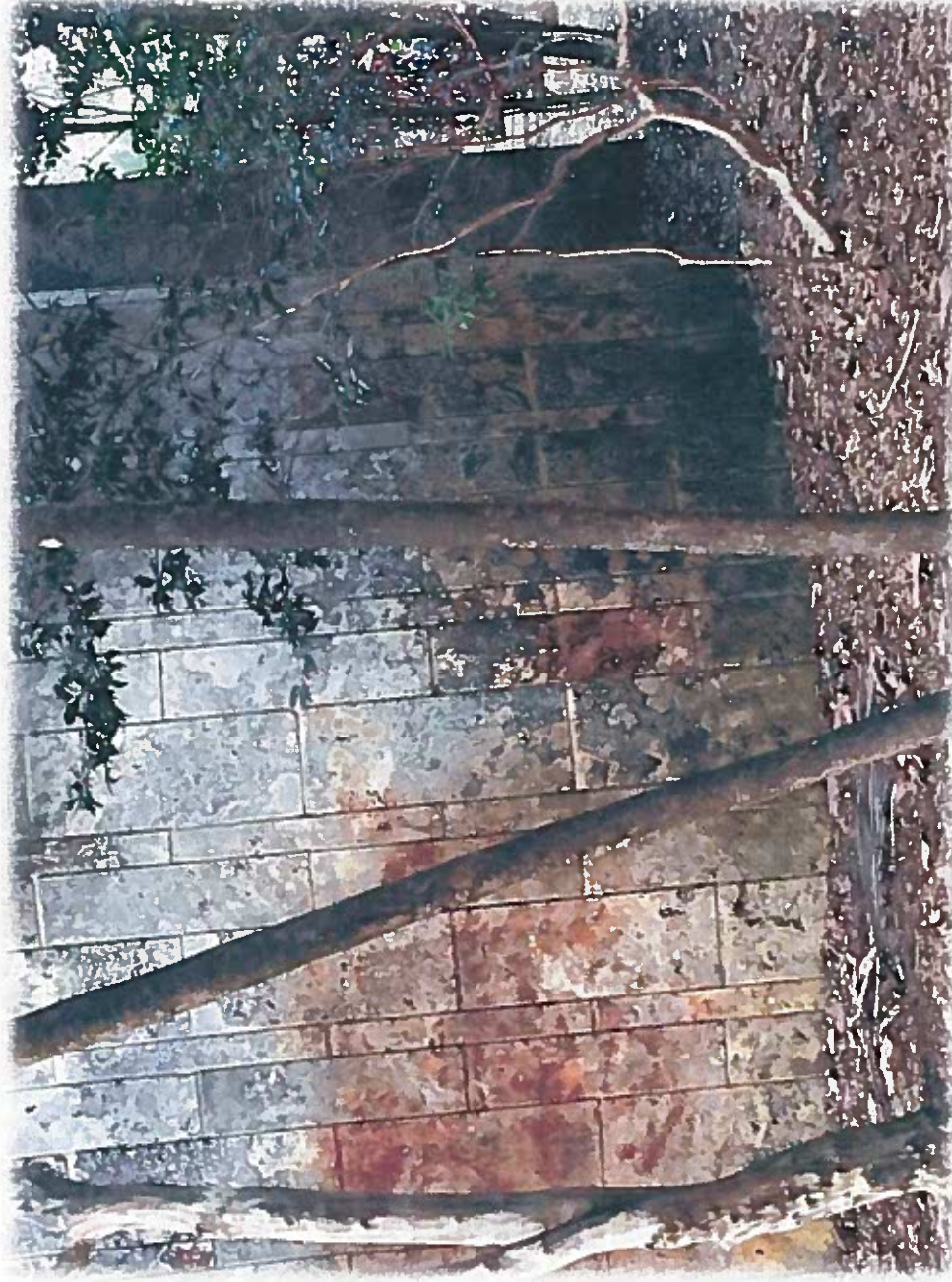
Stained building exterior
