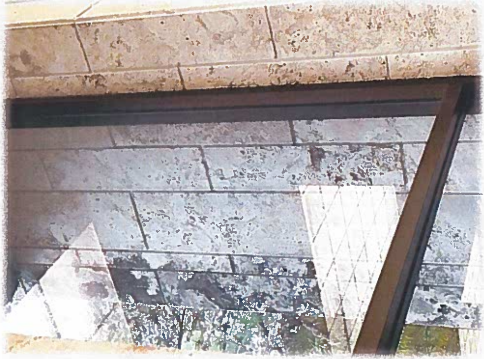
Mold on building exterior
