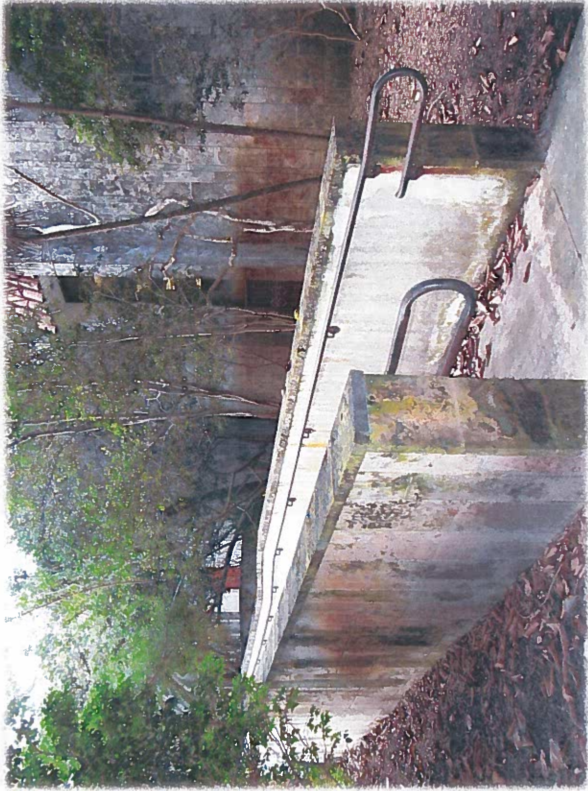
Mold at the handicap entrance
