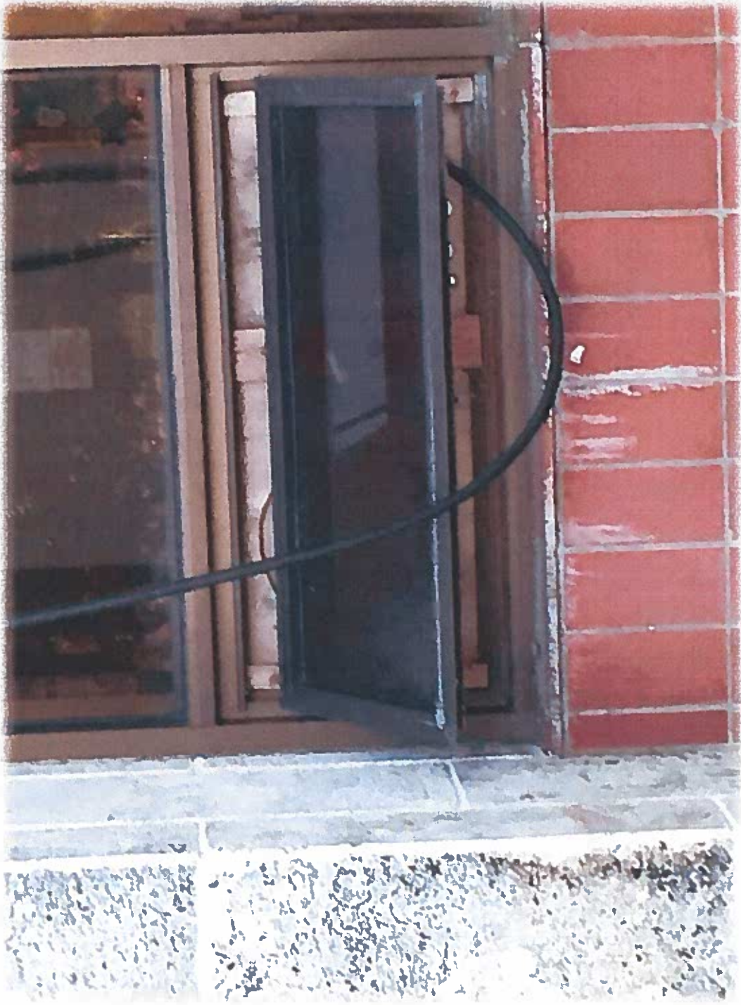
Building exterior electrical cable to portable air-conditioner
