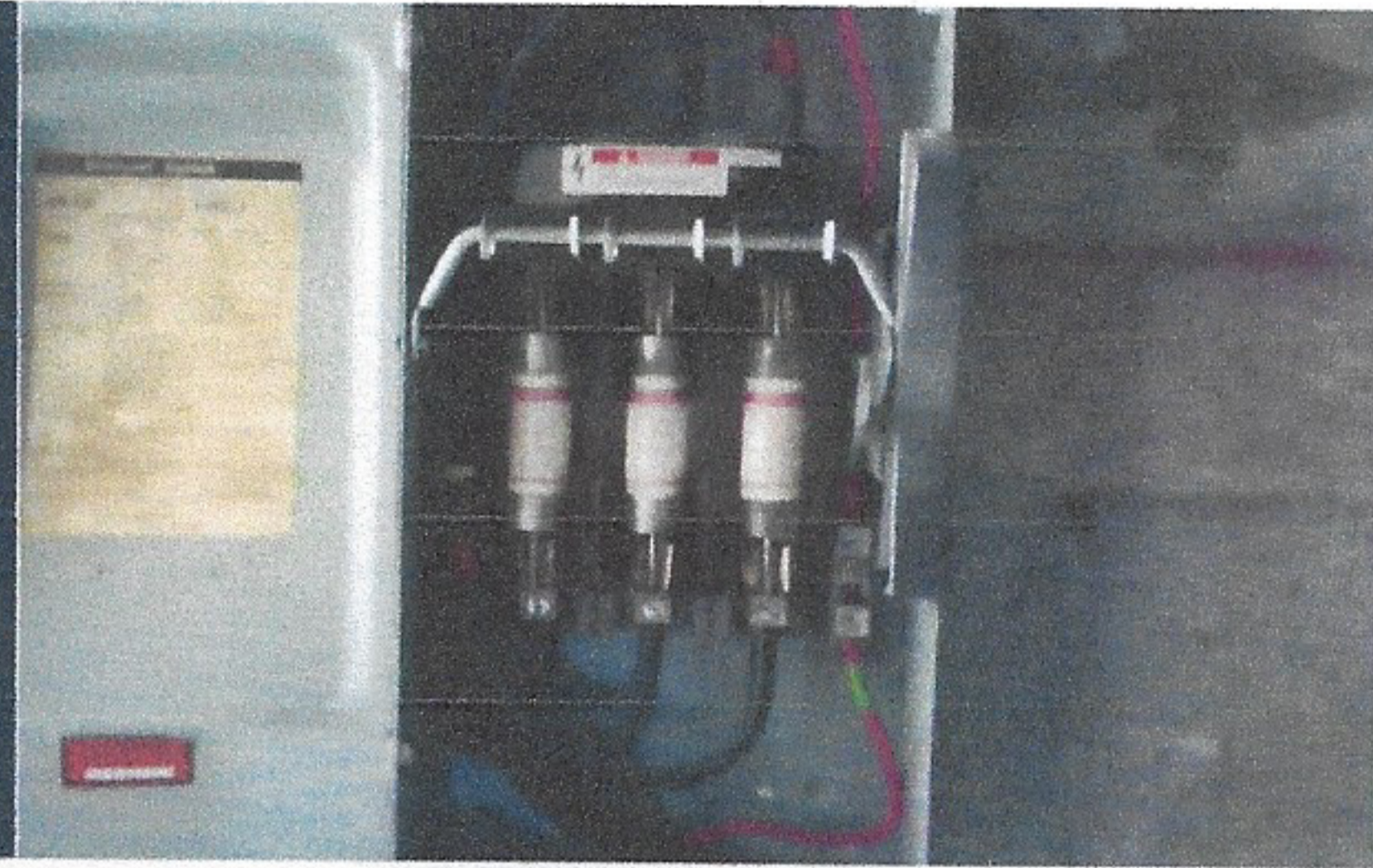
4800 Elevator Sub.jpegAligned Visual Image
