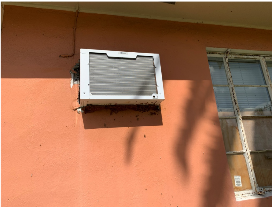
Picture #6 A/C unit not properly encased into the wall.
