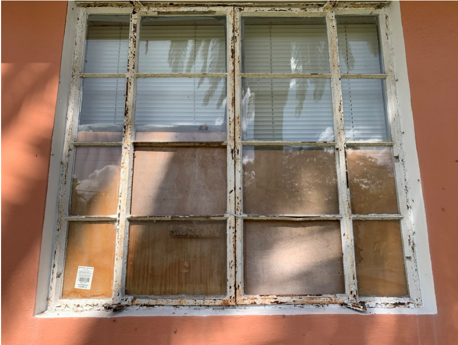
Picture #5 Exterior window rusted and glass panel broken.
