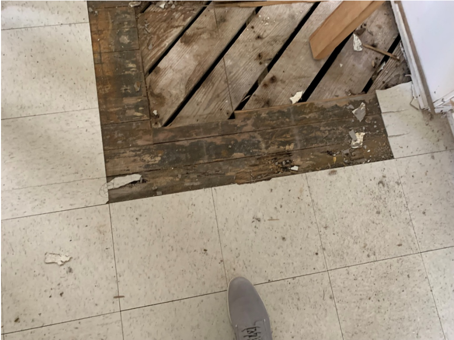
Picture #9 Wood floor damaged by termites.
