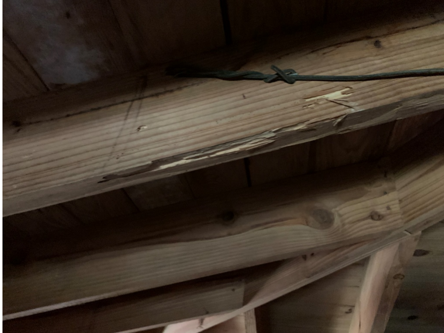
Picture 3 Roof joists damaged by termites.
