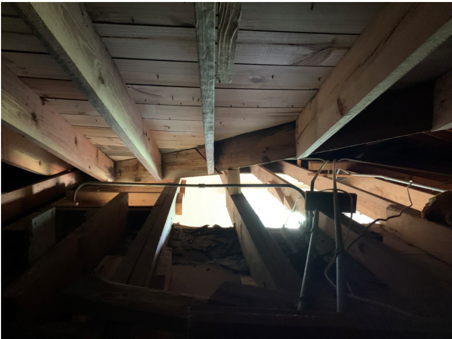
Picture #10 Ridge joist broken.
