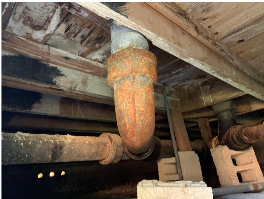
Picture 4 Previously damaged wood floor by water intrusion, not properly repaired. Wood joists supported by unstable blocks and wood posts
