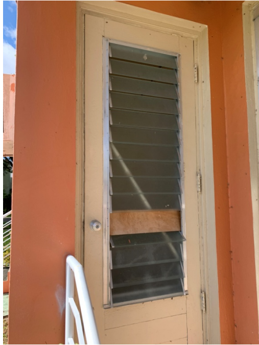
Picture #7 Exterior door very damaged
