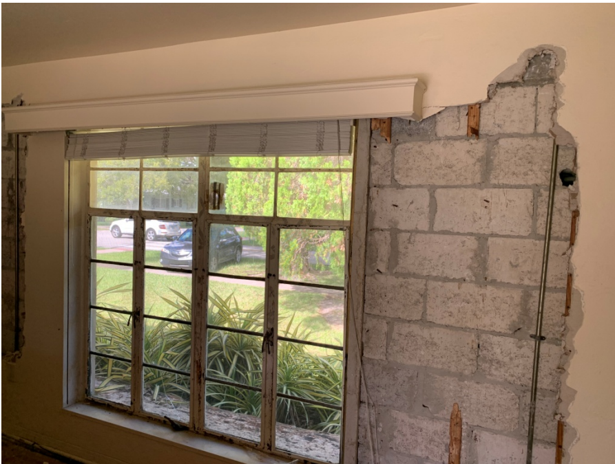
Picture #8 Front widow, very damaged
