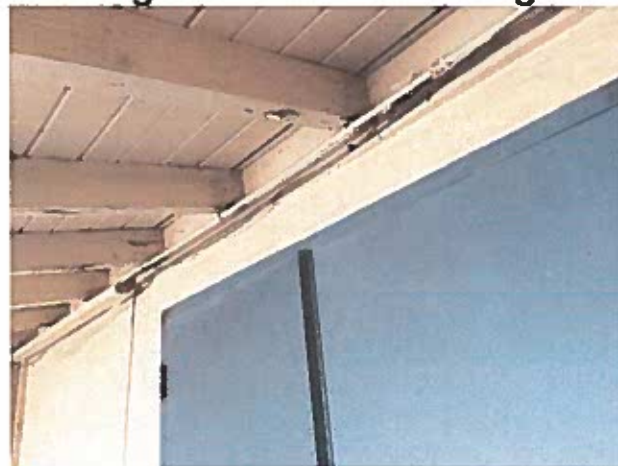
Photograph #5 of previous termite damage at Parking Courtyard Shelter roof joist and deck.
