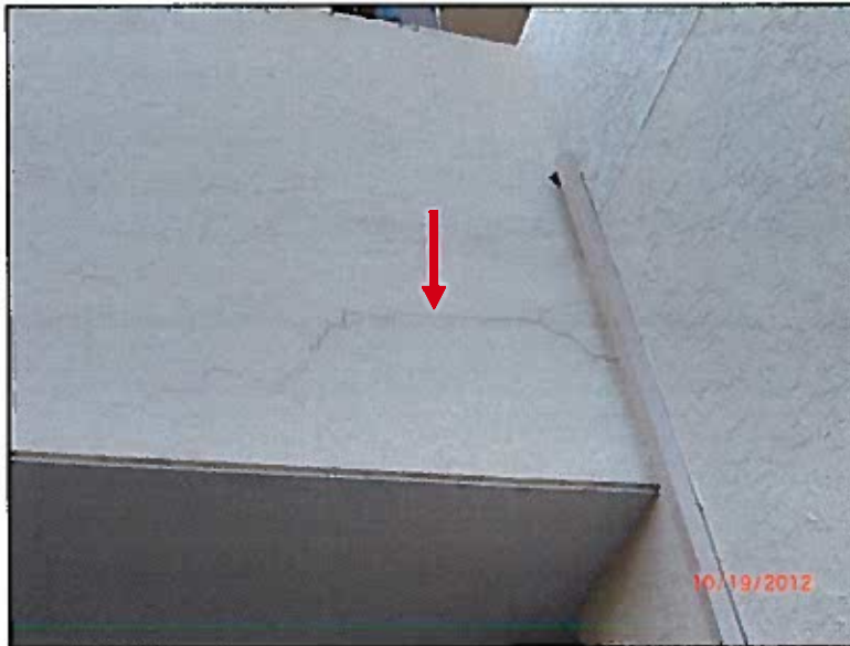
PHOTO # 28: cracking on overhang at West side
