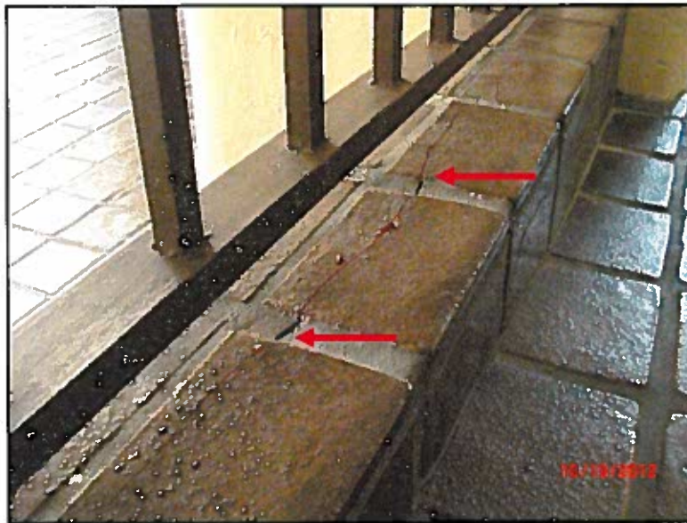
PHOTO # 32: crack along tiled ramp east of main entrance
