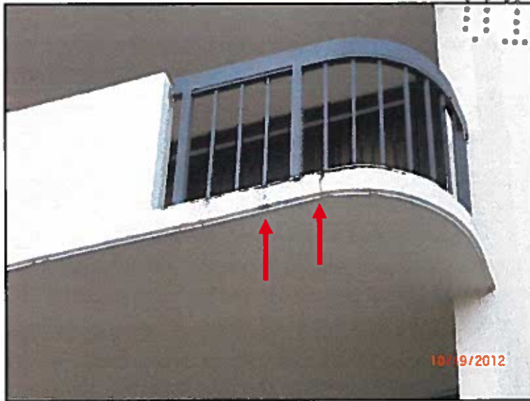
PHOTO # 29: cracking and staining on balcony edge
