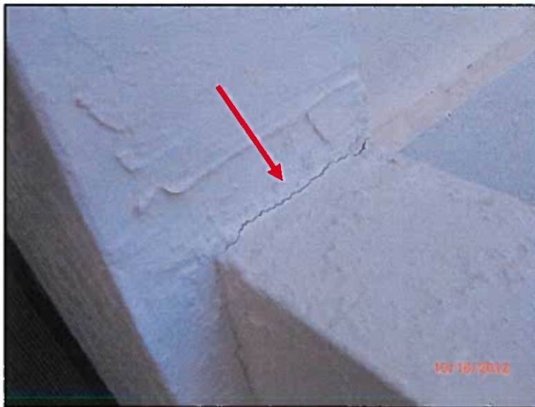
PHOTO # 8: Cracking at connection between balcony wall and bldg. column at Unit #219
