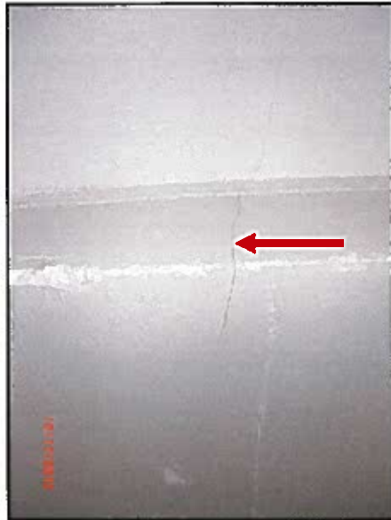
PHOTO # 19: slab cracking at column drop panel between Parking Spaces 248 & 249
