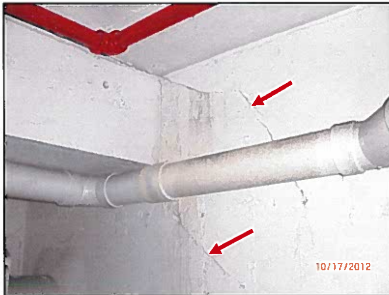
PHOTO # 26: cracking on wall next to Parking Space 51
