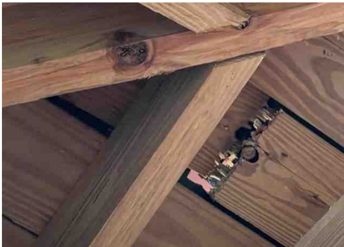
Wood Rot in Trusses
