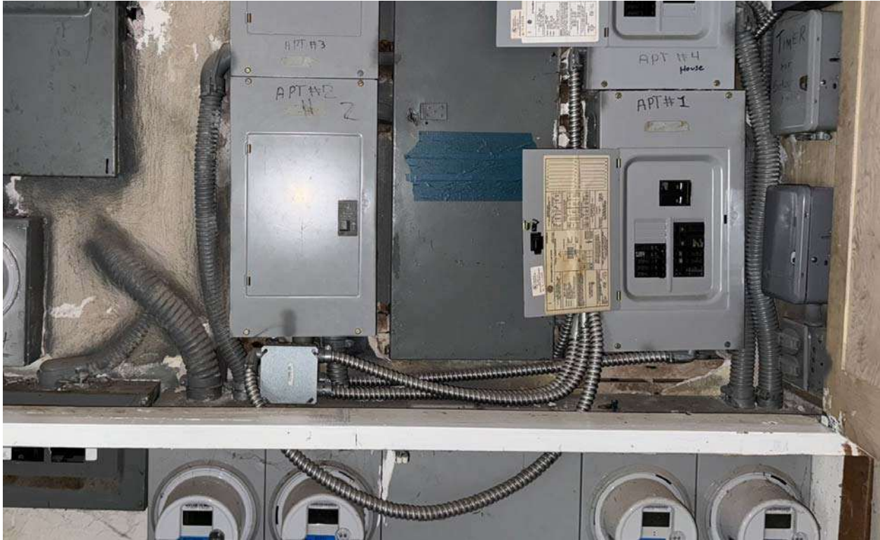
Figure 8 - General Conduit (Photo 12)
