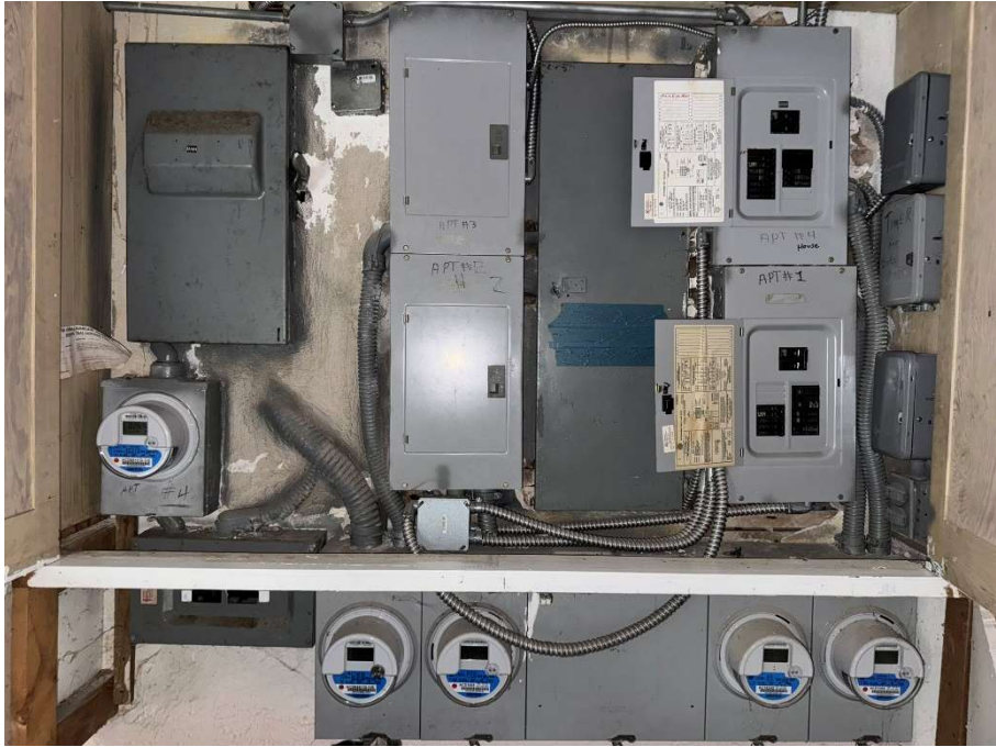
Figure 2 - Electrical Service (Photo 3)
