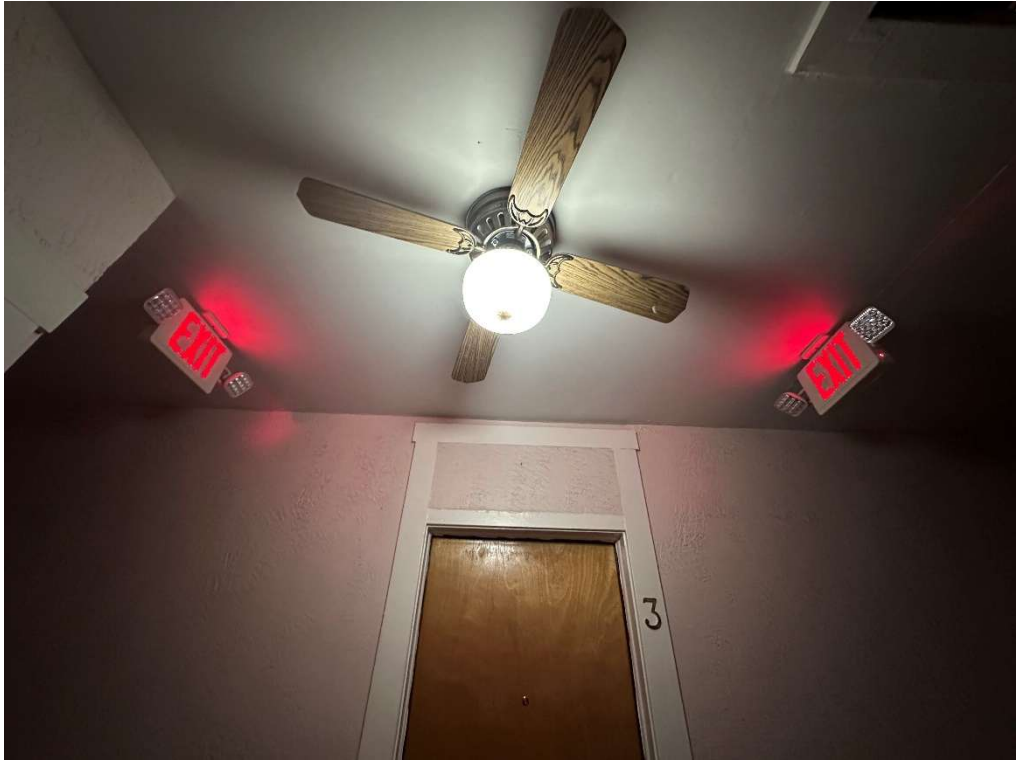
Figure 9 - Existing Emergency lighting (Photo 18)
