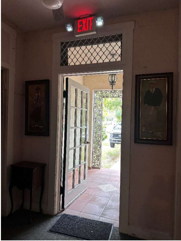
Figure 12 - Existing illuminated exit signs (Photo 22)
