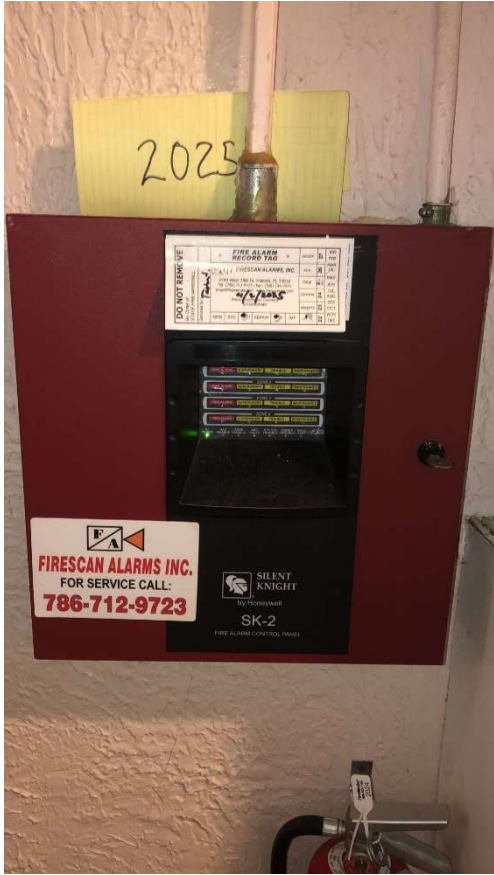
Figure 10 - Existing fire alarm system ( Photo 20)
