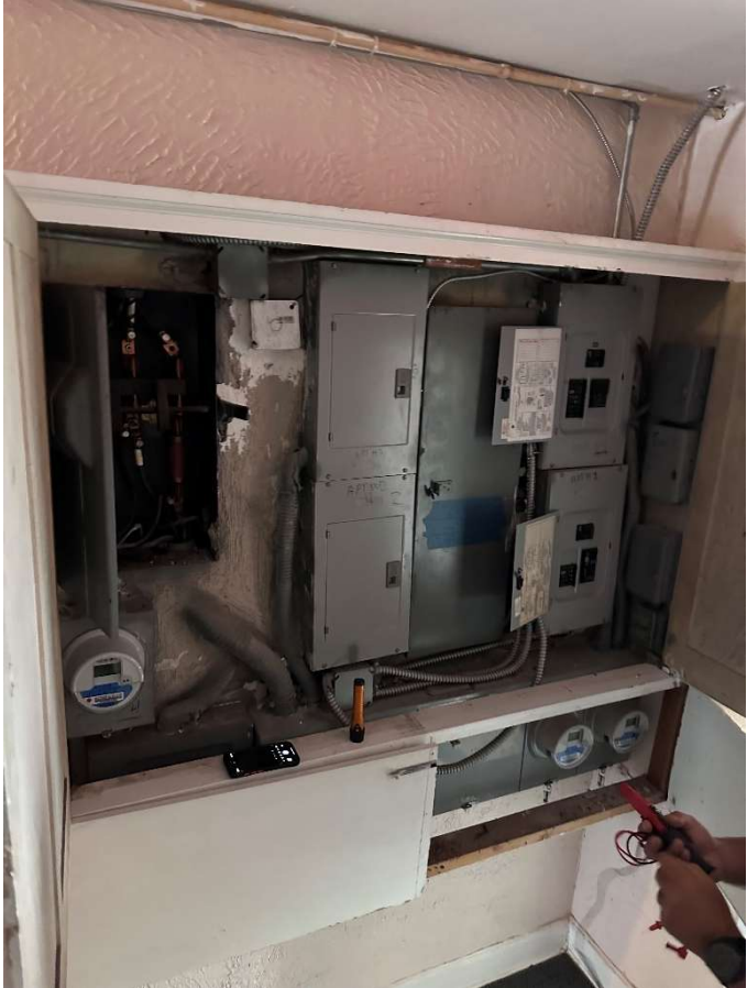
Figure 3 - Clearance around equipment (Photo 4)
