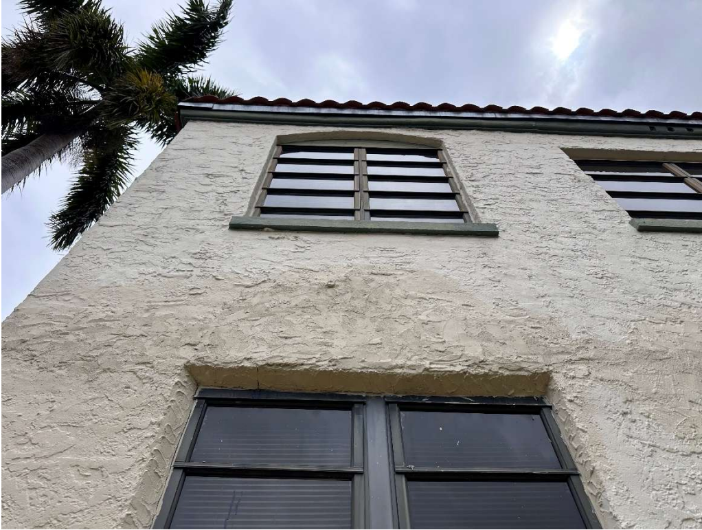
Figure 6 - Previous patching or repairs (Section 5.f.)
