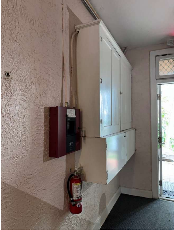
Figure 4 - Clearance around electrical cabinet (Photo 5)
