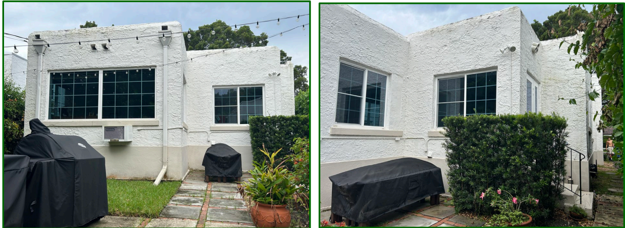
Figures 22: Rear (North) Façade, 2025 Protruding Bay: Originally Sleeping Porch Receding Bay: Originally Back Porch with Stairs
